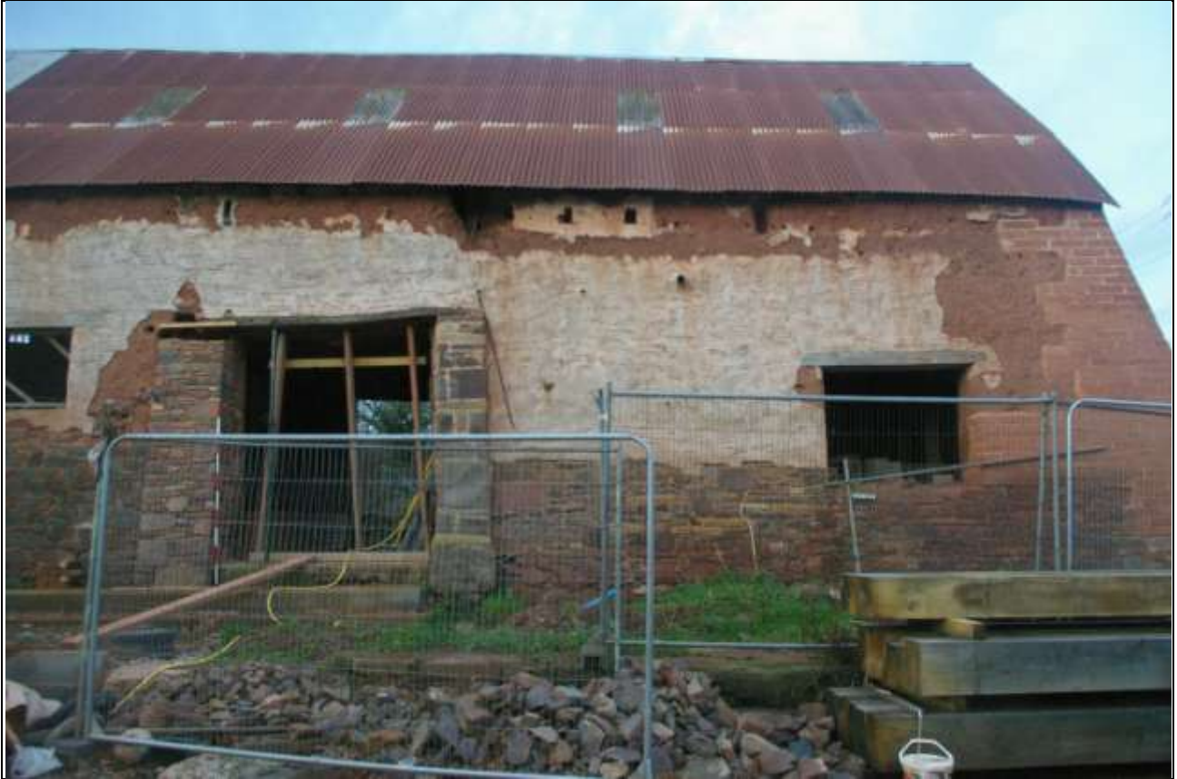
The south-east elevation, at the north end; from the south-east (2m scale).
