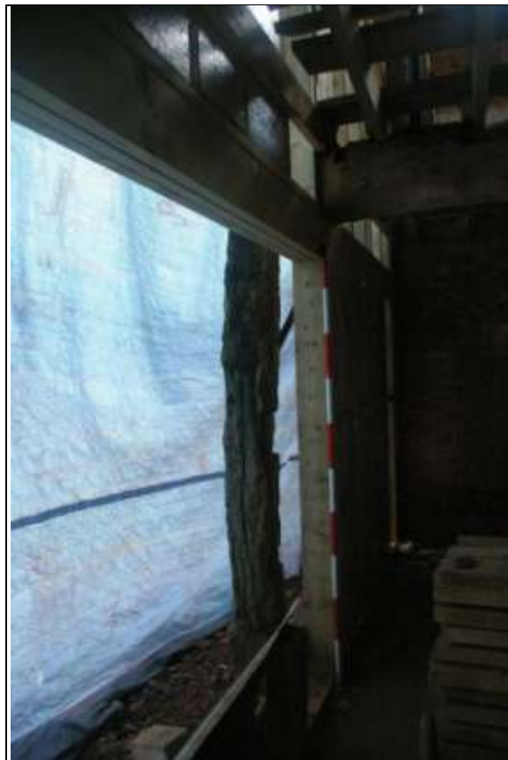
The surviving oak post to the farmyard front of the linhay, at the south end, integral to the elm beam and roof structure; from the west (2m scale).
