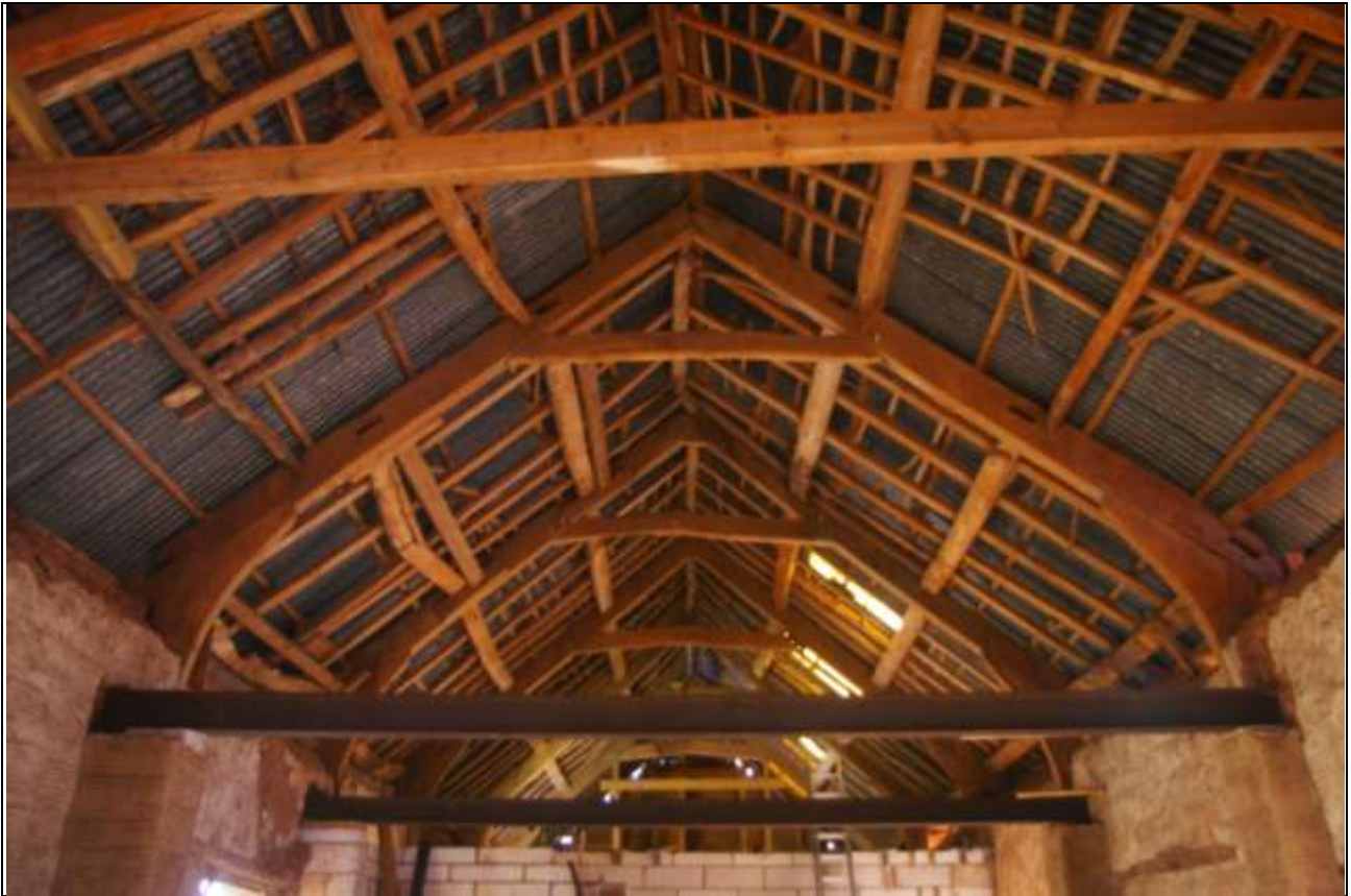
The roof of the earlier phase of the barn; from the south-west.
