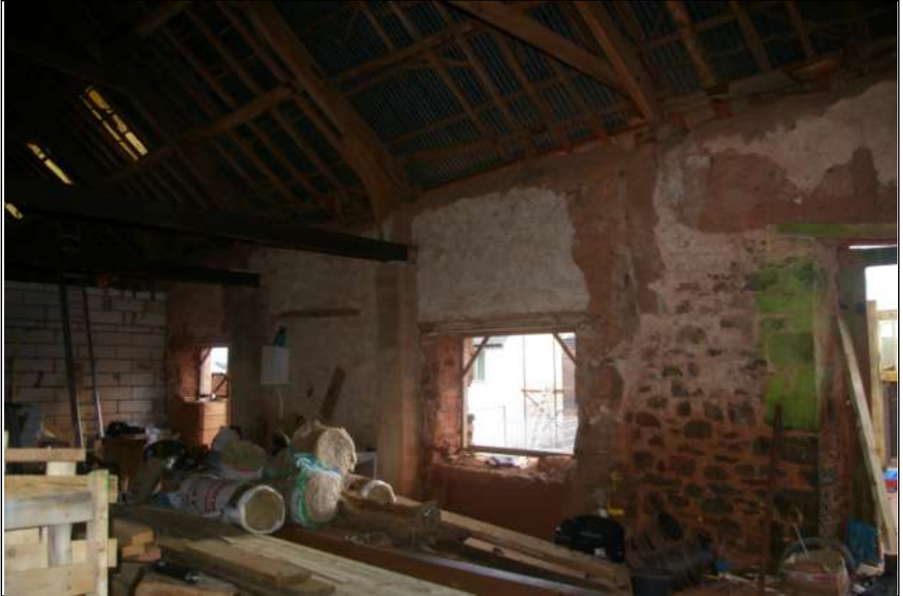
The main open area of the barn towards the north, already partially divided for conversion; from the west.
