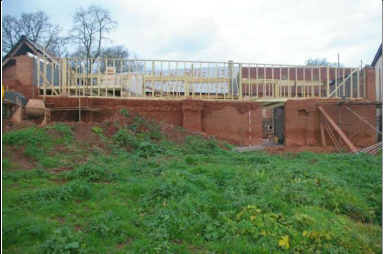
The east corner of the south linhay, rebuilt in handmade cob blocks, using collapsed cob from the site, also showing the restored historic cob south-east wall; from the south-east (2m scale).
