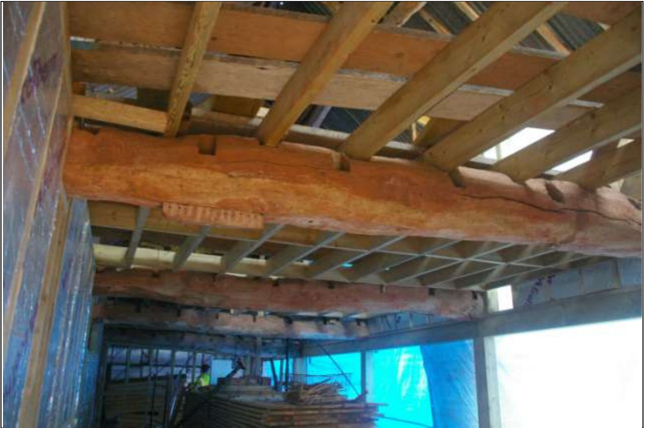
The conserved and reset elm loft beams in the west linhay, incorporated into the new secure first floor; from the south.
