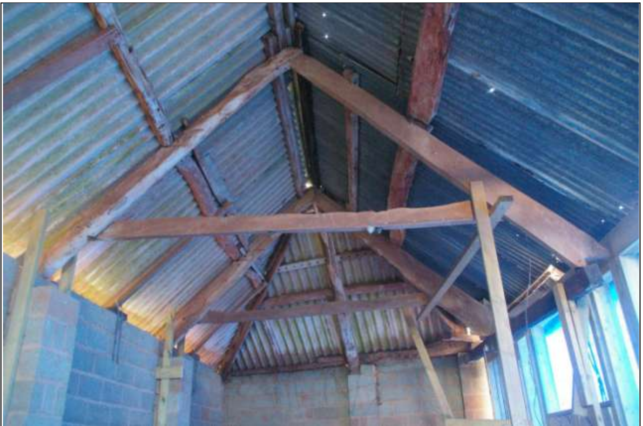
The western end of the west linhay roof, showing the hipped structure and first truss. The roof has been overhauled in the 19 th century; from the south-east.
