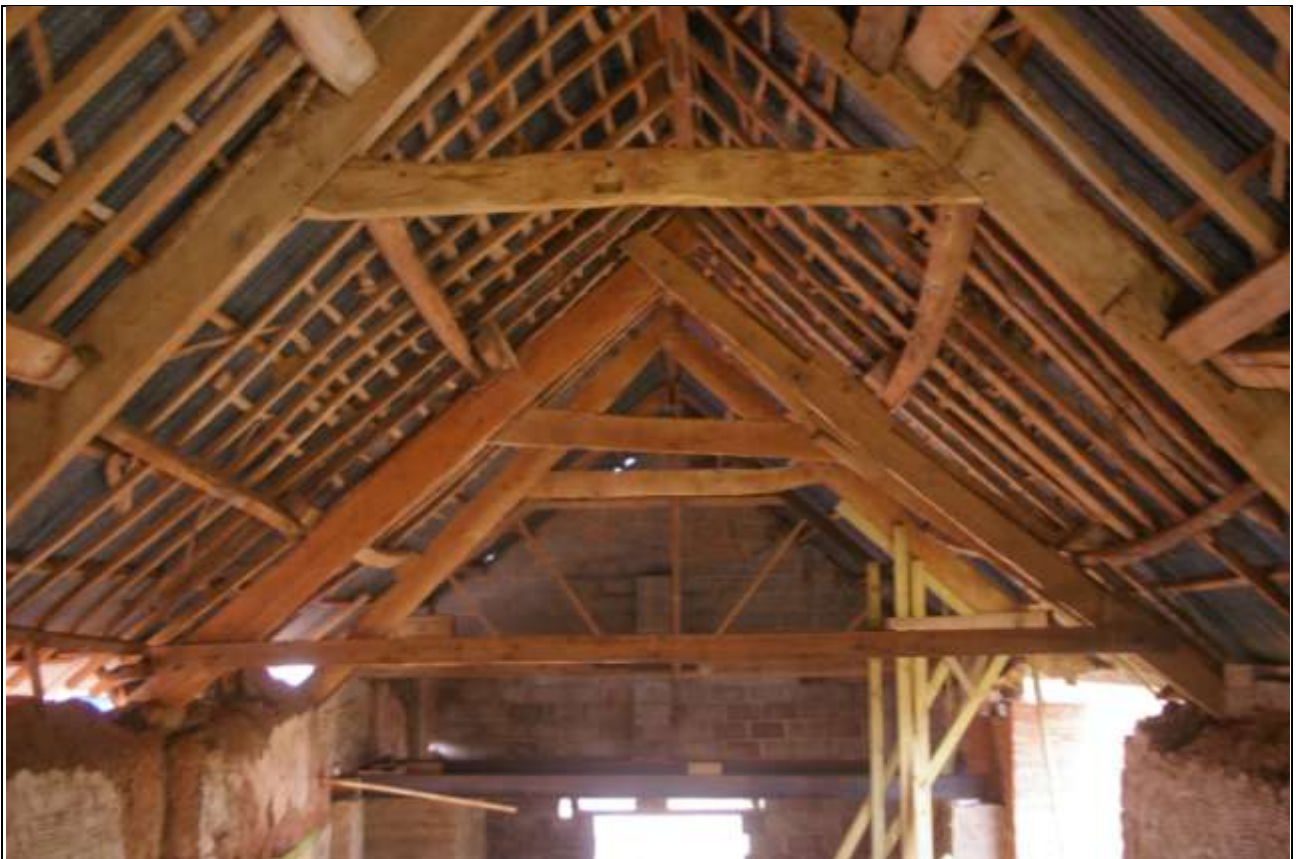
The later roof of the short extended south section of the barn; from the north, north-east.
