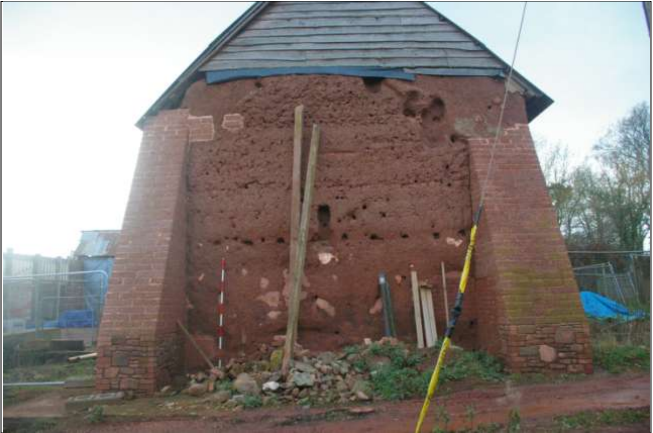
The north-east end of the barn, with poor condition original cob and newly rebuilt cob buttresses; from the north-north-east (2m scale).
