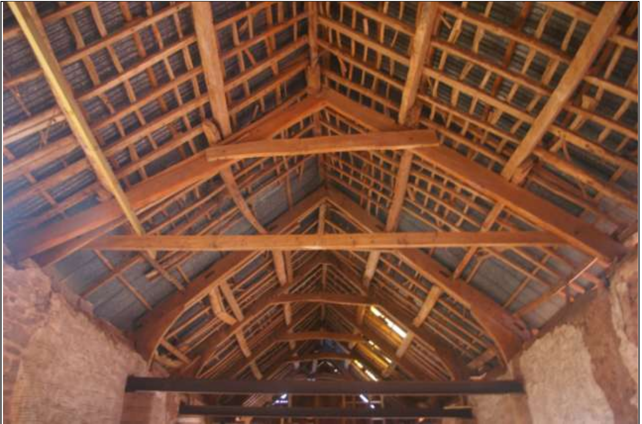
One of the later trusses to the south end of the barn, probably later 17 th or early 18 th century in date, showing how they have been patched and repaired at a later date.
