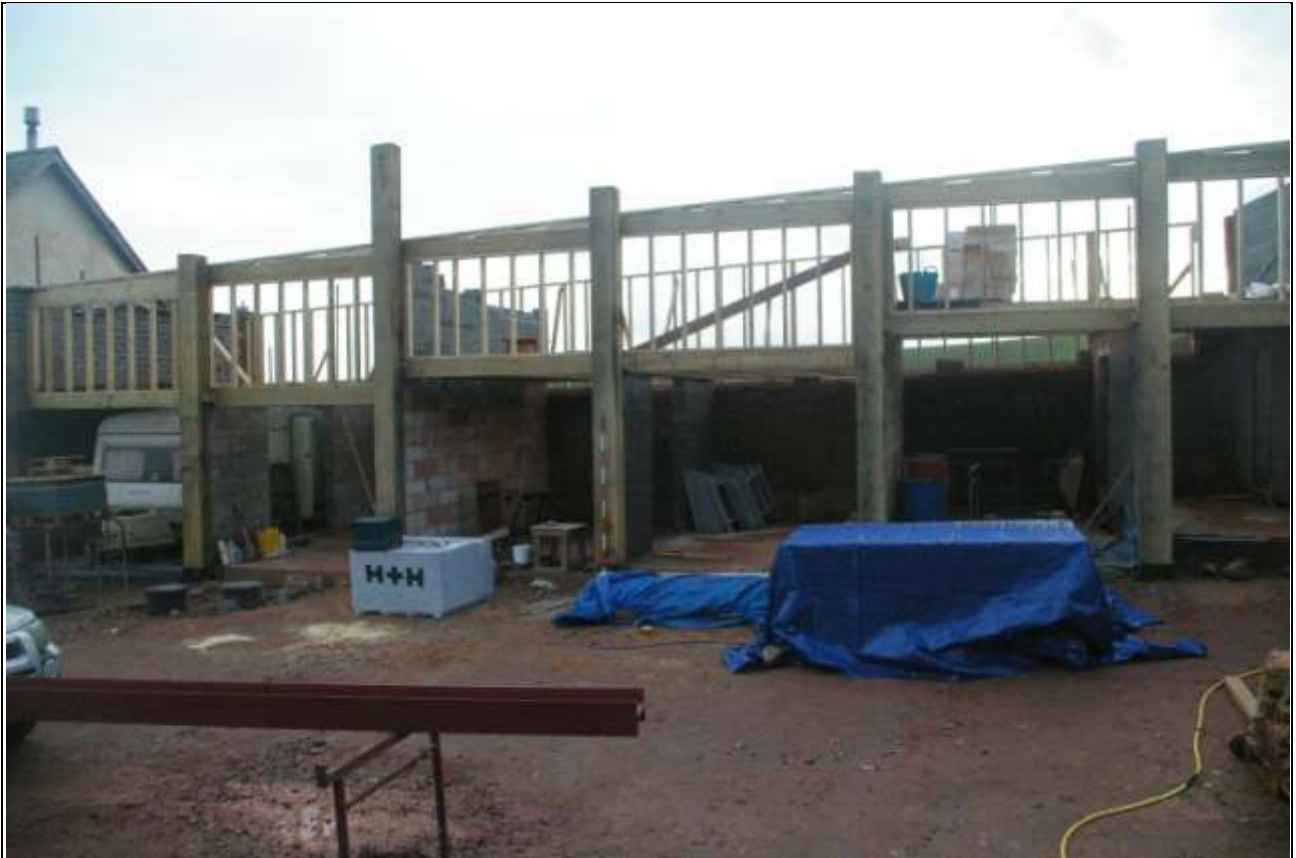
The long north-western elevation of the southern linhay; from the west (2m scale).
