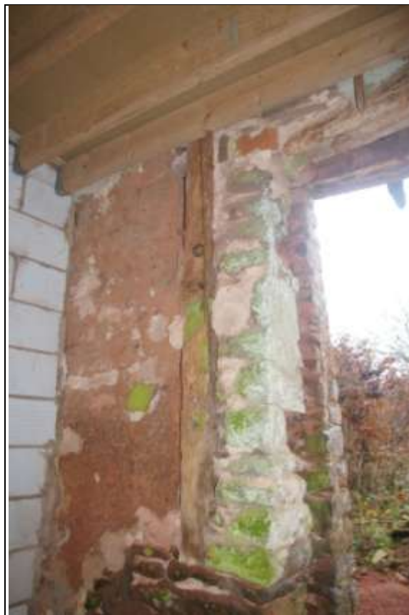
Detail of a jointed cruck truss base, showing an iron ring set in the timber; from the east, north-east.
