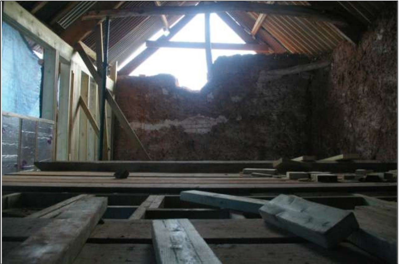
The surviving cob south-west and south-east elevations of the west linhay; from the west, north-west.
