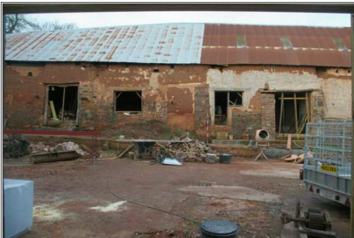
Figure 5: The central section of the south-east elevation of the main barn; from the south-east (2m scale).
