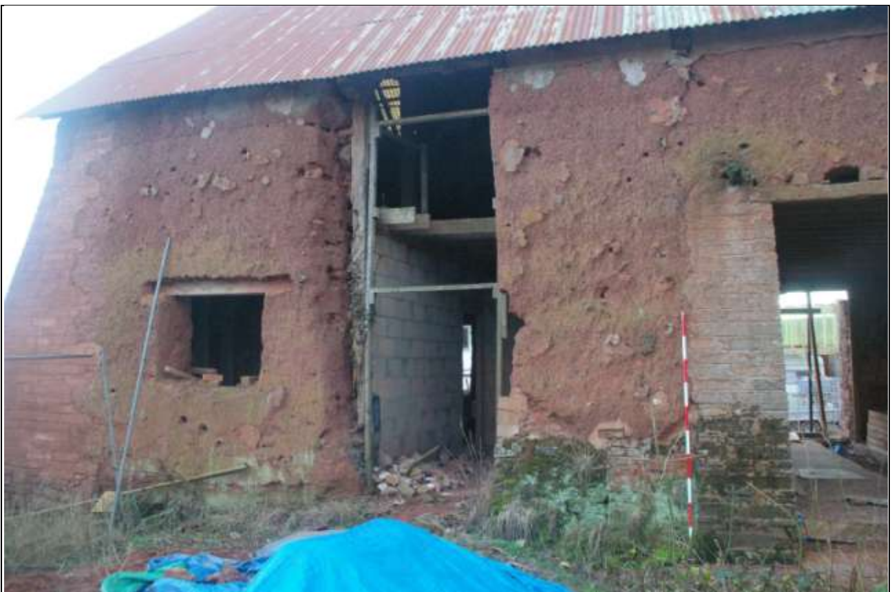
The north-west elevation of the barn, showing the forced openings undertaken by the previous owner; from the west (2m scale).
