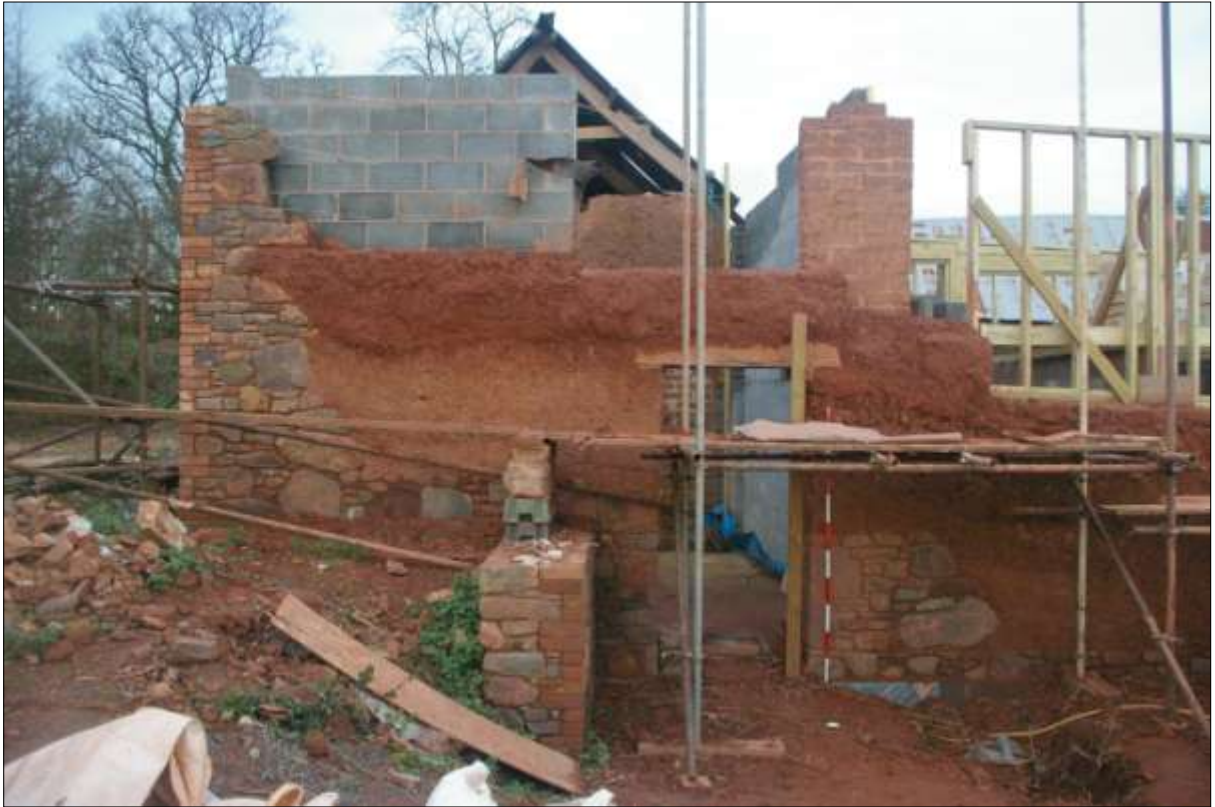
Figure 7: The original structure here had largely collapsed but the remains were suggestive of a possible 19 th century extension for a root house, to serve the linhays and byres; from the south-west (2m scale).
