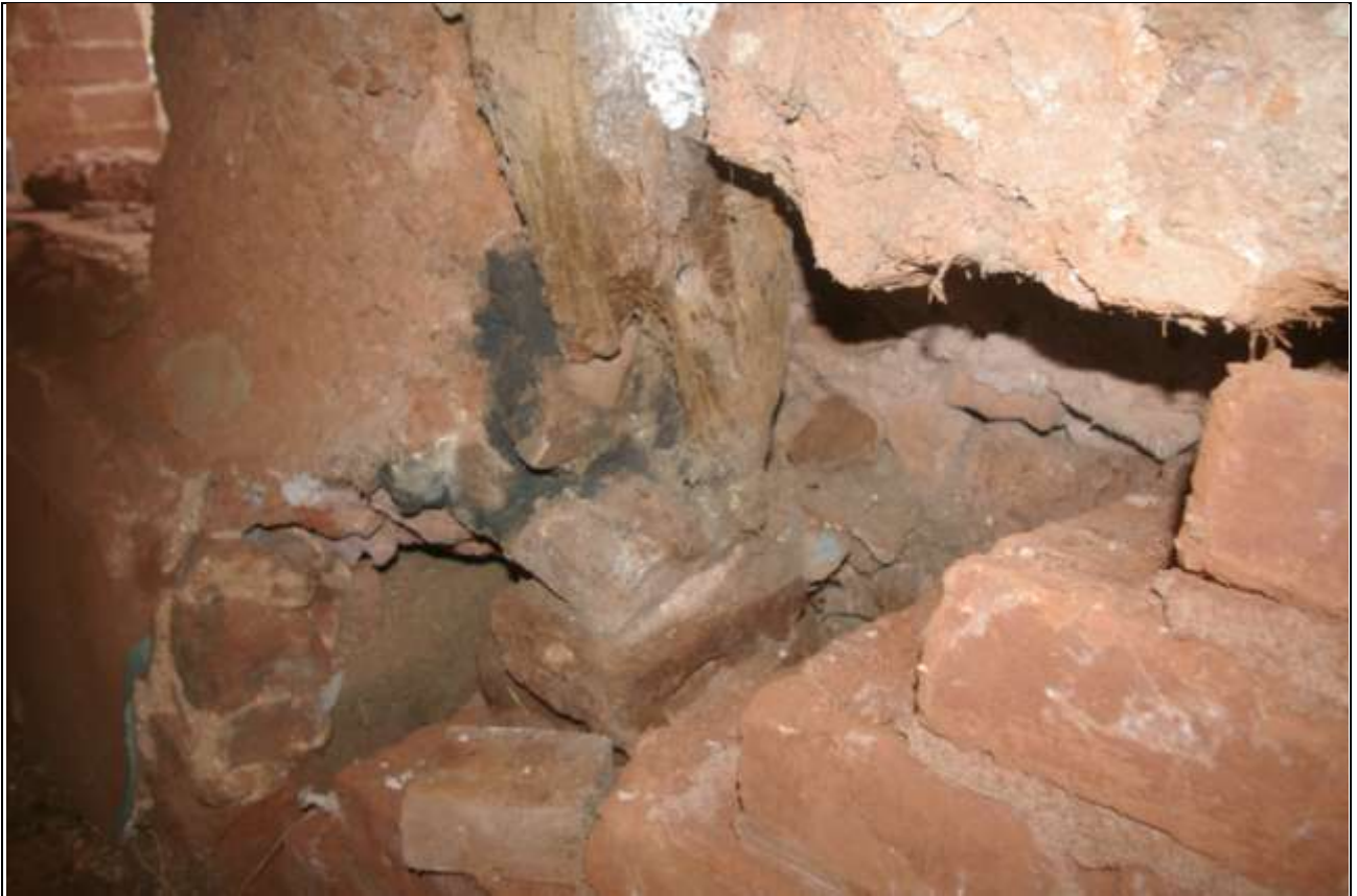
The shaped stone block which provides a pad for the jointed cruck truss to sit upon; the cob inner and stone outer skim of the wall and the heavy breccia blocks which form the plinth upon which the barn is built; from the west, south-west.
