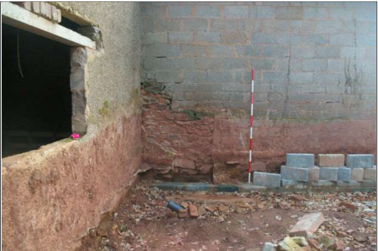
The barn and western linhay where they adjoin, showing the barn has been slightly truncated during rebuilding; from the west (2m scale).
