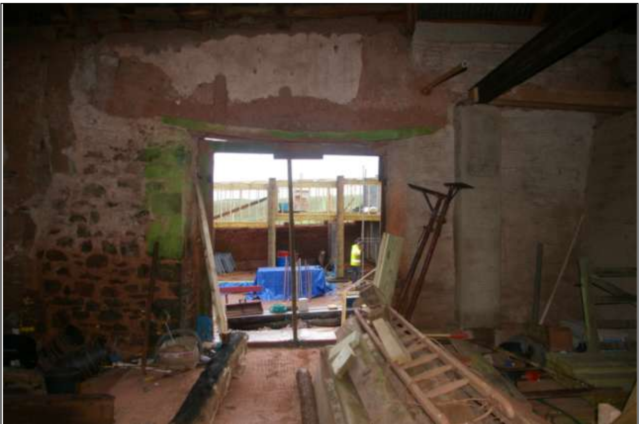
The large barn opening in the south end of the south-east elevation, with rebuilt stone sides, typical 19 th century timber lintel and door frame, with chamfered sides; from the west, north-west.
