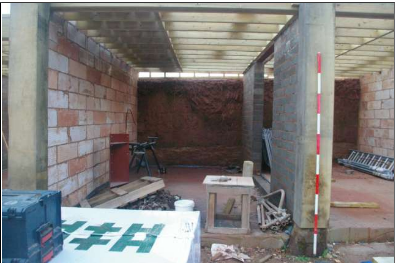
View of the converted south linhay, showing the cob wall to the south-east and the concrete block stores created within the space; from the north-west (2m scale).
