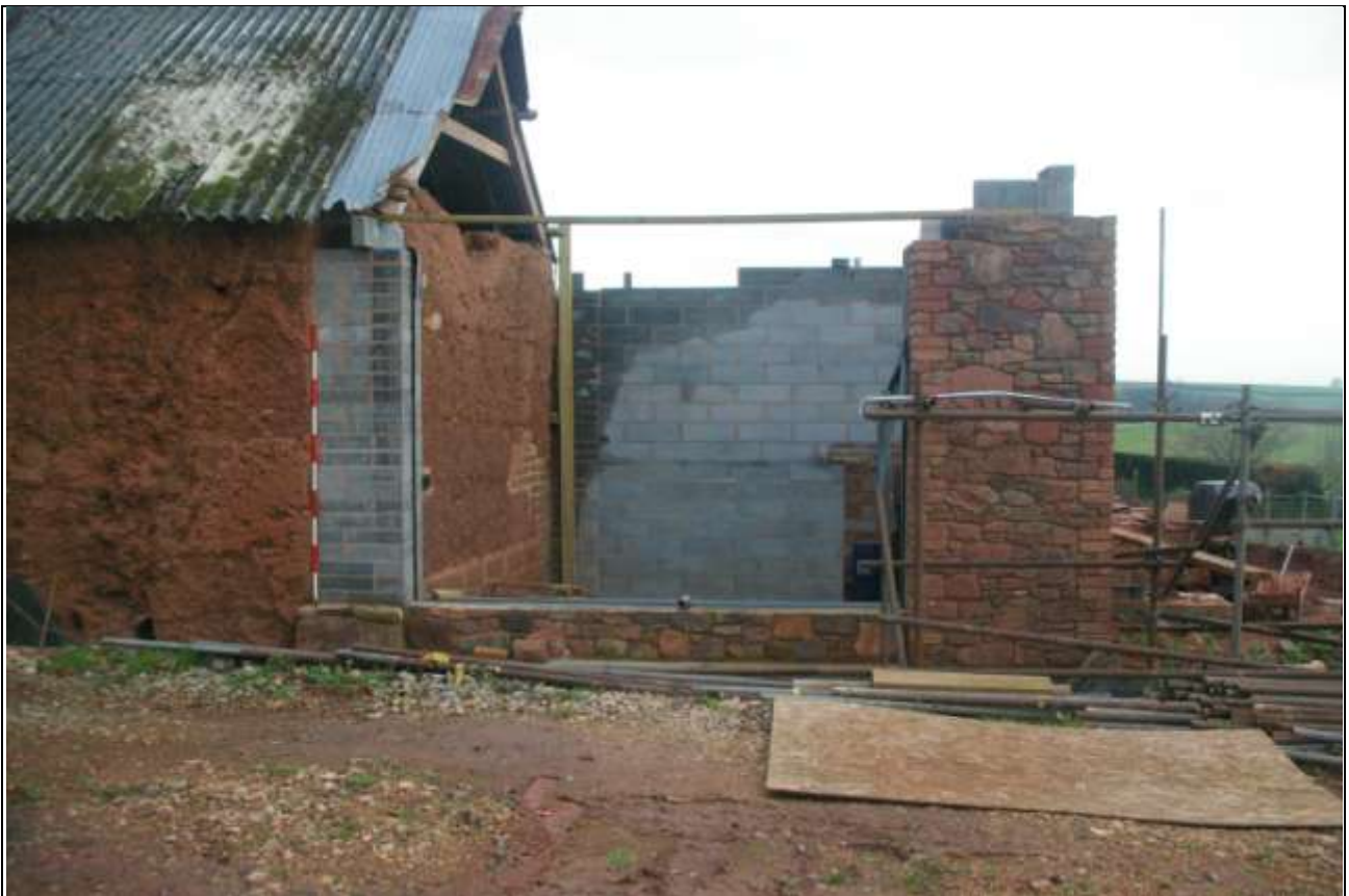
The rebuild of the root house, where the linhays adjoin; from the south-west (2m scale).
