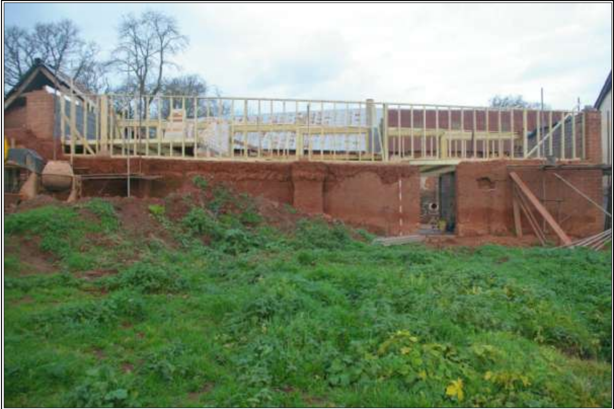
Figure 8: The southern linhay, showing the rebuild with the collapsed cob; from the south-east (2m scale).
