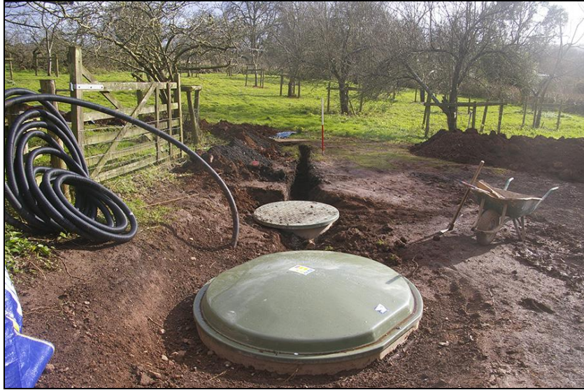
Figure 2: Tanks and west end of the pipe trench; viewed from the north (1m scale).
