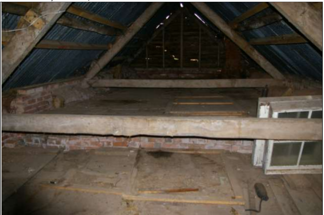
The raised section of loft to the east end, also showing two pairs of the base crucks to the east end; from the west.
