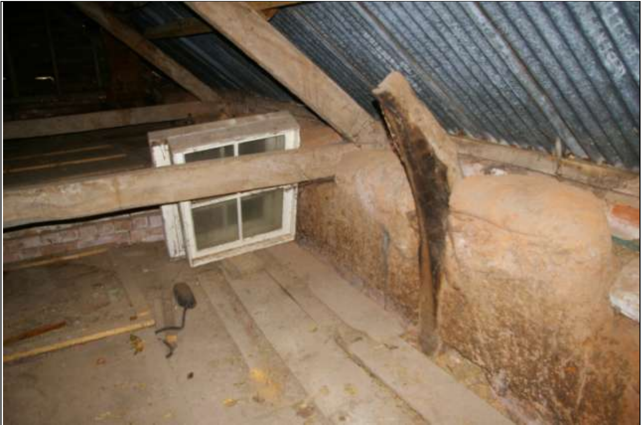
The best preserved base cruck as it rises smoothly into the joint, showing the smoke-blackening from the fire which destroyed this roof; from the north-west.
