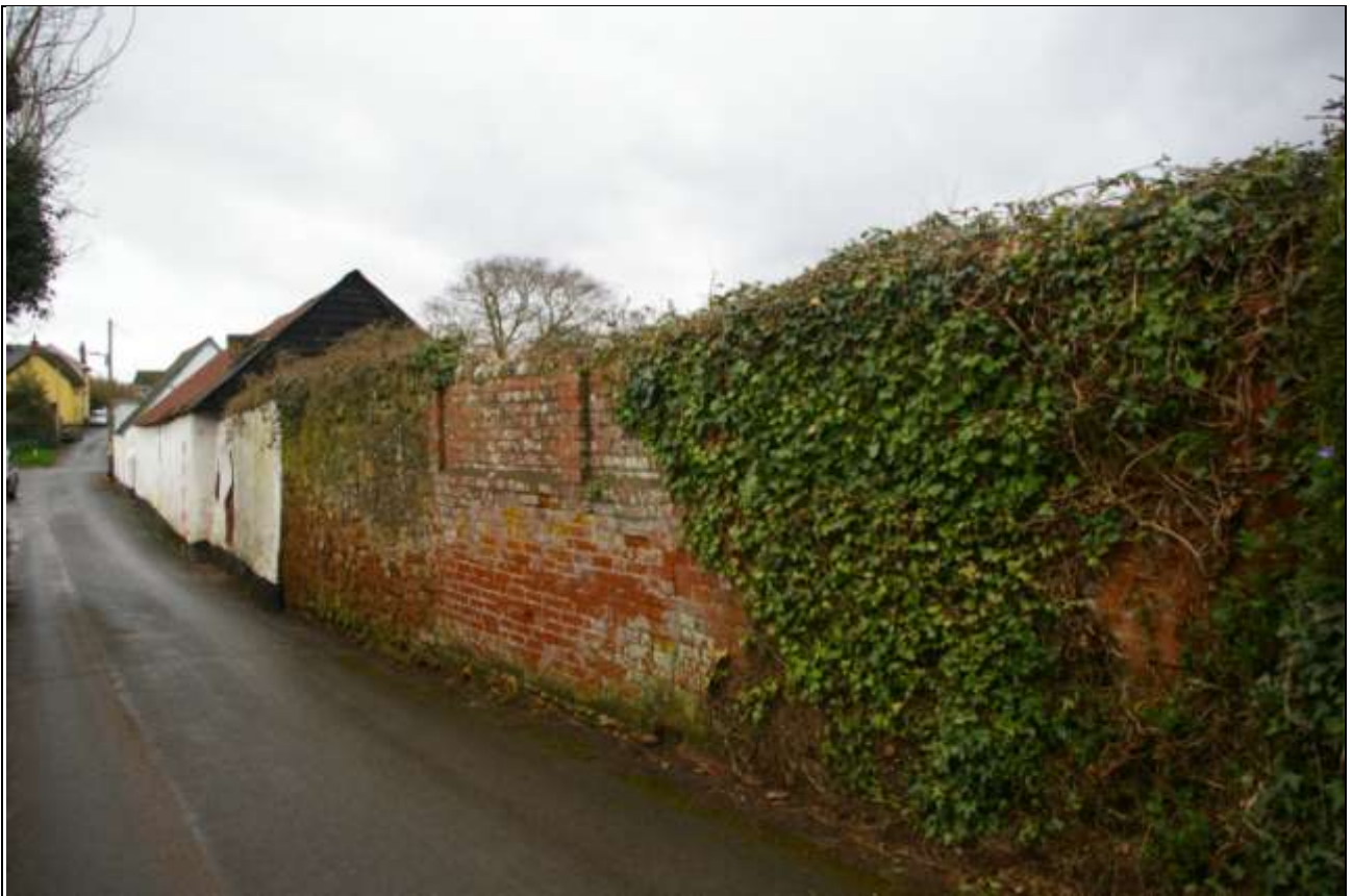
View along the phases of brick, dressed stone blocks and cob of the historic walling along Behind Hayes Lane; from the east, south-east
