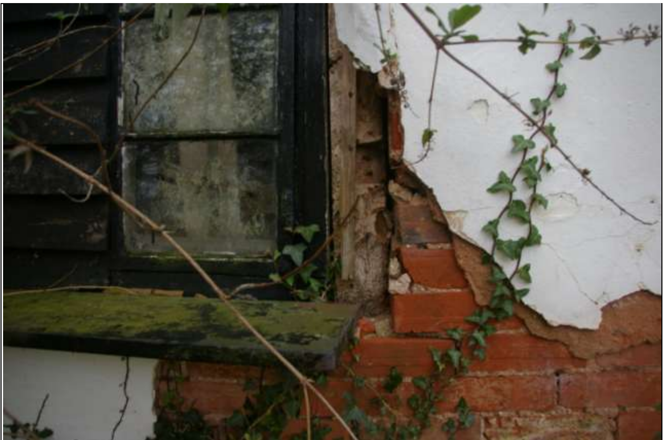
The heavy timbers which line the opening to the window in room 2; this may be the back of the heavy base cruck; from the north.
