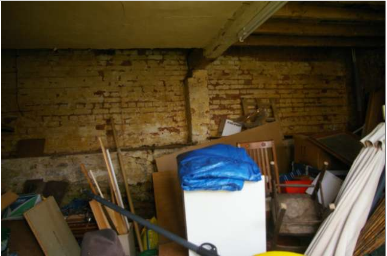
The south interior wall to the west end of the barn, showing the English Bond brickwork; from the north.
