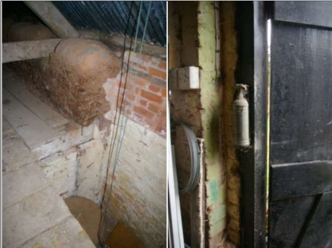
Left: The join between cob and brick on the south wall; from the north-west.
