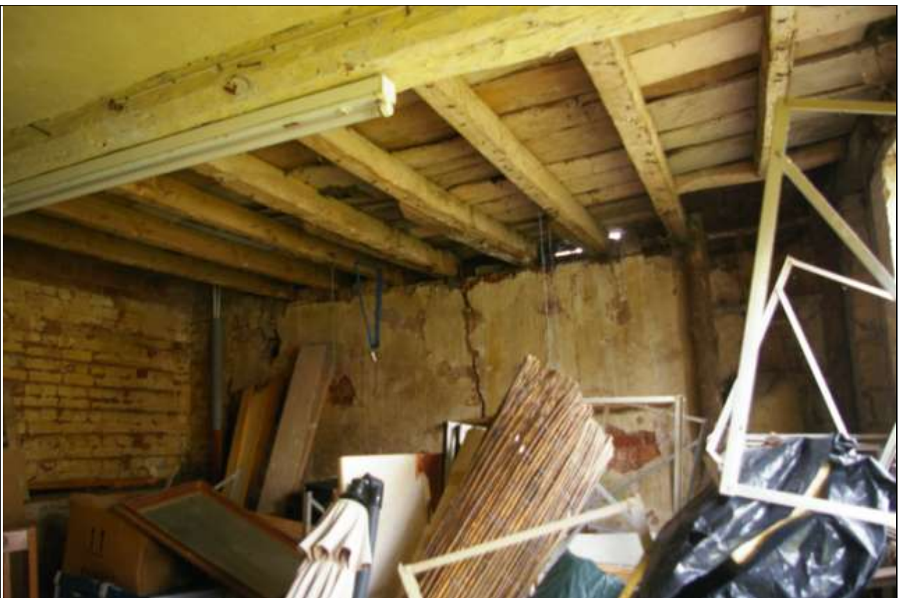
The brick west wall of the barn, showing the plaster on the inner face and heavy 19 th century beams and joists to the loft floor; from the east, north-east.
