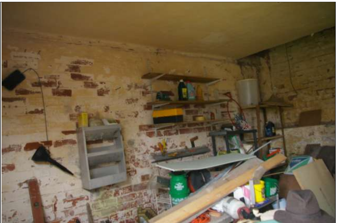
The brick partition wall, clearly not tied into the exterior walls, of Stretcher bond, possibly a later addition; from the north-west.
