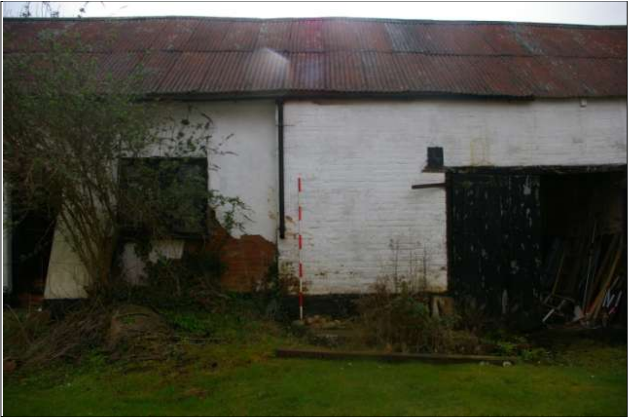
The north elevation, showing the older cob to the east and the brick to the west; from the north.
