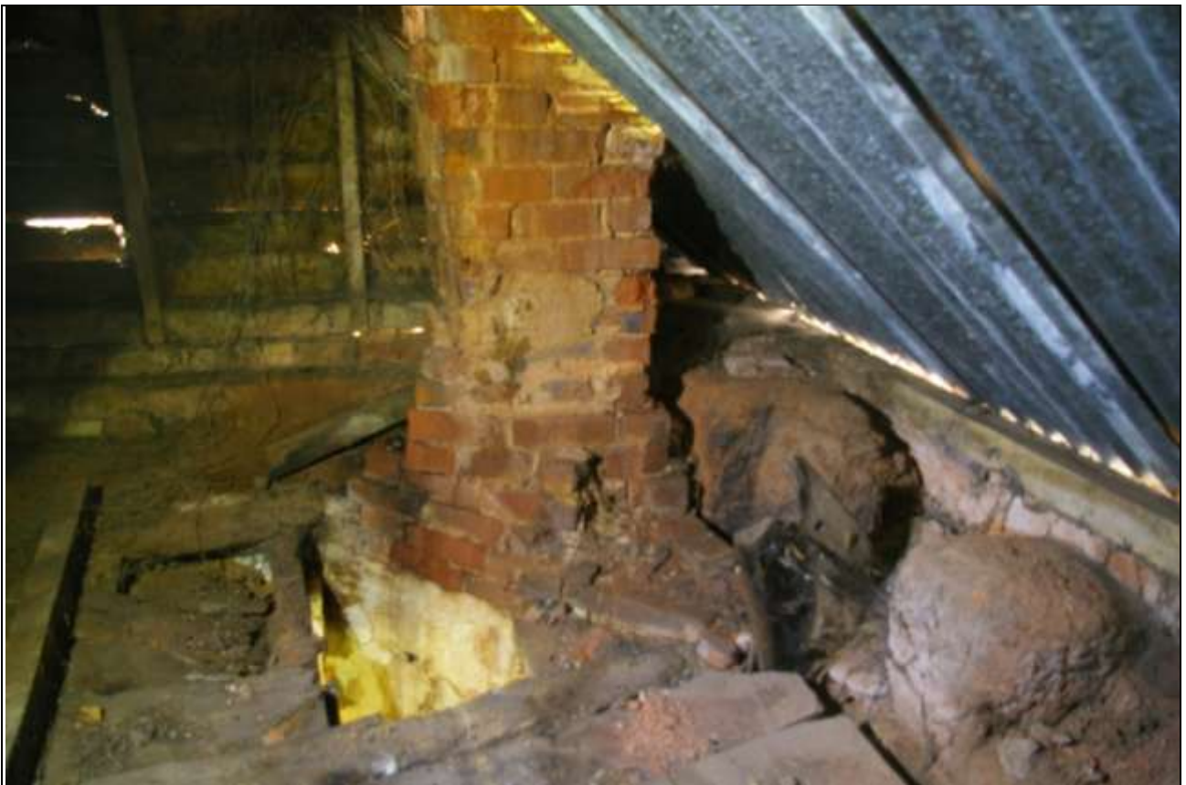
Brick stack, serving fireplace inserted into the room at the east end; from the west, north-west.
