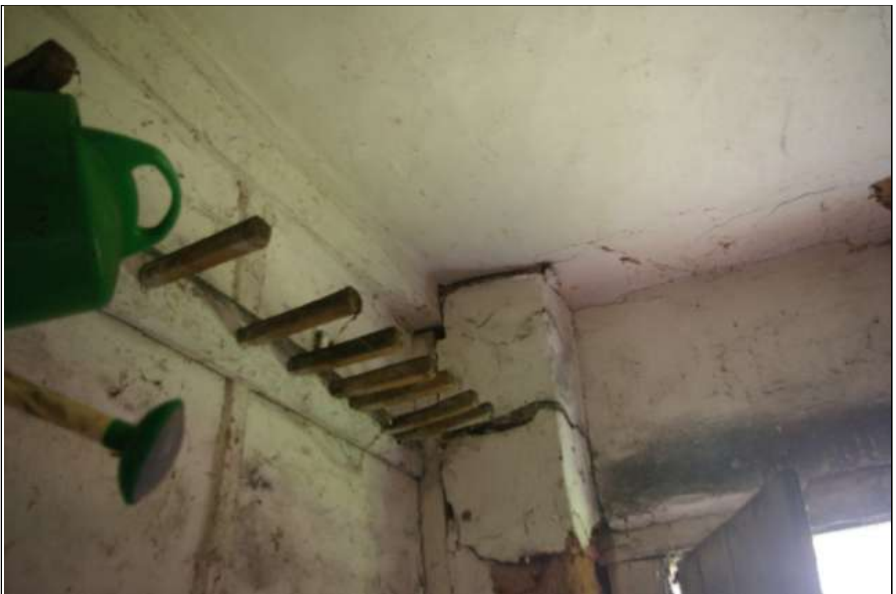
The heavy beam over the partition between room 1 and 2, showing its wide adze cut chamfer and run out stops. Also showing one of the narrow planks and long crude sets of pegs; from the south, south-east.
