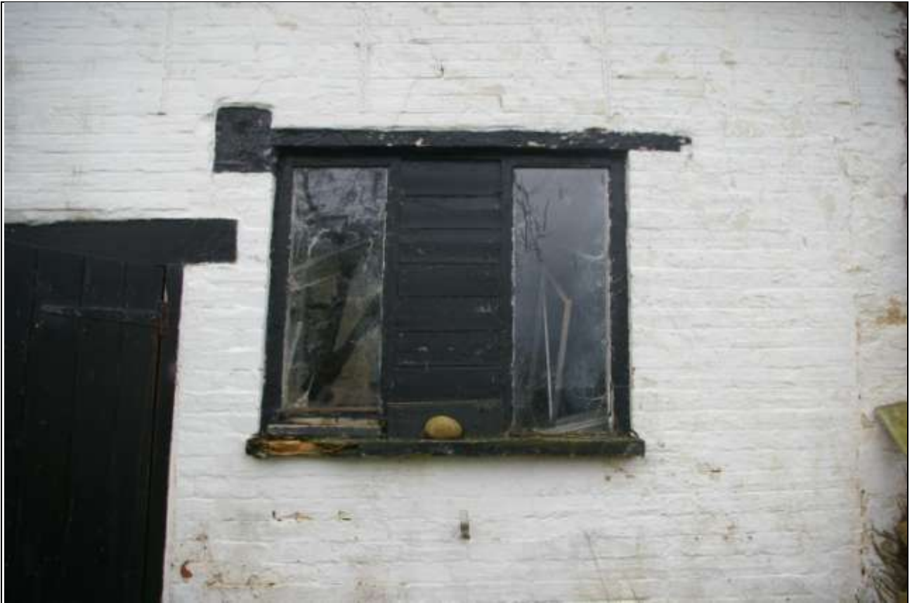
The three light window to the west end of the north elevation; from the north.
