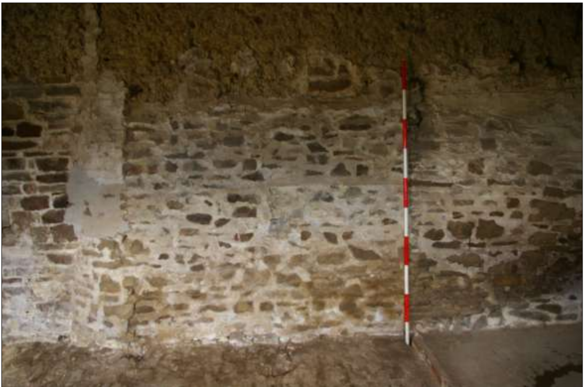
26. DETAIL OF THE INTERNAL ELEVATION OF THE NORTH WALL OF B1, WEST END, SHOWING MARKED PHASING, REBUILD AND INDICATION OF ALTERED USE; VIEWED FROM THE SOUTH (2M SCALE).
