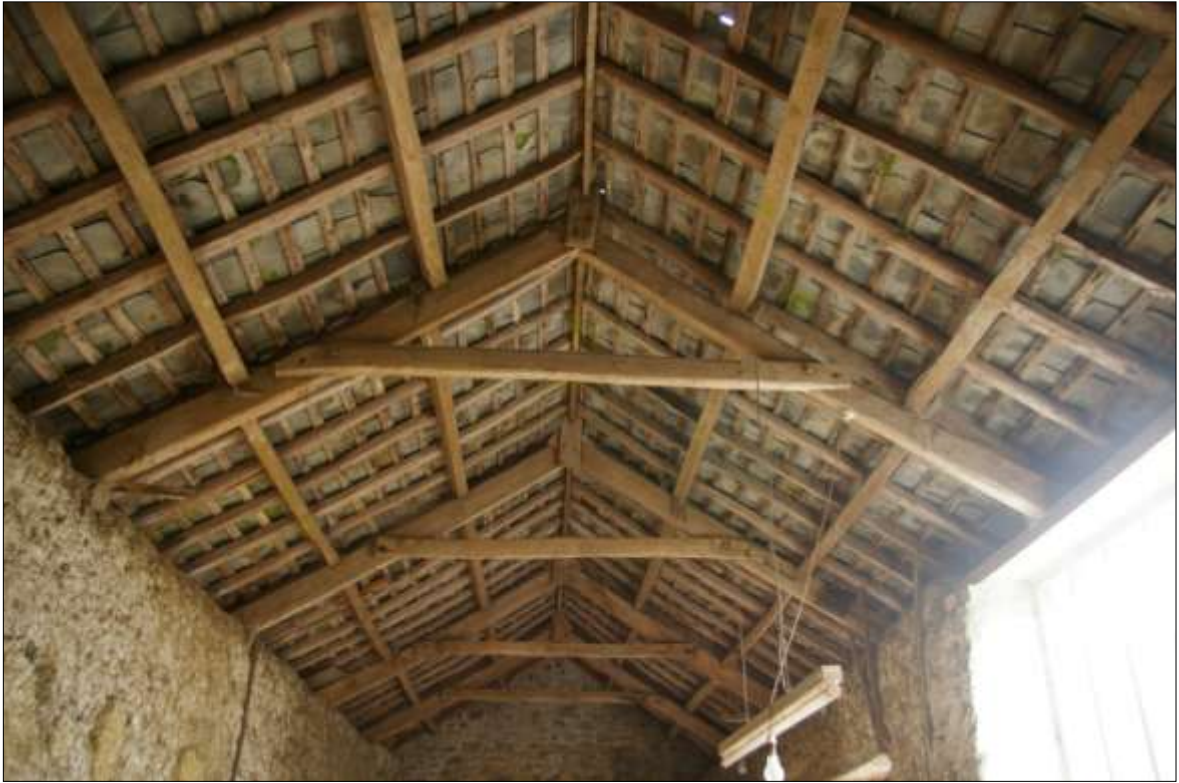
35. VIEW OF THE ROOF STRUCTURE OF B1; VIEWED FROM THE WEST (NO SCALE).
