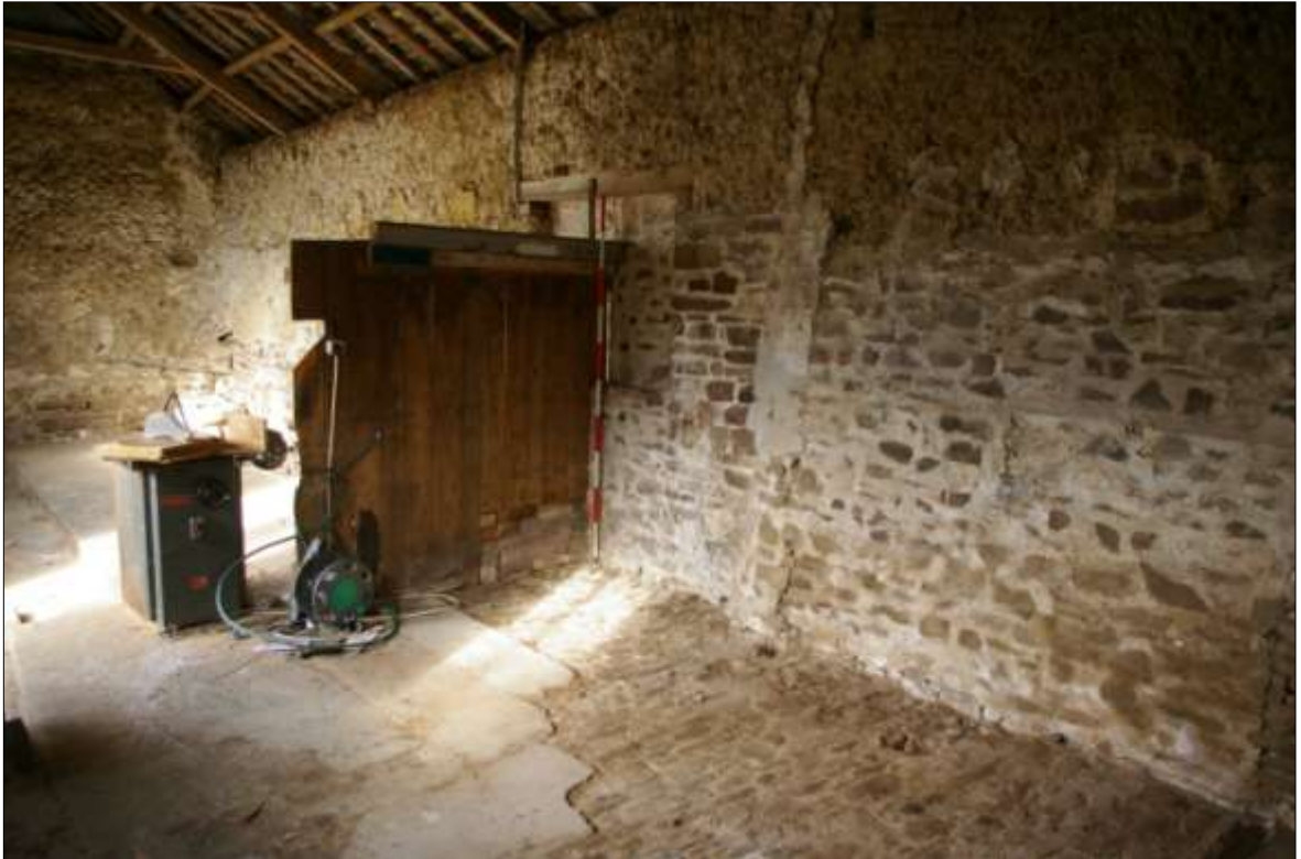
25. DETAIL OF THE COMPLEX PHASES OF BLOCKING OF THE DOORWAY WITHIN THE NORTH WALL OF B1 AND THE TIMBER SCREEN WHICH CURRENTLY DIVIDES THE INTERIOR SPACE OF THE OUTBUILDING; VIEWED FROM THE SOUTH-EAST (2M SCALE).
