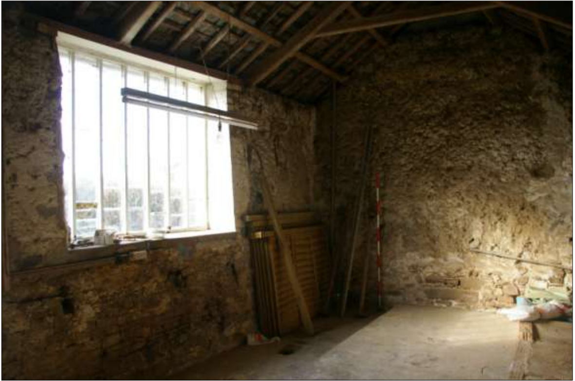
17. DETAIL OF THE SOUTH-WEST CORNER OF B1, SHOWING THE LARGE WINDOW WITHIN THE SOUTH WALL; VIEWED FROM THE NORTH-EAST (2M SCALE).
