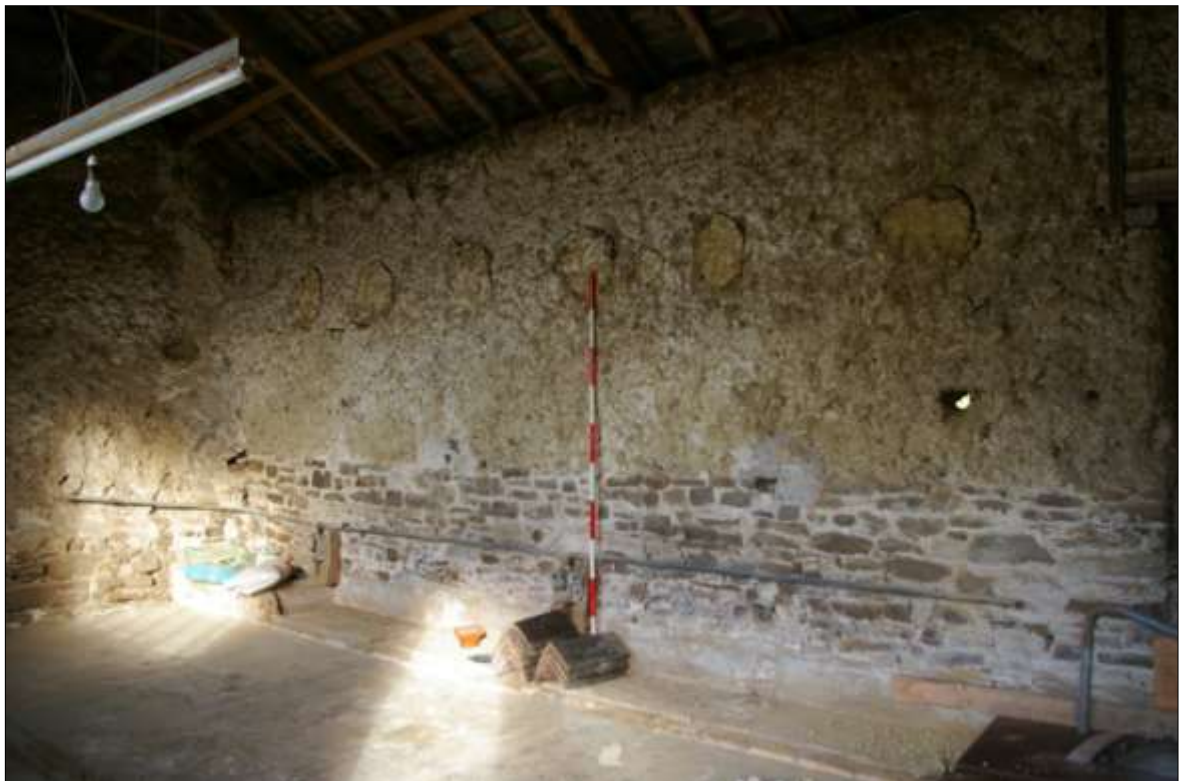
22. INTERNAL SOUTH ELEVATION OF THE NORTH WALL OF B1, WEST END, SHOWING THE INFILLED LARGE SOCKET HOLES FOR HEAVY BEAMS TO SUPPORT A LOFT FLOOR, EXPECTED TO CARRY A HEAVY LOAD; VIEWED FROM THE SOUTH-EAST (2M SCALE).
