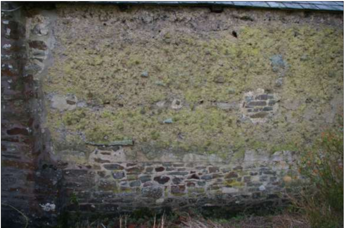
12. DETAIL OF THE DISTURBED COB AND LOOSER RUBBLE 'INFILL' AT THE EASTERN END OF THE NORTH EXTERNAL ELEVATION OF B1; VIEWED FROM THE NORTH (NO SCALE).
