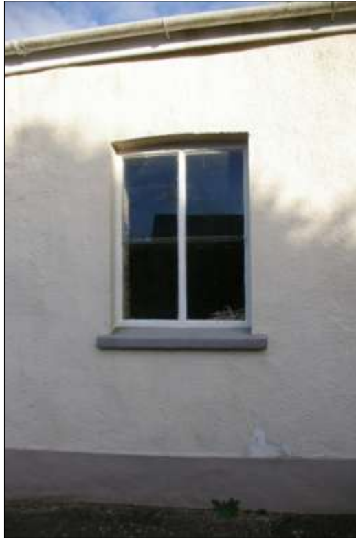
5. DETAIL OF THE TWO LIGHT WINDOW TO THE EAST END OF THE SOUTH EXTERNAL ELEVATION OF B1; VIEWED FROM THE SOUTH (NO SCALE).
