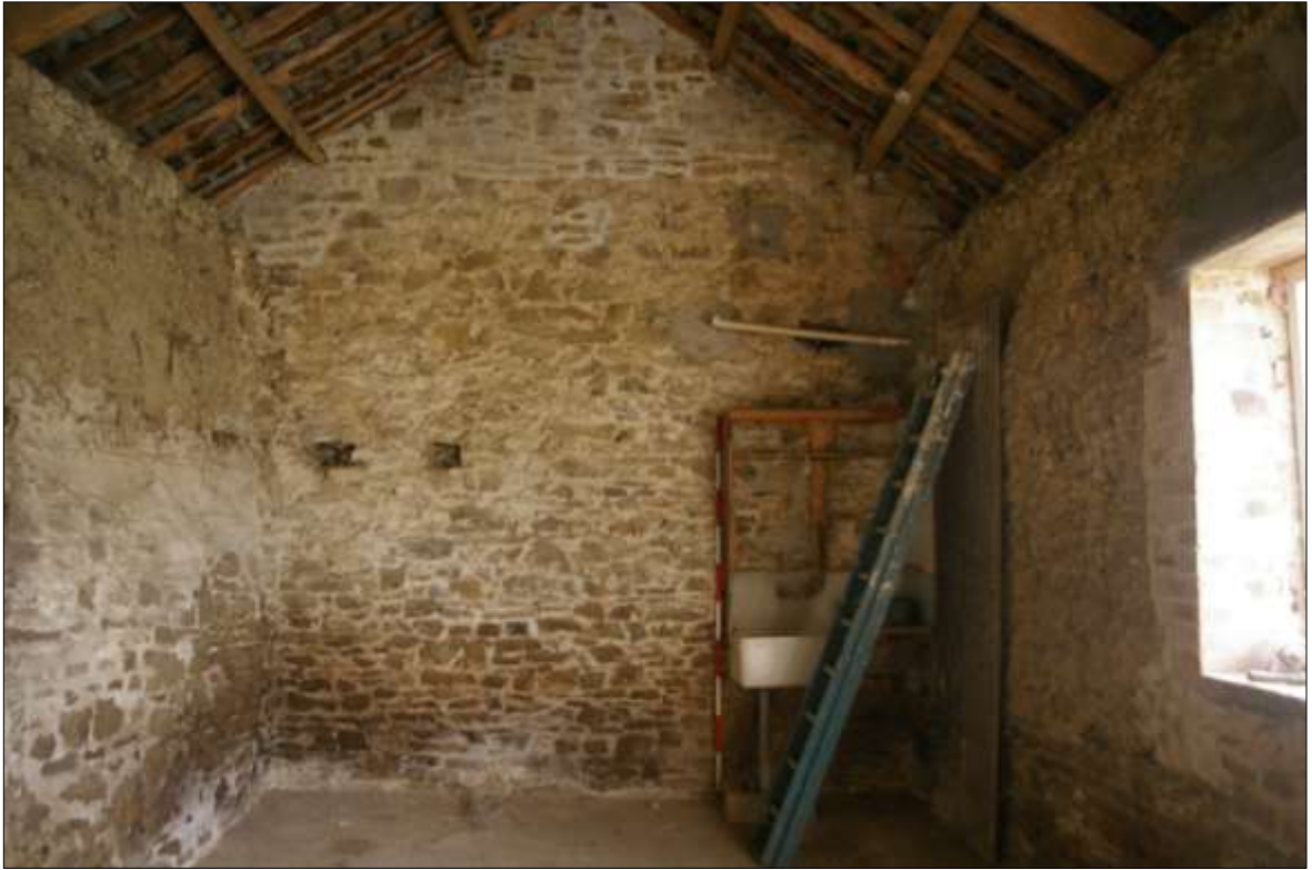
29. THE WEST GABLE OF DEVONIA, FORMING THE EAST WALL OF B1, SHOWING THE MESSILY REBUILT RUBBLE STONE; VIEWED FROM WEST (2M SCALE).
