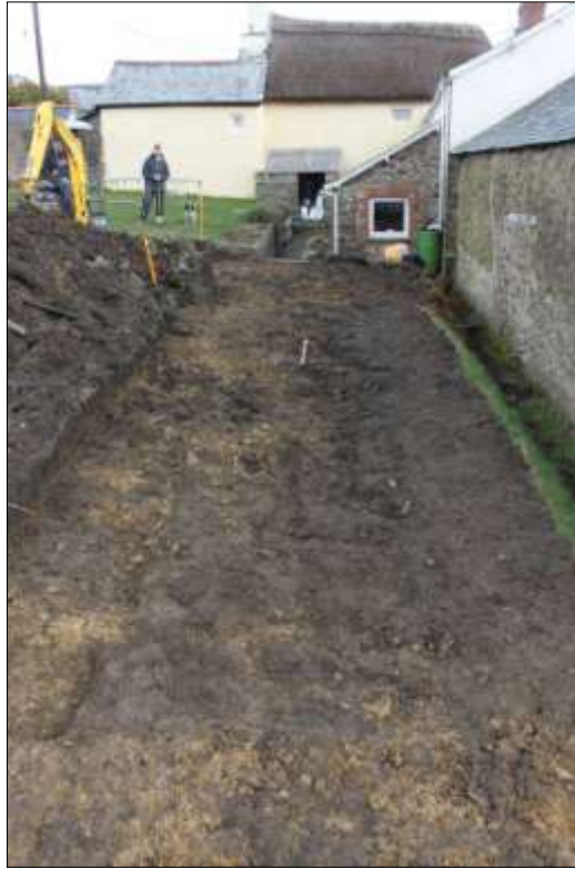
9. VIEW ACROSS EAST END OF SITE SHOWING DISTURBED GROUND ALONG LINE OF MODERN WATER PIPE; VIEWED FROM THE WEST (1M SCALE).
