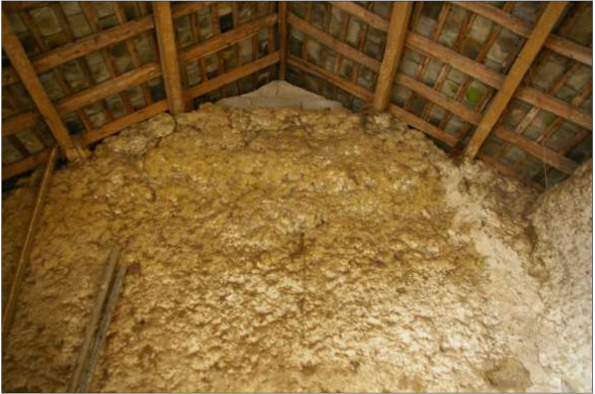
19. DETAIL OF THE INTERNAL WEST GABLE END OF B1 SHOWING THE UPPER REBUILT COB, IN A DIFFERENT MARKEDLY YELLOW COLOUR AND THE DEEP BATTERED SLOPE, POSSIBLY CAUSED BY COB SLUMPING DUE TO POORER QUALITY; VIEWED FROM THE EAST (NO SCALE).
