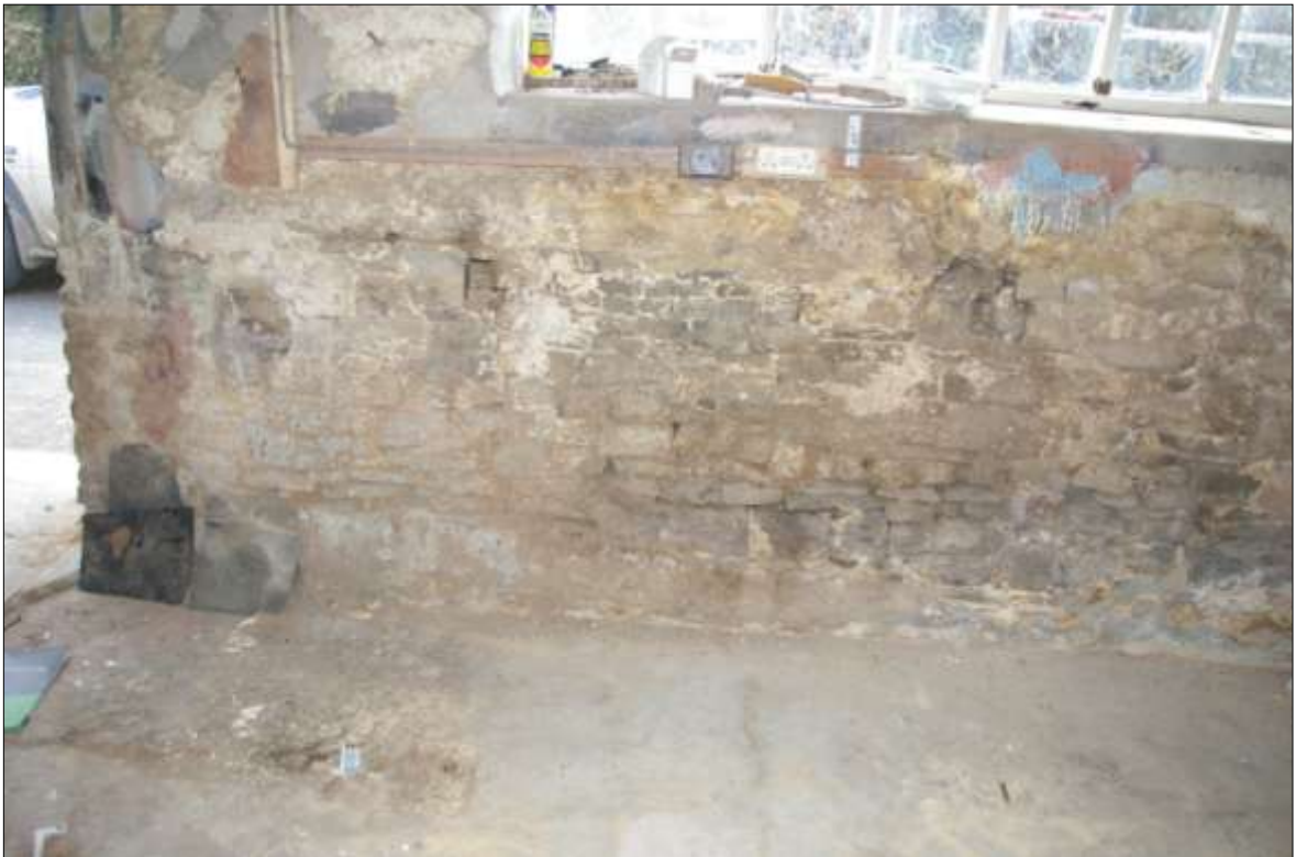
16. DETAIL OF THE INTERNAL ELEVATION OF THE SOUTH WALL OF B1 SHOWING DETAIL OF THE GOOD QUALITY SHAPED BLOCKY SEMI-COURSED EARLY POST-MEDIEVAL STONEMWORK BENEATH THE LARGE WINDOW; VIEWED FROM THE NORTH (NO SCALE).
