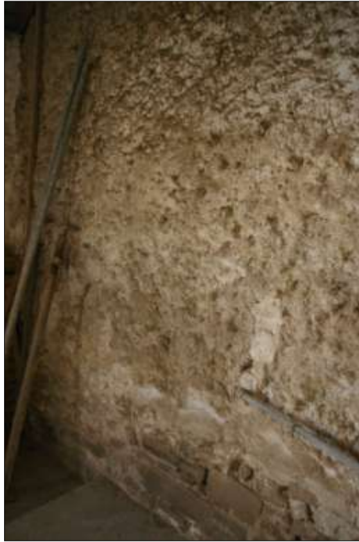
21. DETAIL OF THE INTERNAL ELEVATION OF THE WEST GABLE WALL OF B1 SHOWING THE SLUMPING OF THE COB AND CLEAR BUILD LINES; VIEWED FROM THE NORTH-EAST (NO SCALE).
