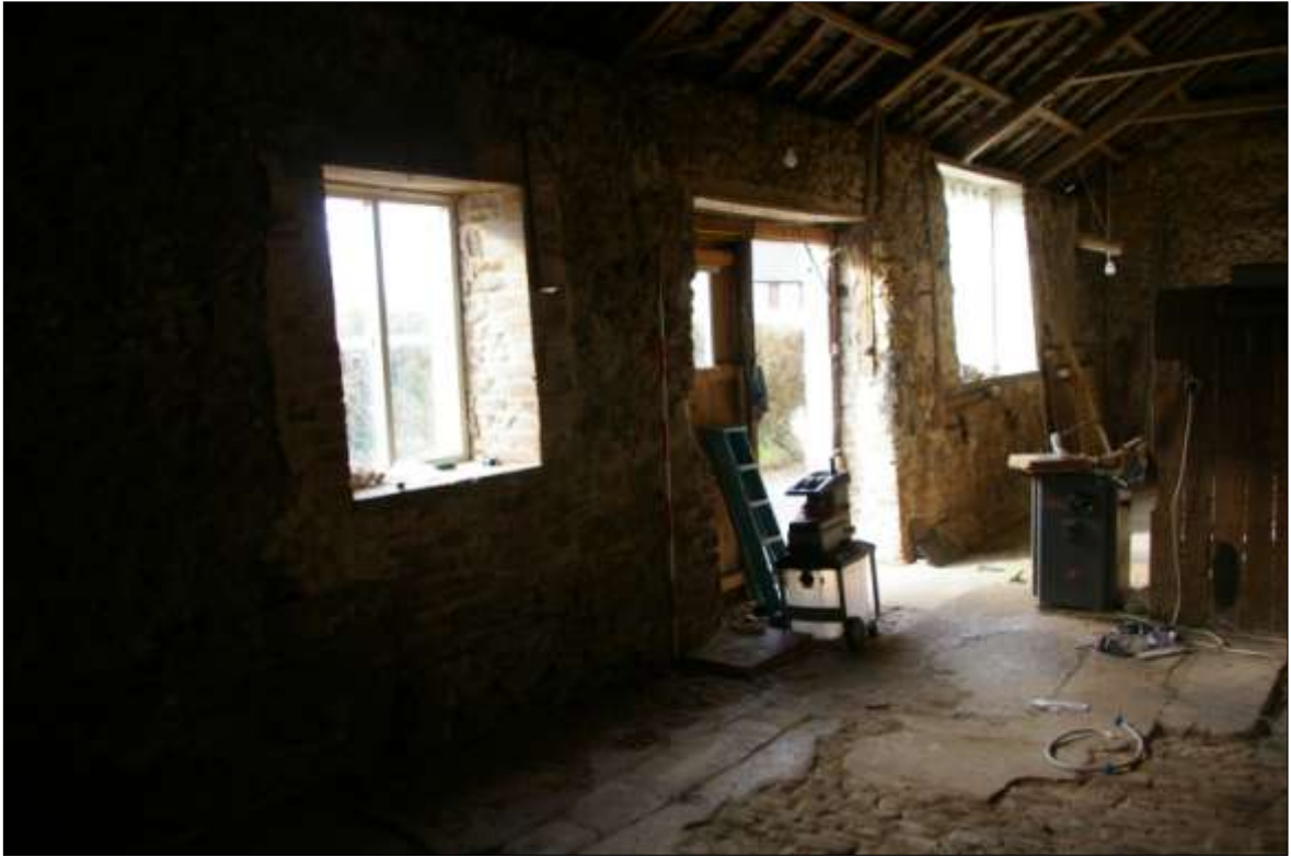
15. INTERNAL NORTH ELEVATION OF SOUTH WALL OF B1; VIEWED FROM THE NORTH-EAST (2M SCALE).
