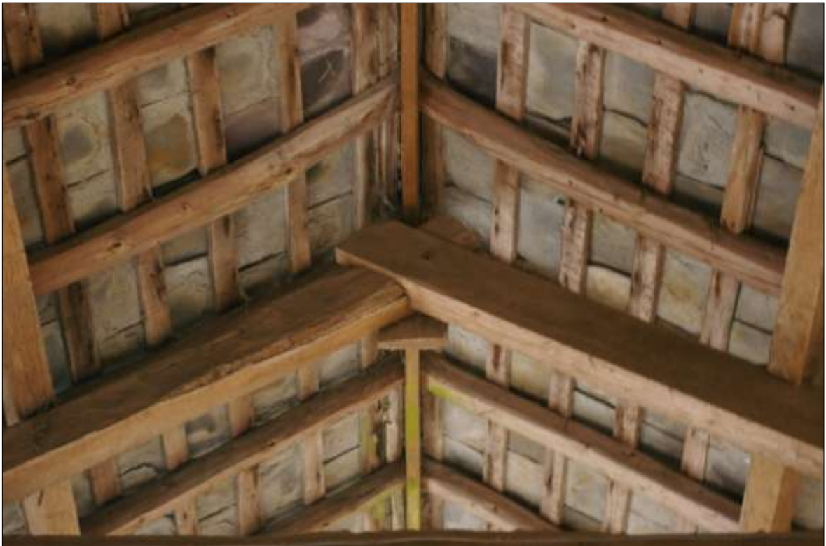
36. DETAIL OF THE ROOF STRUCTURE WITHIN B1 SHOWING THE APEX OF THE TRUSS AND HOW THE RIDGE PLANK, RAFTERS AND BATTENS BELONG TO A MORE MODERN ROOF RESTING ON THE TRUSSES AND ARE NOT CONTEMPORARY, THE TRUSS APEX NOT SUPPORTING IT; VIEWED FROM THE EAST (NO SCALE).
