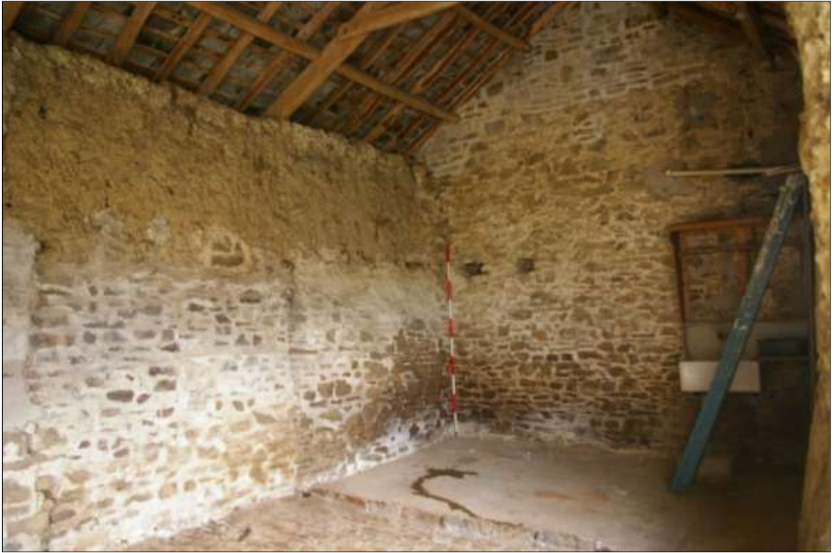
27. DETAIL OF THE INTERNAL NORTH-EAST CORNER OF B1, SHOWING THE RELATIONSHIP OF NORTH WALL AND WEST GABLE OF HOUSE; VIEWED FROM THE SOUTH-WEST (2M SCALE).
