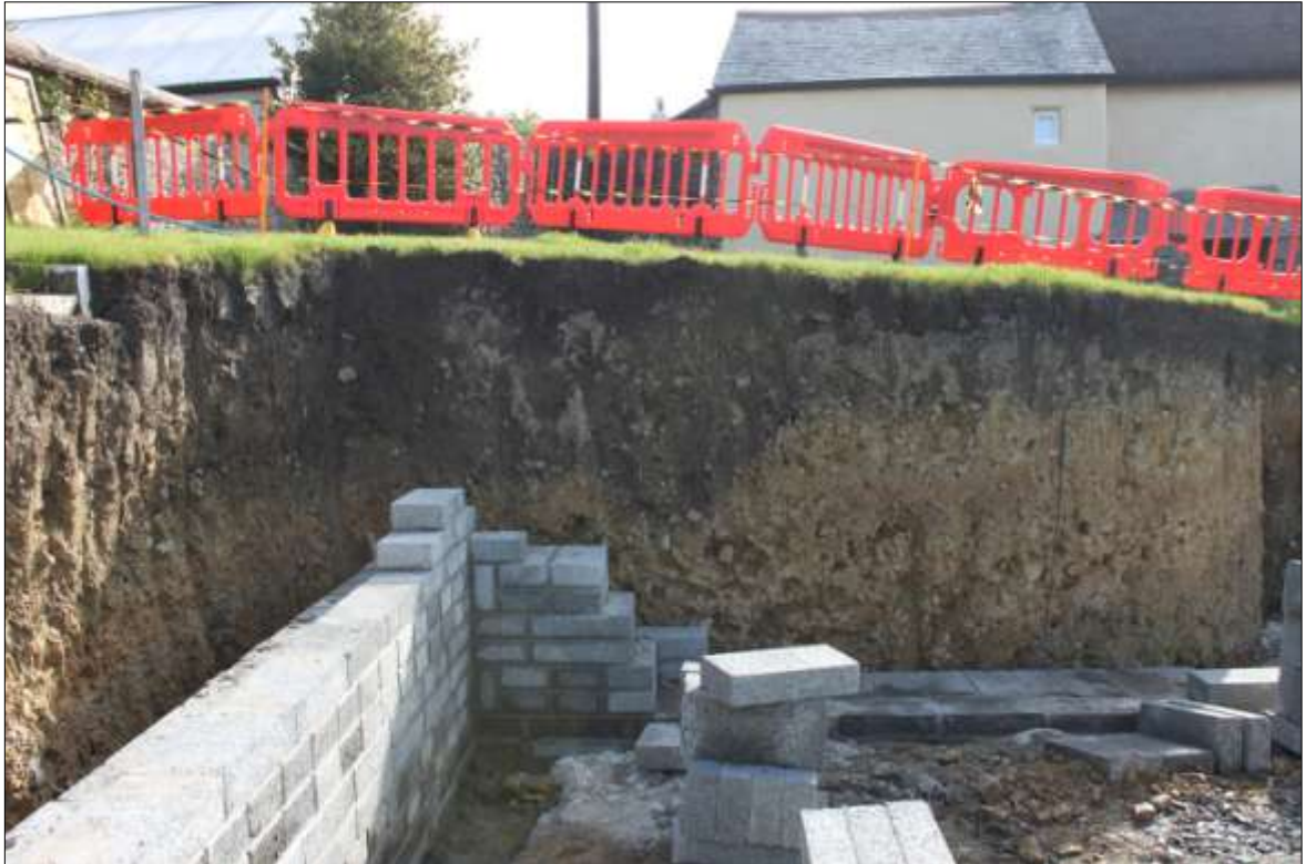
14. EAST FACING SITE SECTION FOLLOWING FULL SITE EXCAVATION, SHOWING DITCH [106] CONTINUING BEYOND THE LIMITS OF EXCAVATION; VIEWED FROM THE WEST (NO SCALE).
