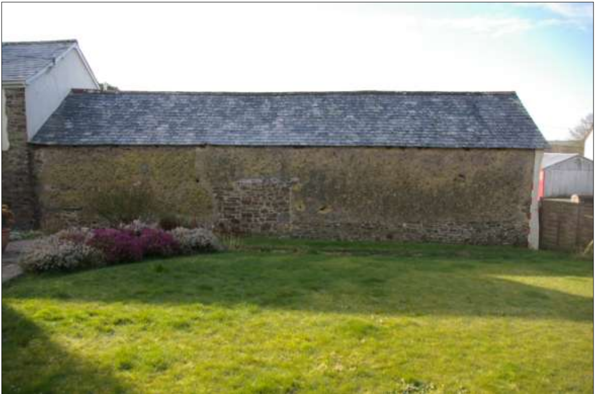
10. THE NORTH EXTERNAL ELEVATION OF B1; VIEWED FROM THE NORTH (2M SCALE).
