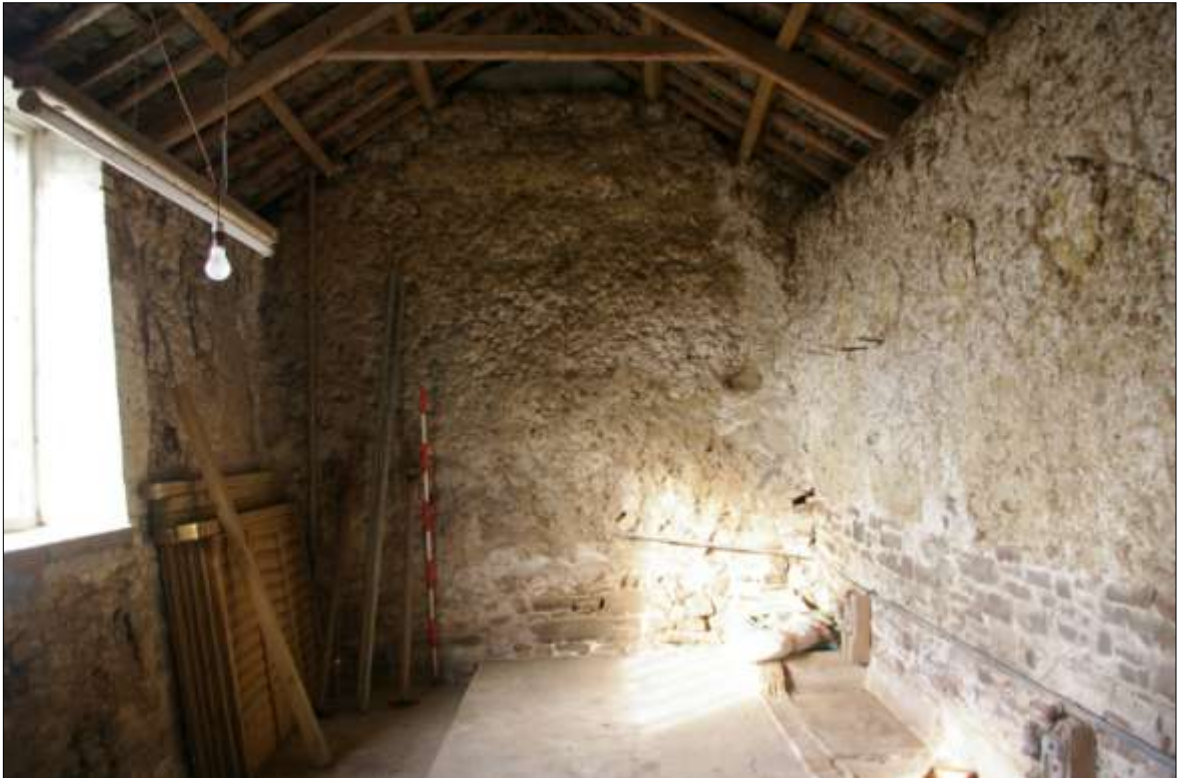
18. INTERNAL ELEVATION OF THE WEST GABLE END OF B1; VIEWED FROM THE EAST (2M SCALE).
