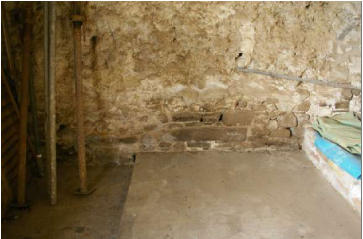
20. DETAIL OF THE LOW AND POORLY BUILT LOOSE RUBBLE TO THE BASE OF THE WEST GABLE WALL OF B1; VIEWED FROM THE EAST (NO SCALE).
