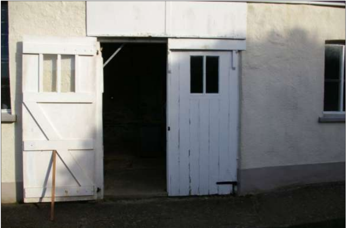
6. DETAIL OF THE CENTRAL DOUBLE DOORWAY IN THE SOUTH EXTERNAL ELEVATION OF B1; VIEWED FROM THE SOUTH (NO SCALE).
