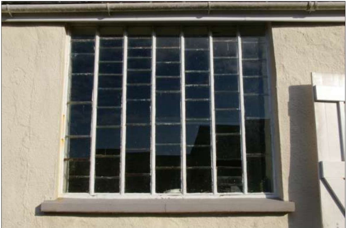
8. DETAIL OF THE WESTERN WINDOW IN THE SOUTH EXTERNAL ELEVATION OF B1; VIEWED FROM THE SOUTH (NO SCALE).
