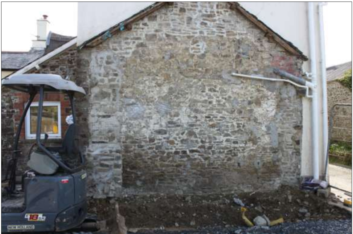
15. VIEW OF THE WEST WALL OF DEVONIA FOLLOWING DEMOLITION OF THE OUTBUILDING, SHOWING EARTH BASE LAYER IDENTIFIED BENEATH THE FLOOR LAYERS; VIEWED FROM THE WEST (NO SCALE).
