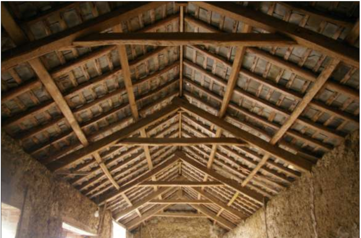
34. VIEW OF THE ROOF STRUCTURE WITHIN B1; VIEWED FROM THE EAST (NO SCALE).
