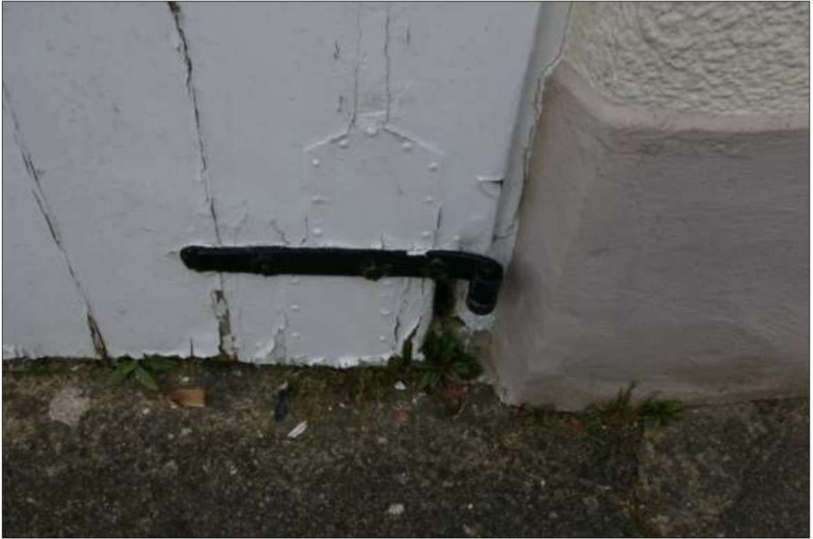
7. DETAIL OF IRONWORK DOOR FURNITURE TO THE DOUBLE DOORS IN SOUTH WALL OF B1; VIEWED FROM THE SOUTH (NO SCALE).
