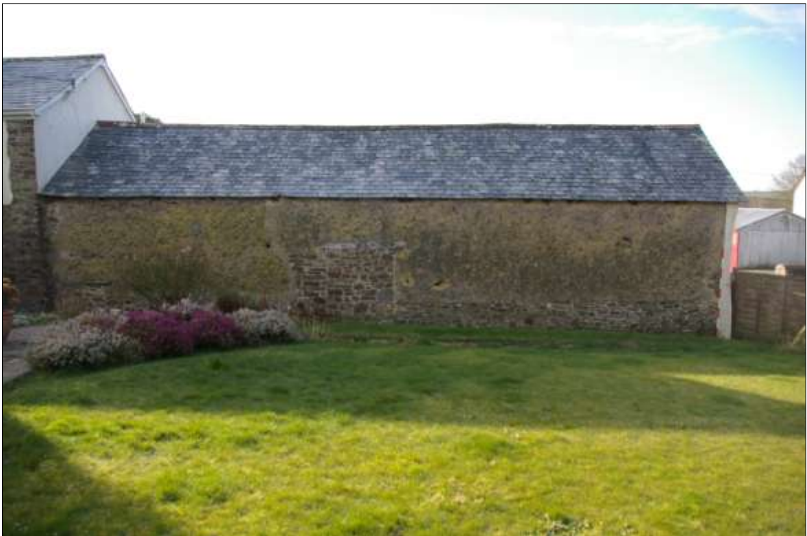
FIGURE 7: THE EXTERNAL ELEVATION OF THE NORTH WALL OF B1 SHOWING PHASES OF THE STONE AND COB CONSTRUCTION, WITH BLOCKED DOORWAY TOWARDS THE CENTRE; VIEWED FROM THE NORTH (2M SCALE).
