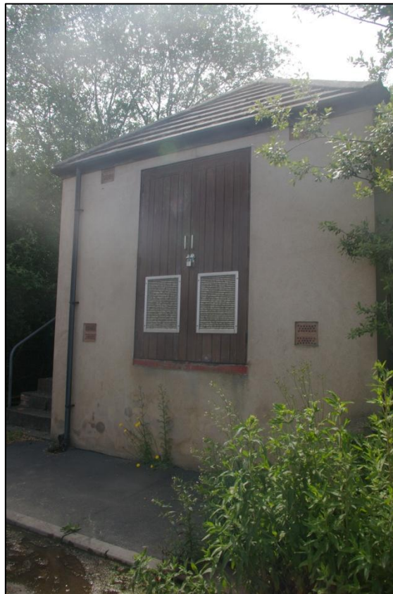
FIGURE 13: VIEW OF THE ELECTRICITY SUBSTATION FOR WESTERN POWER, WHICH STANDS IN A SMALL FENCED ENCLOSURE ON THE EASTERN SIDE OF THE SITE, TOWARDS THE NORTHERN END; FROM THE EAST. NORTH EAST.
