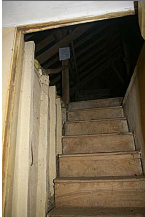
The lath and plaster and timber framing of the loft stair, with timber plank treads and risers; from the west-south-west.
