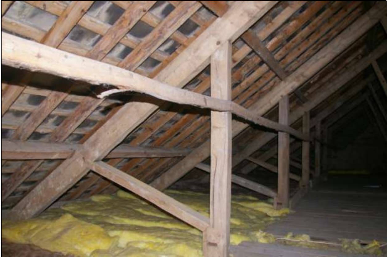
The aisle posts, with additional struts and the later hand-rail; viewed from the north-east.
