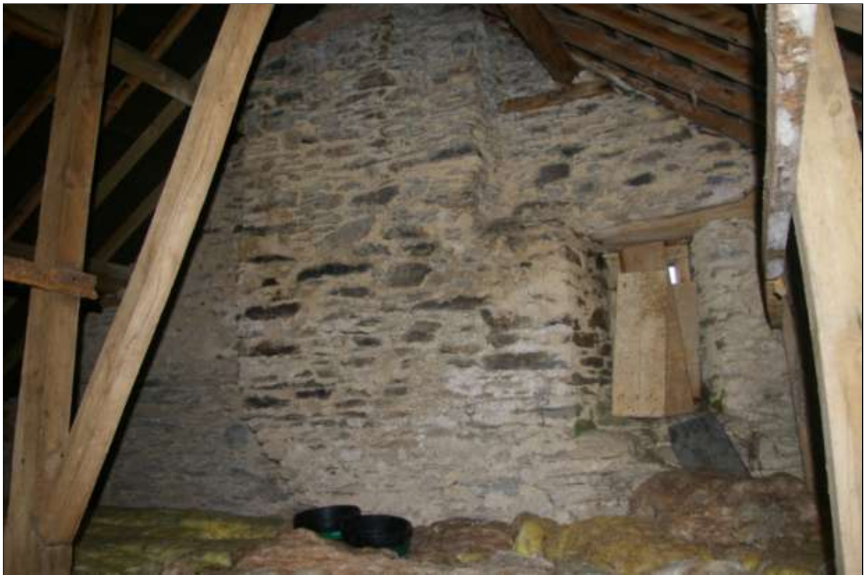
The east gable end wall, with chimney stack and small window; from the south-west.
