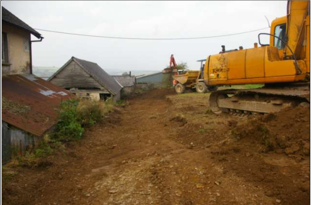
View down Area 1, the open stripped area, with top soil removed; from the east.
