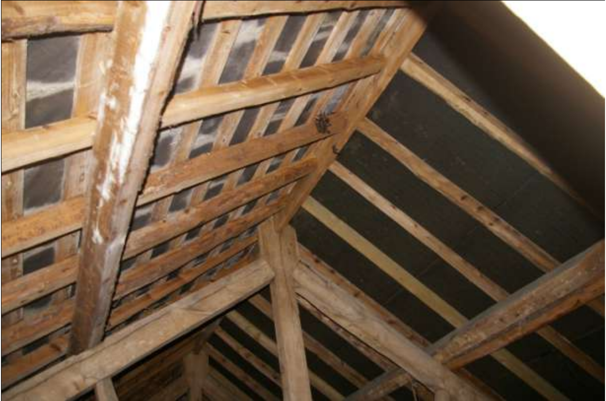
Detail of the ridge pole and upper sets of purlins; from the south-east.
