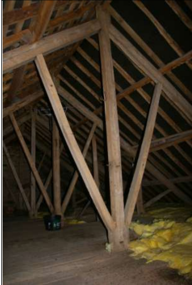
Figure 7: Detail of one of the trusses, king post, with long fine queen struts; from the south-east.
