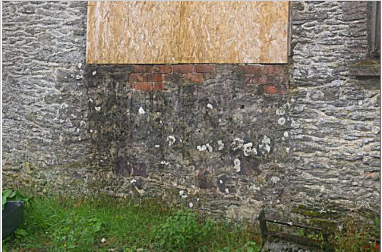
Detail of the blocked window opening, formerly doors, into which the window is set; from the north-west.
