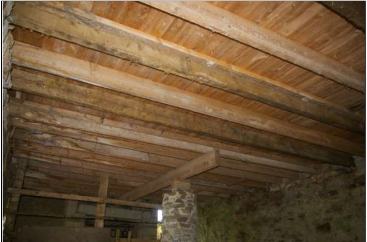
The joists to the west end of the barn, supporting the floor; from the south-east.
