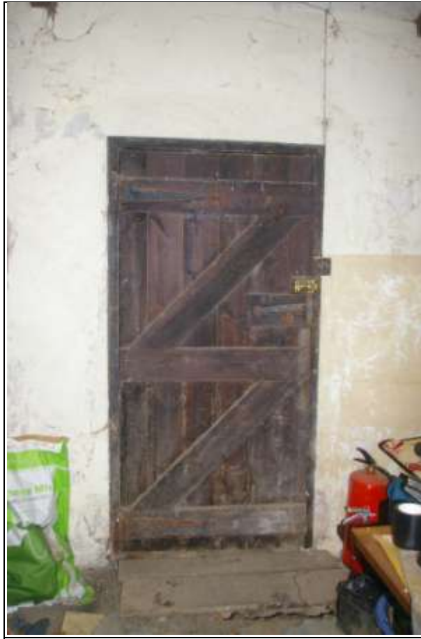
Figure 10: The doorway through the north elevation, which provides access to the first floor; from the south.
