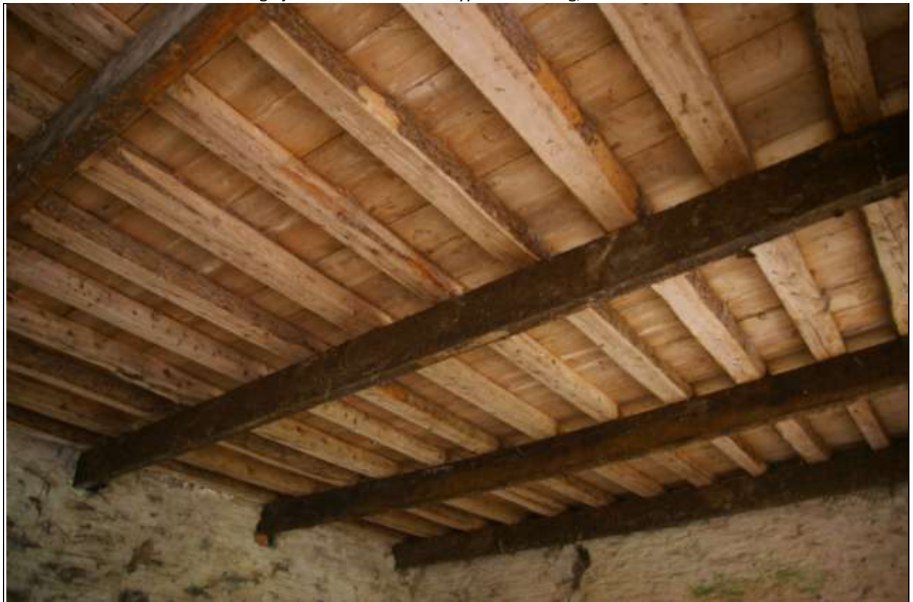
The heavy two phases of joists to the east end of the floor; from the south-west.
