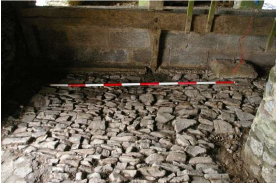
Concrete block wall and timber partition to the west end of the cobbled floor, with 2m scale; from the east.
