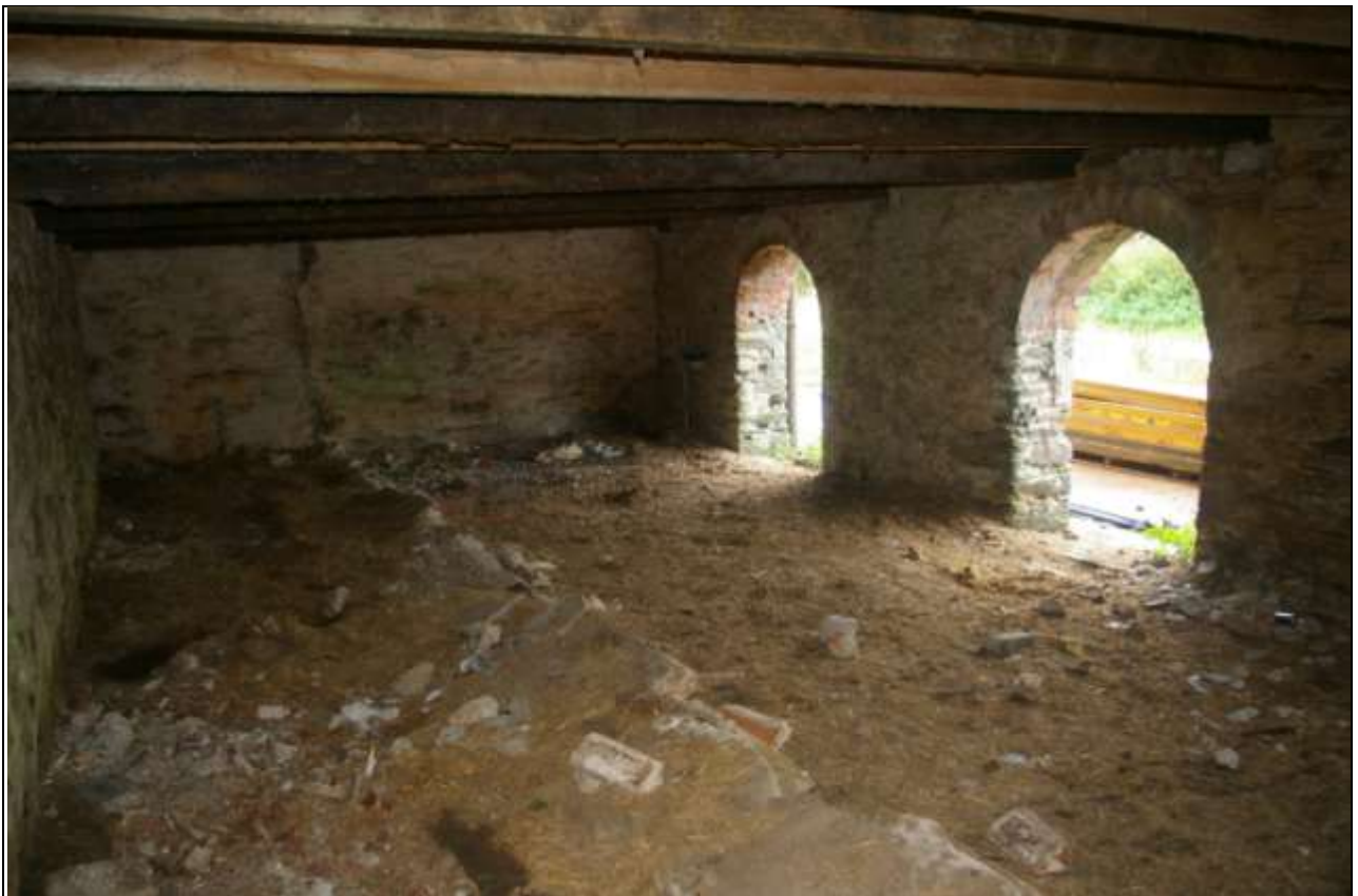
The ground floor interior, part raised feed passage and demolished troughs; from the north-west.
