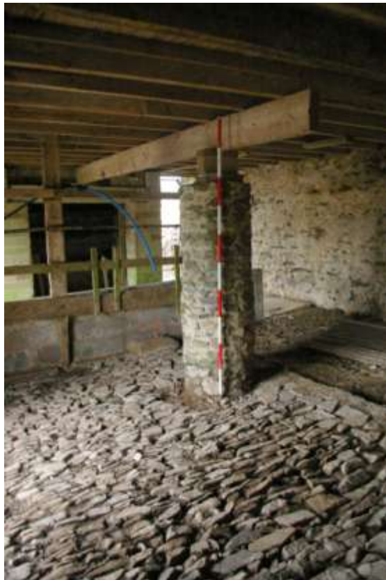
Stone pillar, forced into the cobbled floor, with 2m scale; from the south-east.
