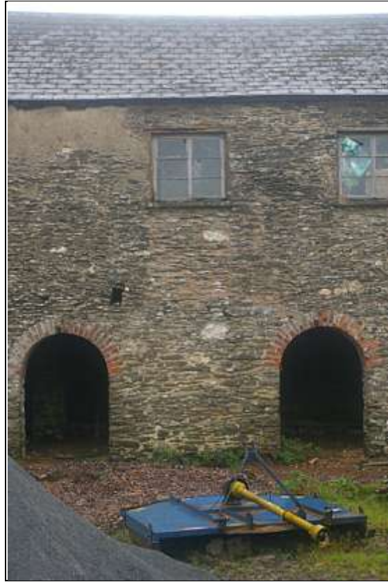
View of the metal window in the blocked loading door opening, to the centre of the south elevation; from the south.
