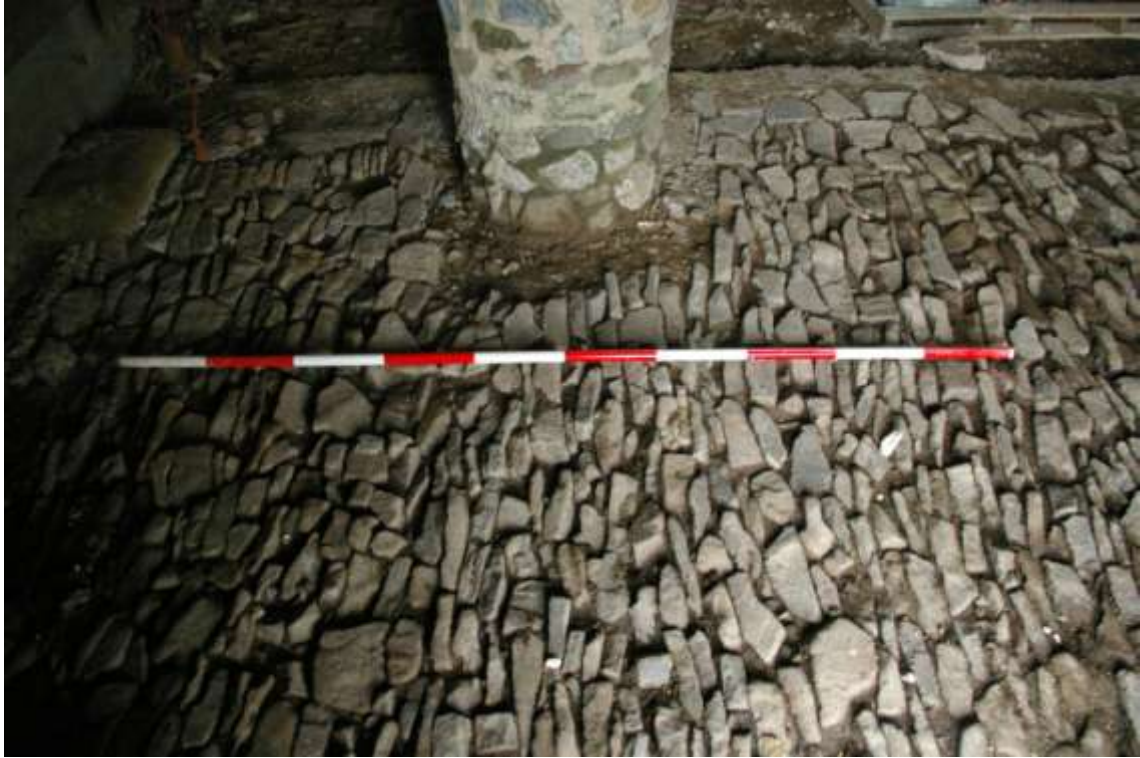
Damaged section of floor with stone pillar inserted; from the south.
