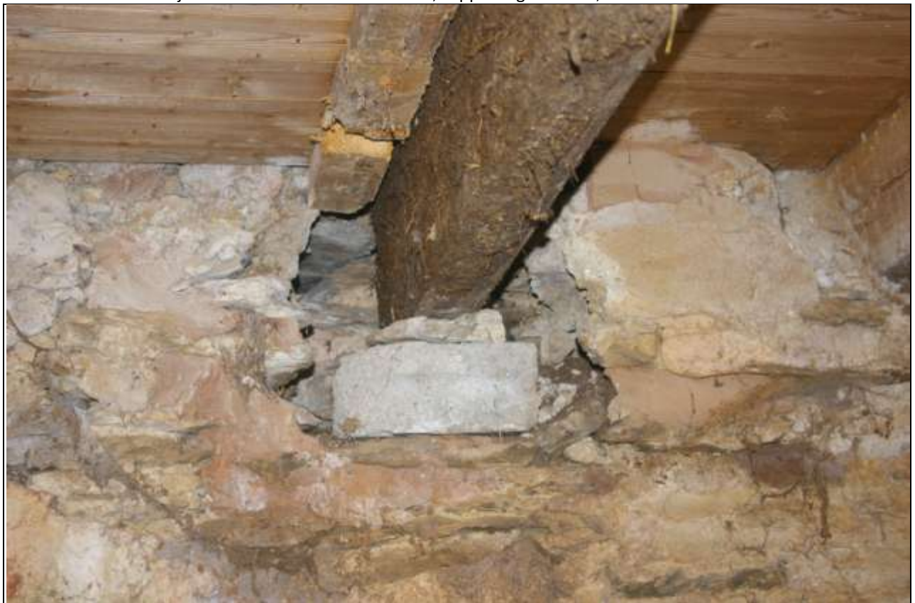
Detail of one of the joists to the east end, resting on a loose stack of rubble and a concrete block.
