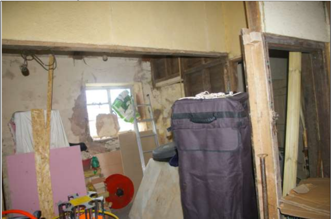
The hallway area to the east of the first floor; from the north-north-east.
