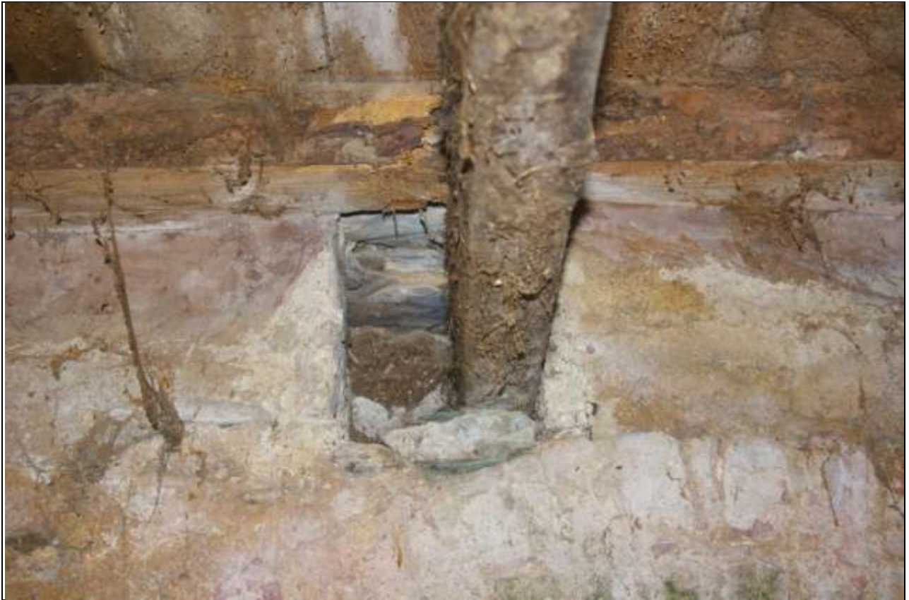
Detail showing the size and form of the built sockets, within the structure; from the north.
