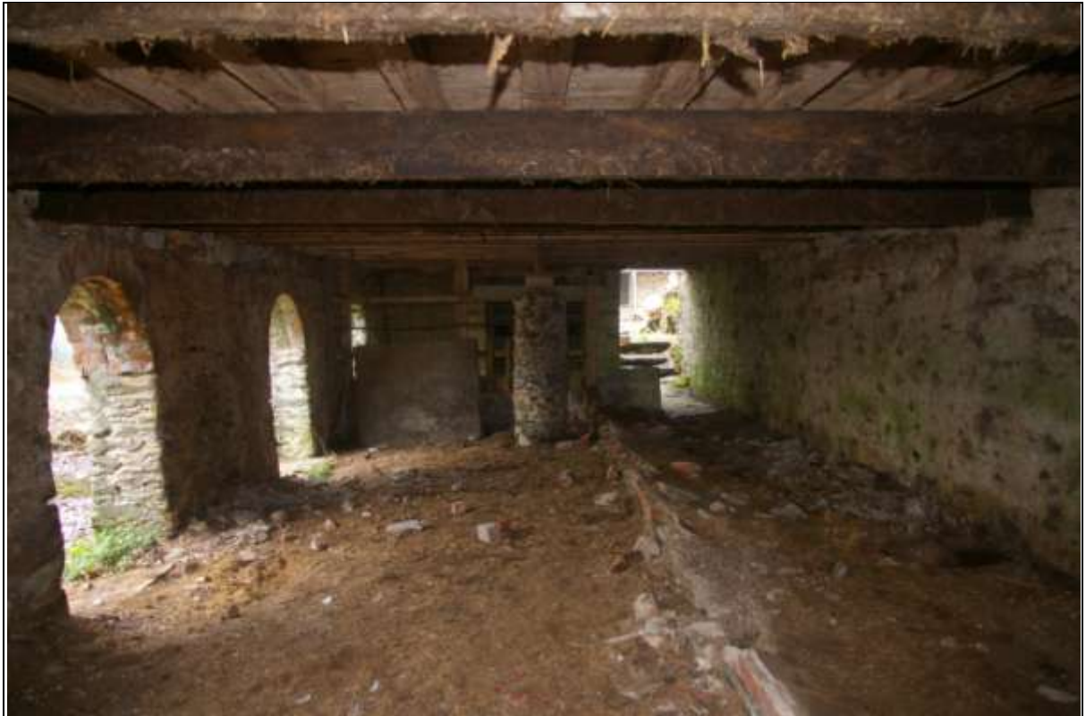
Figure 9: The ground floor interior of the East Barn; viewed from the east.
