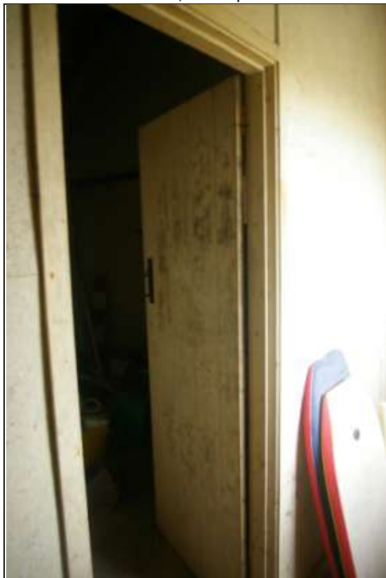
One of the plank doors providing access off the corridor; from the south-west.
