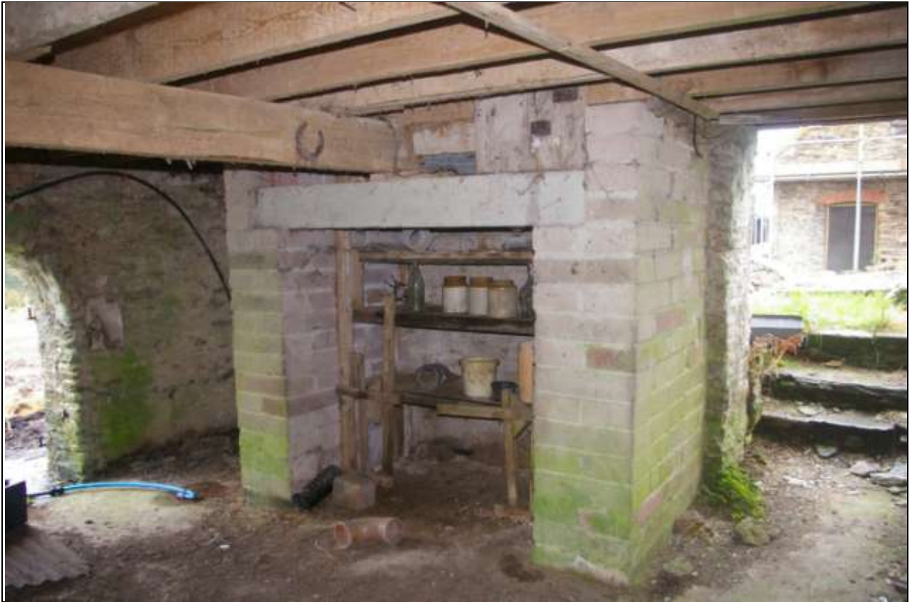
The large concrete block structure which supports the first floor brick chimney stack; from the north-north-east.
