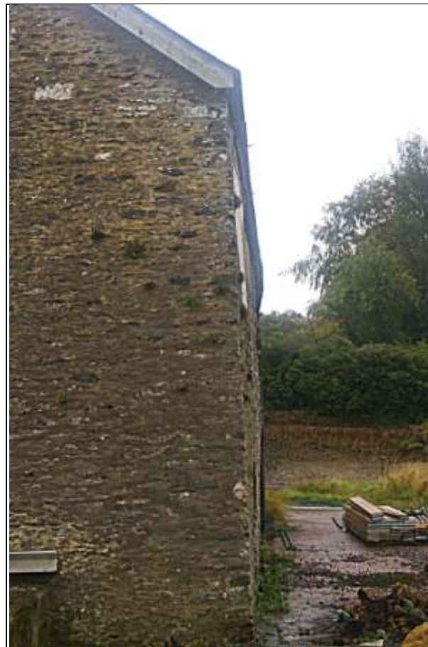
View down the front, south elevation, showing the bowed profile of the wall; from the west.
