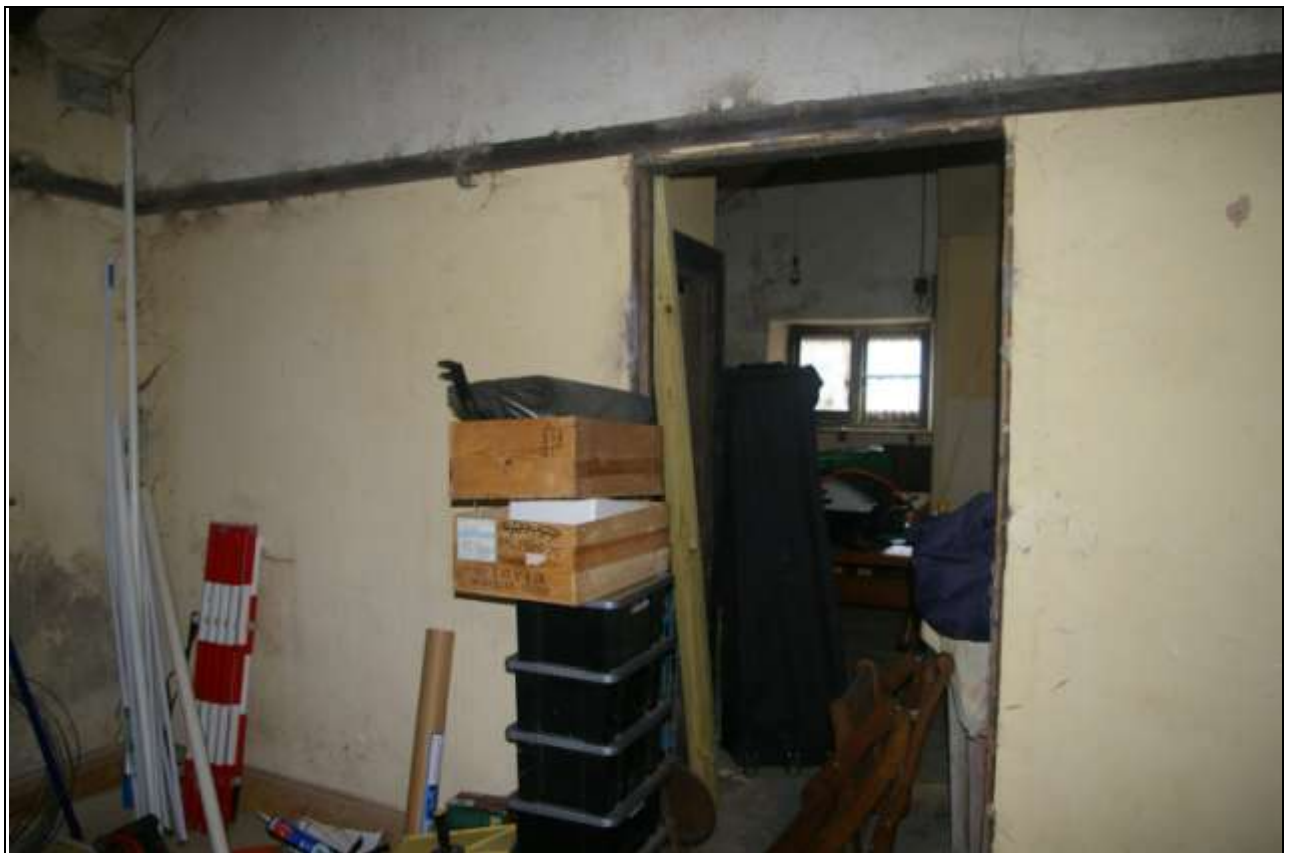
Detail of the skirting and picture rail in the artist's studio; from the west-south-west.
