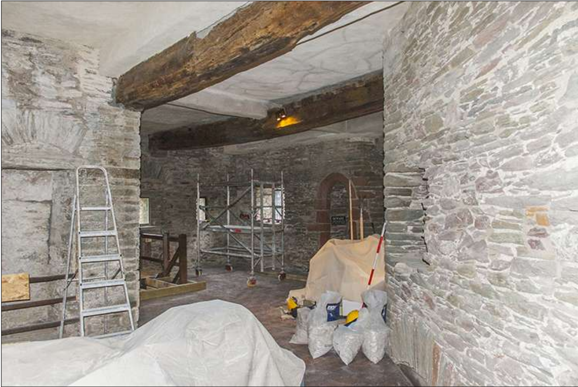
Figure 2: 6060 View through from the round tower into the main chamber; viewed from the north-west.
