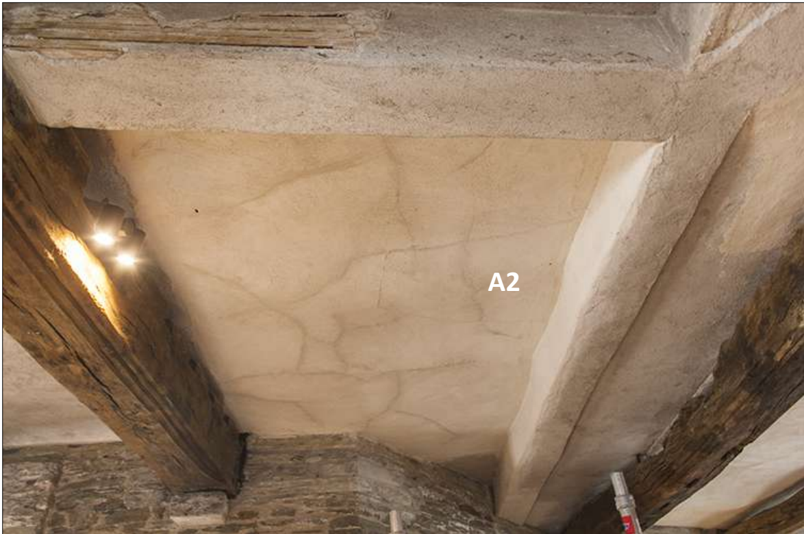
Figure 17: 6020 Area 2 scratch marks; viewed from the north east.
