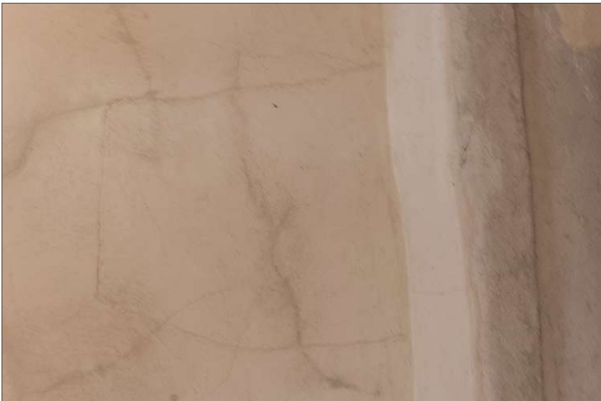
Figure 18: 6094 Area 2 scratch marks; viewed from the east.
