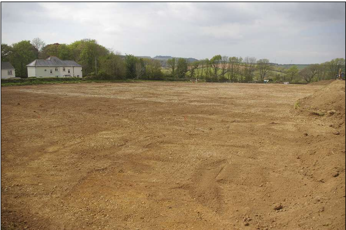
SITE SHOT FROM THE SOUTH-EAST CORNER; VIEWED FROM THE SOUTH-EAST (NO SCALE).
