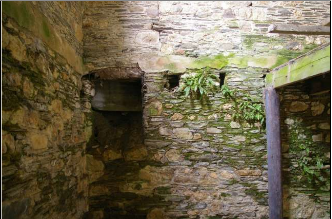
FIGURE 41: THE FORCED OPENING IN THE NORTH-WEST CORNER OF BARN B; FROM THE SOUTH.
