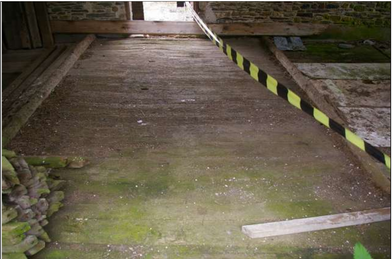
FIGURE 5: SECONDARY PEGGED THRESHING FLOOR BARN B, SERVED BY CART DOOR AND WINNOWING DOOR; FROM THE NORTH.
