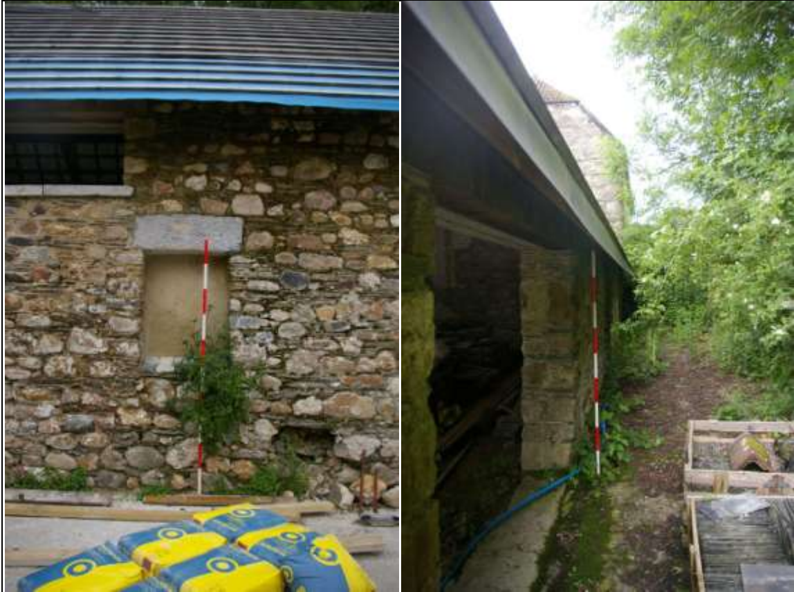
FIGURE 76: LEFT: ONE OF THE BLOCKED OPENINGS IN BARN D; FROM THE SOUTH (2M SCALE). RIGHT: THE NORTH ELEVATION OF BARN D; FROM THE EAST (2M SCALE).
