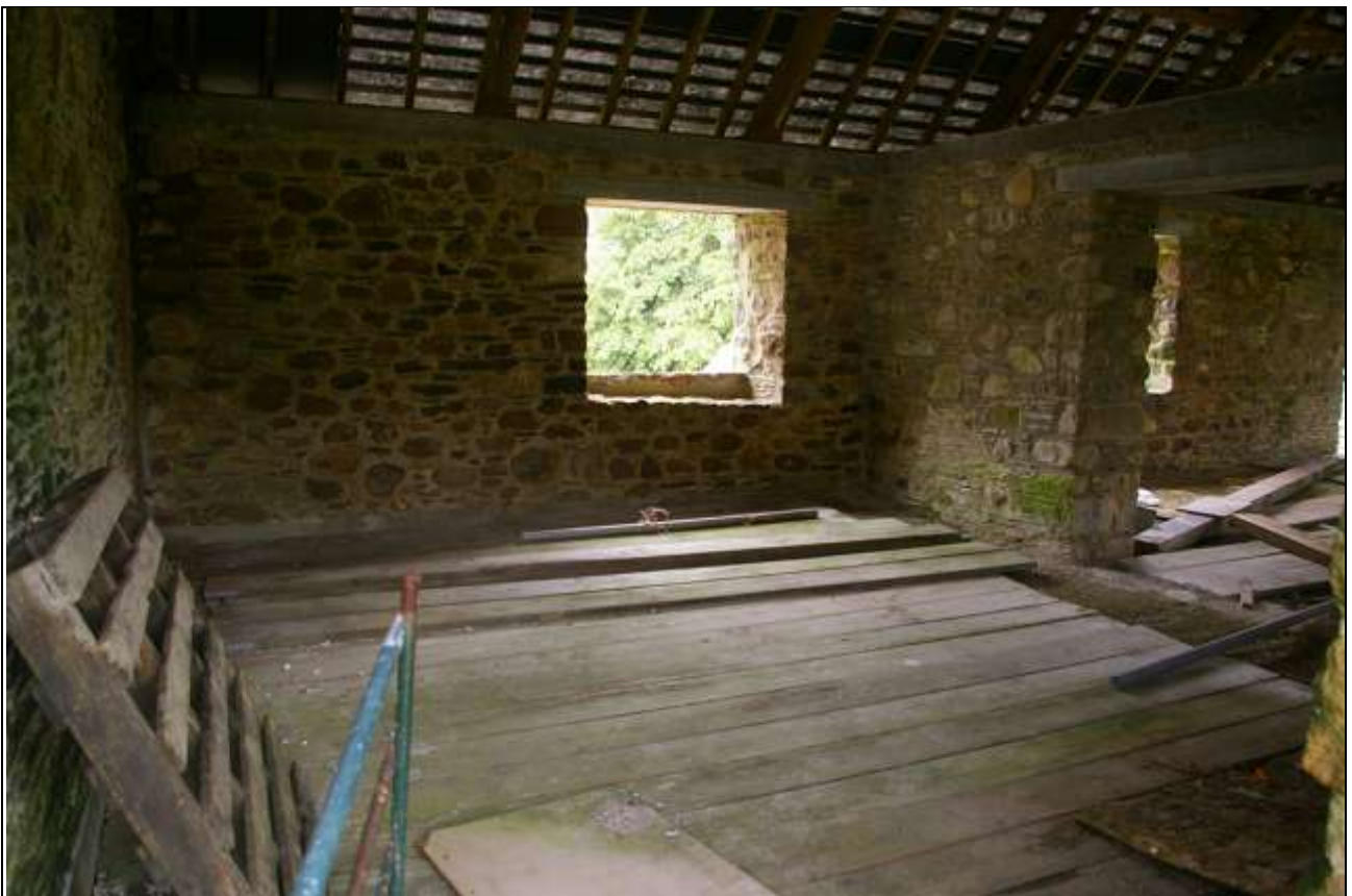
FIGURE 9: SMALL COMPARTMENT TO NORTH IN BARN A, FIRST FLOOR; FROM THE NORTH-WEST.
