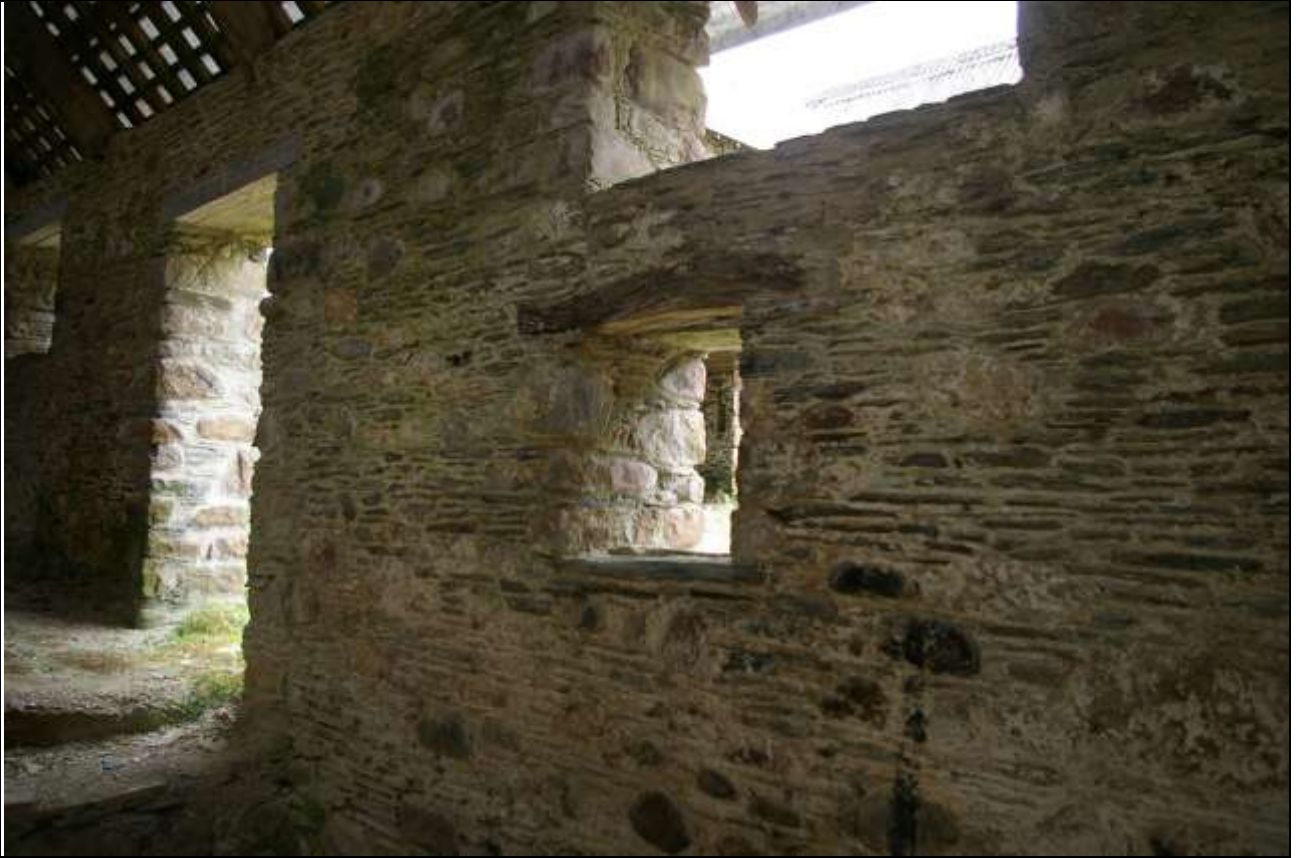
FIGURE 62: RARE SURVIVAL OF A HISTORIC LINTEL IN BARN C, TO ONE OF THE SMALL WINDOWS, TO THE EAST END OF THE NORTH WALL; FROM THE SOUTH-EAST.
