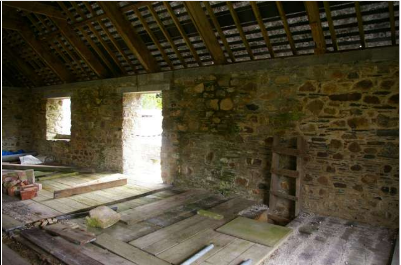
FIGURE 16: INTERIOR FACE OF THE LONG EAST WALL, AT LOFT HEIGHT, SHOWING MODERN CONCRETE RING BEAM; FROM THE SOUTH-WEST.
