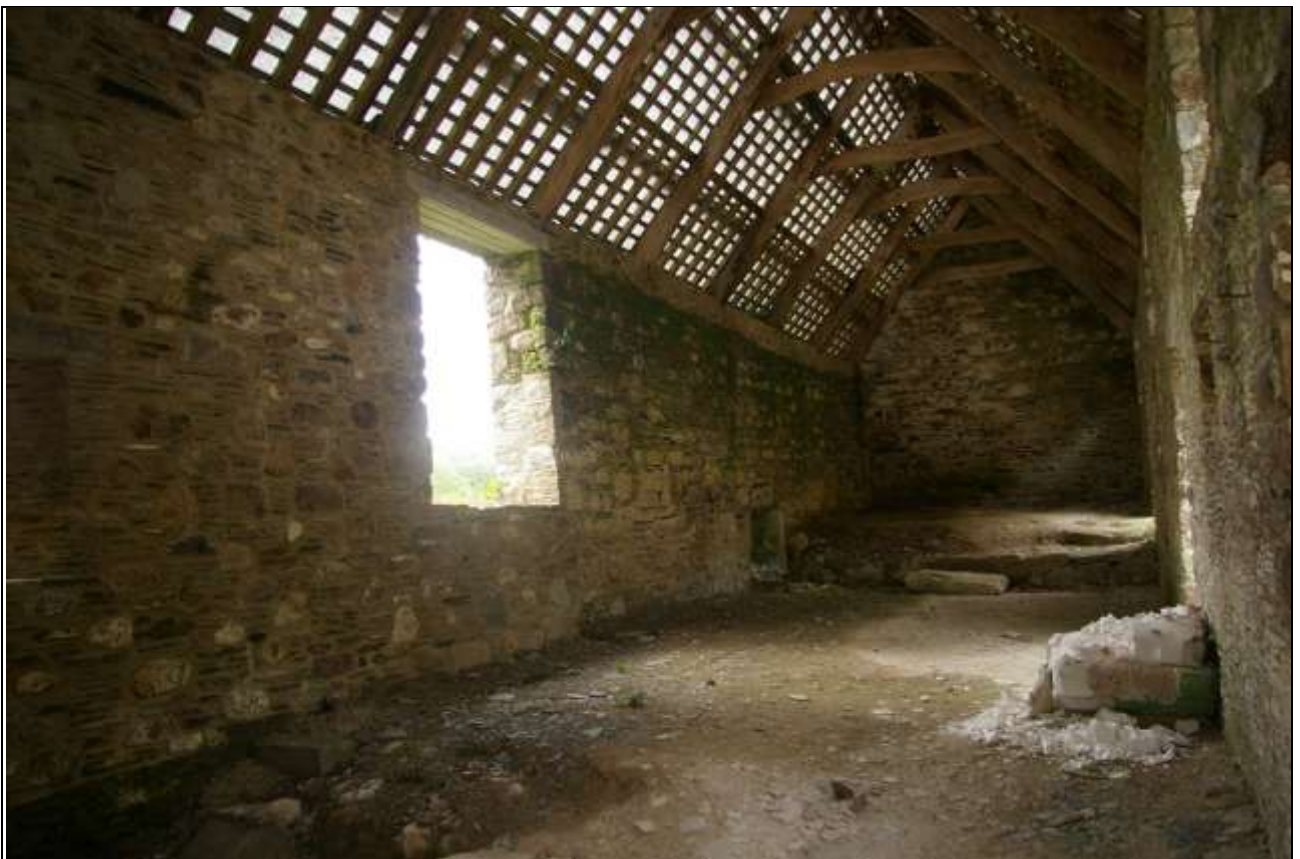
FIGURE 69: THE INTERIOR FACE OF THE SOUTH WALL, BARN C; FROM THE NORTH-EAST.
