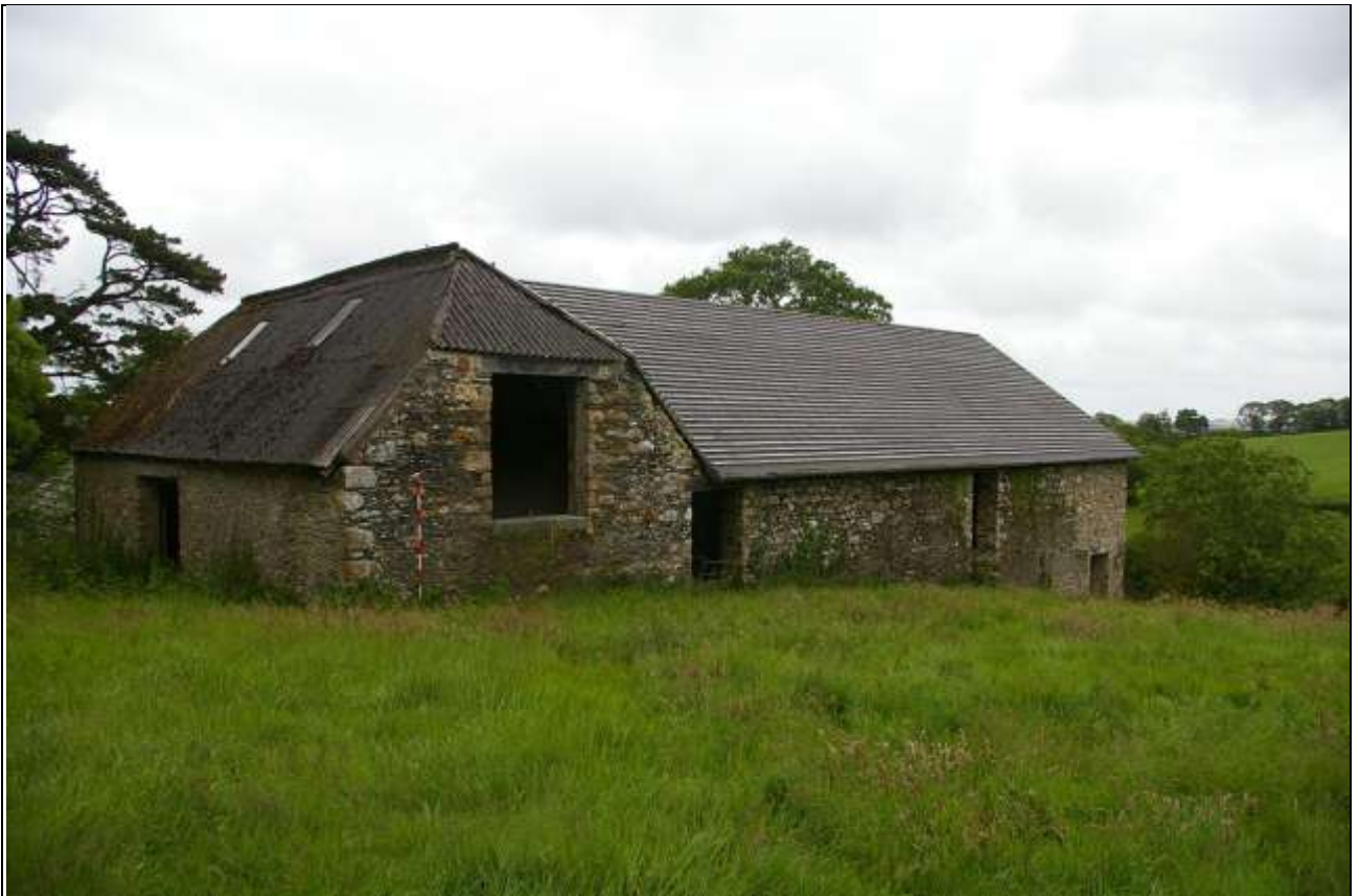
FIGURE 7: BARN B AND A, CONTIGUOUS WEST ELEVATIONS; FROM THE WEST-NORTH-WEST (2M SCALE).
