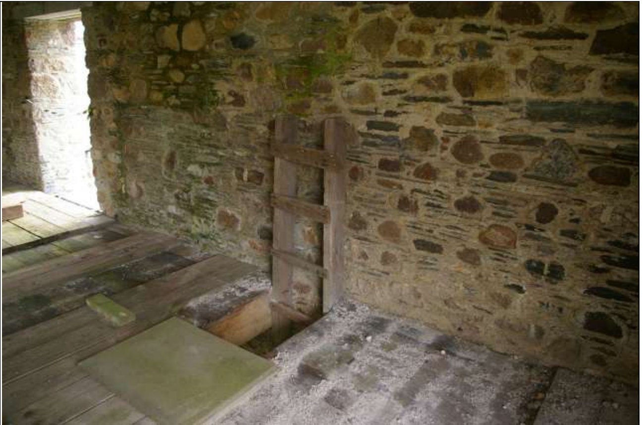
FIGURE 14: LOFT LADDER BARN A AGAINST THE EAST WALL, SOUTH END, LEADING UP FROM COW HOUSE; FROM THE SOUTH-WEST.
