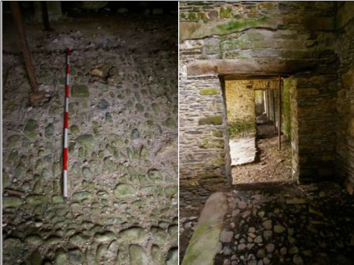
FIGURE 34: LEFT: DETAIL OF ONE OF THE DRESSED STONE PADS FOR THE PARTITION POSTS IN BARN B'S COBBLED FLOOR AND PROFILE OF DRAIN; FROM THE SOUTH (2M SCALE). RIGHT: THE DOOR LEADING THROUGH TO THE FEED CHANNEL OF BARN A, FROM BARN B; FROM THE NORTH.
