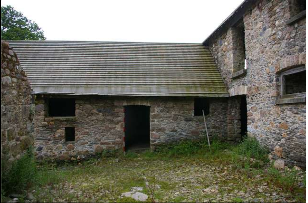
FIGURE 30: BARN C, UPPER WEST END, WHERE IT ADJOINS BARN A; FROM THE NORTH (2M SCALE).
