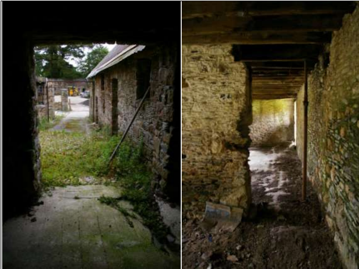
FIGURE 58: LEFT: VIEW FROM BARN A, DOWN THE SURVIVING SLOPING SECTION OF COBBLED YARD, ALONG THE NORTH WALL OF BARN C; FROM THE WEST. RIGHT: THE OPENING TO THE SOUTH COMPARTMENT, BARN A, THE FEED CHANNEL, WITH ALL FITTINGS REMOVED AND HISTORIC LINTEL REMOVED; FROM THE NORTH.
