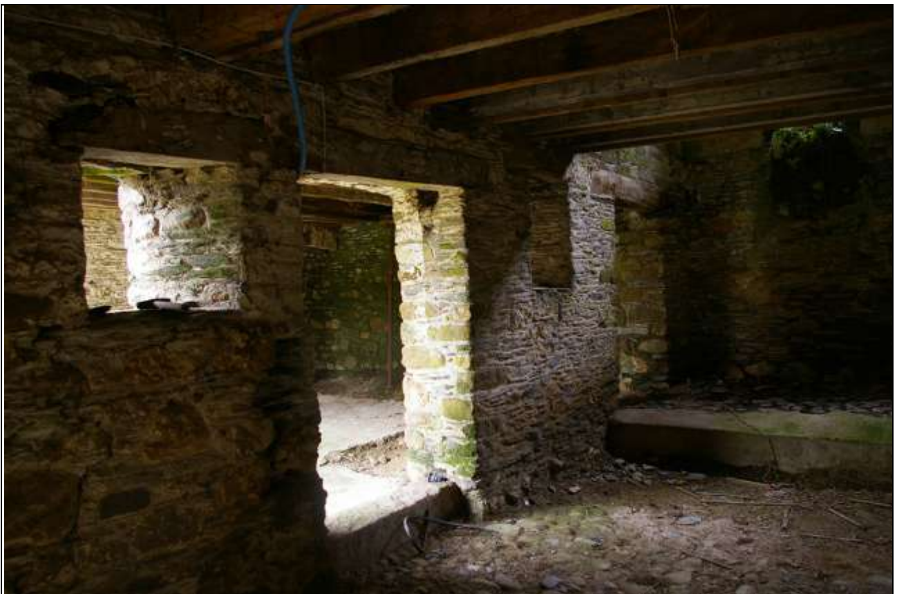
FIGURE 39: THE PAIRED DOORS AND AIR VENTS IN THE SOUTH WALL OF BARN B.
