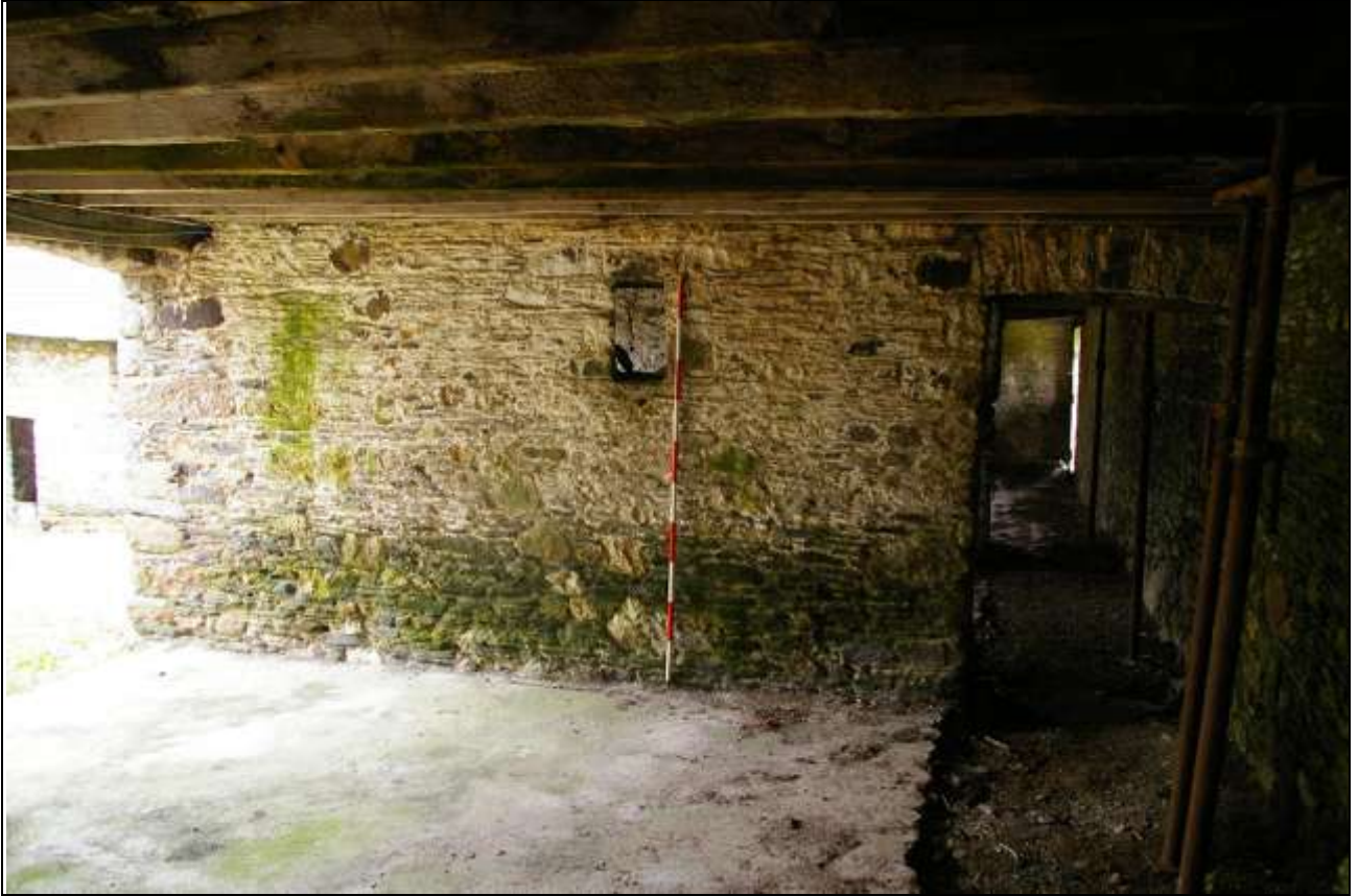
FIGURE 46: STONE PARTITION WALL TO NORTH AND CENTRAL COMPARTMENT IN BARN A; FROM THE NORTH-WEST (2M SCALE).
