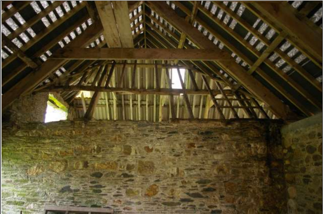
FIGURE 18: THE ARRANGEMENT OF ROOFS TO THE NORTH END, WHERE THE HISTORIC ROOF OF BARN B WAS CLEARLY SEALED AND NOT CONTIGUOUS WITH BARN A, SUGGESTIVE OF AN ORIGINAL LOWER ROOF HEIGHT FOR BARN A. THE MORE MODERN CURRENT ROOF IN BARN A AWKWARDLY ABUTS THAT OF BARN B; FROM THE SOUTH.
