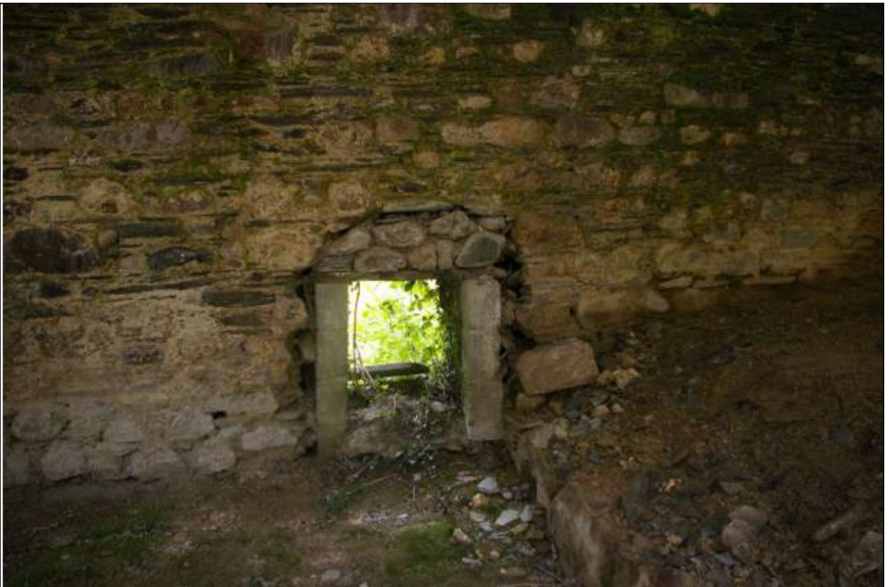
FIGURE 63: A FORCED OPENING IN THE SOUTH WALL OF BARN C, WESTERN END; FROM THE NORTH-NORTH-EAST.
