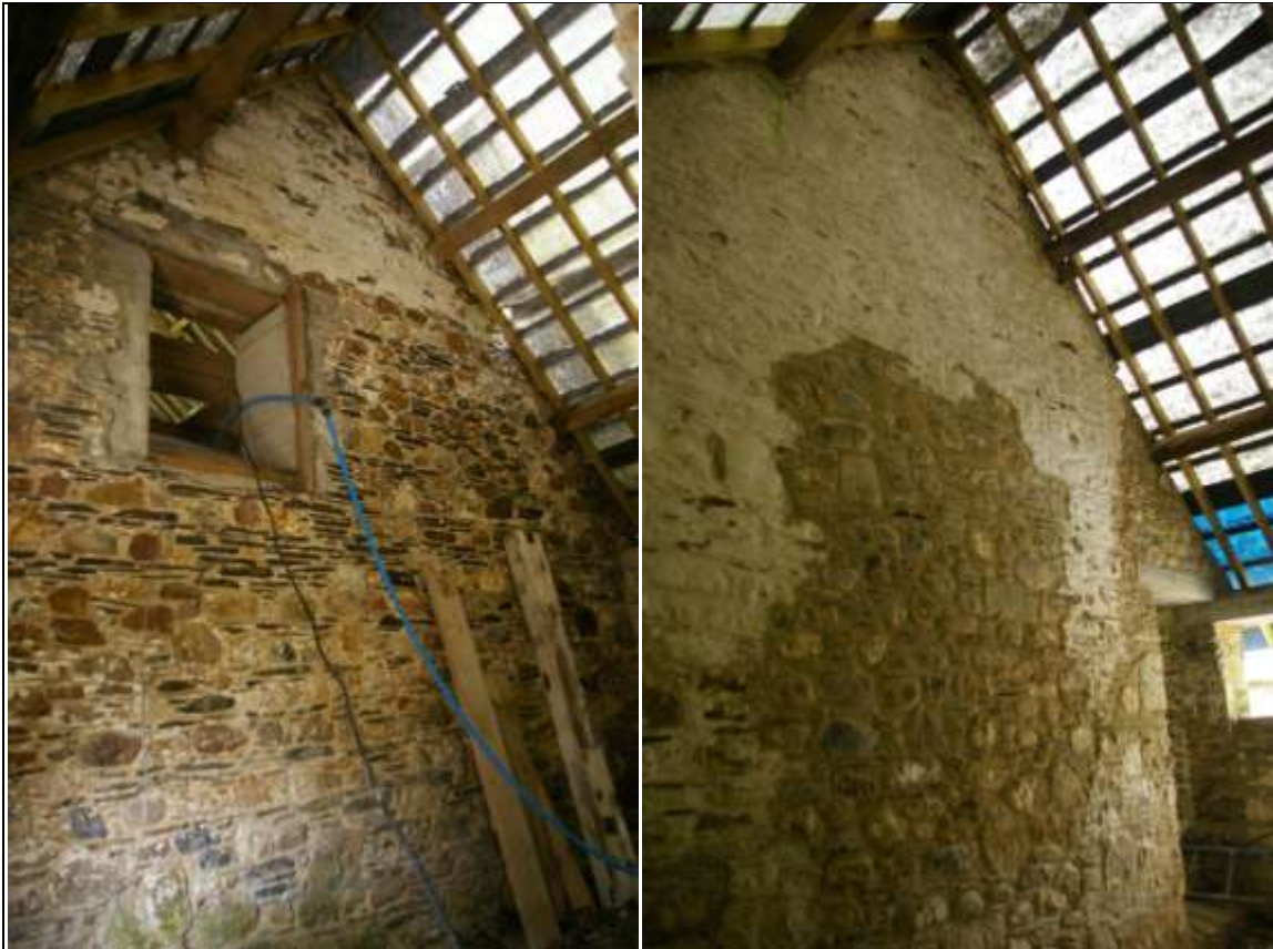
FIGURE 83: LEFT: THE FORCED OPENING IN THE WALL OF BARN D, LEADING INTO BARN D; FROM THE EAST, SOUTH-EAST. RIGHT: BARN D, COMPARTMENT PARTITION WALL TO WEST END; FROM THE NORTH-WEST.
