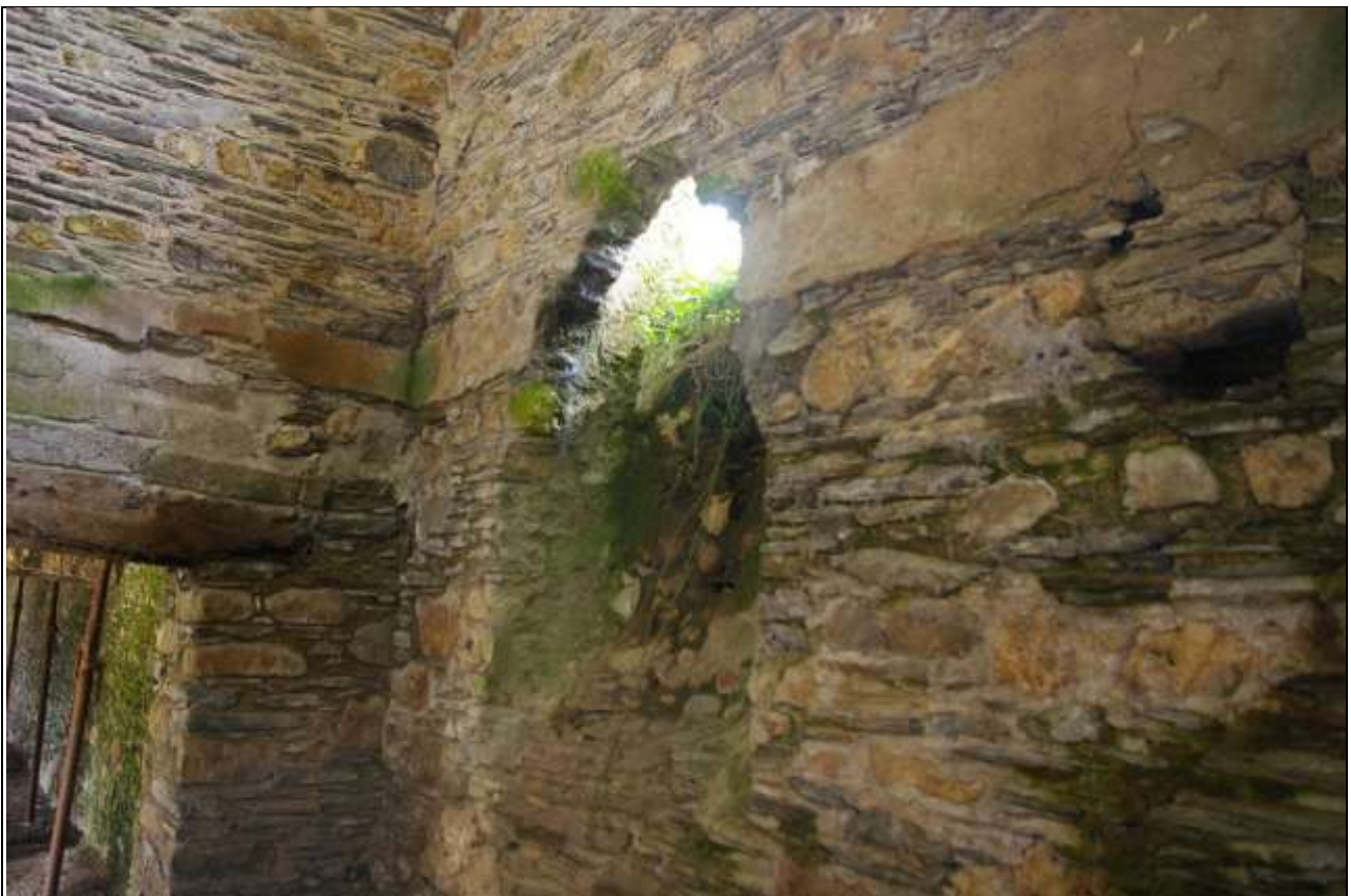
FIGURE 43: THE FORCED OPENING IN THE WEST WALL OF BARN B; FROM THE NORTH-EAST.
