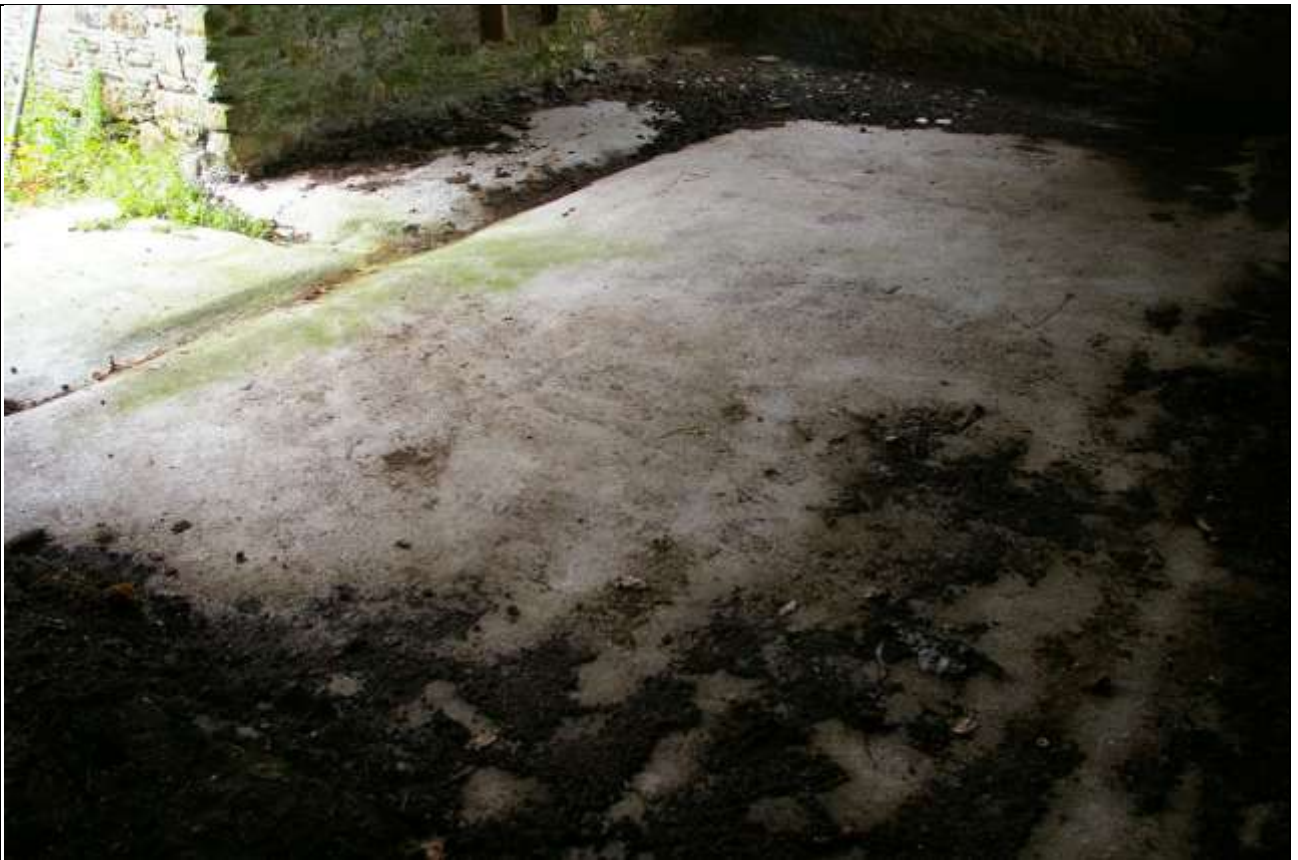
FIGURE 53: THE FLOOR IN THE LARGE SOUTH COMPARTMENT OF BARN A, COBBLES, COVERED BY A THIN LAYER OF CONCRETE, WITH DRAIN TO EAST SIDE; FROM THE NORTH-WEST.
