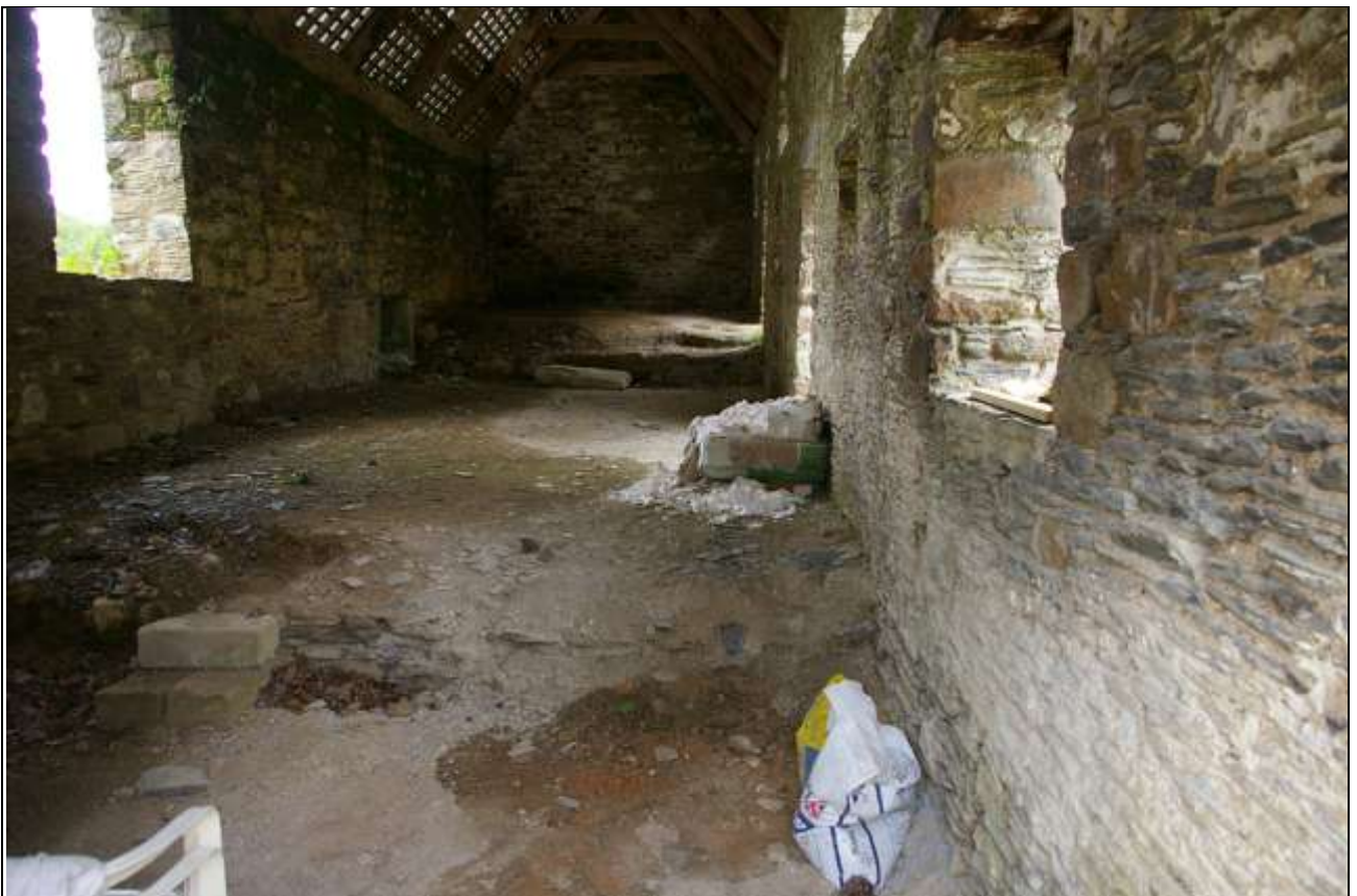
FIGURE 71: VIEW OF THE INTERIOR SPACE OF BARN C, STRIPPED OUT, AS VIEWED FROM DOOR IN EAST ELEVATION.
