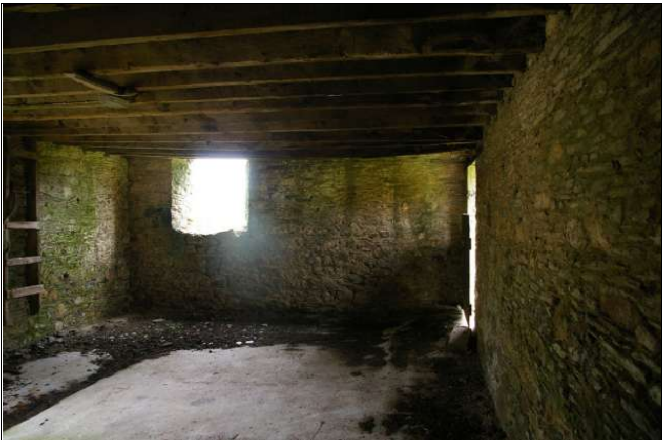
FIGURE 55: THE INTERIOR FACE OF THE SOUTH WALL, BARN A; FROM THE NORTH-WEST.
