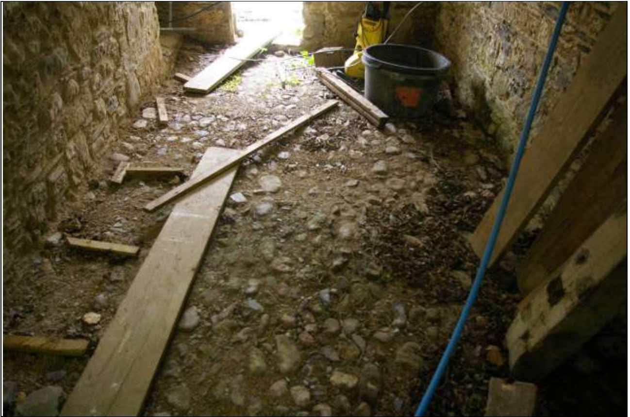
FIGURE 84: THE ROUGHER COBBLED FLOOR IN BARN D, COMPARTMENT AGAINST BARN B; FROM THE NORTH.
