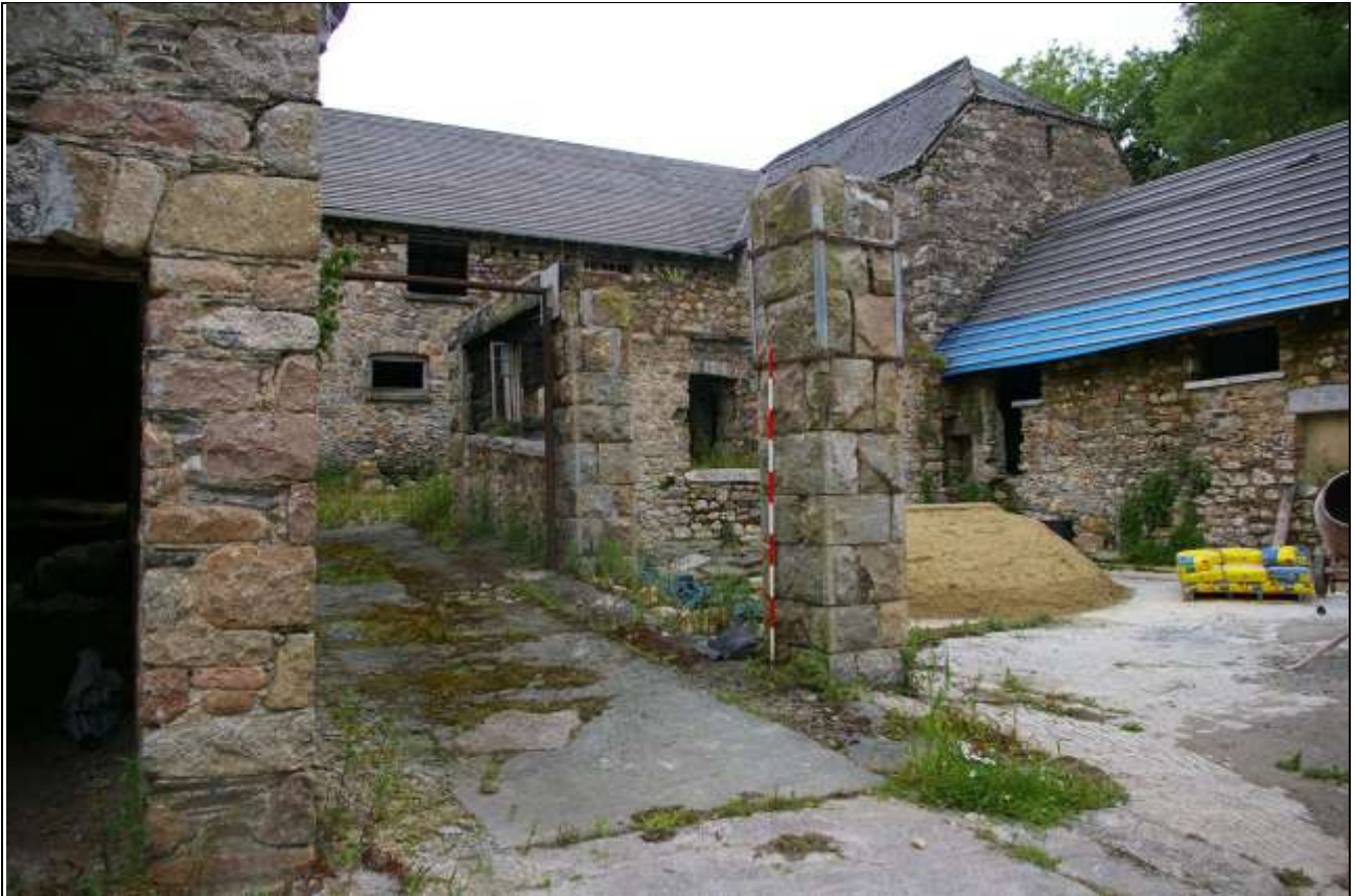
FIGURE 74: THE WESTERN END OF BARN E, MORE SUBSTANTIAL THAN THE REST, WITH SURVIVING BOARDING AND ONE STONE WALL; FROM THE SOUTH-EAST (2M SCALE).
