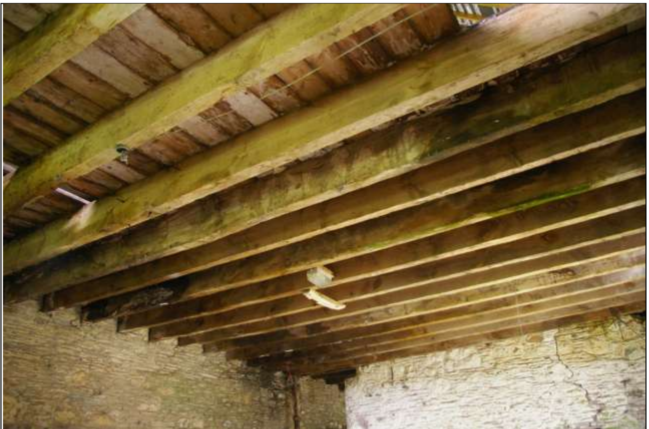
FIGURE 57: THE LOFT FLOOR IN THE SOUTH END OF BARN A; FROM THE SOUTH-EAST.
