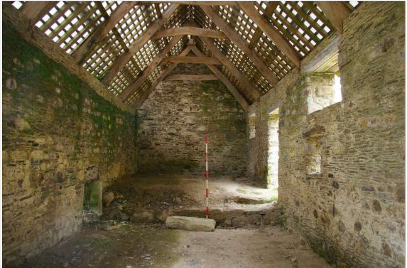
FIGURE 61: THE UPPER LEVEL IN BARN C, WITH LOW SECTION OF SURVIVING RETAINING/PARTITION WALL; FROM THE EAST (2M SCALE).
