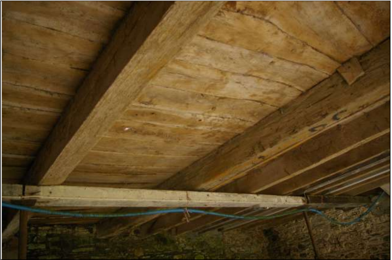
FIGURE 40: VIEW OF THE HEAVY JOISTS AND PEGGED LINES OF BRACING IN THE LOFT FLOOR IN BARN B, WHERE THE SECONDARY THRESHING FLOOR IS ATTACHED.
