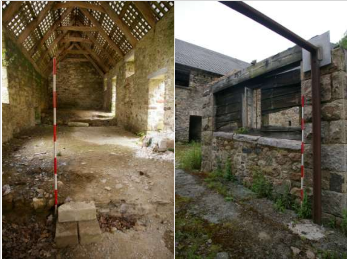
FIGURE 66: LEFT: THE INTERIOR OF BARN C FROM THE EAST (2M SCALE). RIGHT: VIEW OF THE WEST WALL OF BARN E, FROM WITHIN THE COBBLED YARD; FROM THE SOUTH-WEST (2M SCALE).
