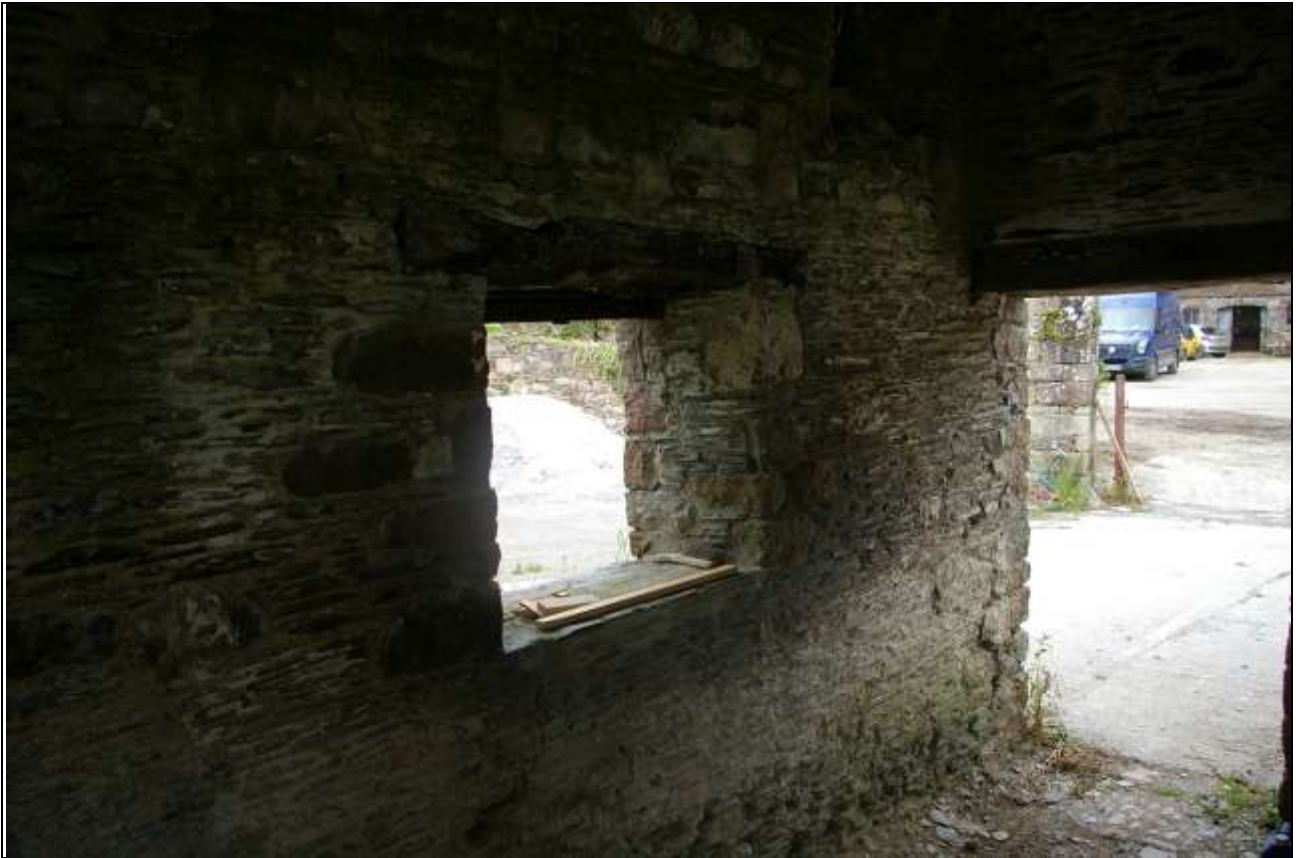
FIGURE 65: WIDER ANGLE SHOWING WINDOW AND DOOR TO THE NORTH-EAST CORNER OF BARN C; FROM THE SOUTH-WEST
