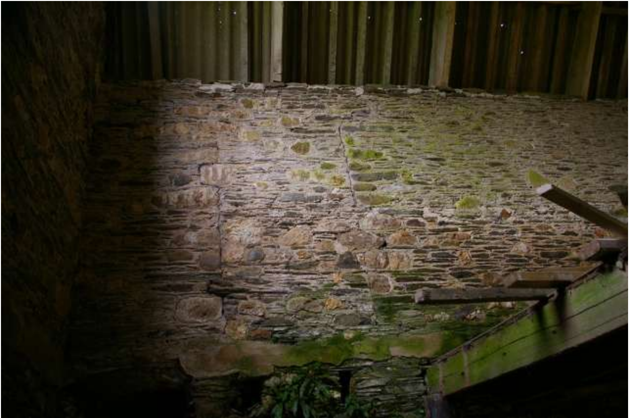
FIGURE 42: THE FIRST FLOOR BLOCKED DOORWAY IN THE NORTH WALL OF BARN B; FROM THE SOUTH.
