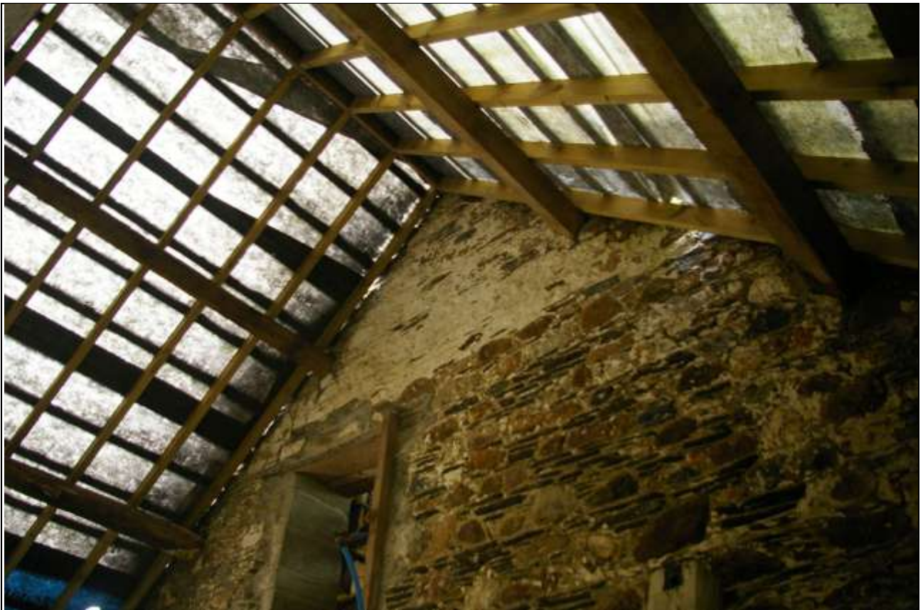
FIGURE 85: SIMPLE PURLINS TO THE WEST OF BARN D, AS IT ABUTS BARN B, POSSIBLY A REPLACEMENT ROOF; FROM THE NORTH-EAST.
