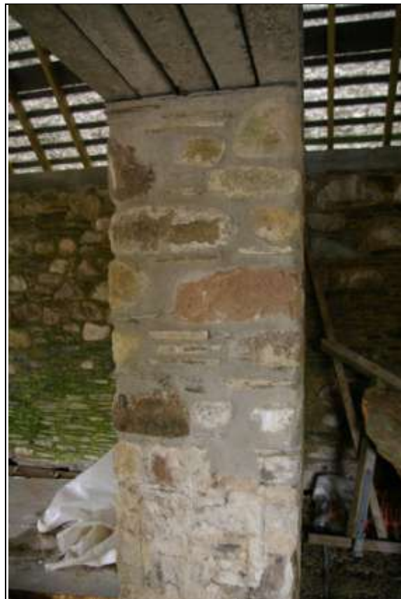
FIGURE 19: THE HEAVY PARTITION WALL IN BARN A, WITH CONCRETE LINTELS INSERTED; FROM THE EAST.
