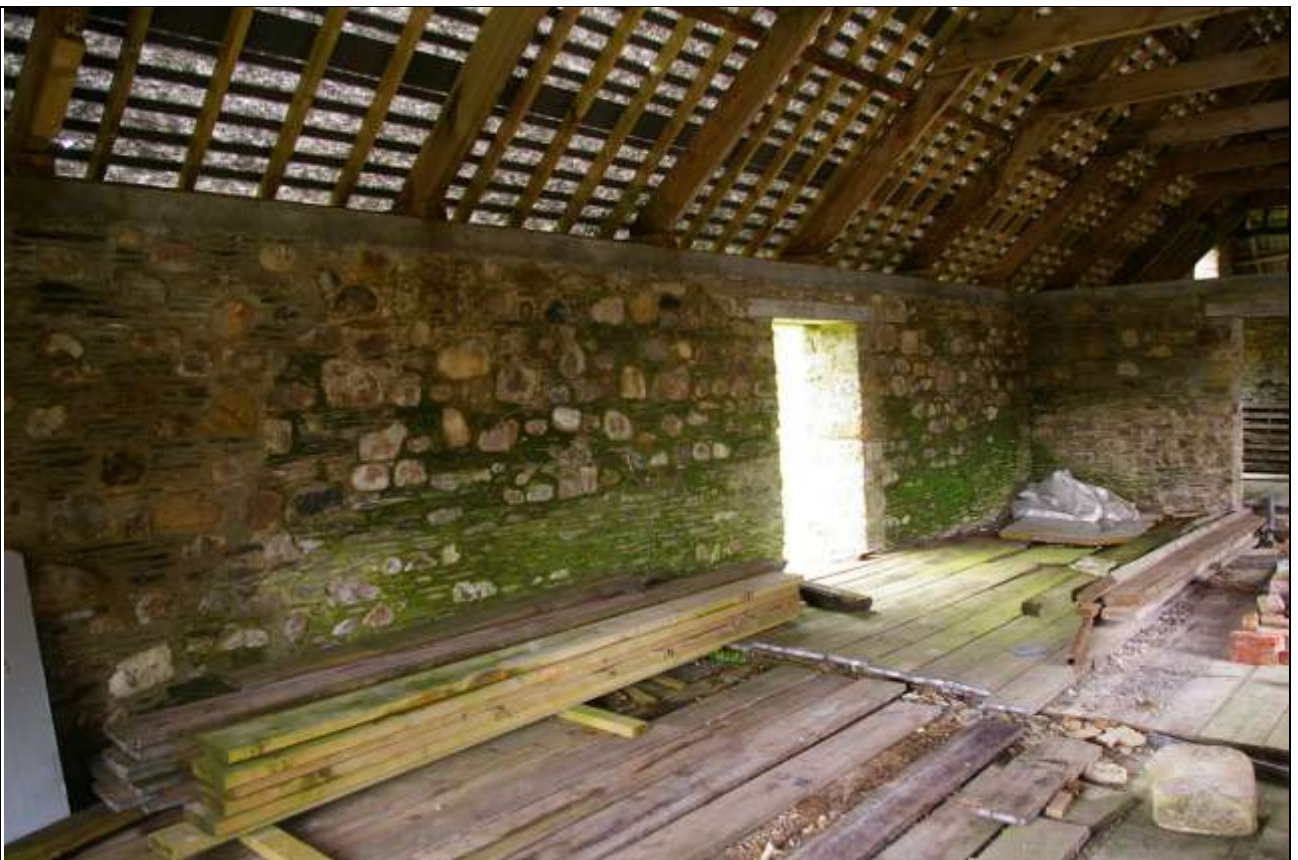
FIGURE 15: INTERIOR FACE OF LONG WEST WALL, AT LOFT HEIGHT, SHOWING MODERN CONCRETE RING BEAM; FROM THE SOUTH-EAST.
