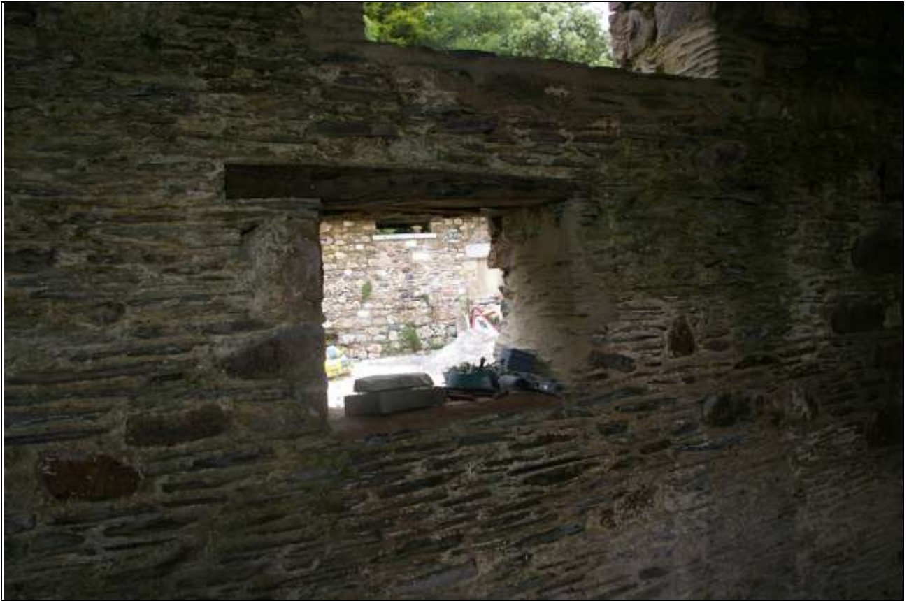
FIGURE 64: THE LARGER WINDOW TO THE EAST IN THE NORTH WALL OF BARN C, WITH SURVIVING HISTORIC TIMBER LINTEL AND PART OF A WINDOW FRAME; FROM THE SOUTH-SOUTH-WEST.
