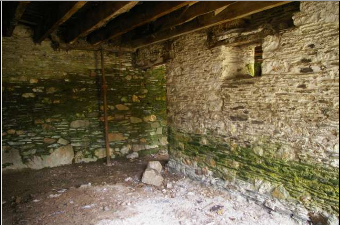
FIGURE 50: PARTITION WALL BETWEEN THE CENTRAL AND NORTH COMPARTMENTS IN BARN A, SHOWING AIR VENT AND OPENING FOR FEED CHANNEL.
