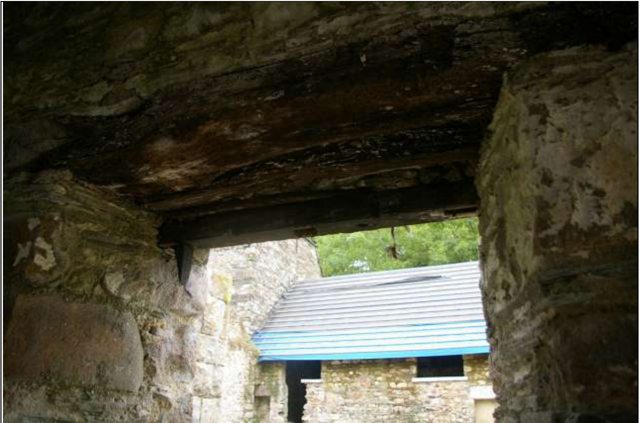
FIGURE 70: DETAIL OF SURVIVING LINTEL AND WINDOW FRAME WITH BROKEN TIMBER SQUARE GLAZING BAR; FROM THE SOUTH-EAST.
