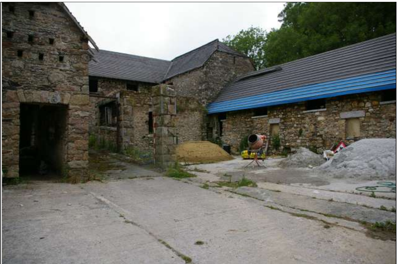
FIGURE 73: BARN E, THE OPEN-SIDED STRUCTURE SUPPORTED ON HEAVY LIMESTONE BLOCK PIERS; FROM THE SOUTH-EAST (2M SCALE).
