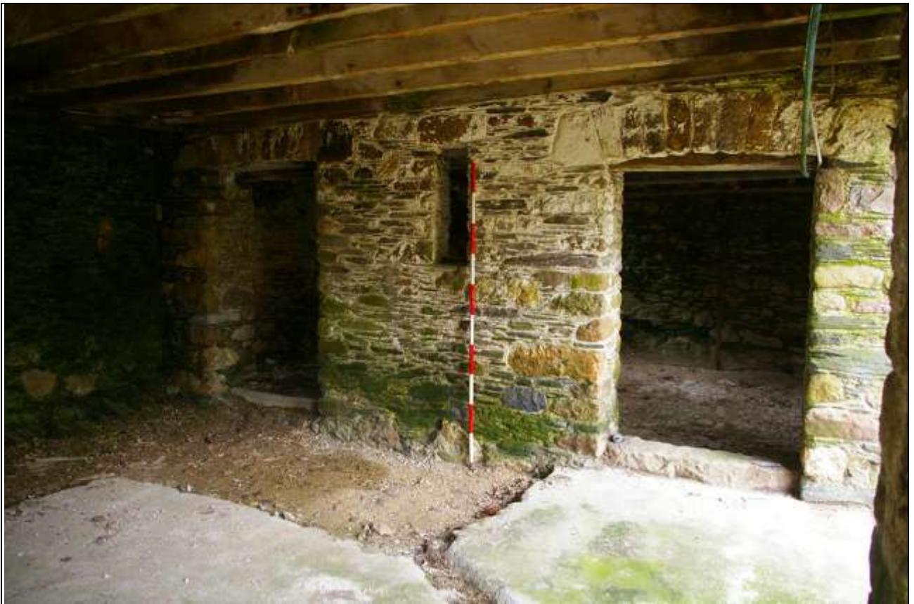
FIGURE 47: SOUTH WALL OF BARN B, WITHIN NORTH COMPARTMENT OF BARN A; FROM THE SOUTH-EAST (2M SCALE).
