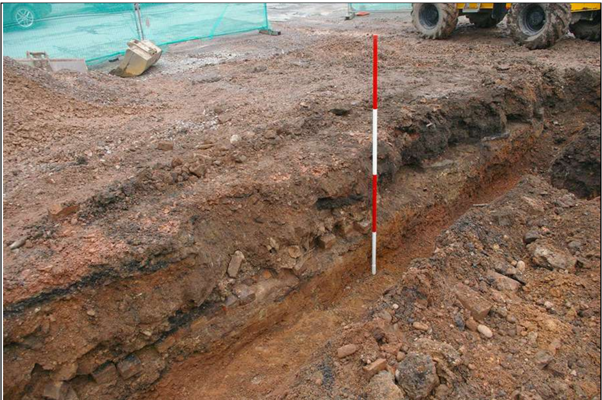
HOUSE PLOT 2, SOUTH-WEST FACING SECTION OF NORTH-WEST FOUNDATION TRENCH, OBLIQUE, SHOWING FLOOR SURFACES (155) AND (167); VIEWED FROM THE WEST (2M SCALE).
