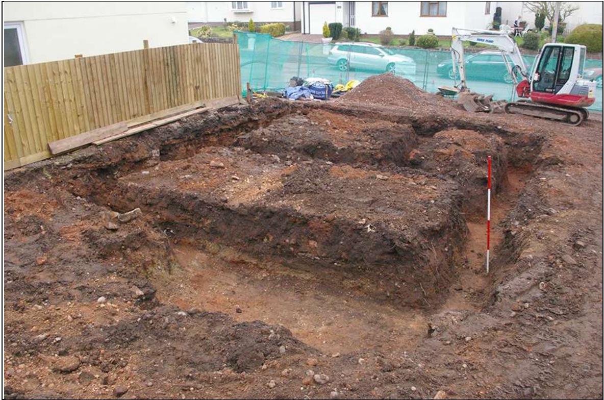
HOUSE PLOT 2, SITE SHOT SHOWING FOUNDATION TRENCHES AND SOIL LAYER (163); VIEWED FROM THE SOUTH (2M SCALE).
