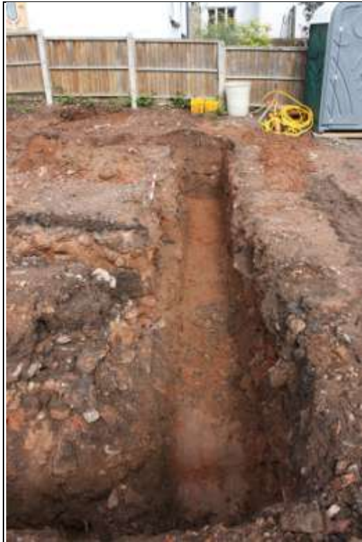
HOUSE PLOT 1, VIEW ALONG NORTH-EAST FOUNDATION TRENCH SHOWING WALL {137} WITH FLOOR (138); VIEWED FROM THE SOUTH-EAST (1M SCALE).
