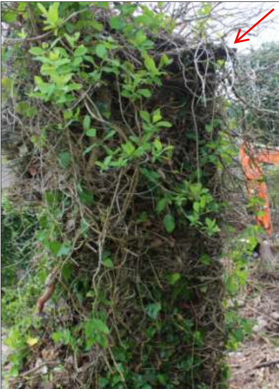
B2: the north-east corner of B2 at first-floor level, with cast-iron guttering indicated; viewed from the east (scale 2m).
