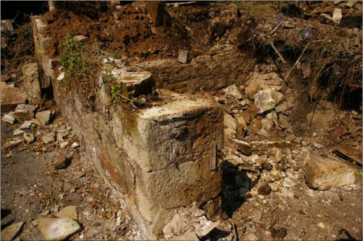
B4: the south-west corner of B4 after the removal of the rubble infill but before demolition; viewed from the south-east.
