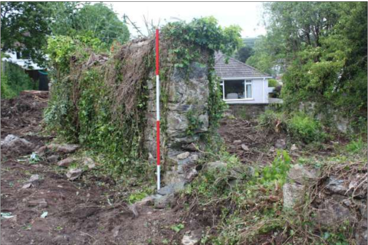
B1: as above, the southern end that formerly abutted the corner of B2; viewed from the south (scale 2m).
