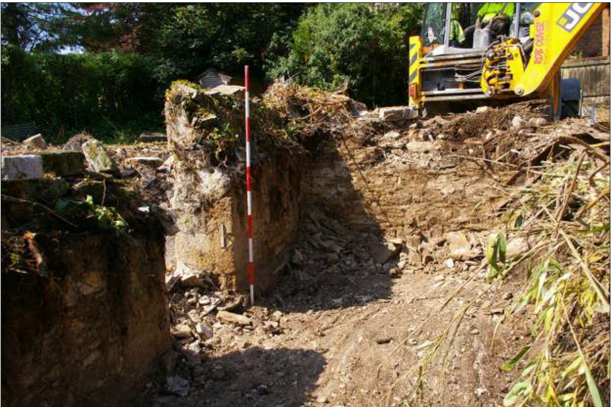
B4: the interior of B4 after the removal of the rubble infill, showing the western doorway in the south wall and the concrete floor; viewed from the east (scale 2m).
