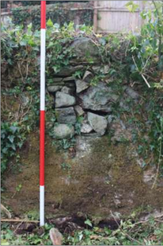
B2: the blocked ventilation slit in the west wall; viewed from the east (scale 2m).
