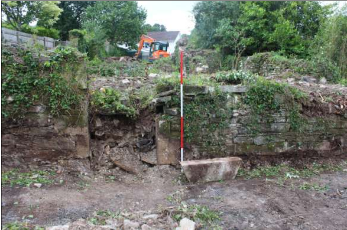
FIGURE 10: THE WESTERN DOORWAY [19] IN THE SOUTH WALL OF B4, WITH SHAPED LINTEL; VIEWED FROM THE SOUTH (SCALE 2M).
