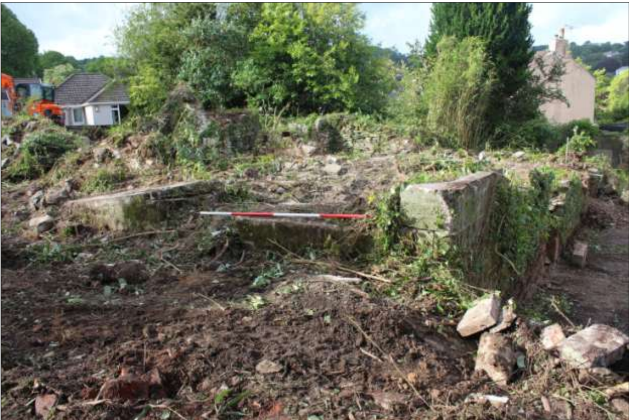
B4: the remains of the concrete ramp and platform to the west of B4; viewed from the west (scale 2m).
