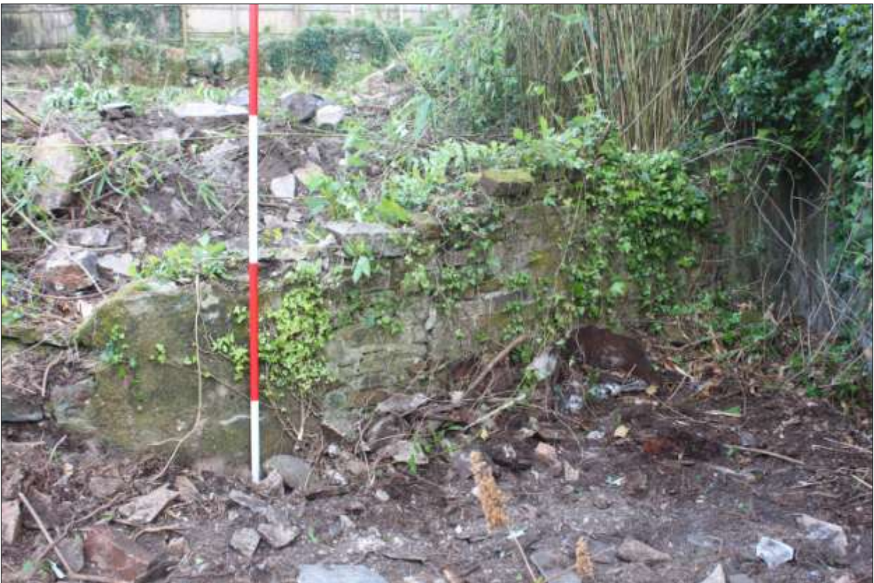
B5: the east wall of B5; viewed from the south-east (scale 2m).
