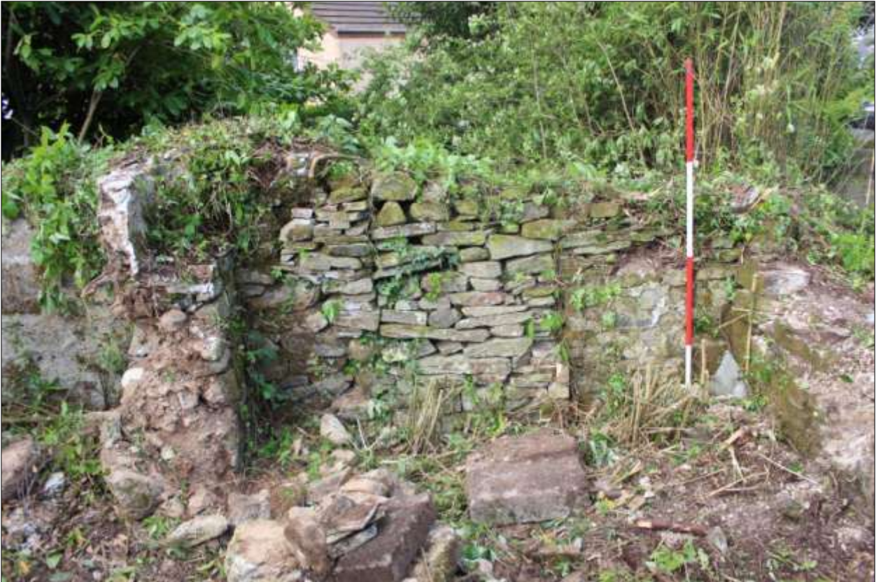
B3: the east wall of B3; viewed from the west (scale 2m).
