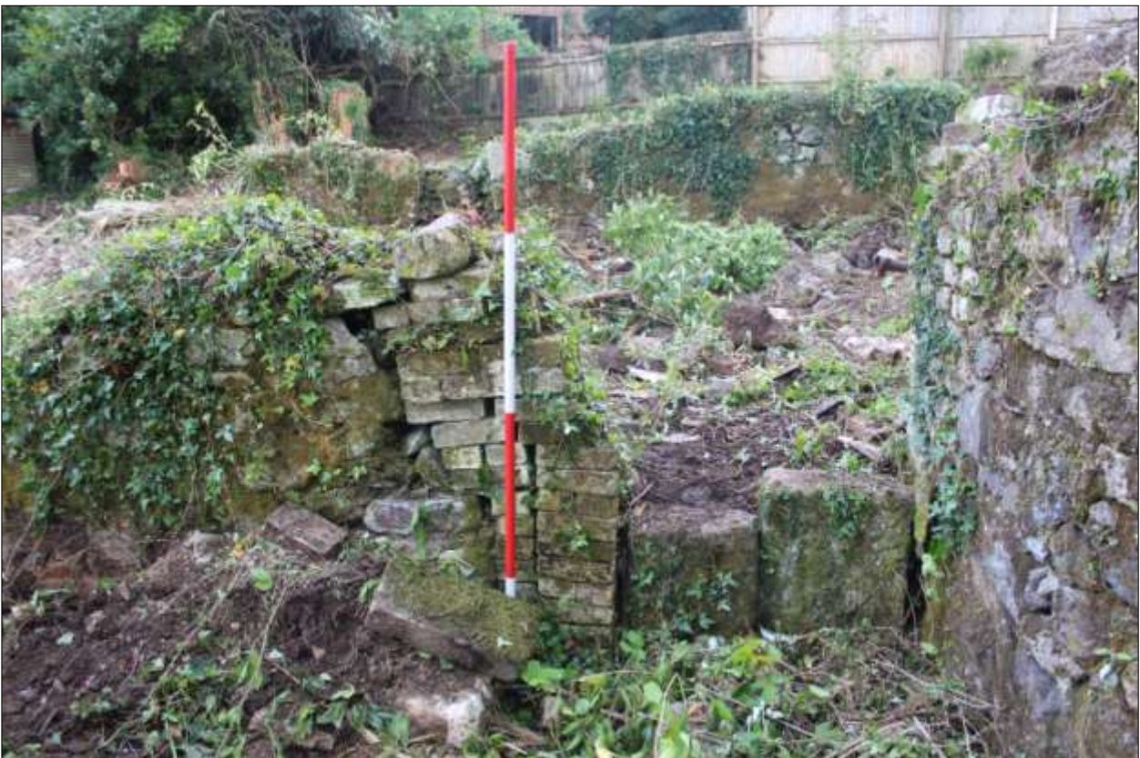
B2: the brick reveal to the north door in the east wall, and blocking with granite slabs; viewed from the east (scale 2m).
