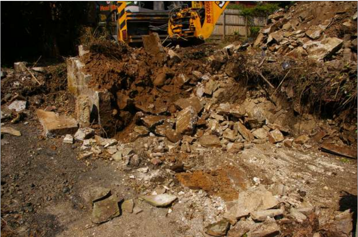
B4: as above, showing the lack of foundations; viewed from the south-east.
