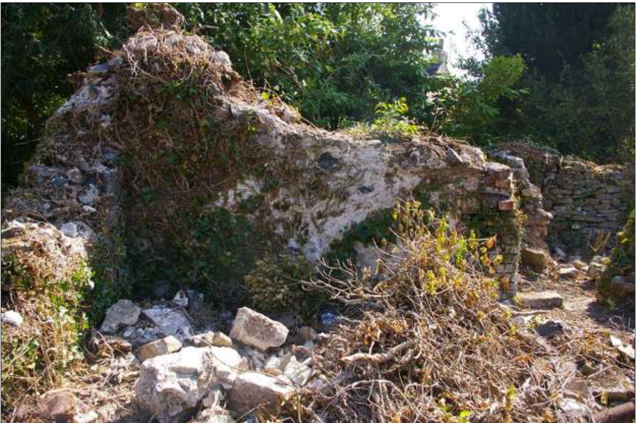
B2: the north-east angle of B2 showing the inner face plastered and whitewashed; viewed from the west.
