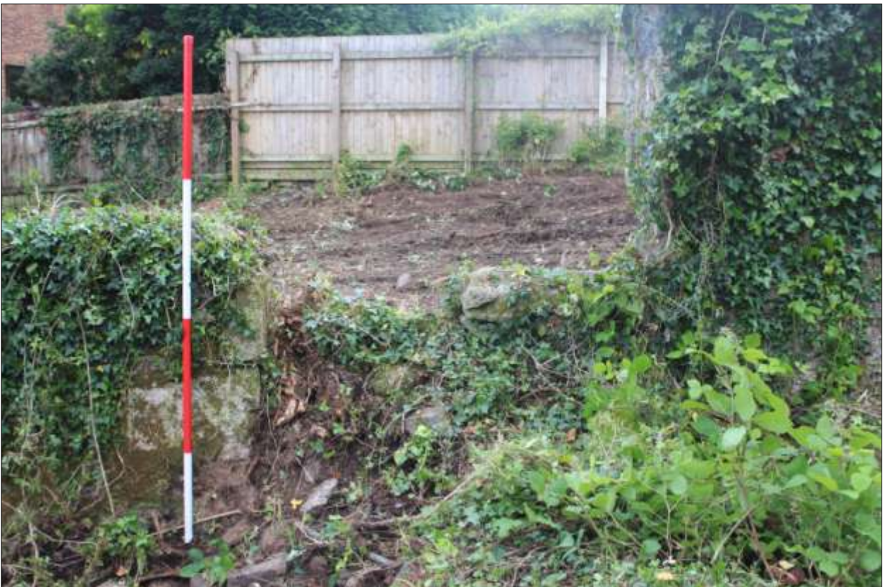
B2: partly-blocked opening (window?) at the northern end of the west wall; viewed from the east (scale 2m).
