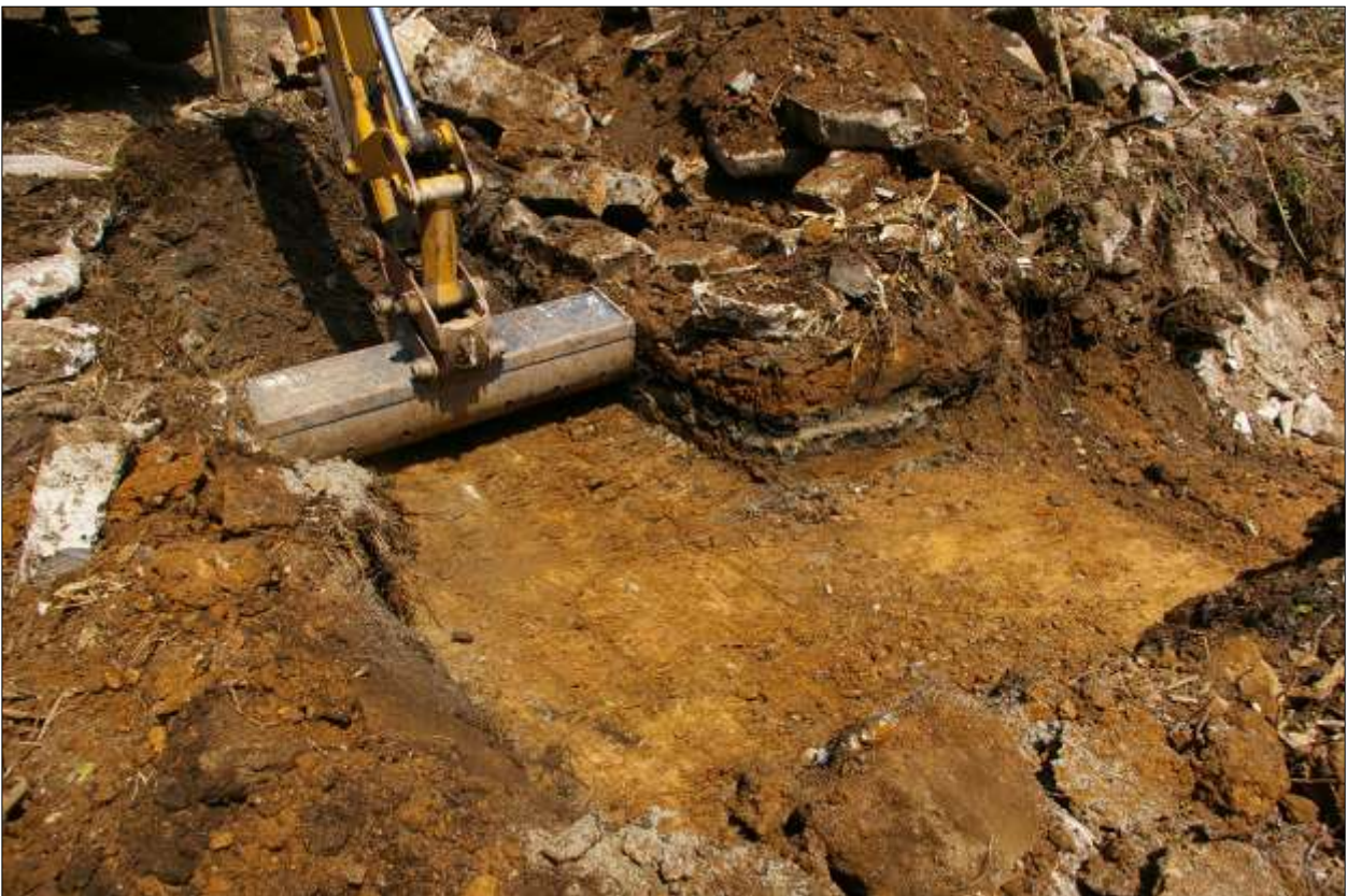
Area B: the dogleg foundation trench to the west of B4; viewed from the south.
