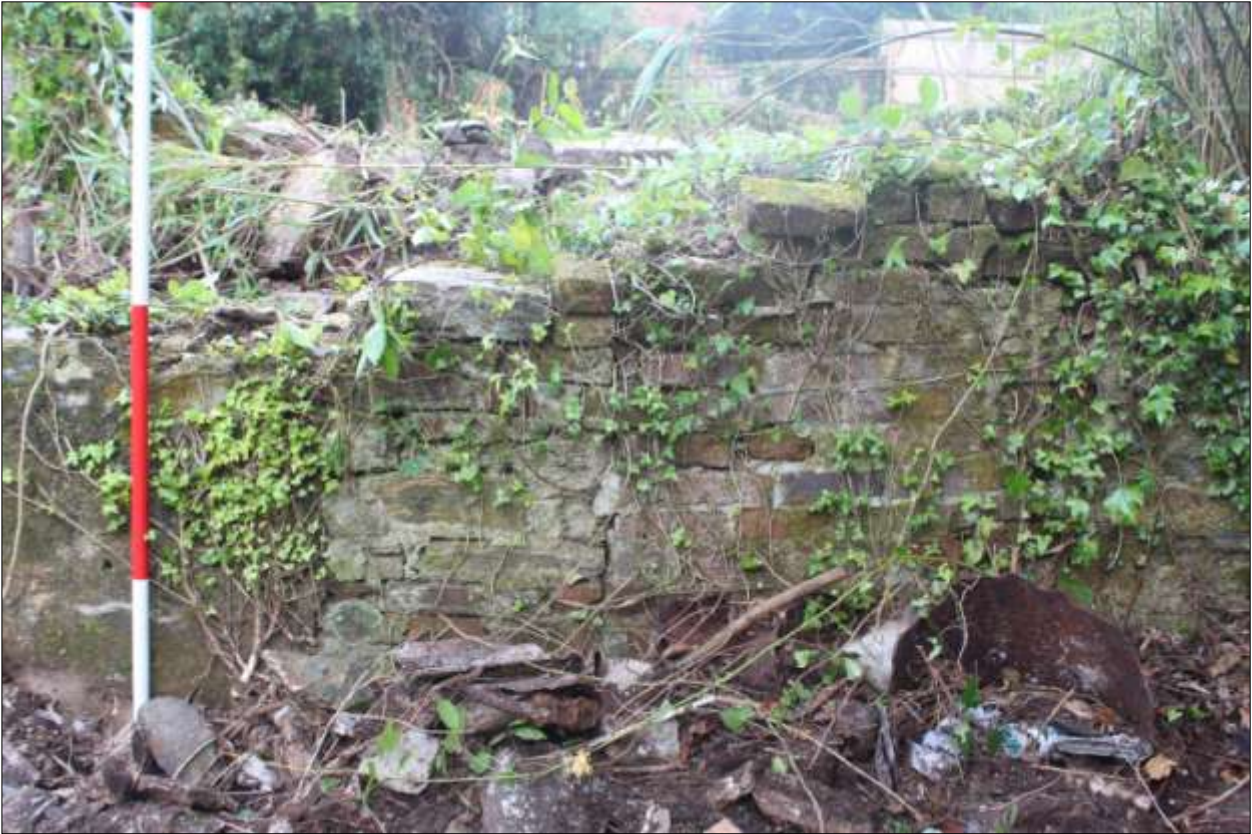
B5: as above, detail of the brick and stone blocking; viewed from the east (scale 2m).
