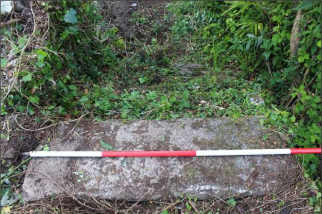
B2: the top granite tread of the steps; viewed from the south (scale 2m).
