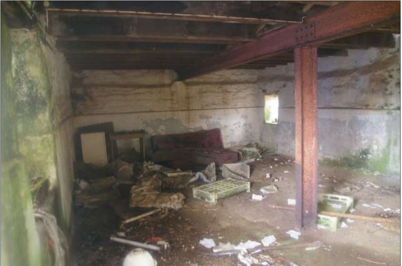
B2.2, NORTHERN GF ROOM, SHOWING THE REMAINS OF HEAVIER WALLS, SLIGHTLY BATTERED TO THE BASE; VIEWED FROM THE SOUTH-WEST.
