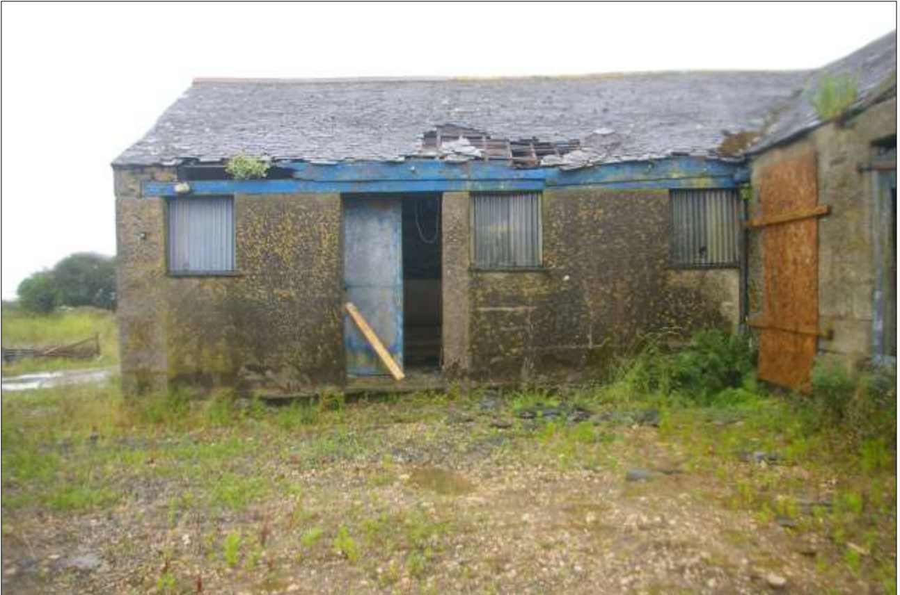
B5, NORTH-EAST ELEVATION, WITH CENTRAL GRANITE PILLAR AND OPENINGS INFILLED IN CONCRETE BLOCK (BO10, BO11); VIEWED FROM THE NORTH-EAST.
