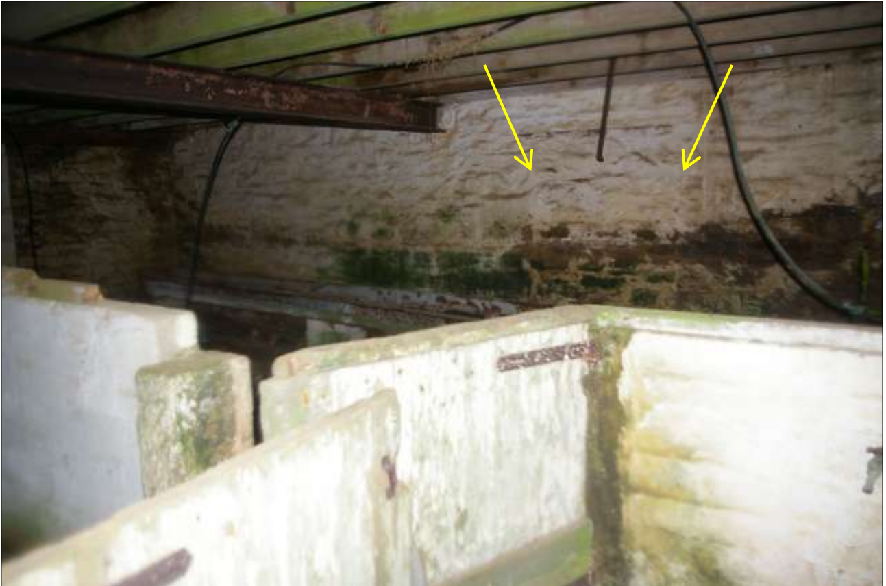
B1.2, WESTERN GF ROOM, SHOWING THE BLOCKED DOORWAY (BO3) (INDICATED); VIEWED FROM THE EAST-NORTH-EAST.
