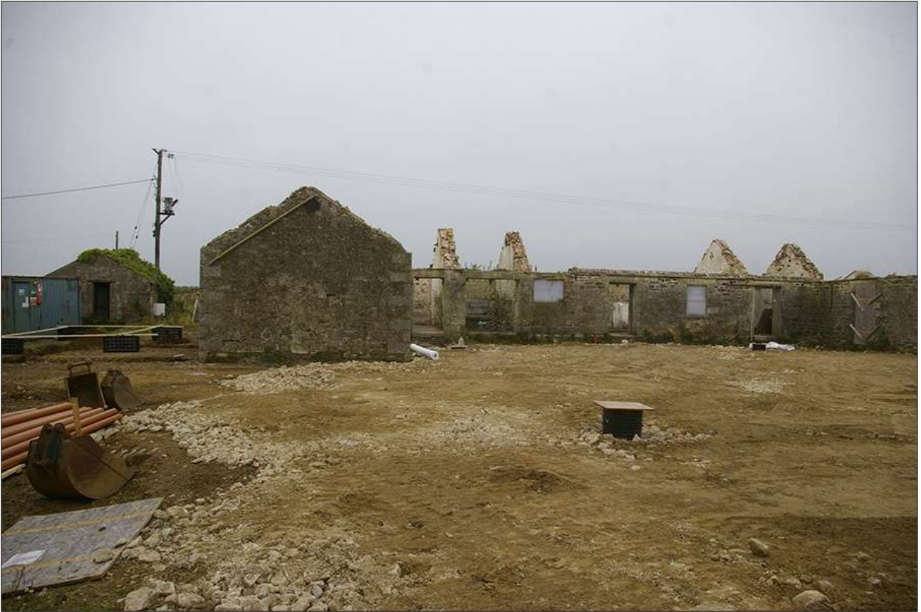
B4 AND B5, SOUTH-EAST ELEVATIONS AND CENTRAL YARD AREA, DURING WORKS; VIEWED FROM THE SOUTH-EAST.
