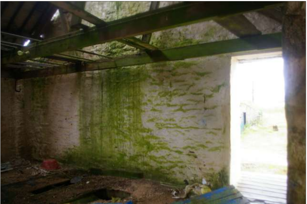
B1.3, FF ROOM, SHOWING THE NORTH-WEST GABLE AND FORCED DOORWAY (D5); VIEWED FROM THE EAST.
