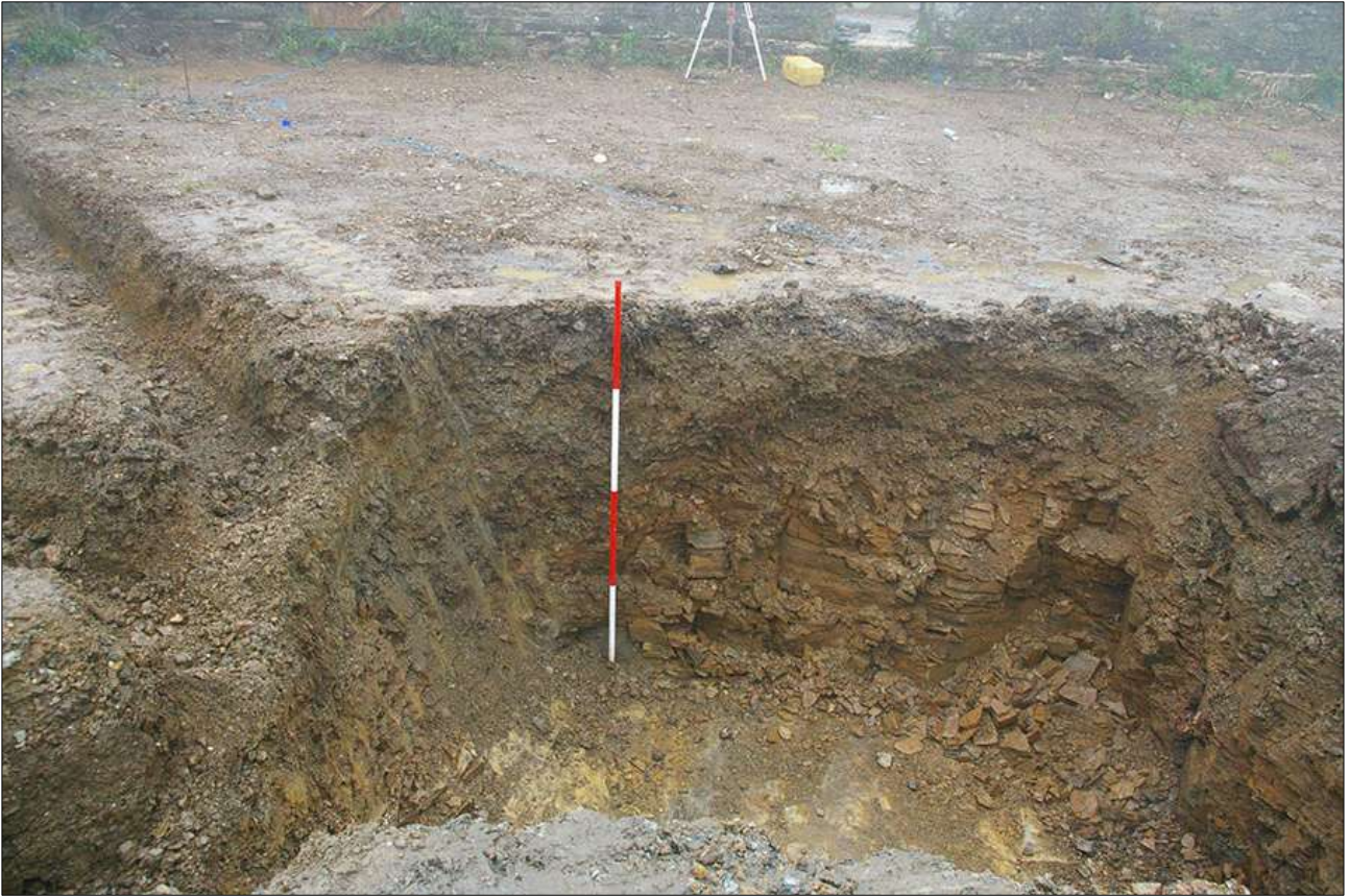
SOAKAWAY NO.1 IN SOUTH-WEST CORNER OF THE YARD; VIEWED FROM THE SOUTH-WEST (SCALE 2M).
