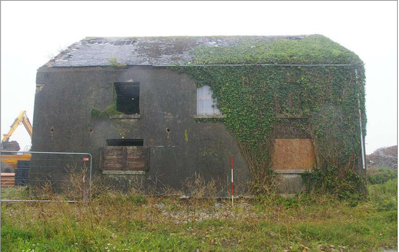
B1, SOUTH-WEST ELEVATION; VIEWED FROM THE SOUTH-WEST (SCALE 2M). BO2 VISIBLE JUST TO THE LEFT OF THE RANGING POLE.
