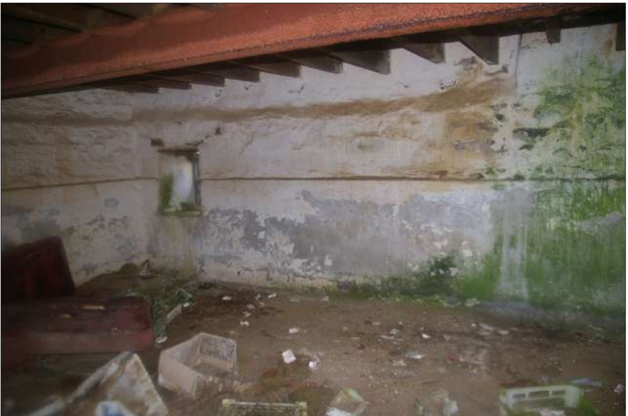
B2.2, NORTHERN GF ROOM, THE NORTH-EAST CORNER OF THE ROOM WITH SMALL FORCED WINDOW (W8); VIEWED FROM THE SOUTH-WEST.
