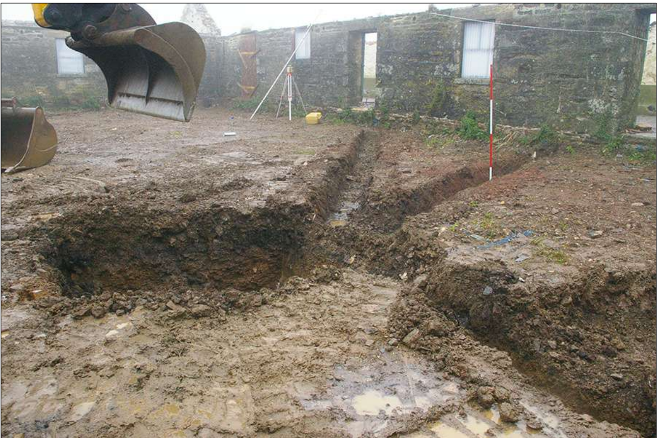
SOAKAWAY NO.2 AND TRENCHES IN THE NORTH-EAST CORNER OF THE YARD; VIEWED FROM THE WEST (SCALE 2M).
