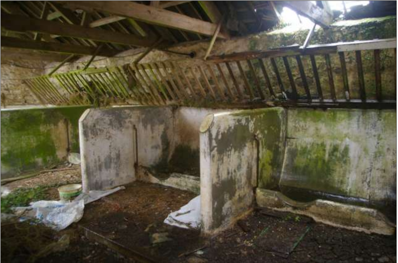
B4.2, SOUTH ROOM, THE CONCRETE STALLS AND TIMBER HAYRACKS; VIEWED FROM THE NORTH-EAST.
