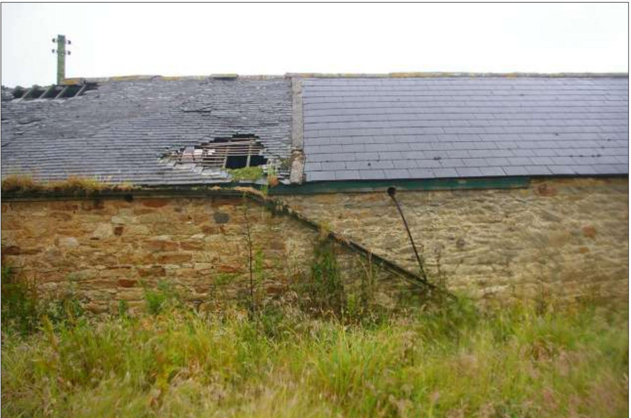
B4 (LEFT) AND B5 (RIGHT), SHOWING THE STONEMWORK; VIEWED FROM THE WEST-NORTH-WEST.
