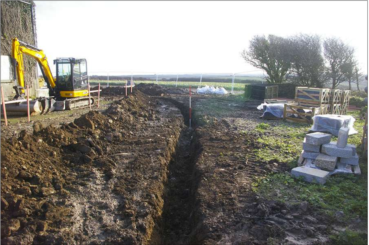
WATER PIPE BESIDE B1; VIEWED FROM THE NORTH-WEST (SCALE 2M).
