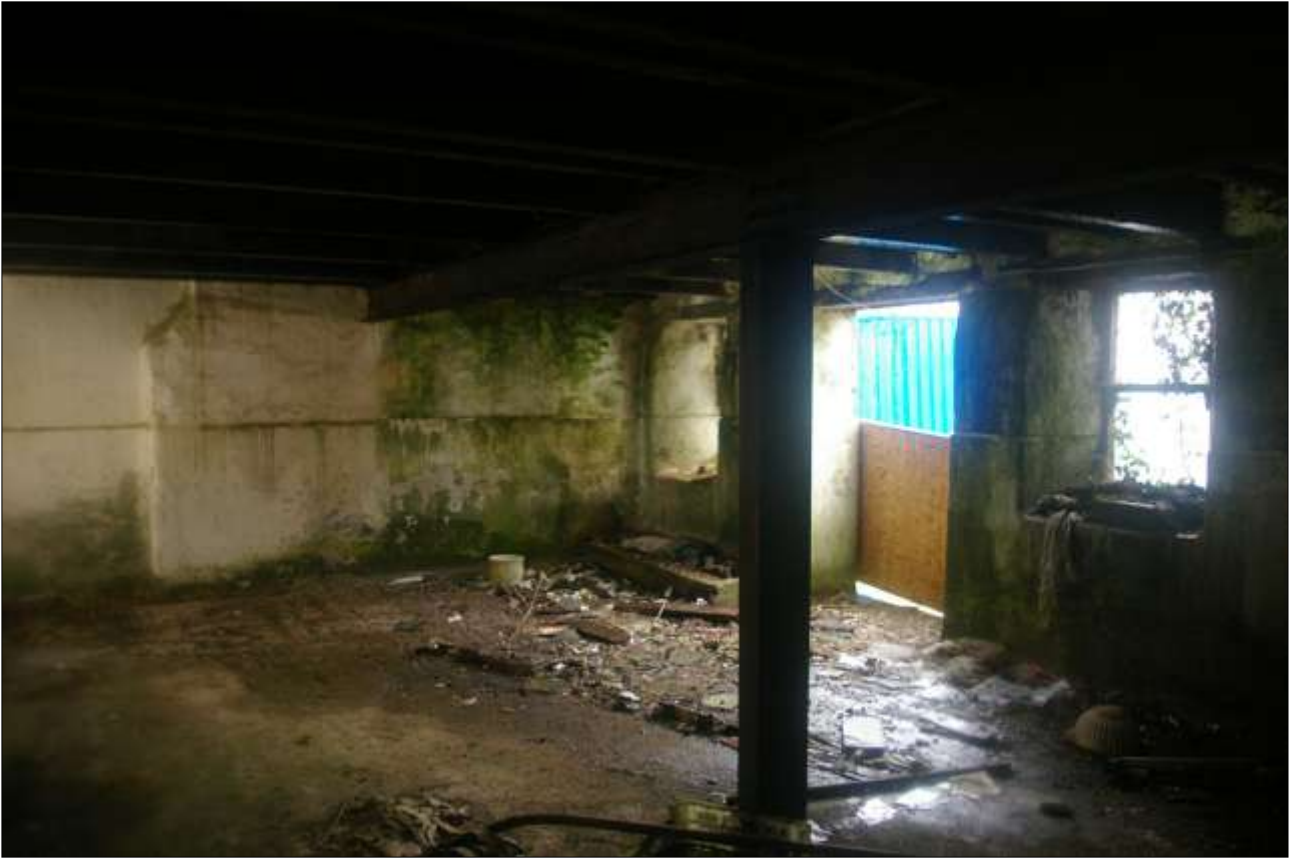
B2.2, NORTHERN GF ROOM, VIEW OF THE SOUTH-WEST CORNER OF THE ROOM, WITH FORCED DOORWAY (D7) AND WINDOWS (W13, W14); VIEWED FROM THE EAST.
