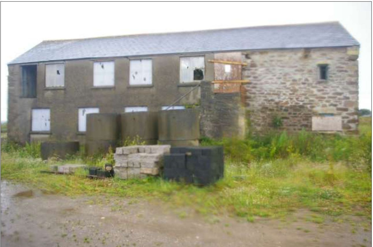
B2, SOUTH-EAST ELEVATION, MOST OF WHICH HAS BEEN REBUILT IN CONCRETE BLOCK; VIEWED FROM THE EAST-SOUTH-EAST.
