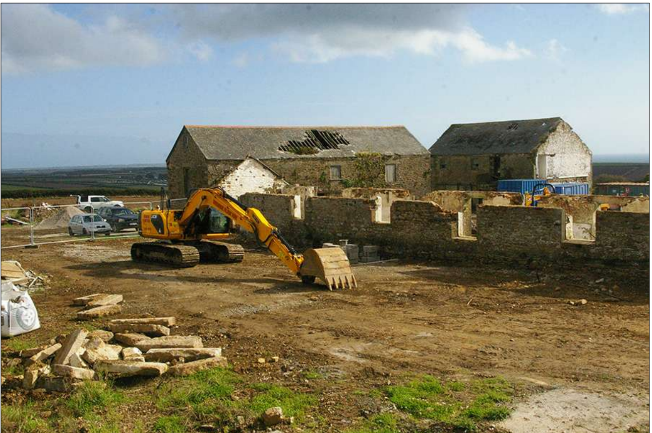
B2 AND B3, WITH B1 IN THE BACKGROUND, DURING WORKS; VIEWED FROM THE NORTH-EAST.
