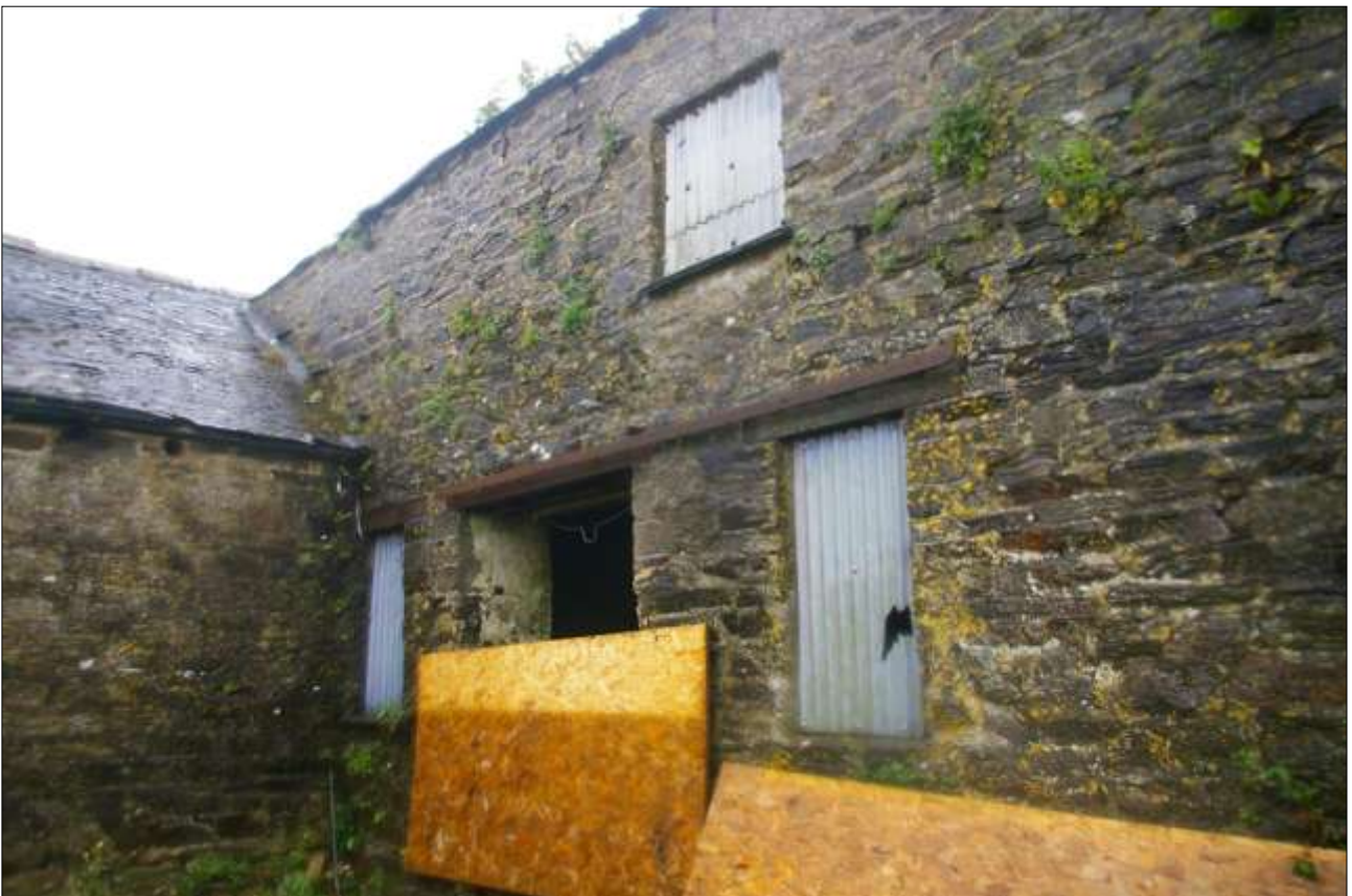
B2, THE NORTH-WEST ELEVATION IN ANGLE BETWEEN B2 AND B3, SHOWING THE FORCED DOORWAY (D7) AND TWO FORCED WINDOWS AT GF LEVEL (W13, W14); VIEWED FROM THE WEST-SOUTH-WEST.
