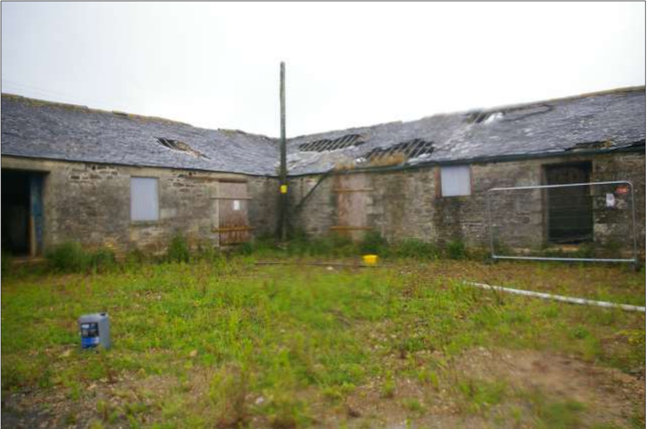
B3 (RIGHT) AND B4 (LEFT), THE ANGLE BETWEEN THE TWO BUILDINGS; VIEWED FROM THE SOUTH.
