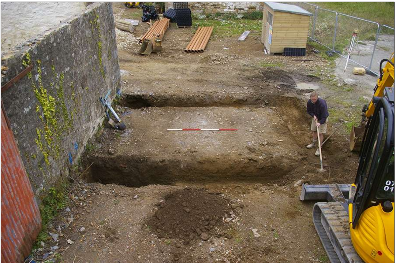
FOUNDATION TRENCH NEXT TO B5, WITH DITCH [107] TO THE LEFT; VIEWED FROM THE NORTH-WEST (SCALE 2M).
