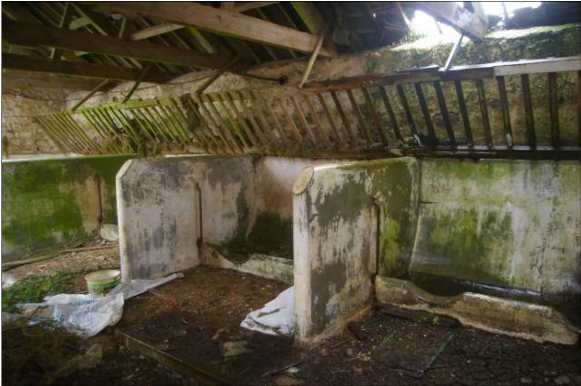
FIGURE 15: B4, SOUTHERN ROOM, THE CONCRETE STALLS AND TIMBER HAYRACKS; VIEWED FROM THE NORTH-EAST.
