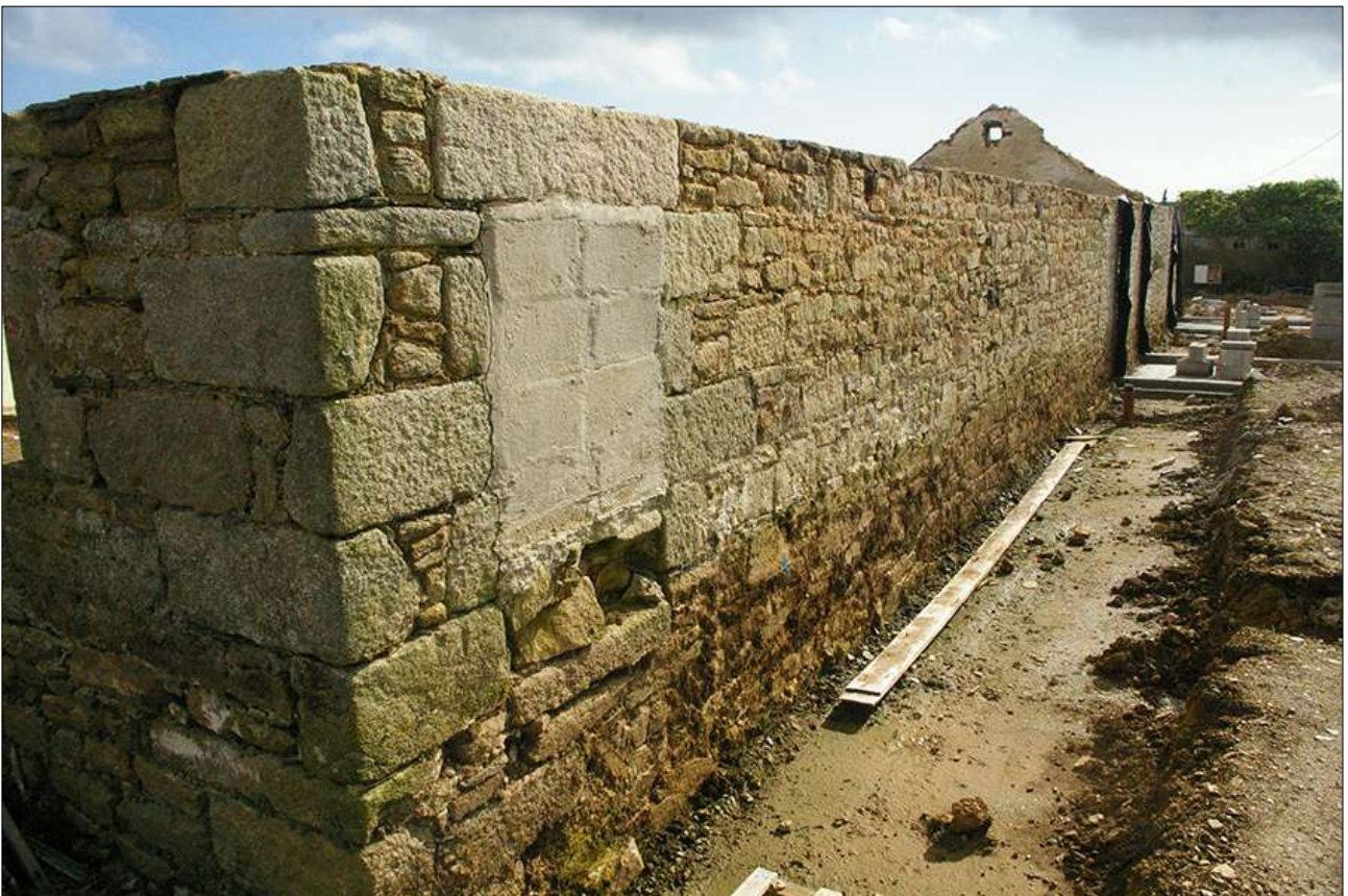
B4, DURING WORKS, SHOWING THE RAISES IN THE STONEMWORK; VIEWED FROM THE WEST-NORTH-WEST.
