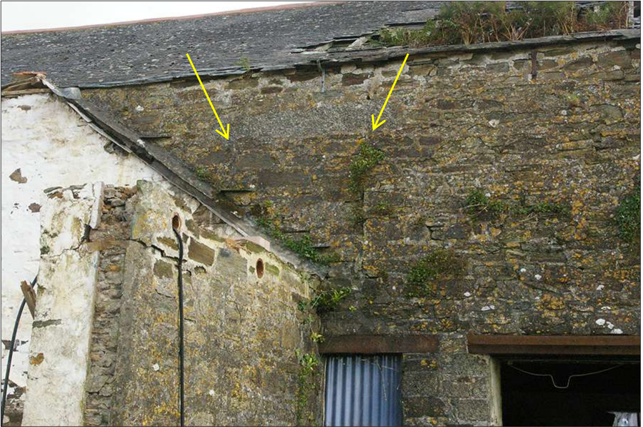
B2, THE NORTH-WEST ELEVATION ABOVE B3, SHOWING THE BLOCKED FF WINDOW (BO7) (INDICATED); VIEWED FROM THE WEST.
