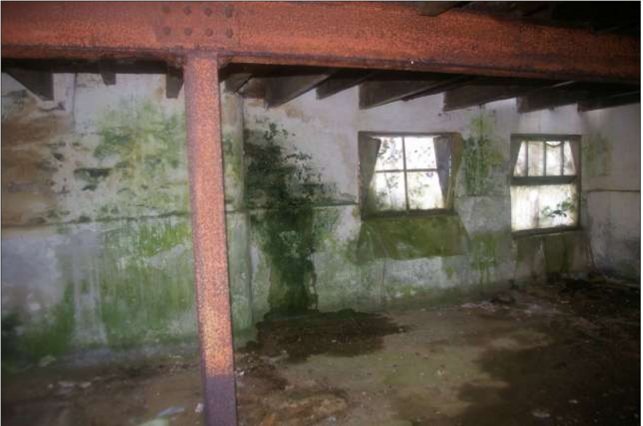
B2.2, NORTHERN GF ROOM, SHOWING THE NARROW CONCRETE BLOCK WALL AND THE TWO METAL HOPPER WINDOWS (W9, W10); VIEWED FROM THE WEST.
