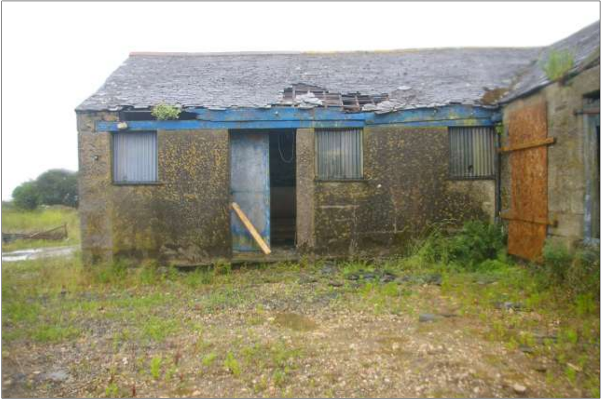
FIGURE 16: B5, NORTH-EAST ELEVATION, WITH CENTRAL GRANITE PILLAR AND OPENINGS INFILLED IN CONCRETE BLOCK; VIEWED FROM THE NORTH-EAST.
