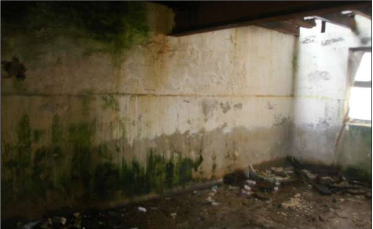
B2.1, SOUTHERN GF ROOM, SHOWING THE INTERNAL DIVIDING WALL; VIEWED FROM THE WEST-SOUTH-WEST.
