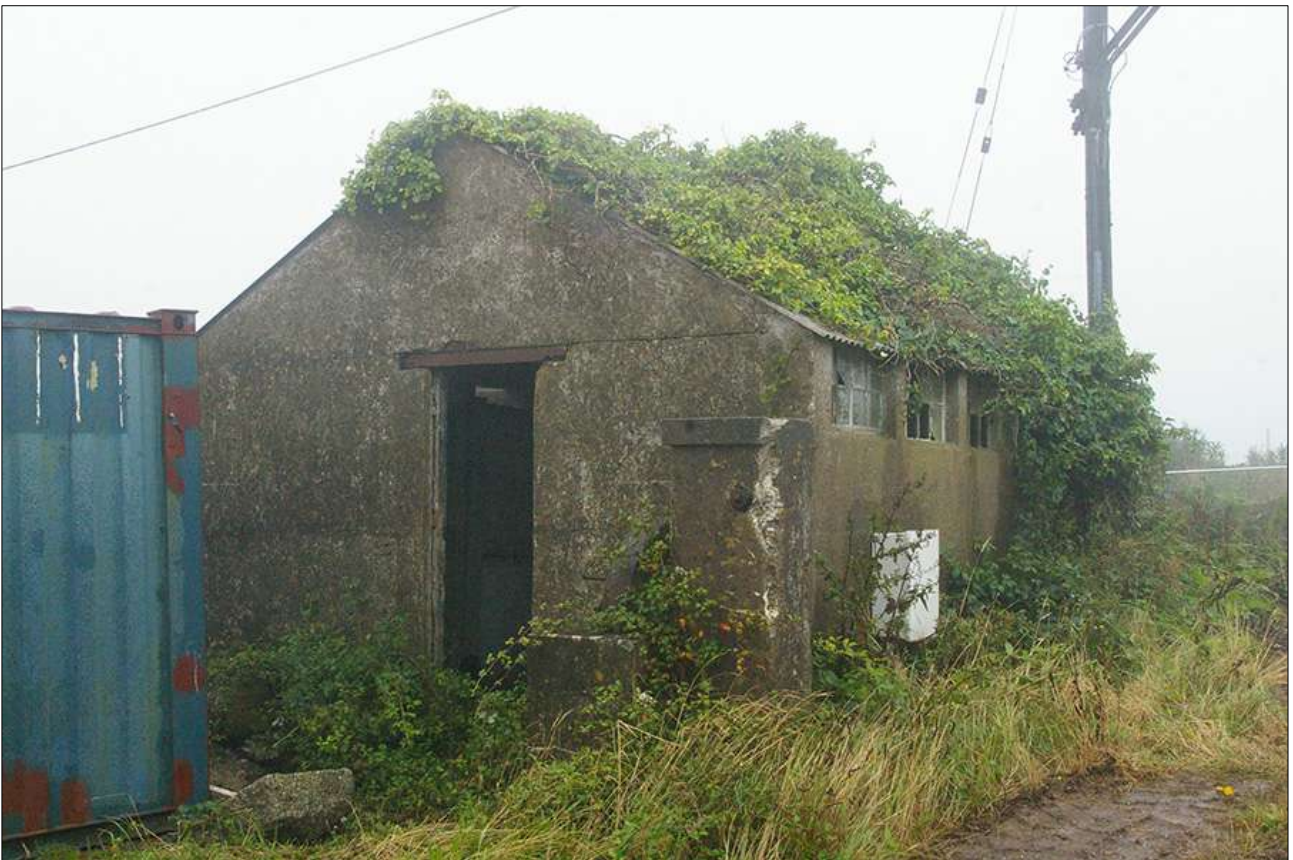
B6, A CONCRETE-BLOCK BUILDING TO THE WEST OF THE HISTORIC BARNs; VIEWED FROM THE EAST.
