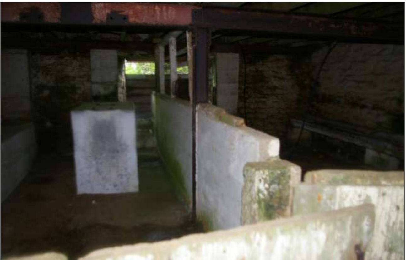
B1.2, WESTERN GF ROOM, SHOWING THE PART-BLOCKED WINDOW, CONCRETE BLOCK PENS AND LARGE CONCRETE PLINTH; VIEWED FROM THE NORTH-EAST.
