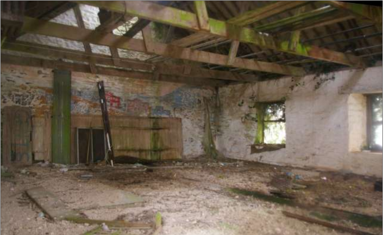
B1.3, FF ROOM, SHOWING THE PAINTED MURAL (S6); VIEWED FROM THE NORTH-NORTH-WEST.
