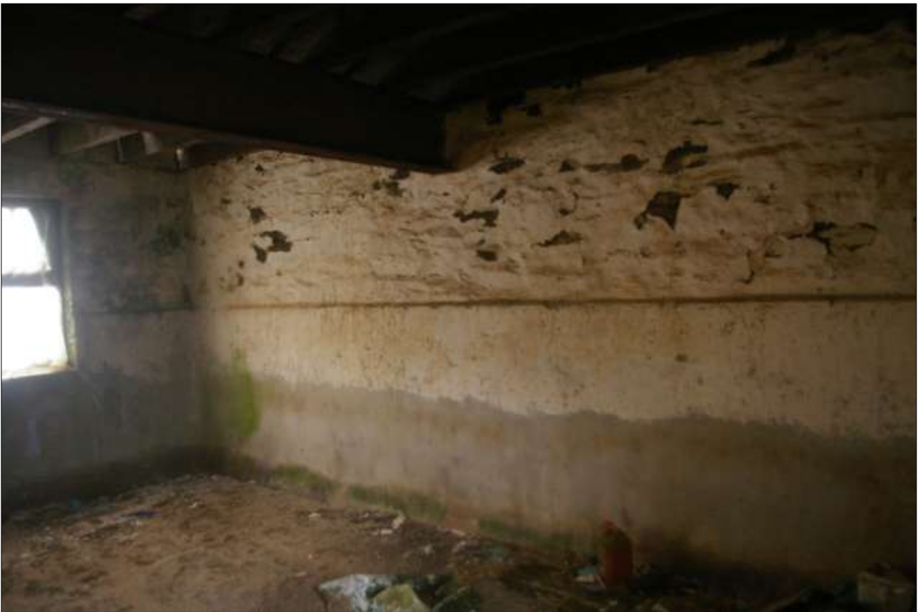
B2.1, SOUTHERN GF ROOM, SHOWING THE GABLE WALL; VIEWED FROM THE WEST-NORTH-WEST.
