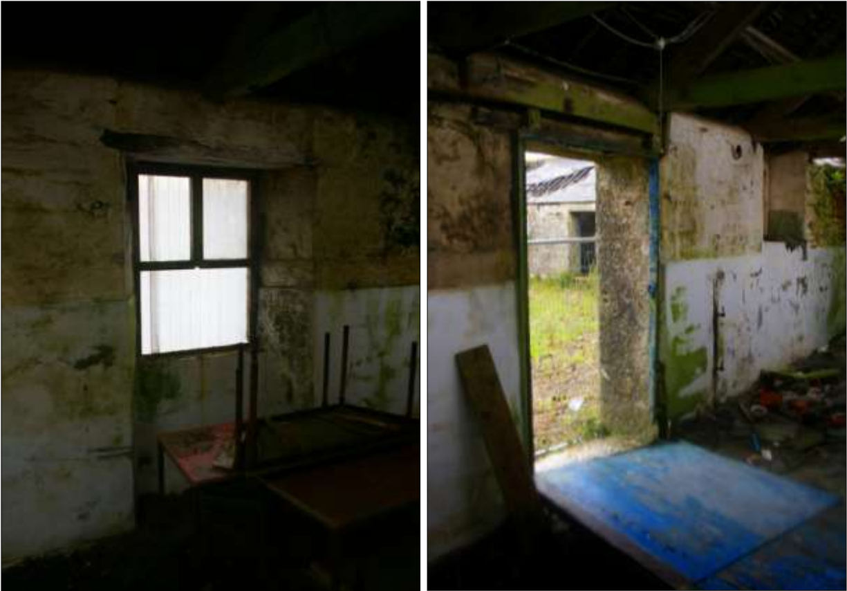
LEFT: B3.2, THE ONE ORIGINAL WINDOW (W24), SET INTO A SHALLOW ALCOVE IN THE SOUTH-WEST WALL; VIEWED FROM THE NORTH-EAST. RIGHT: B3.2, ONE OF THE ORIGINAL DOORWAYS (D12) IN THE SOUTH-WEST WALL. THE MECHANISM FOR A SLIDING DOOR SURVIVES IN SITU ; VIEWED FROM THE EAST-NORTH-EAST.
