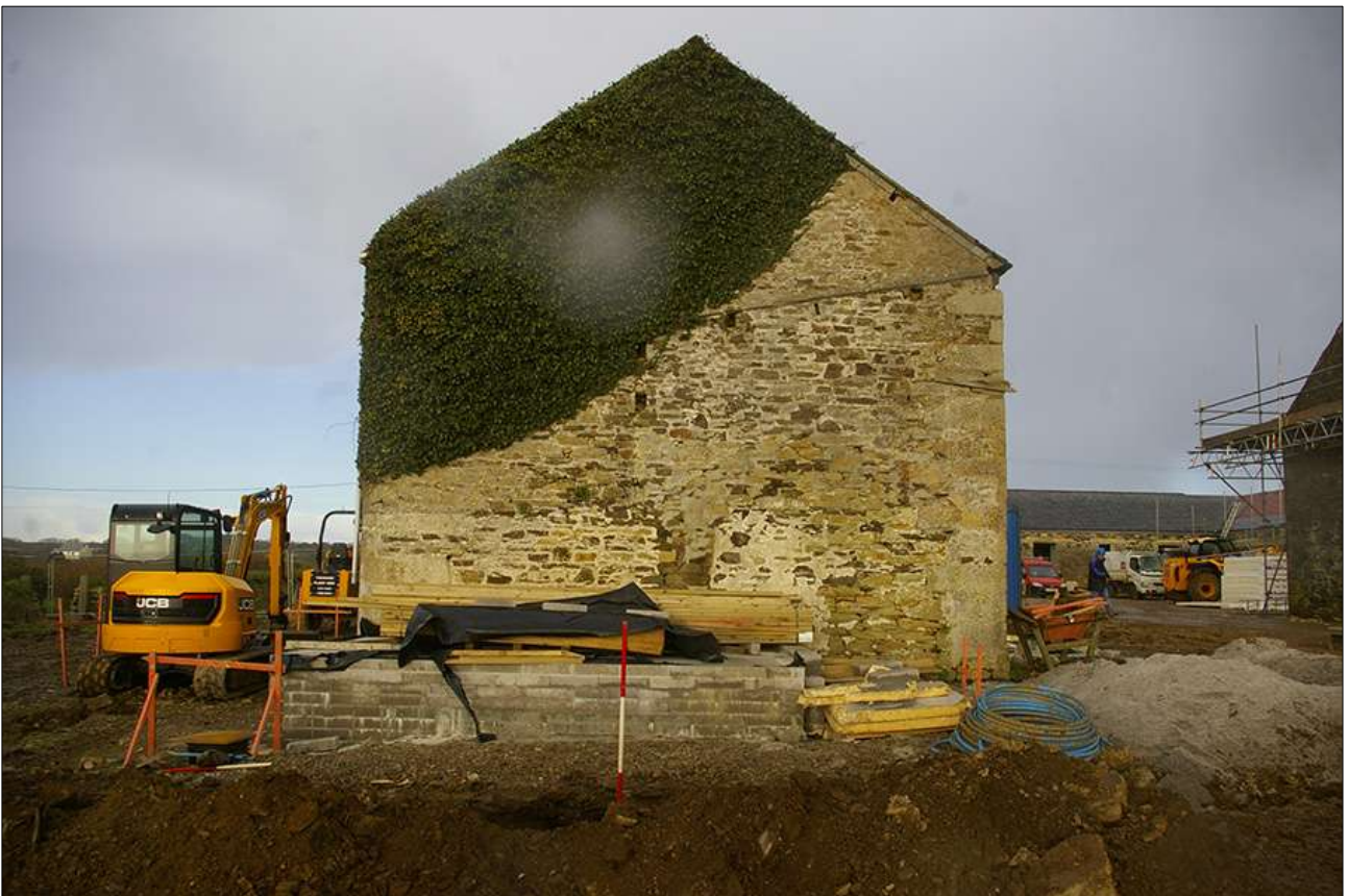
SOUTH-EAST ELEVATION OF B1 IN RELATION TO WATER PIPE TRENCH. THE SOUTH-WEST END OF WALL {313} IS MARKED BY THE RANGING POLE (SCALE 2M).
