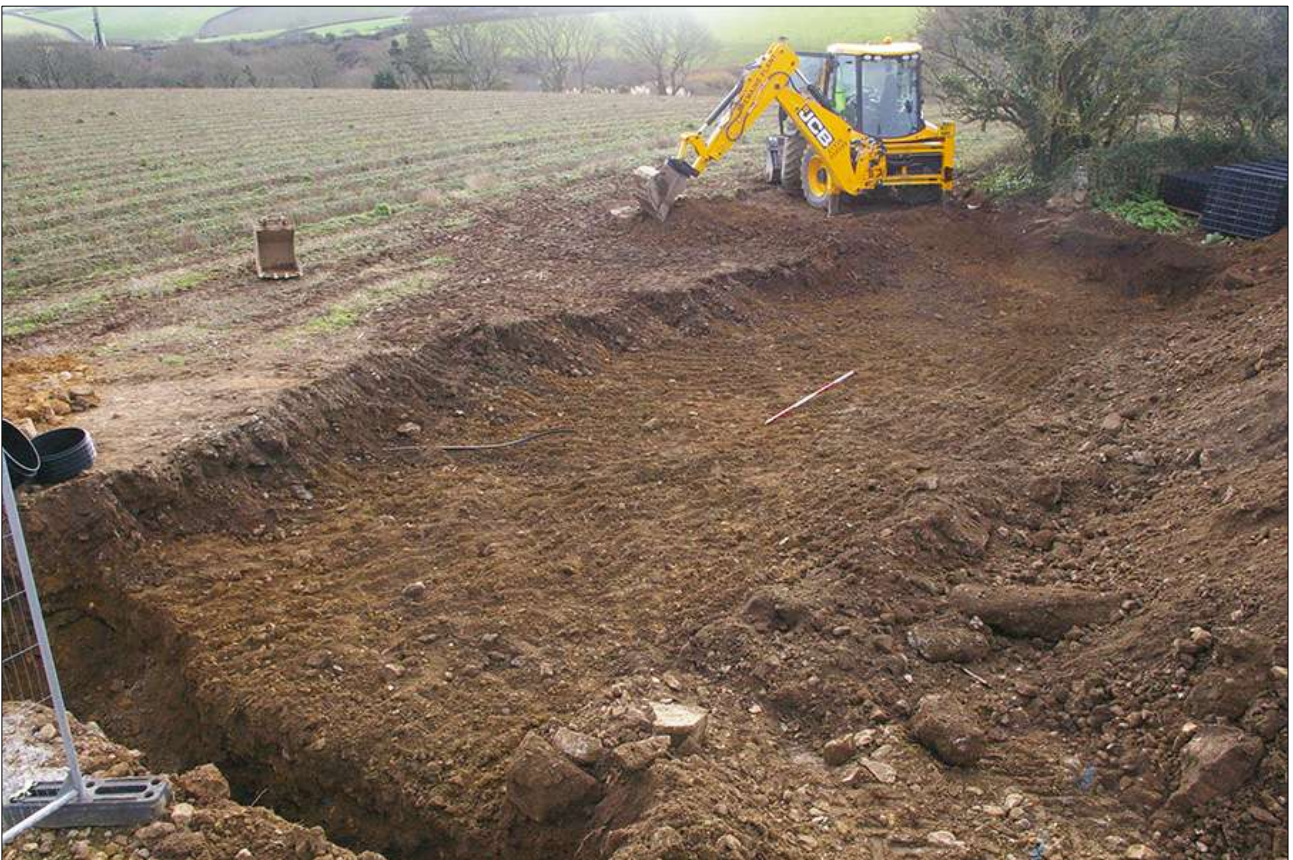
THE LARGE SOAKAWAY TRENCH EAST OF B1, POST-EXCAVATION; VIEWED FROM THE NORTH-NORTH-EAST (SCALE 2M).
