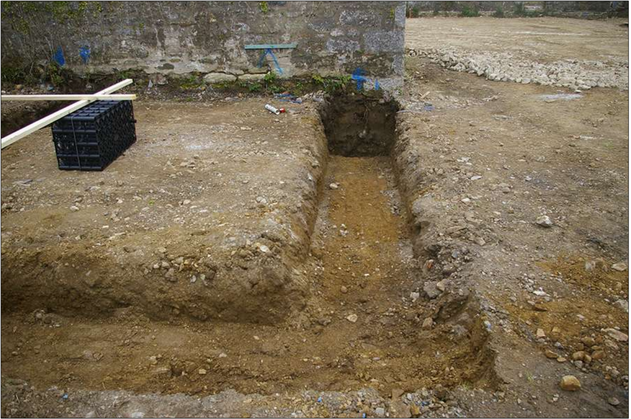
THE FOUNDATION TRENCH NEXT TO B5, THE SOUTH-EASTERN PART; VIEWED FROM THE SOUTH-WEST.
