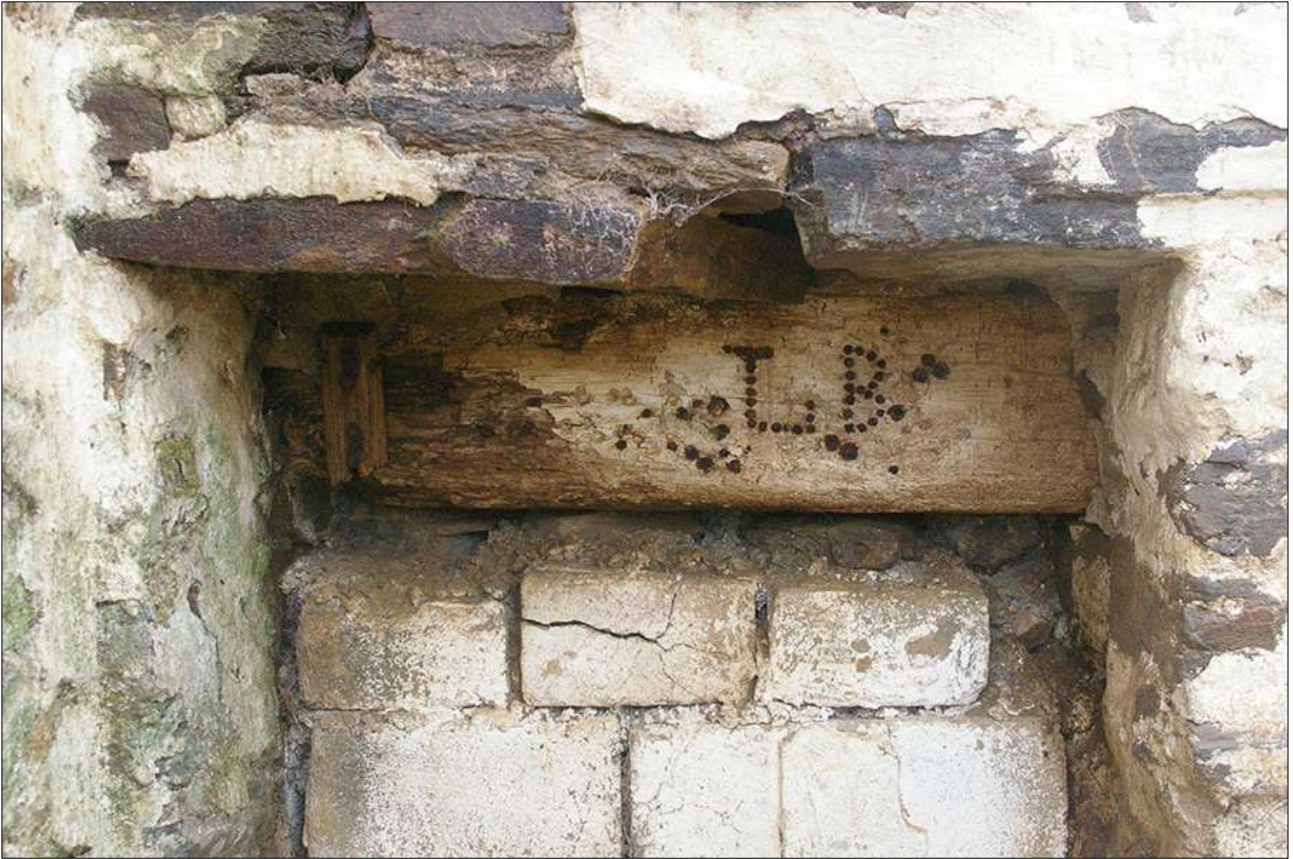
B3, AS ABOVE, DETAIL OF THE LINTEL OF THE BLOCKED DOORWAY (BO6) FROM B2.2 INTO B3.1; VIEWED FROM THE NORTH-WEST.
