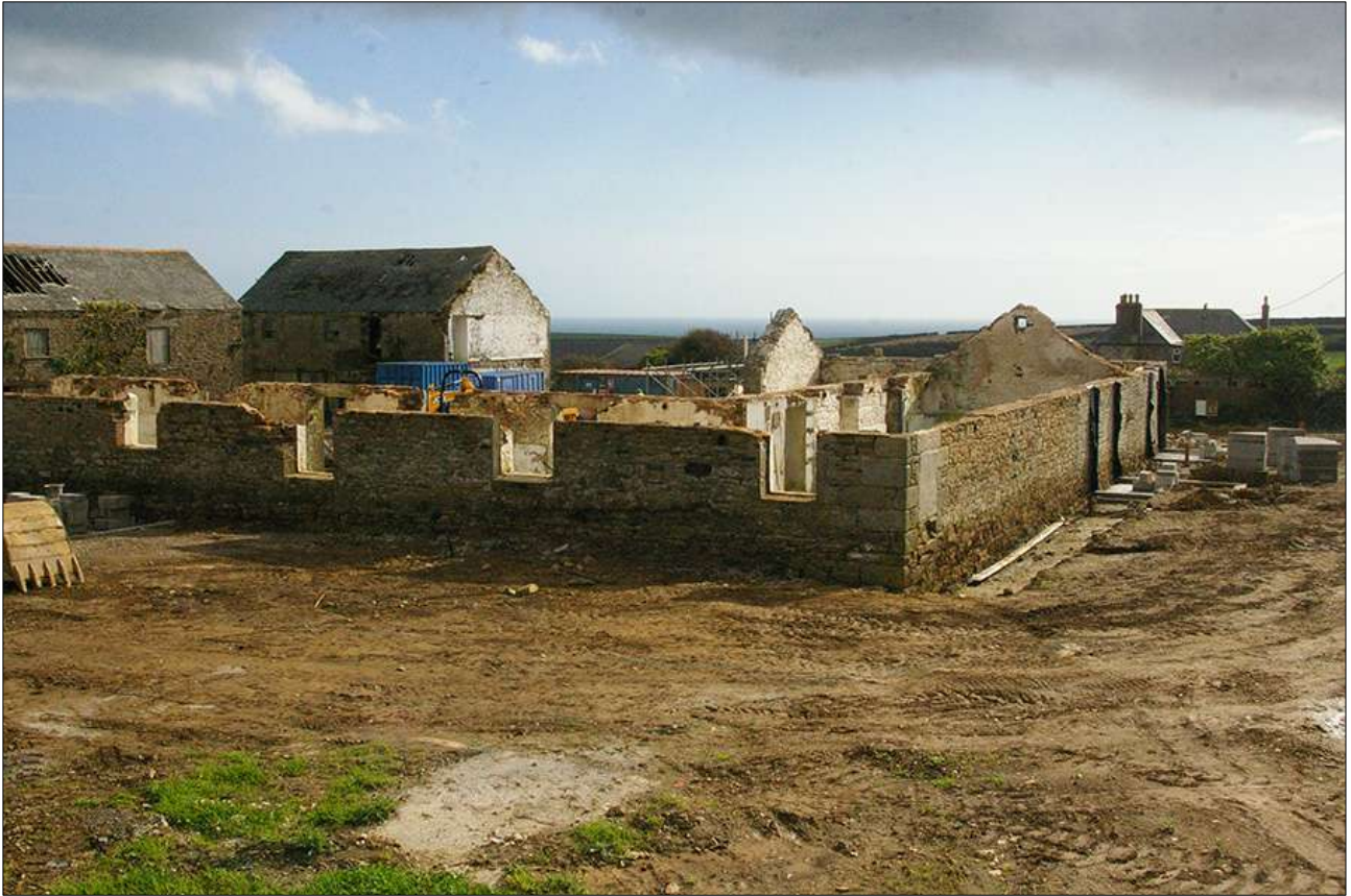
B3 AND B4, WITH B1 AND B5 IN THE BACKGROUND, DURING WORKS; VIEWED FROM THE NORTH.
