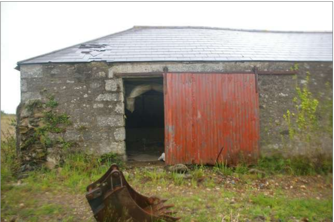
B5, SOUTH-WEST ELEVATION, SHOWING THE WIDE DOORWAY (D23) INTO THE SOUTH-WESTERN ROOM; VIEWED FROM THE SOUTH-WEST.
