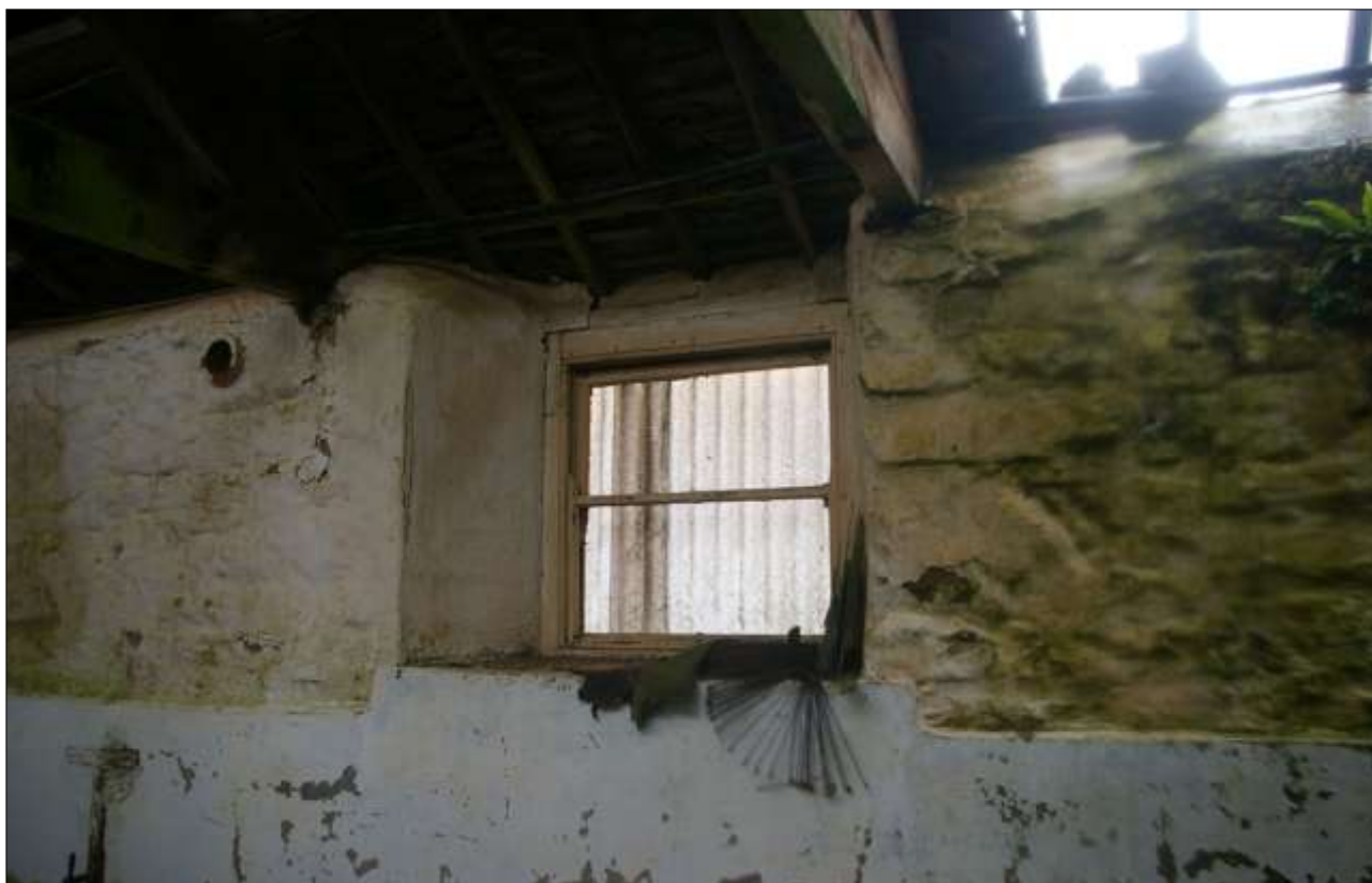
B3.2, A SASH WINDOW (W30) OF LATE 19 TH OR EARLY 20 TH CENTURY DATE IN A FORCED OPENING IN THE NORTH-EAST WALL; VIEWED FROM THE NORTH.
