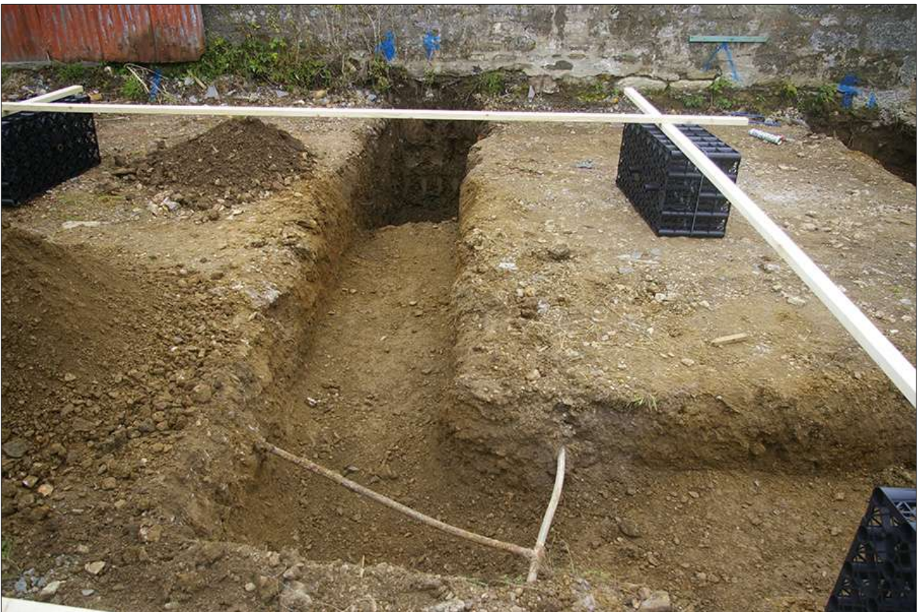
THE FOUNDATION TRENCH NEXT TO B5, THE NORTH-WESTERN PART; VIEWED FROM THE SOUTH-WEST.
