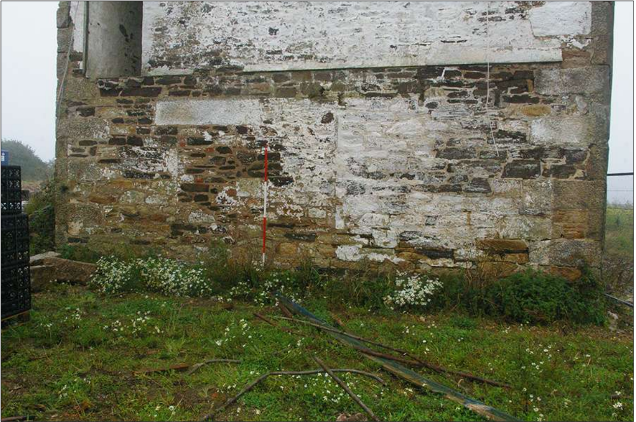
B1, DETAIL OF THE GF NORTH-WEST ELEVATION; VIEWED FROM THE WEST (SCALE 2M). BO3 VISIBLE JUST TO THE LEFT OF THE RANGING POLE.
