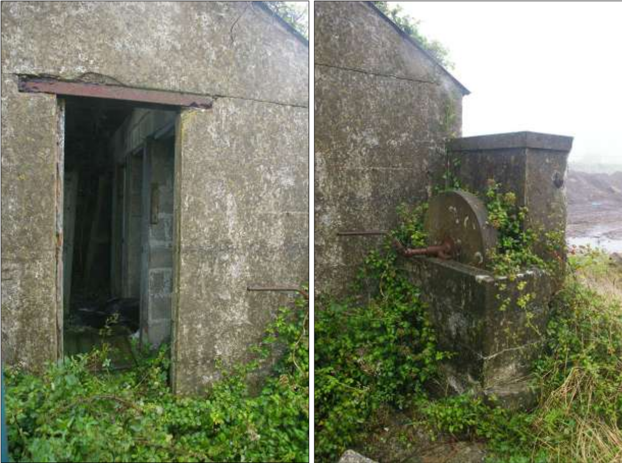
LEFT: B6, SHOWING THE CONCRETE CUBICLES INSIDE THE BUILDING; VIEWED FROM THE EAST-SOUTH-EAST. RIGHT: B6, GRINDSTONE NEXT TO DOOR; VIEWED FROM THE SOUTH.
