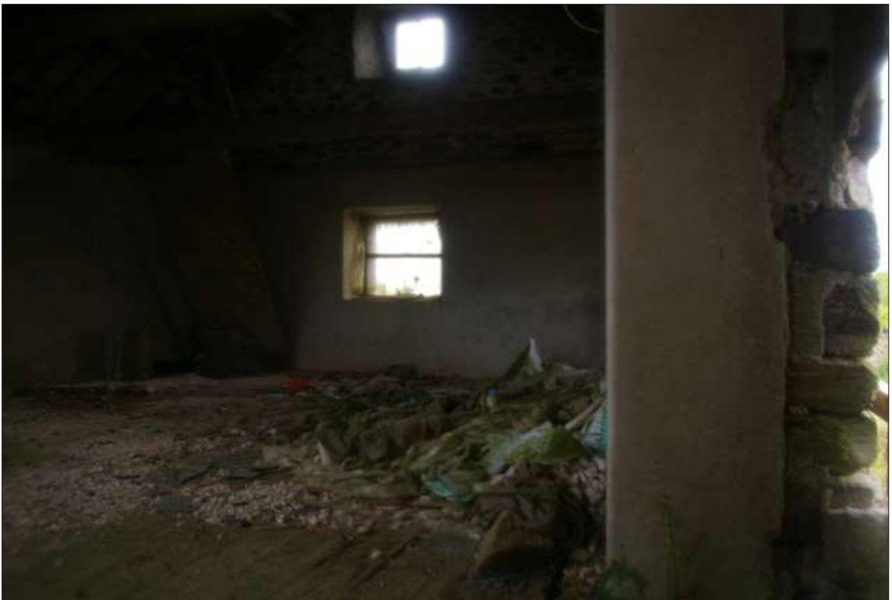
B2.3, FF ROOM, SHOWING THE NORTH GABLE AND INFILLED LOADING DOOR (D8, W22); VIEWED FROM THE SOUTH.
