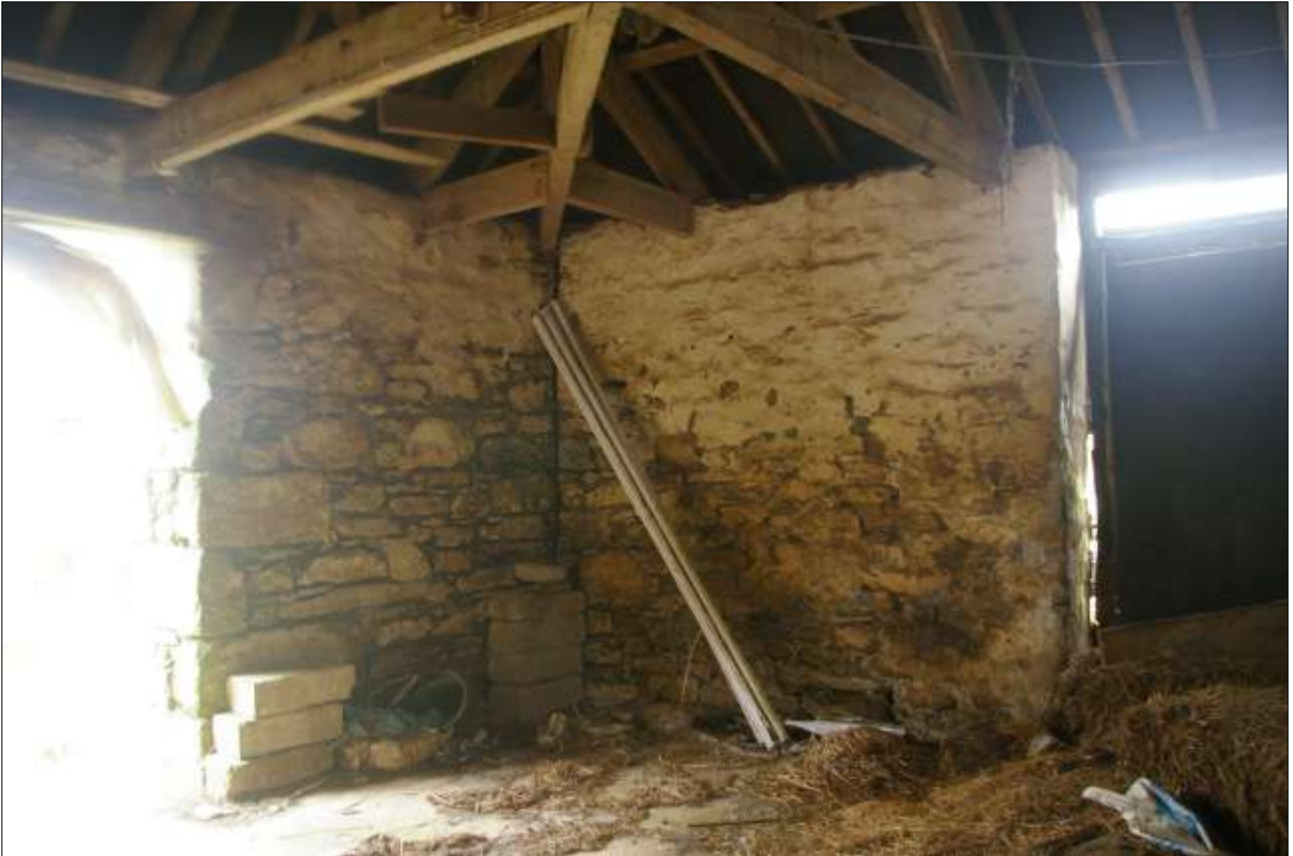
B5.2, SOUTH-WEST ROOM, SHOWING THE SOUTH-WEST ANGLE AND REBUILT SECTION OF WALL; VIEWED FROM THE EAST-NORTH-EAST.
