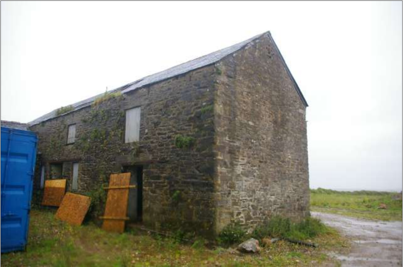
B2, SOUTH-WEST AND NORTH-WEST ELEVATIONS, SHOWING THE ROUGHLY-DRESSED GRANITE LINTELS TO THE TWO SURVIVING ORIGINAL WINDOWS (W20, W21) AND GROUND FLOOR DOOR (D6); VIEWED FROM THE WEST-SOUTH-WEST.
