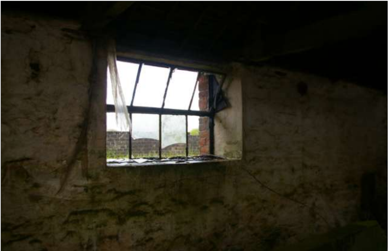
B3.2, ONE OF THE FORCED WINDOWS (W27) IN THE NORTH-EAST WALL. THE OPENING HAS BRICK REVEALS AND PATCHING TO EACH SIDE, AND FEATURES A METAL HOPPER CASEMENT WINDOW; VIEWED FROM THE WEST.
