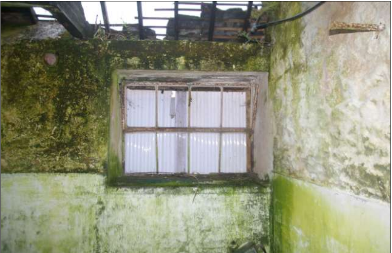
B4.2, SOUTH ROOM, SOUTH-EAST ELEVATION, A METAL HOPPER WINDOW (W32) IN A FORCED OPENING; VIEWED FROM THE WEST-NORTH-WEST.
