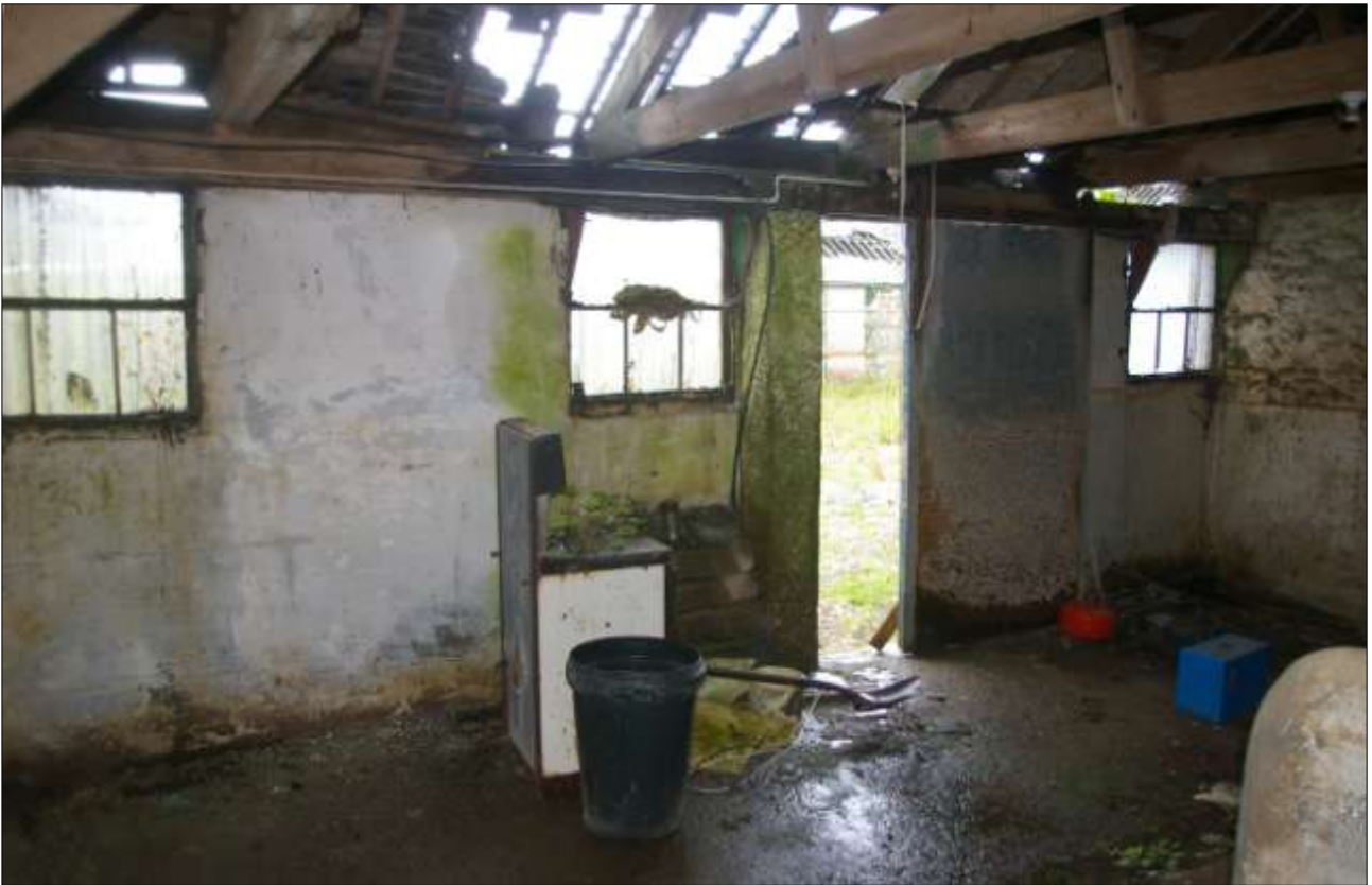
B5.3, EAST ROOM, NORTH-EAST ELEVATION, SHOWING CONCRETE WALLS AND METAL HOPPER WINDOWS (W33, W34, W35; VIEWED FROM THE WEST-SOUTH-WEST).
