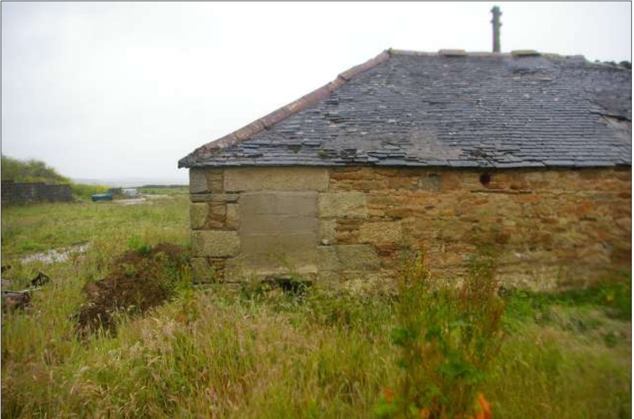
B3, BLOCKED DOORWAY (B08) AT THE NORTH-WEST CORNER, REBUILT TO PROVIDE ACCESS TO FEED CHANNEL; VIEWED FROM THE NORTH-WEST.
