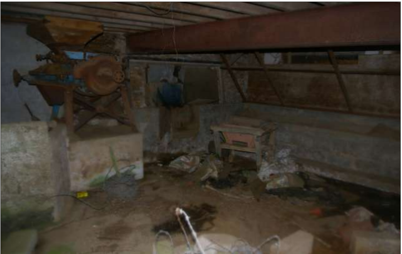
B1.1, EASTERN GF ROOM, SHOWING THE MODERN CONCRETE TROUGHS AND HAYRACK, AS VIEWED FROM THE DOORWAY (D3) INTO THE WESTERN ROOM; VIEWED FROM THE NORTH-WEST.
