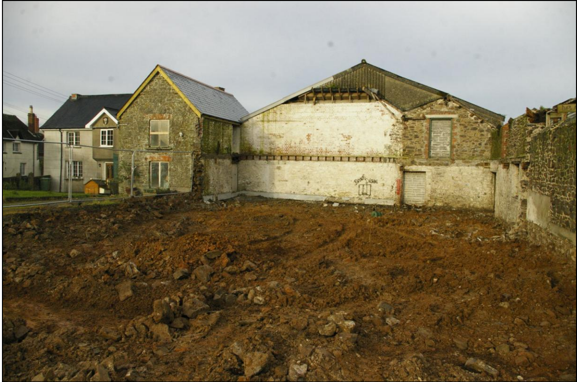
FIGURE 2: GENERAL SITE VIEW FOLLOWING REMOVAL OF CONCRETE FLOOR SURFACES SHOWING EXTENT OF TRUNCATION CAUSED BY CONSTRUCTION OF NOW DEMOLISHED BUILDINGS; VIEWED FROM THE SOUTH-EAST (NO SCALE).
