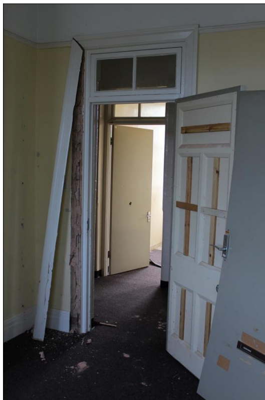
66. VIEW OF THE DOOR IN THE NORTH-EAST WALL OF ROOM F25, DEMONSTRATING IT TO BE A 1913 ORIGINAL; VIEWED FROM THE SOUTH-EAST.
