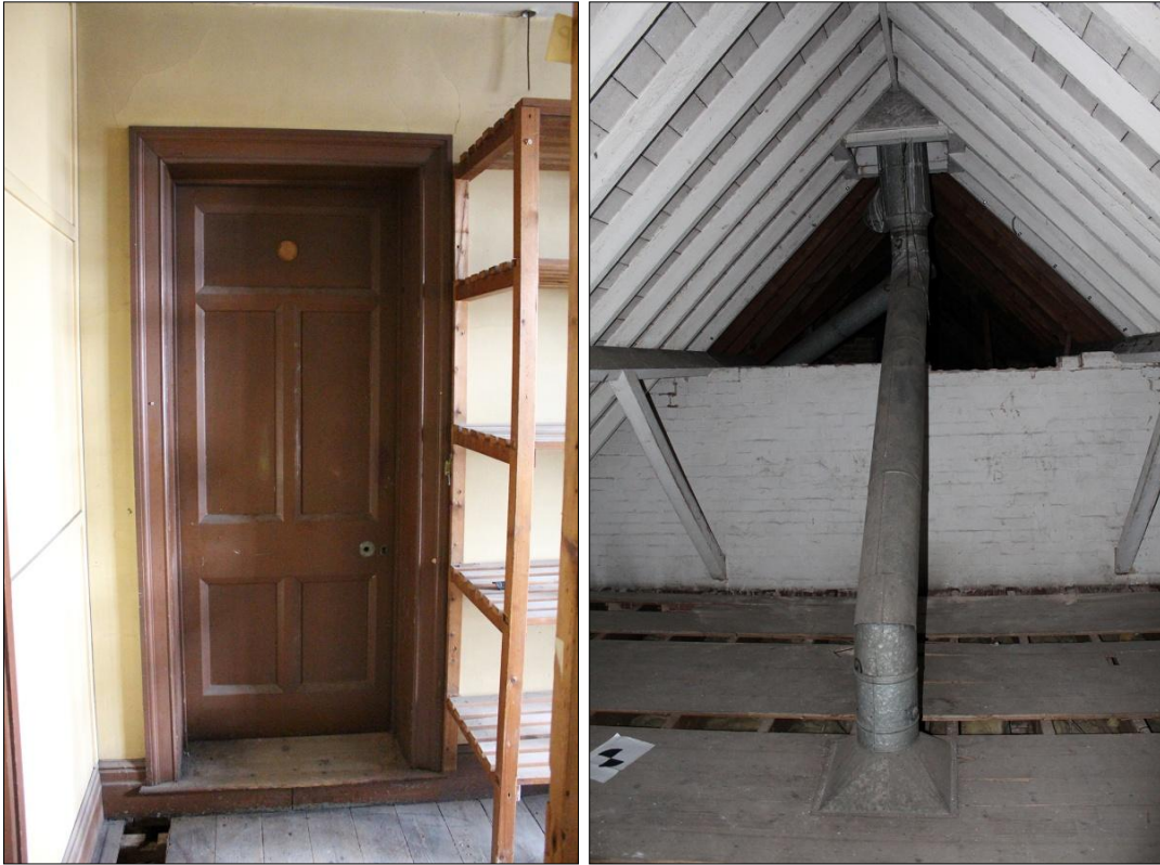
LEFT: 86. DETAIL OF THE DOOR OPENING IN THE SOUTH-EAST WALL OF ROOM S12; VIEWED FROM THE NORTH-WEST. RIGHT: 87. DETAIL OF THE METAL CHIMNEY FLUE WITHIN ROOM S13; VIEWED FROM THE NORTH-WEST.
