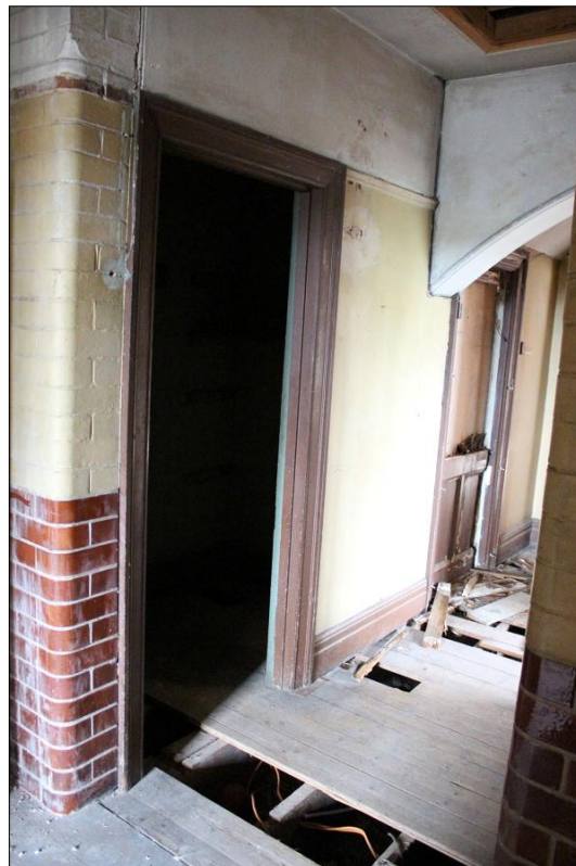
91. DETAIL OF THE DOOR OPENINGS IN THE NORTH-WEST WALL OF CORRIDOR S8; VIEWED FROM THE SOUTH-EAST.
