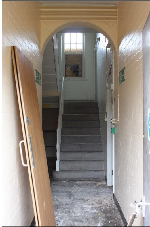
32. VIEW OF REAR ENTRANCE CORRIDOR ROOM 31, EAST WING OF BUILDING; VIEWED FROM THE NORTH-EAST.
