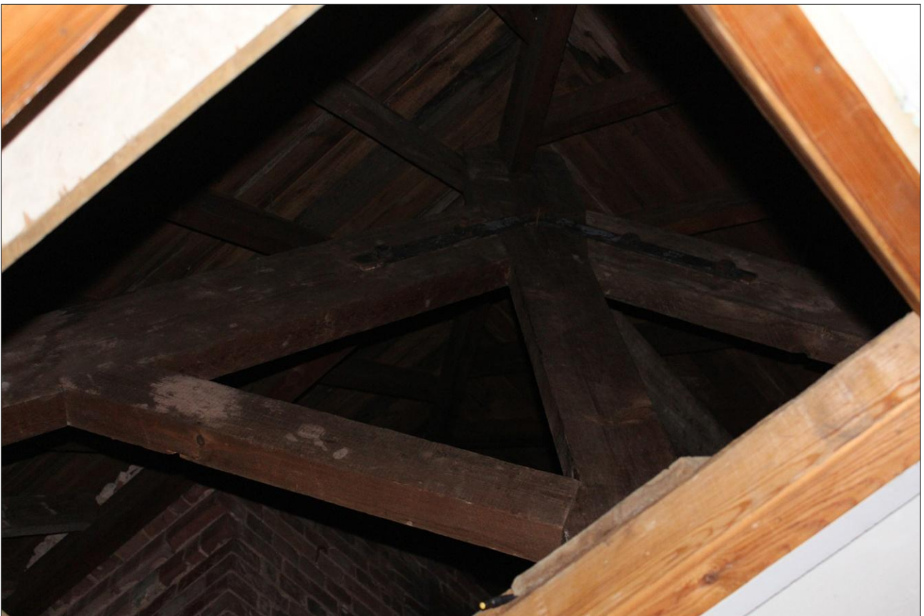
105. DETAIL OF THE ROOF STRUCTURE ABOVE CORRIDOR S8; VIEWED FROM THE NORTH-WEST.
