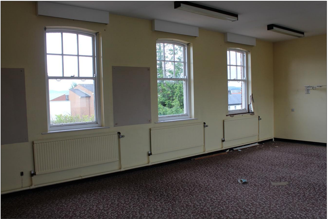
56. VIEW OF ROOM F1, WINDOW OPENINGS IN SOUTH-WEST WALL; VIEWED FROM THE EAST.
