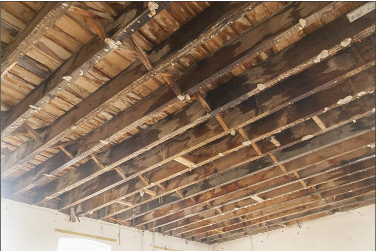
114. DETAIL OF THE HEAVY JOISTS IN ROOM F26; VIEWED FROM THE SOUTH.
