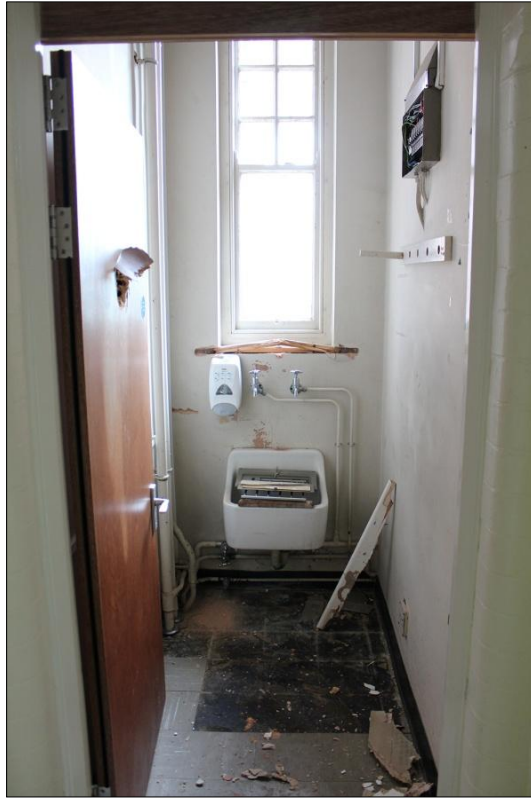
63. DETAIL OF F15 SHOWING INDICATING FORMER FUNCTION AS BATHROOM; VIEWED FROM THE SOUTH-WEST.
