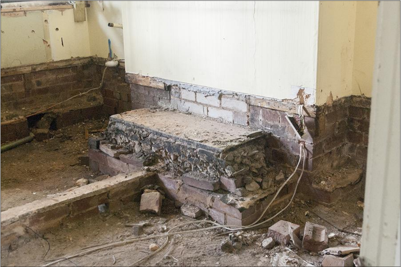
111. AS ABOVE, DETAIL OF THE HEARTH SHOWING HOW IT HAS BEEN RAISED WITH A COARSE AGGREGATE; VIEWED FROM THE NORTH-EAST.
