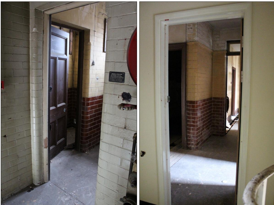
LEFT: 78. DETAIL OF DOOR OPENING IN NORTH-EAST WALL OF ROOM S3, LOOKING THROUGH INTO S2; VIEWED FROM THE SOUTH.
