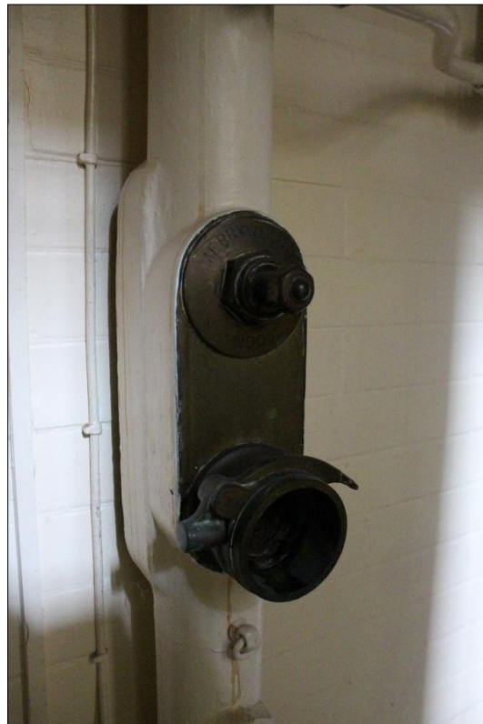
50. DETAIL OF THE FIRE HYDRANT IN THE MAIN CORRIDOR, ROOM 14; VIEWED FROM THE WEST.
