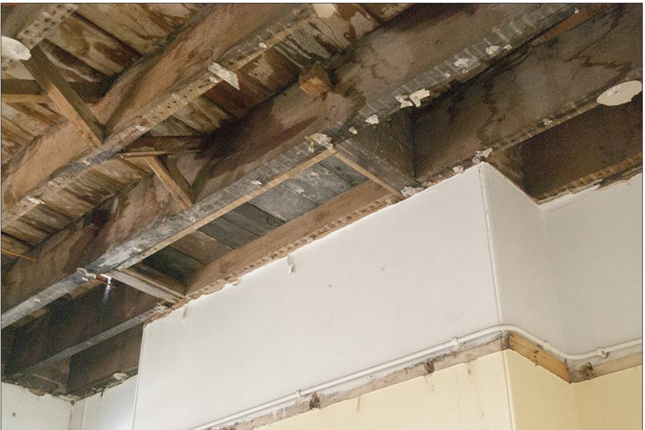
112. ROOM G36, DETAIL OF THE JOISTS SUPPORTING THE HEARTH IN ROOM F25; VIEWED FROM THE NORTH-EAST.
