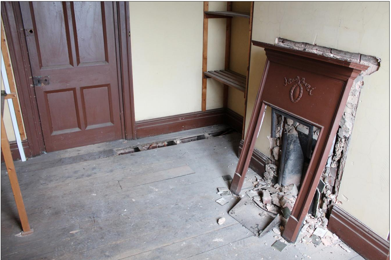
81. DETAIL OF THE FIREPLACE IN THE SOUTH-EAST WALL OF ROOM S6; VIEWED FROM THE SOUTH-WEST. THE FIREPLACE WAS TORN OFF TO CHECK FOR ASBESTOS.
