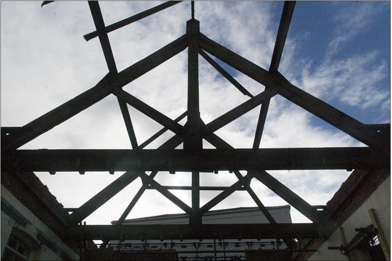
115. THE HEAVY KINGPOST ROOF TRUSSES ABOVE ROOM F26; VIEWED FROM THE NORTH-WEST.
