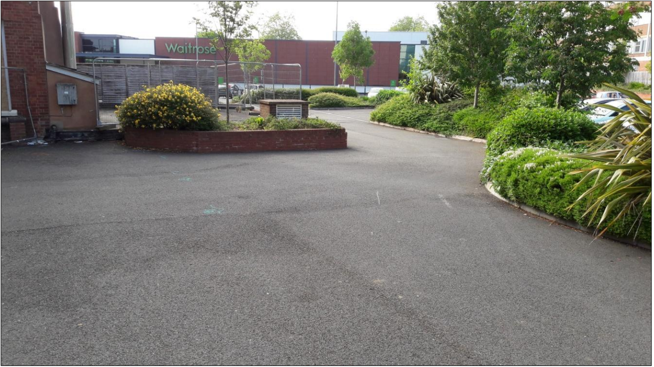
3. CAR PARK AREA TO REAR (NORTH) OF BUILDING; VIEWED FROM THE EAST (NO SCALE).
