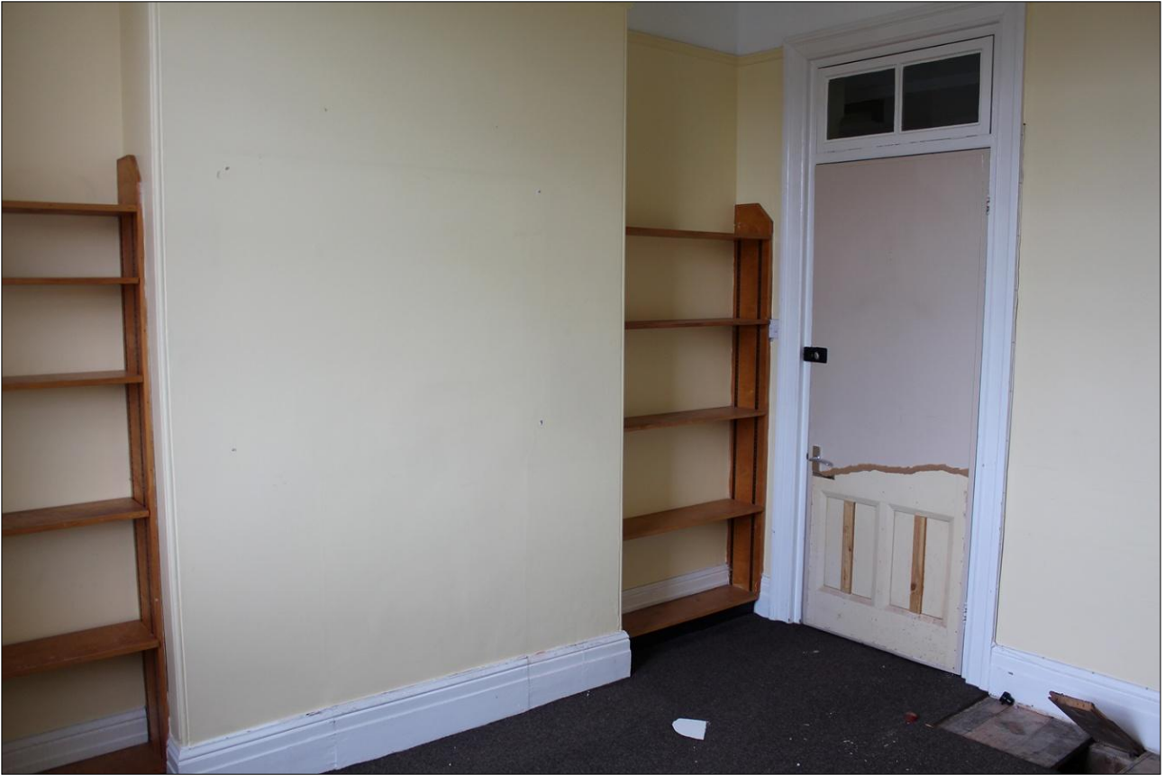
61. VIEW OF ROOM F14 SHOWING THE BLOCKED FIREPLACE IN THE NORTH-WEST WALL; VIEWED FROM THE SOUTH-EAST.
