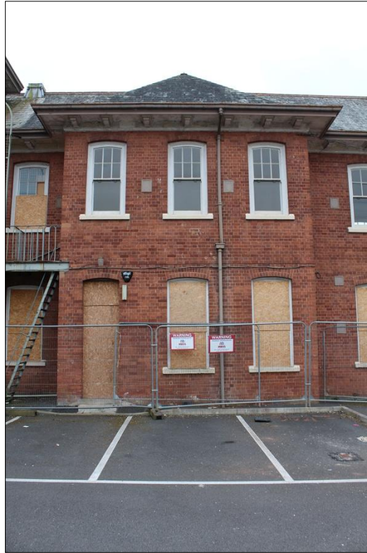
15. REAR (NORTH-EAST) EXTERNAL ELEVATION OF BUILDING, WEST END; VIEWED FROM THE NORTH-EAST.
