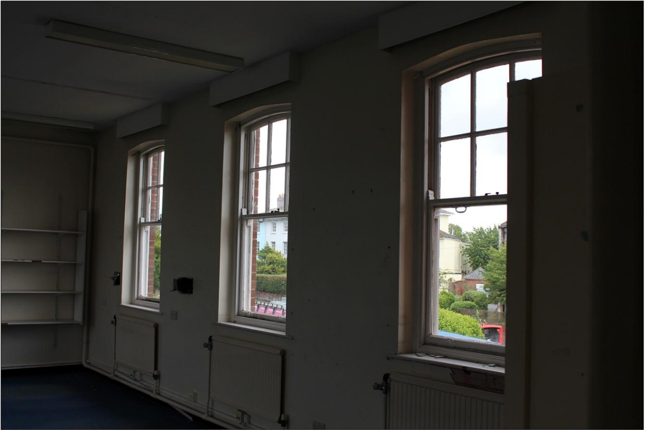
67. DETAIL OF WINDOW OPENINGS IN THE SOUTH-WEST WALL OF ROOM F26; VIEWED FROM THE NORTH-WEST.
