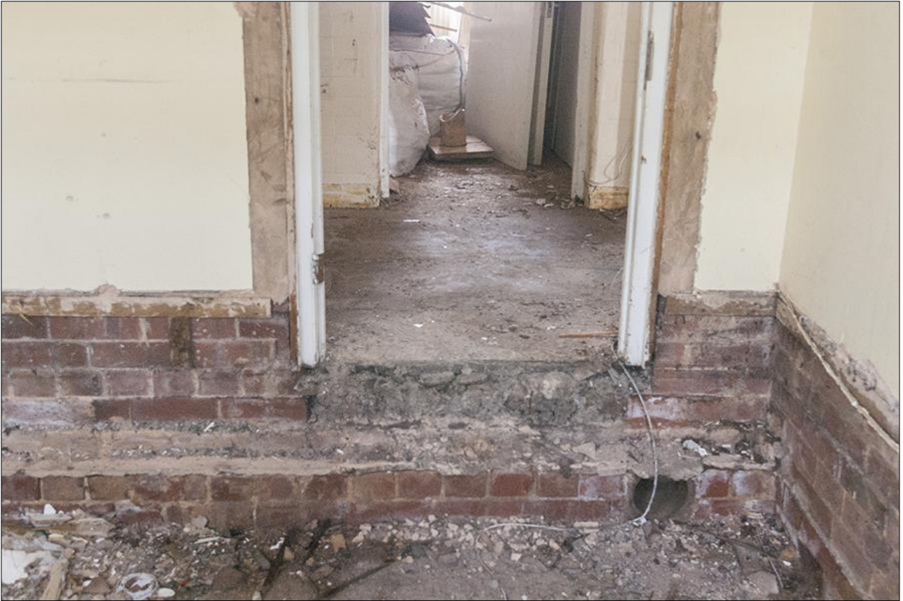
113. THE DOORWAY IN ROOM G36, SHOWING HOW THE LEVEL IN THE CORRIDOR WAS RAISED WITH A COARSE AGGREGATE; VIEWED FROM THE SOUTH-WEST.
