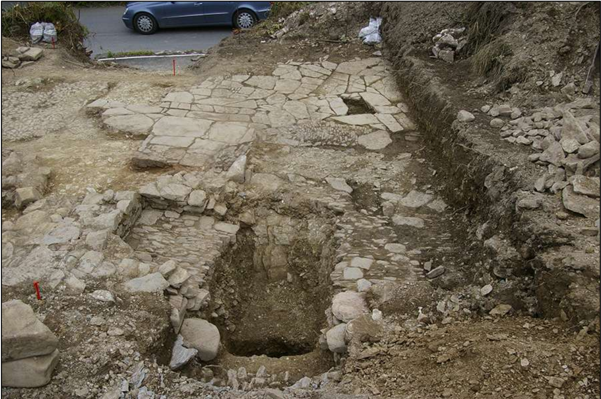
SITE SHOT, MID EXCAVATION, WEST HALF OF THE SITE; VIEWED FROM THE NORTH-EAST (NO SCALE).
