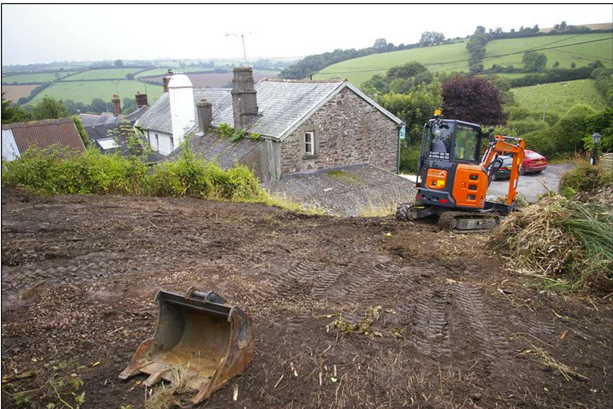
SITE SHOT FROM THE NORTH-WEST CORNER; VIEWED FROM THE NORTH (NO SCALE).
