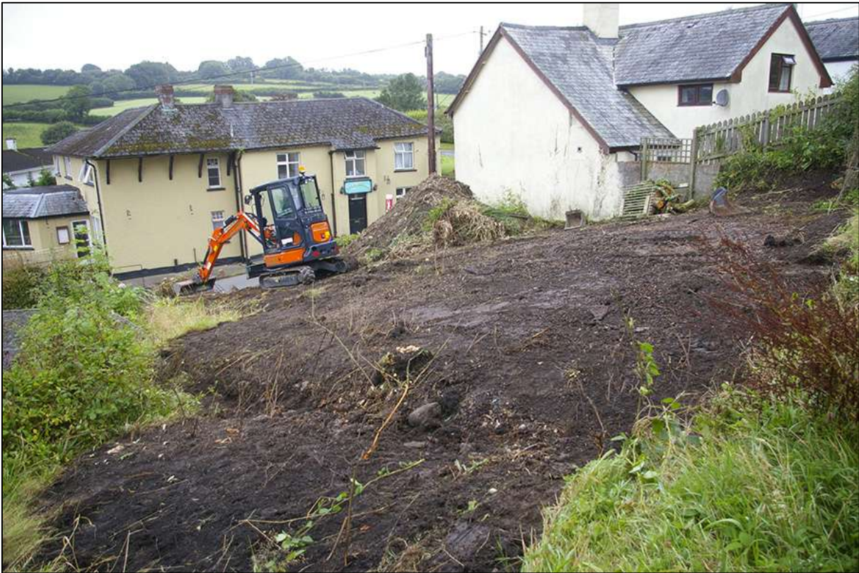
SITE SHOT FROM THE NORTH-EAST CORNER; VIEWED FROM THE EAST (NO SCALE).
