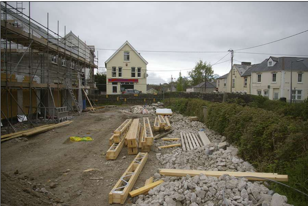
FIGURE 18: SOUTH-WEST EDGE OF THE SITE, BESIDE THE RIVER; VIEWED FROM THE NORTH-WEST.
