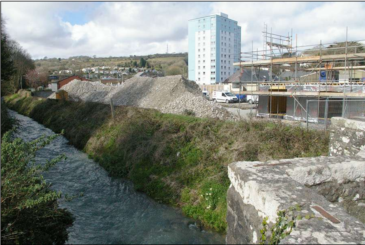
FIGURE 7: SITE UNDER CONSTRUCTION FROM THE FAR SIDE OF THE 'OLD BRIDGE'; VIEWED FROM THE SOUTH-WEST.
