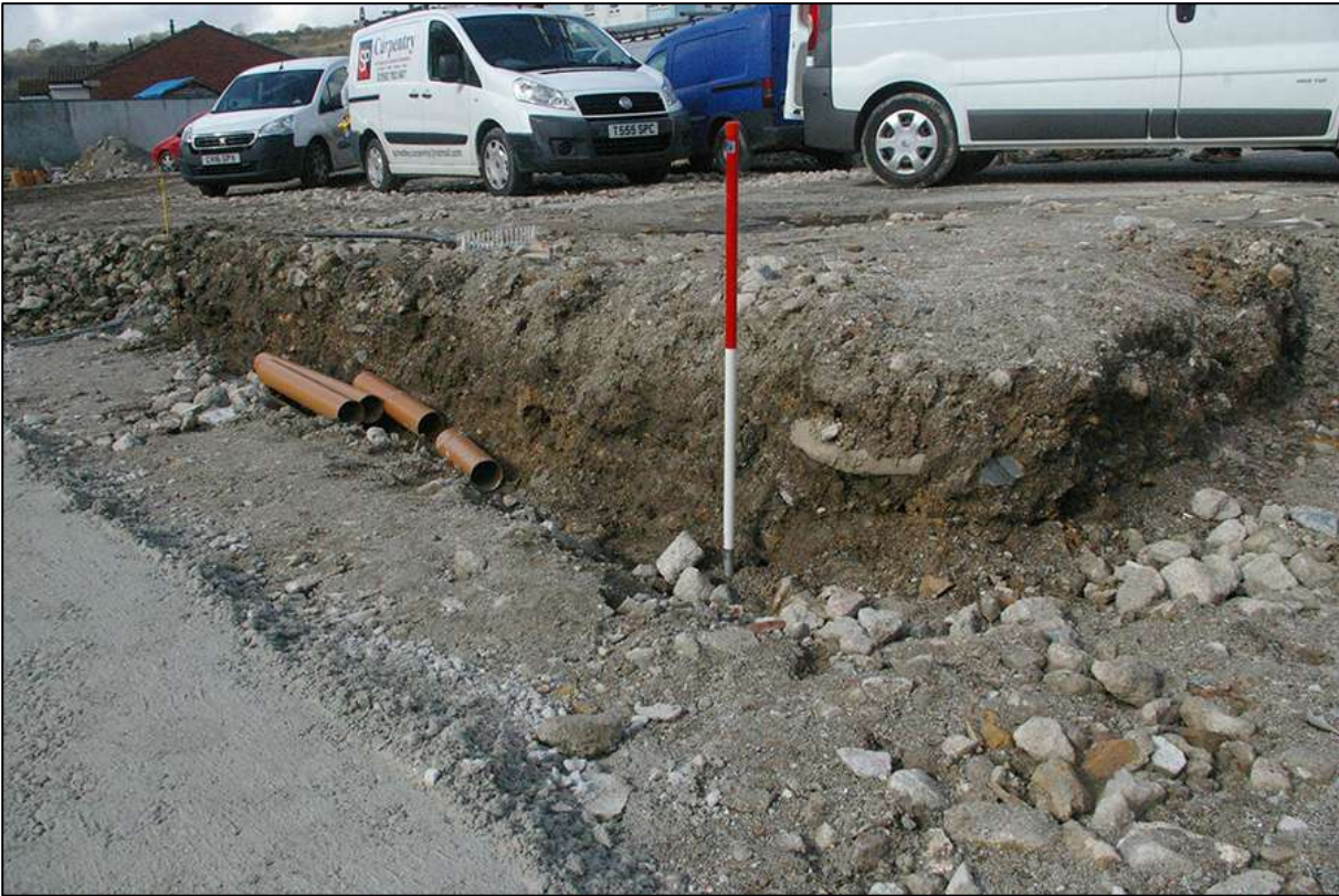
FIGURE 9: SECTION OF LARGE EXCAVATED AREA, MID-EXCITATION; VIEWED FROM THE SOUTH (1M SCALE).
