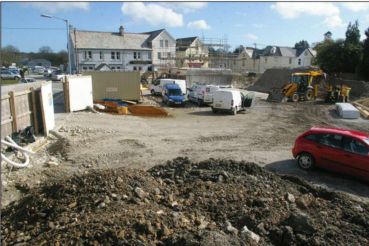
FIGURE 8: SITE SHOT FROM THE NORTH CORNER OF THE SITE; VIEWED FROM THE NORTH.
