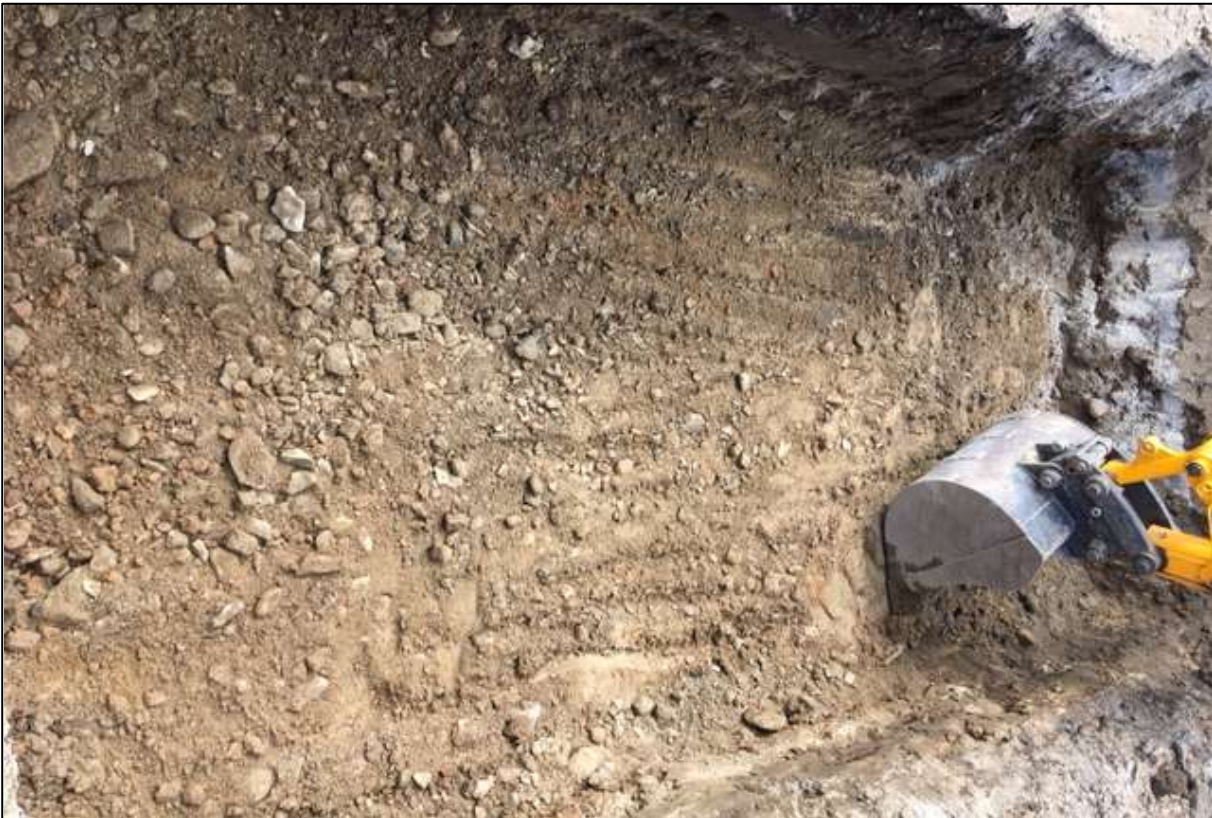
FIGURE 22: SMALL TRENCH IN THE NORTH CORNER OF THE SITE, IMAGE ROTATED 90° COUNTER CLOCKWISE; VIEWED FROM THE NORTH.
