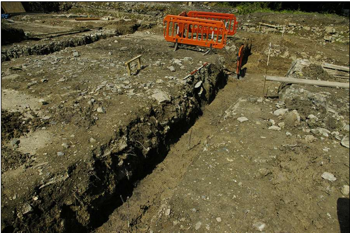
AREA 01 MIDDLE FOUNDATION TRENCH, NORTH-EAST FACING SECTION, OBLIQUE; VIEWED FROM THE EAST-NORTH-EAST (2M SCALE).
