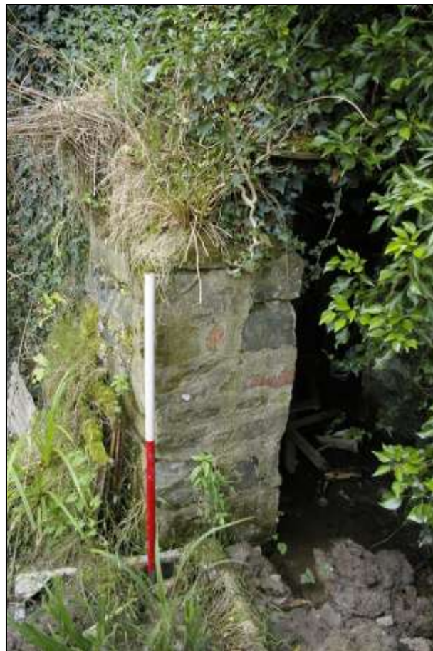
BUILDING 6 DETAIL OF REPAIRS TO NORTH WALL; VIEWED FROM THE NORTH-WEST (1M SCALE).
