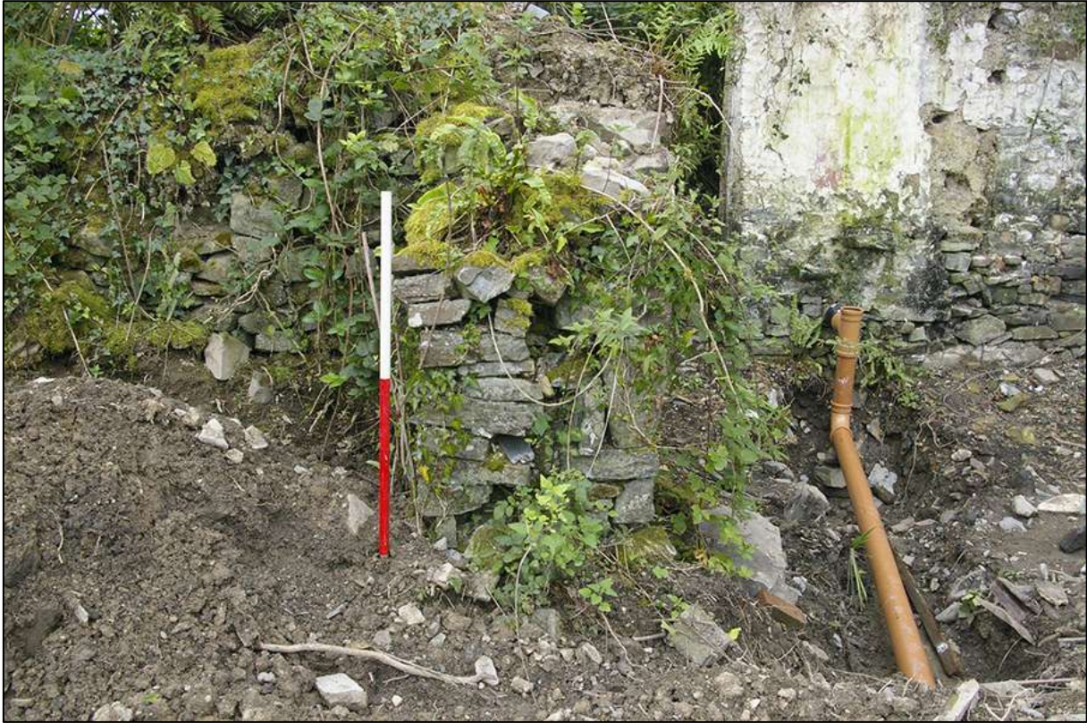
WALL 5 DETAIL OF NORTHERN RETURN AT WEST END; VIEWED FROM THE NORTH-EAST (1M SCALE).
