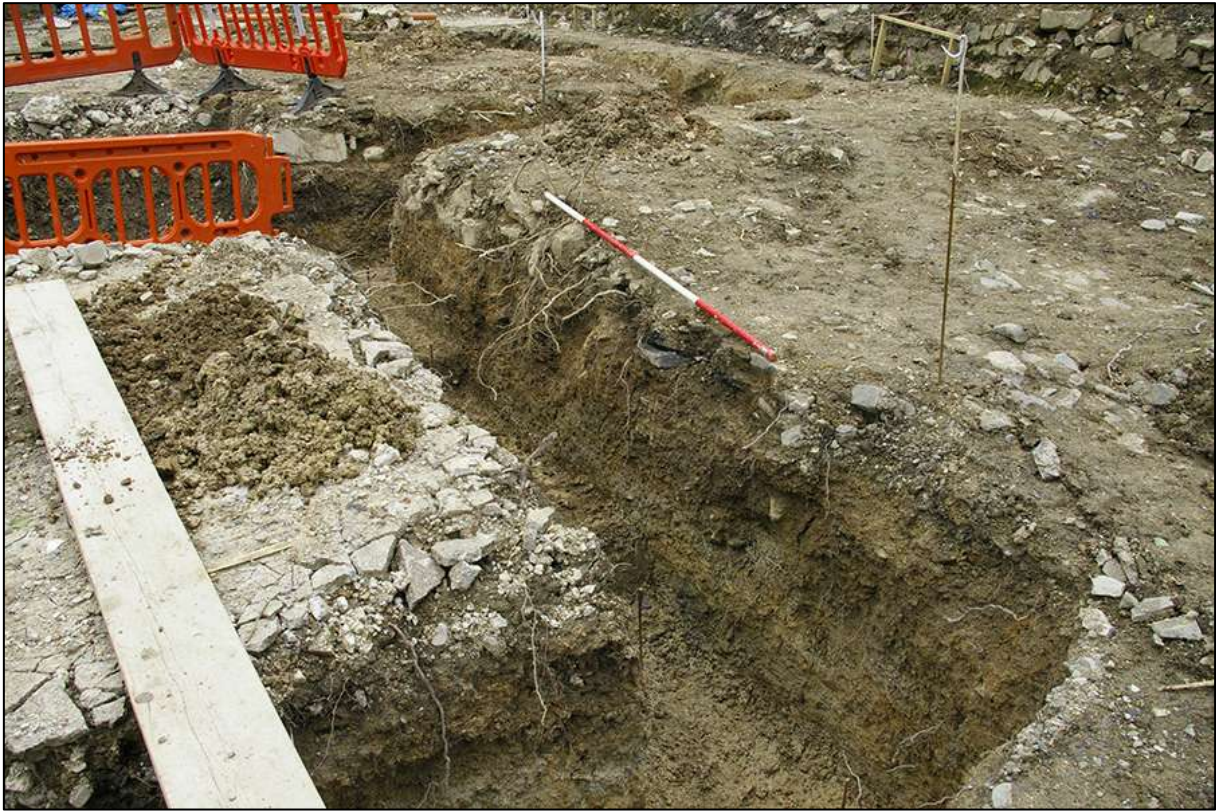
AREA 01 NORTH-WESTERN FOUNDATION TRENCH, SOUTH-EAST FACING SECTION, OBLIQUE; VIEWED FROM THE NORTH-EAST (2M SCALE).
