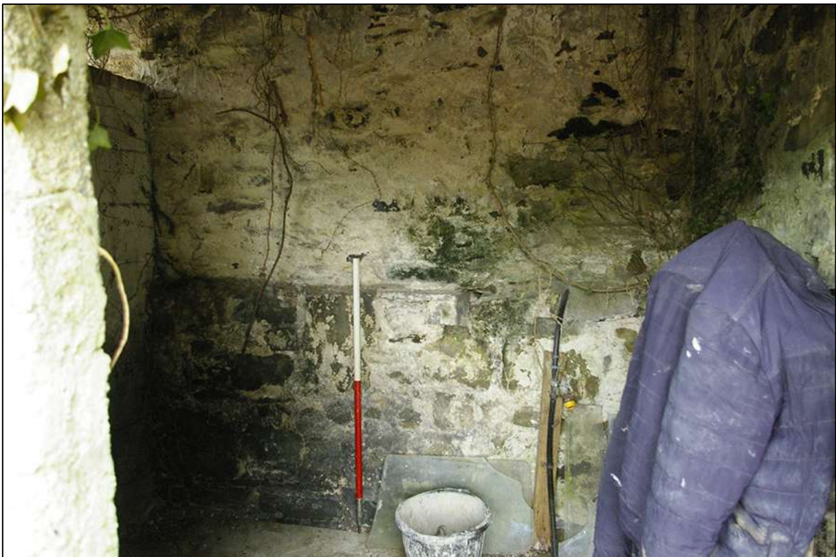
BUILDING 2 INTERNAL NORTH-EAST ELEVATION (SOUTH WALL, WALL 4); VIEWED FROM THE NORTH-EAST (1M SCALE).
