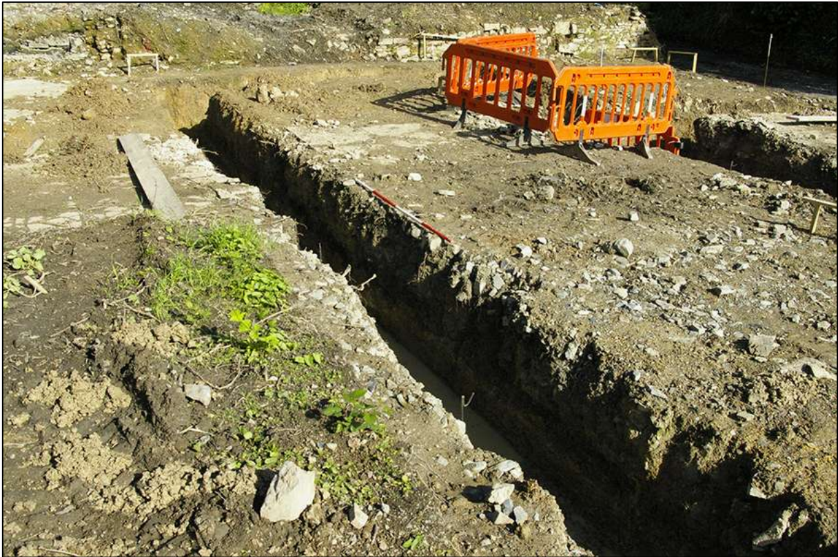
AREA 01 SOUTHERN FOUNDATION TRENCH, SOUTH-WEST FACING SECTION, OBLIQUE; VIEWED FROM THE SOUTH-EAST (2M SCALE).
