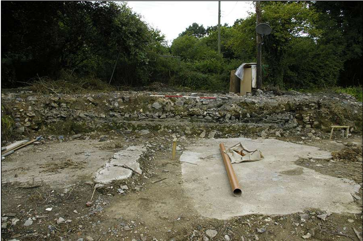
GENERAL SITE SHOT, SHOWING BACKFILL RUBBLE WITHIN BUILDING 1 (BEHIND AND BENEATH SCALE); VIEWED FROM THE SOUTH-EAST (2M SCALE).
