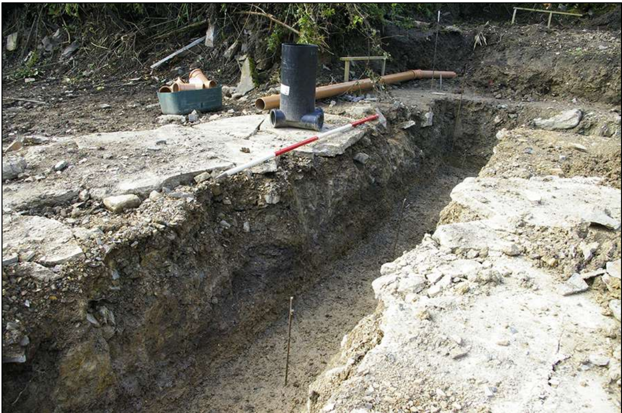
AREA 01 SOUTH-EASTERN FOUNDATION TRENCH, NORTH-WEST FACING SECTION, OBLIQUE; VIEWED FROM THE NORTH-NORTH-WEST (2M SCALE).
