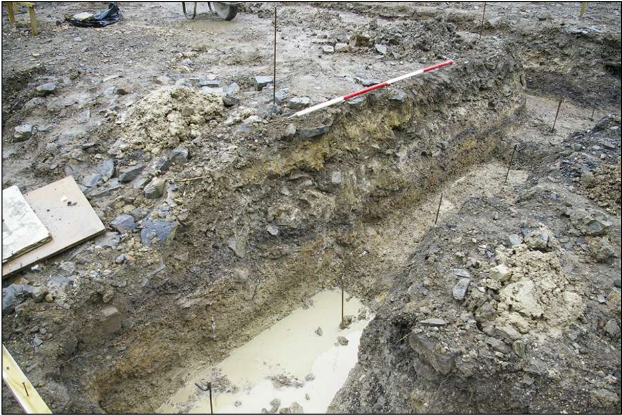
AREA 01 NORTH-EASTERN FOUNDATION TRENCH, NORTH-WEST FACING SECTION, OBLIQUE; VIEWED FROM THE NORTH-NORTH-WEST (2M SCALE).
