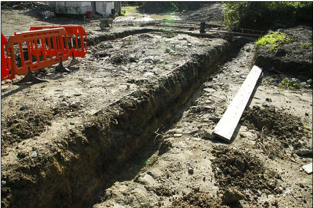
AREA 01 SOUTHERN FOUNDATION TRENCH, SOUTH-WEST FACING SECTION, OBLIQUE; VIEWED FROM THE WEST-SOUTH-WEST (2M SCALE).
