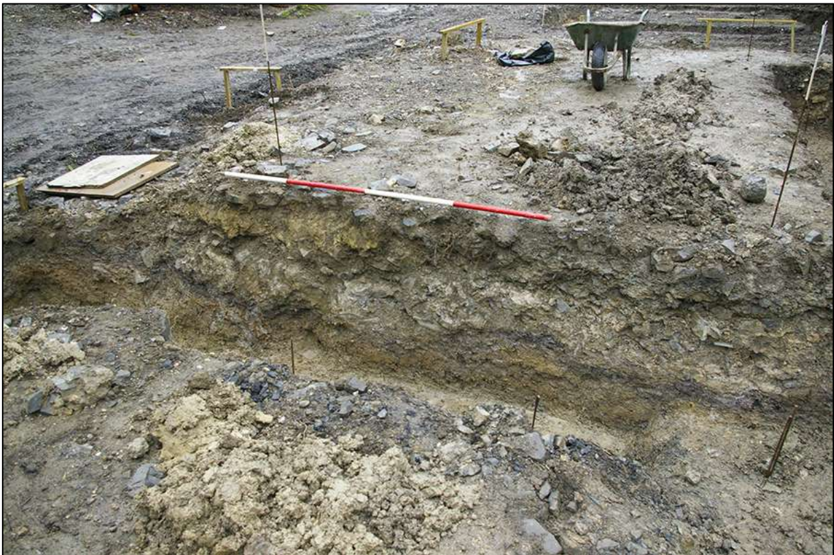
AREA 01 NORTH-EASTERN FOUNDATION TRENCH, NORTH-WEST FACING SECTION, OBLIQUE; VIEWED FROM THE SOUTH-WEST (2M SCALE).
