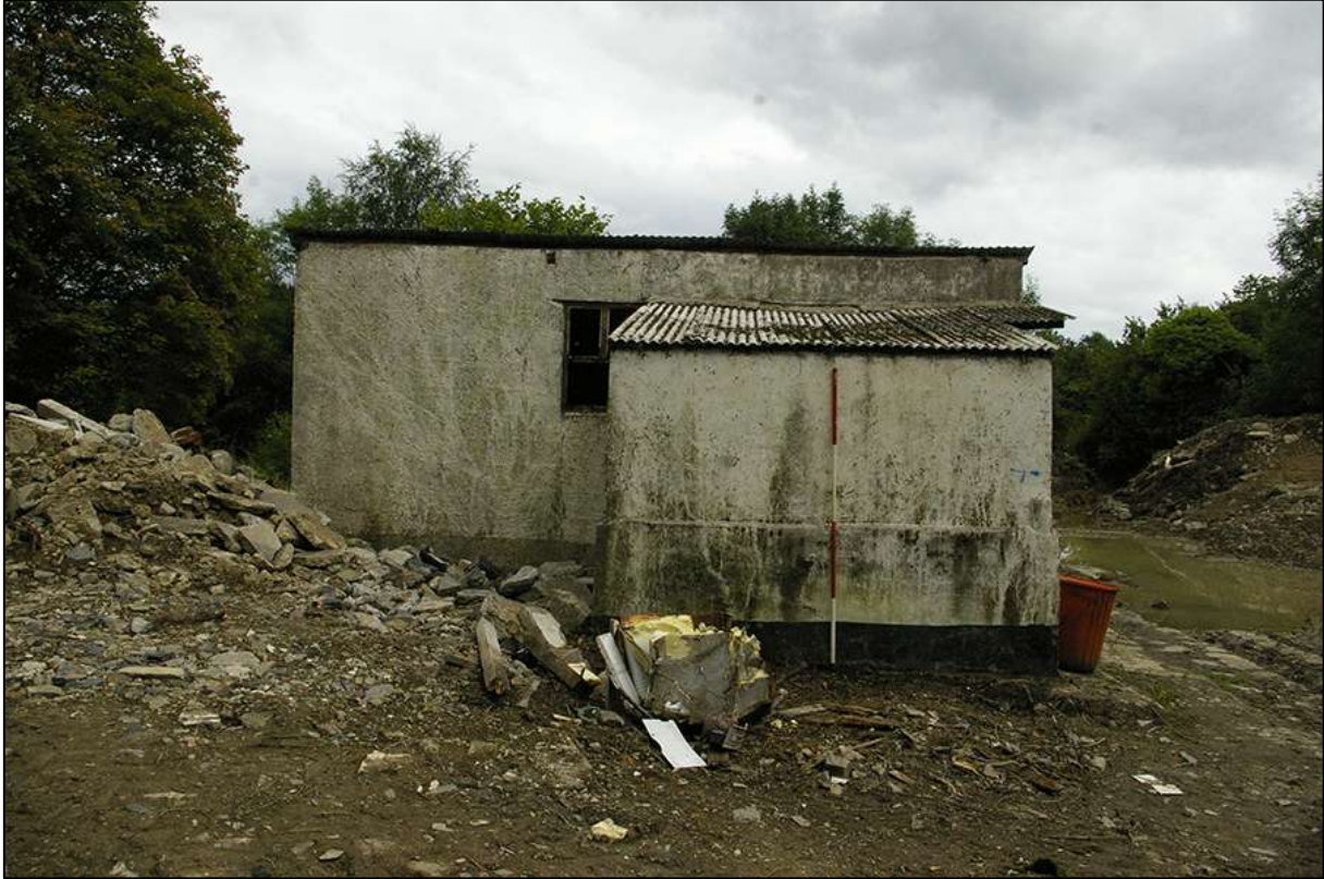
BUILDING 5 EXTERNAL NORTH-WEST ELEVATION (WEST WALL); VIEWED FROM THE NORTH-WEST (2M SCALE).
