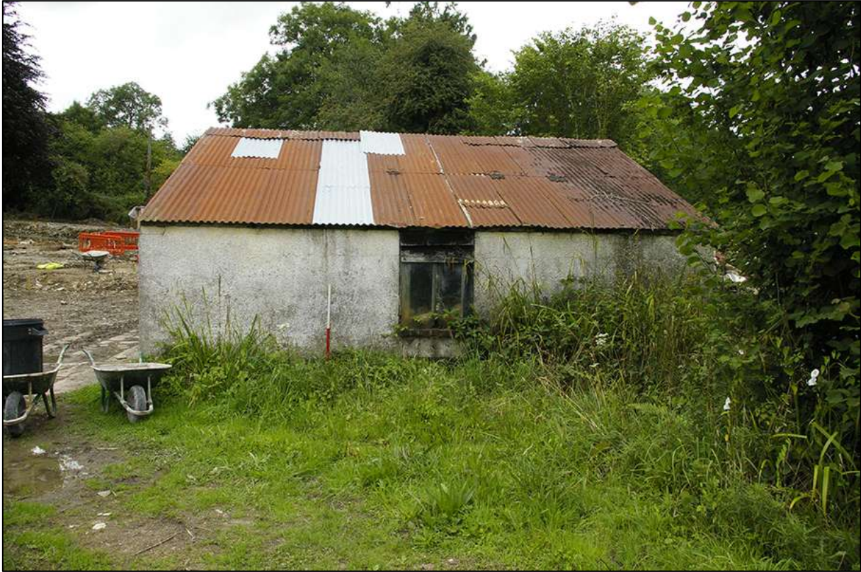
BUILDING 5 EXTERNAL SOUTH-EAST ELEVATION (EAST WALL); VIEWED FROM THE SOUTH-EAST (1M SCALE).
