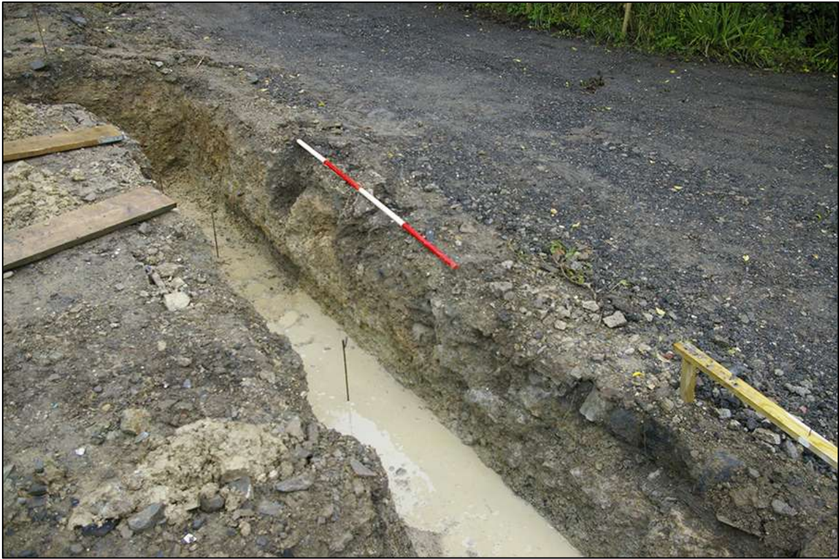
AREA 01 NORTHERN FOUNDATION TRENCH, SOUTH-WEST FACING SECTION, OBLIQUE; VIEWED FROM THE SOUTH-EAST (2M SCALE).
