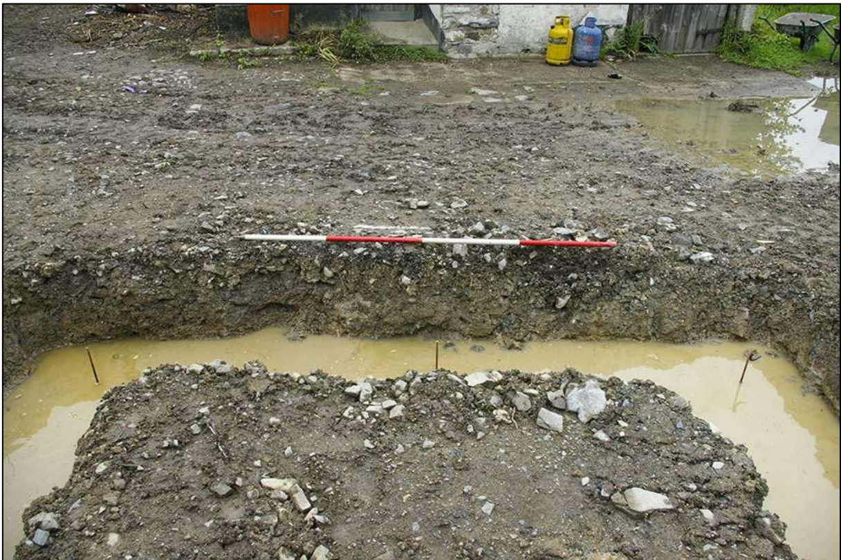
AREA 02 NORTHERN FOUNDATION TRENCH, SOUTH-WEST FACING SECTION; VIEWED FROM THE SOUTH-WEST (2M SCALE).
