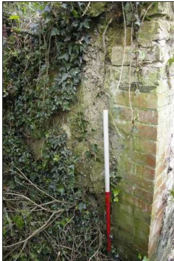
WALL 4 DETAIL OF BRICK REPAIRS AT EASTERN END; VIEWED FROM THE EAST (1M SCALE).
