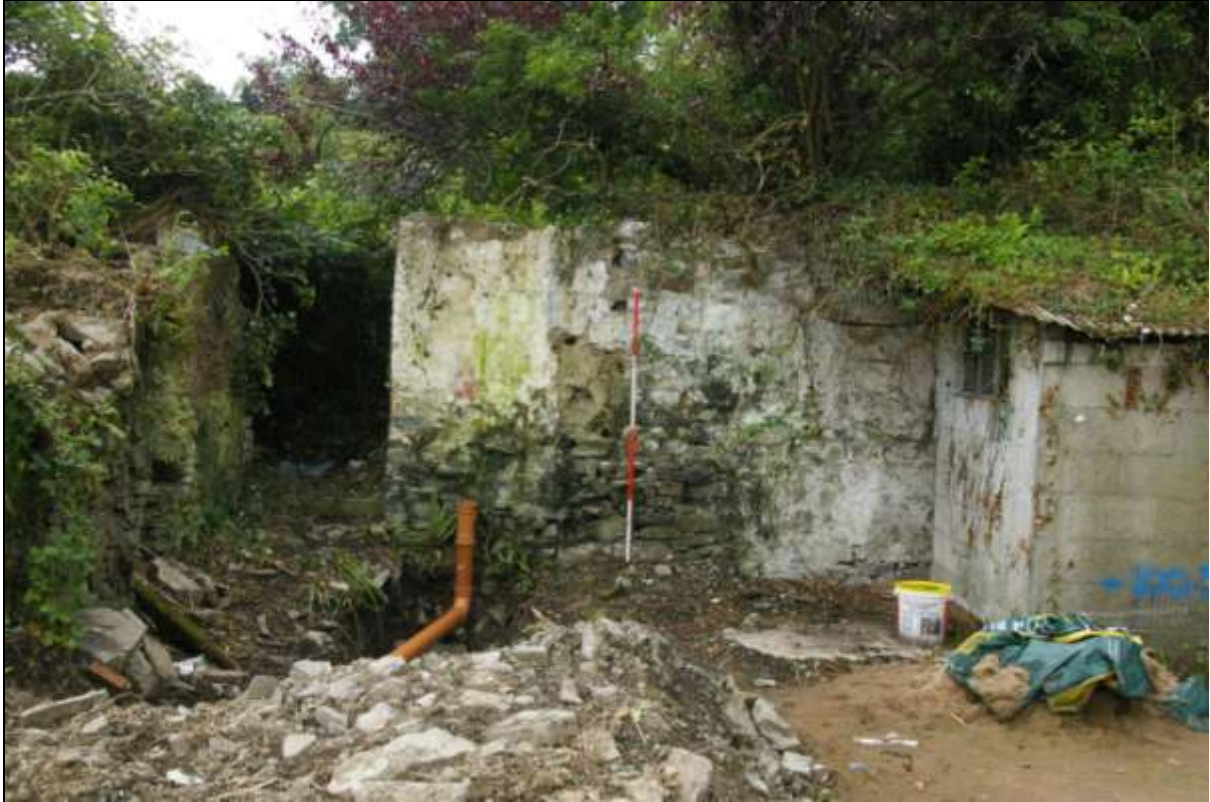
FIGURE 9: WALL 4 NORTH-EAST ELEVATION, EAST END, SHOWING SCARRING OF REMOVED WALL; VIEWED FROM THE NORTH-EAST (2M SCALE).
