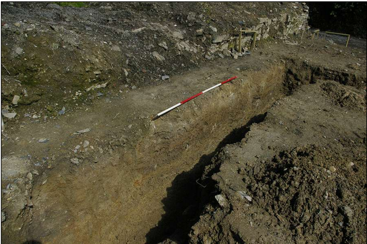
AREA 01 SOUTH-WESTERN FOUNDATION TRENCH, SOUTH-EAST FACING SECTION, OBLIQUE; VIEWED FROM THE SOUTH-SOUTH-EAST (2M SCALE).
