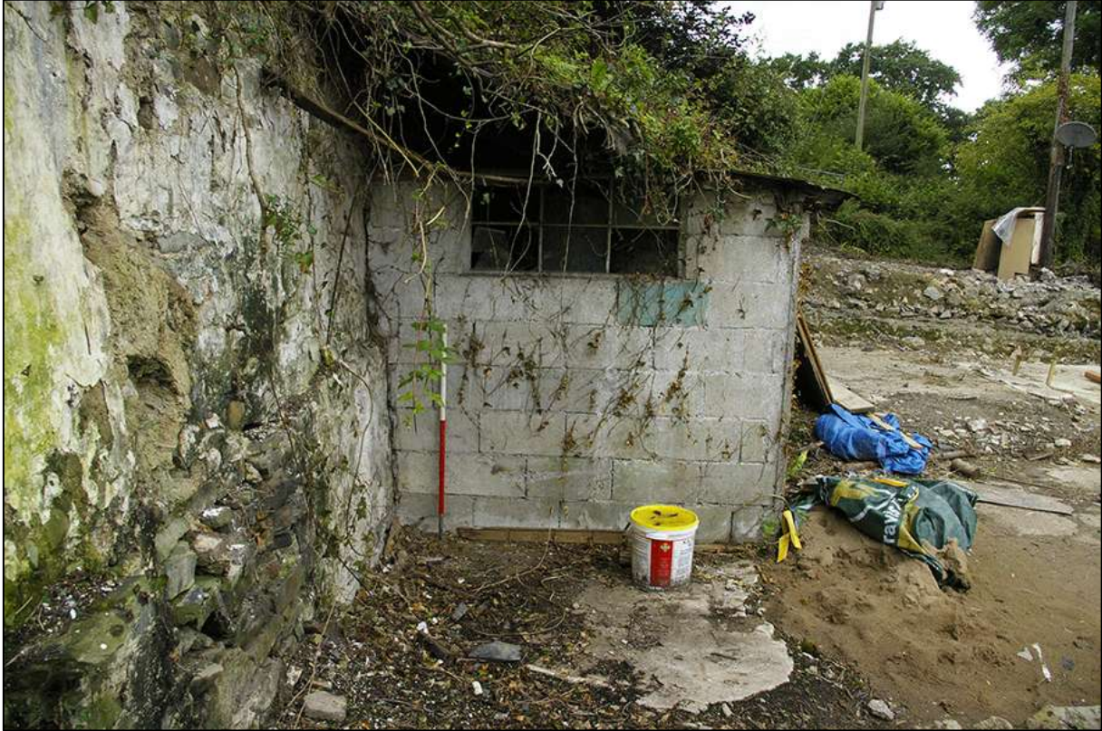
BUILDING 2 EXTERNAL SOUTH-EAST ELEVATION (EAST WALL); VIEWED FROM THE SOUTH-EAST (1M SCALE).
