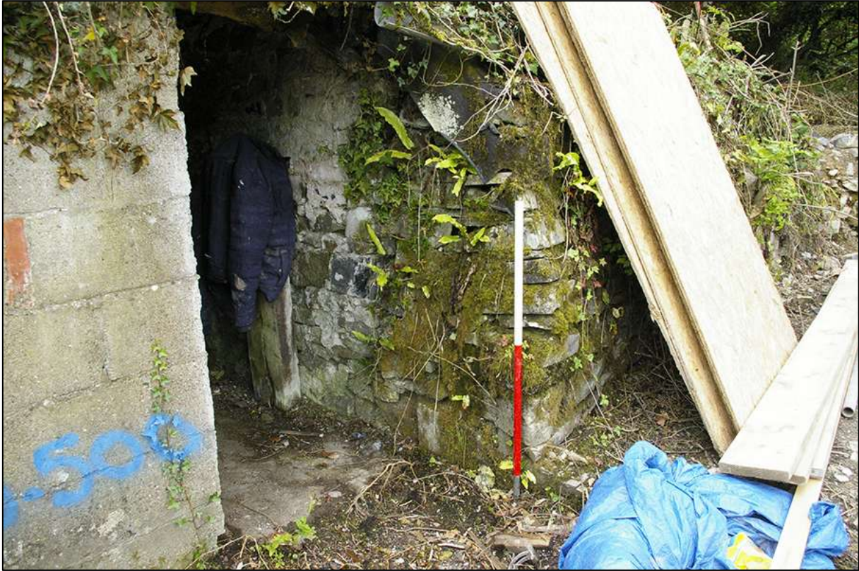
WALL 3, DETAIL OF JOIN WITH WALL 4; VIEWED FROM THE EAST (1M SCALE).
