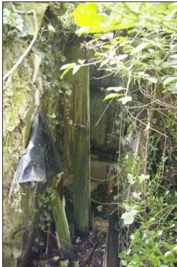
BUILDING 4 EXTERNAL NORTH-WEST ELEVATION (WEST WALL); VIEWED FROM THE NORTH-WEST (NO SCALE).
