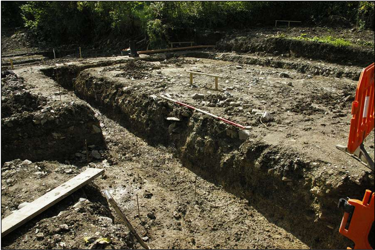
AREA 01 MIDDLE FOUNDATION TRENCH, NORTH-EAST FACING SECTION, EAST END, OBLIQUE; VIEWED FROM THE NORTH-WEST (2M SCALE).
