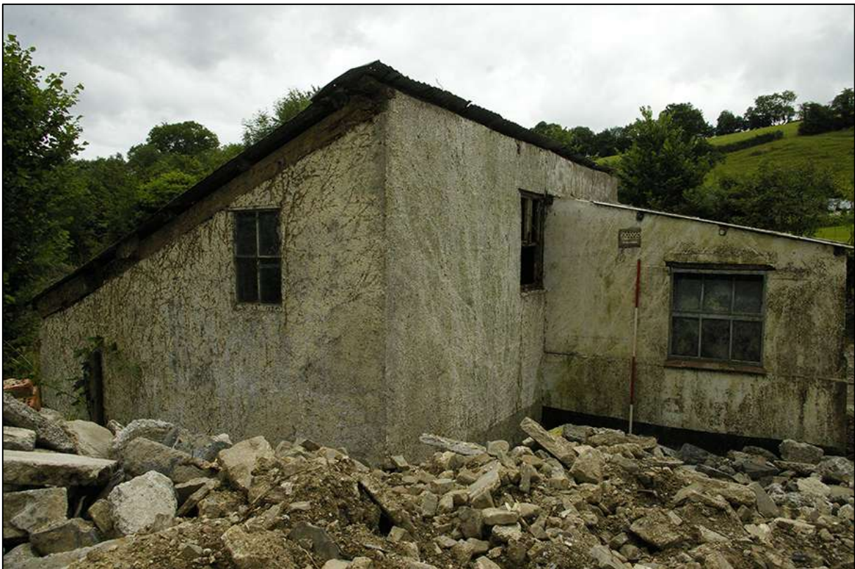
BUILDING 5 EXTERNAL NORTH-EAST AND NORTH-WEST ELEVATIONS (NORTH & WEST WALLS); VIEWED FROM THE NORTH (2M SCALE).
