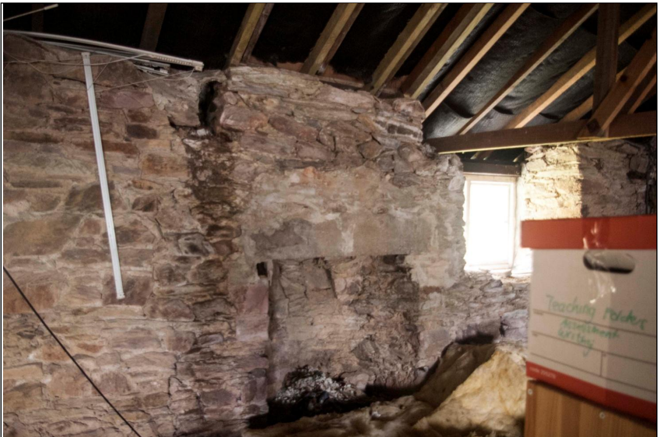
View of the stack and forced fireplace, with rounded hearth, within the second floor of the east range, of c.1800 date; from the north-west.
