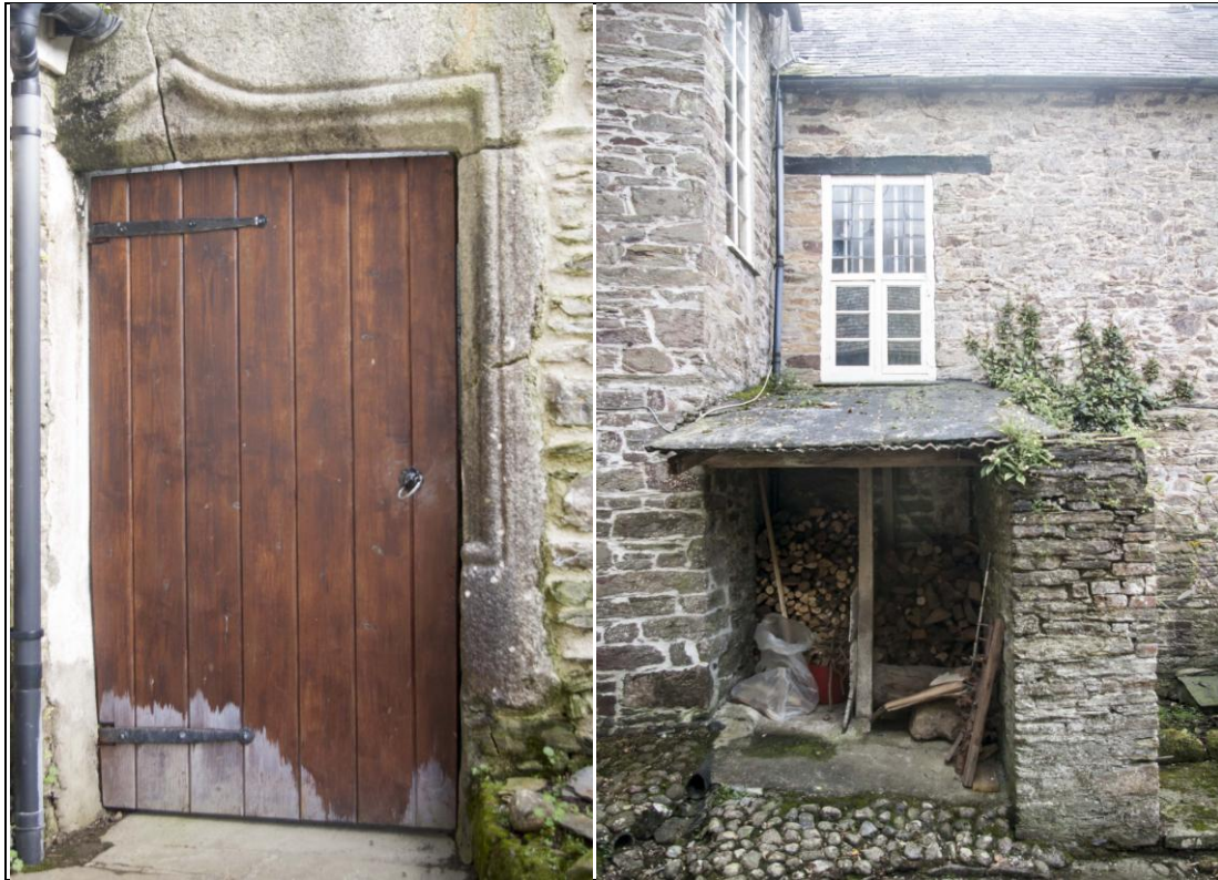
Left: Fireplace surround, 17 th century, in east garden wall, repurposed as a doorway; from the west-south-west. Right: Eastern stair turret, serving south range, abutted by modern log store roof, with 19 th century wall of demolished lean-to to west (right); from the north.
