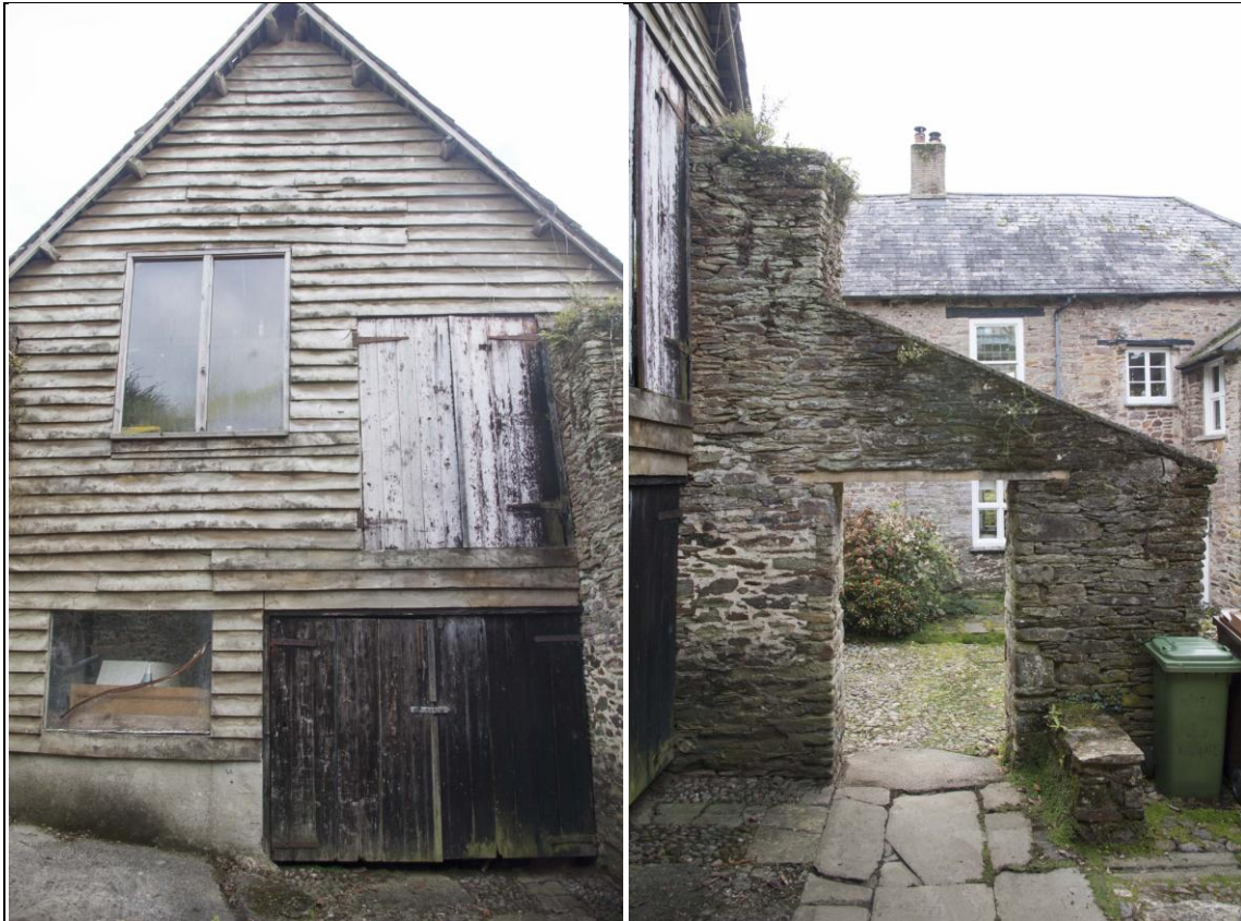
Left: The 1960s timber clad and framed west wall of the standing remains of the north range; from the west. Right: The original central door of the north range, within a surviving section of wall; from the north.
