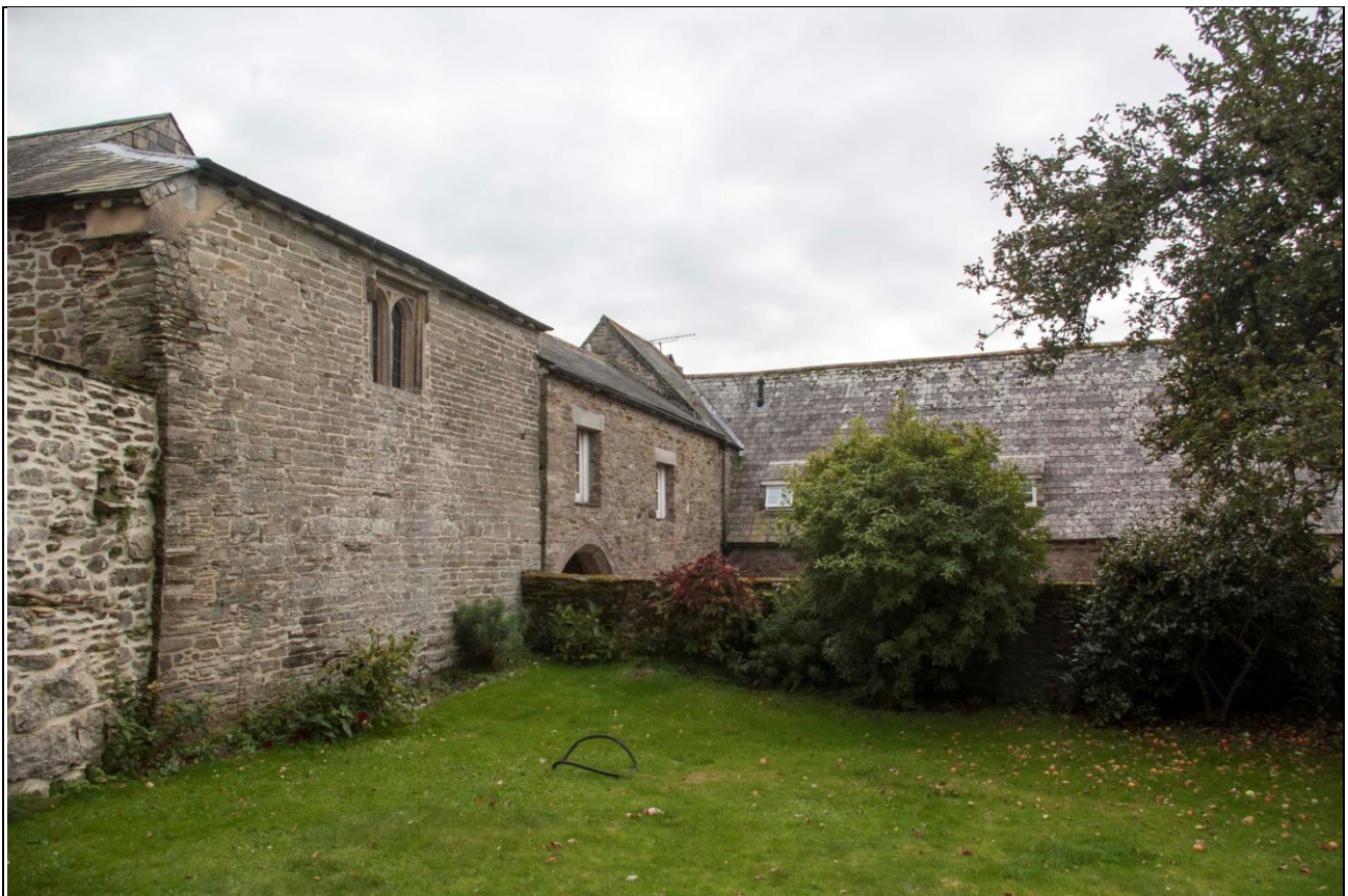
The stables and 'gatehouse' range to the south-east of Old Trine, exhibiting some very high quality fragmentary building remains, with ashlar stonework; from the north-north-west.
