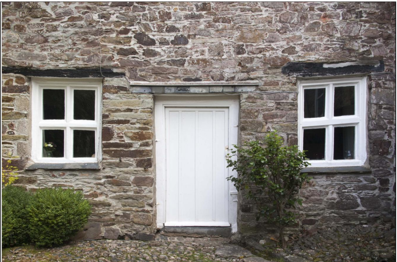
View of the central door and flanking windows, of 17 th century date, in the ground floor of the east range, facing into the courtyard; from the west.
