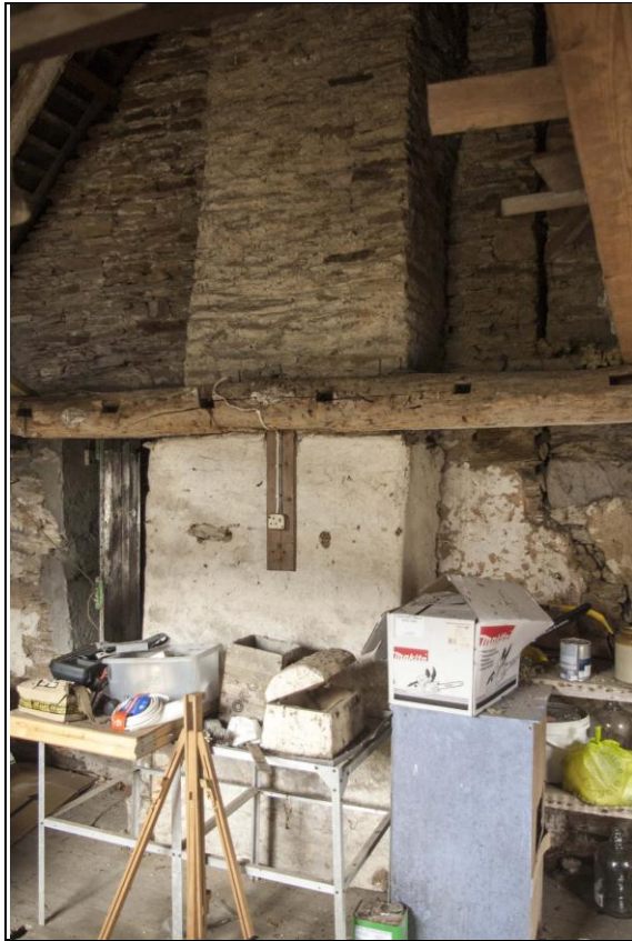
Wider view of the series of stacks and forced door in the east wall of the north range; from the south-west. 3
