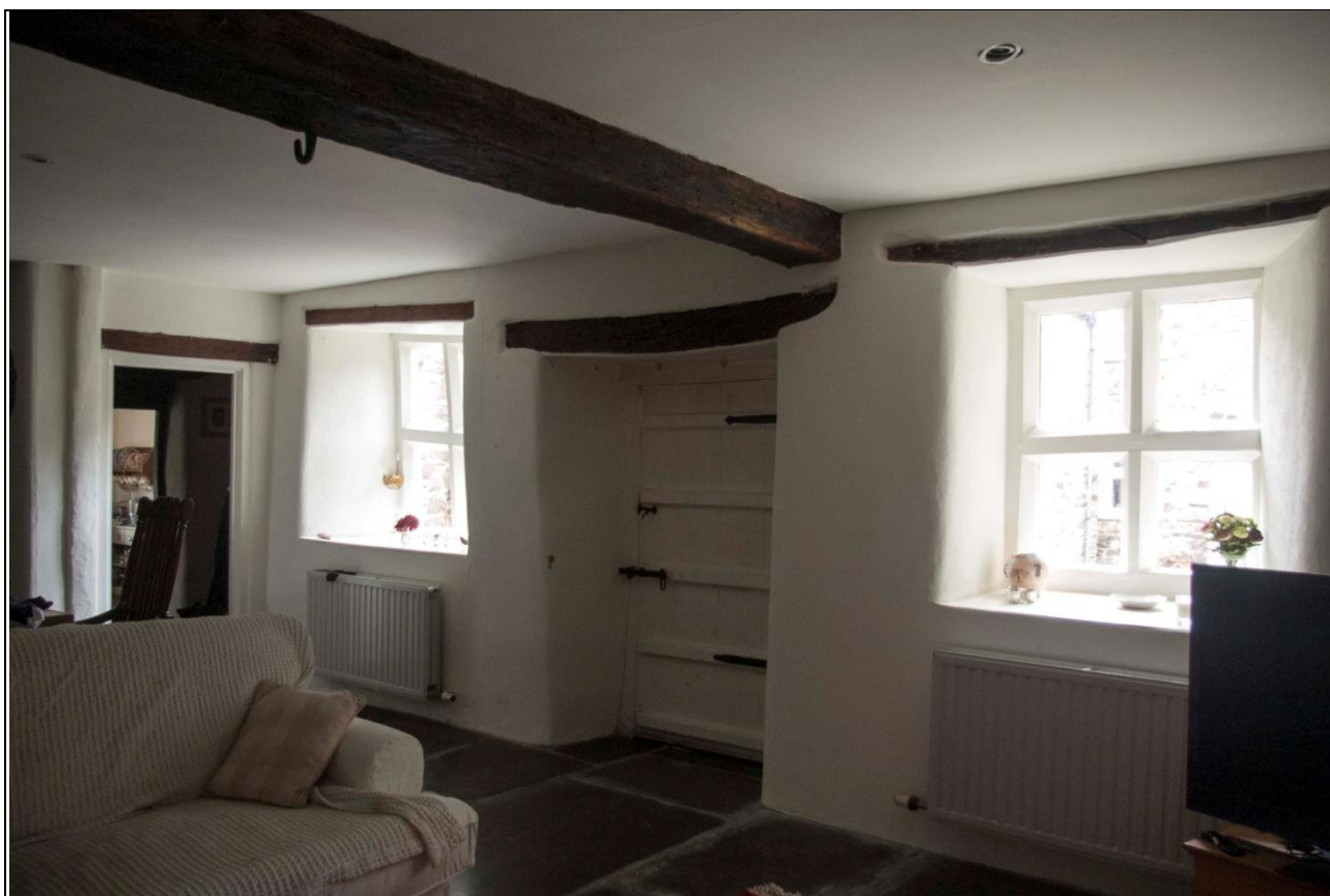
View of the west wall of the east range, at ground floor level, interior face, showing the door and flanking windows and massive first floor ceiling beam; from the north-east.
