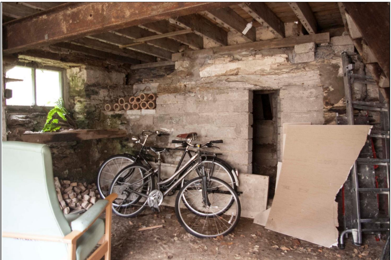
The series of stack and oven structures to the east end of the north range, showing significant intervention in the 1960s; from the south-west.
