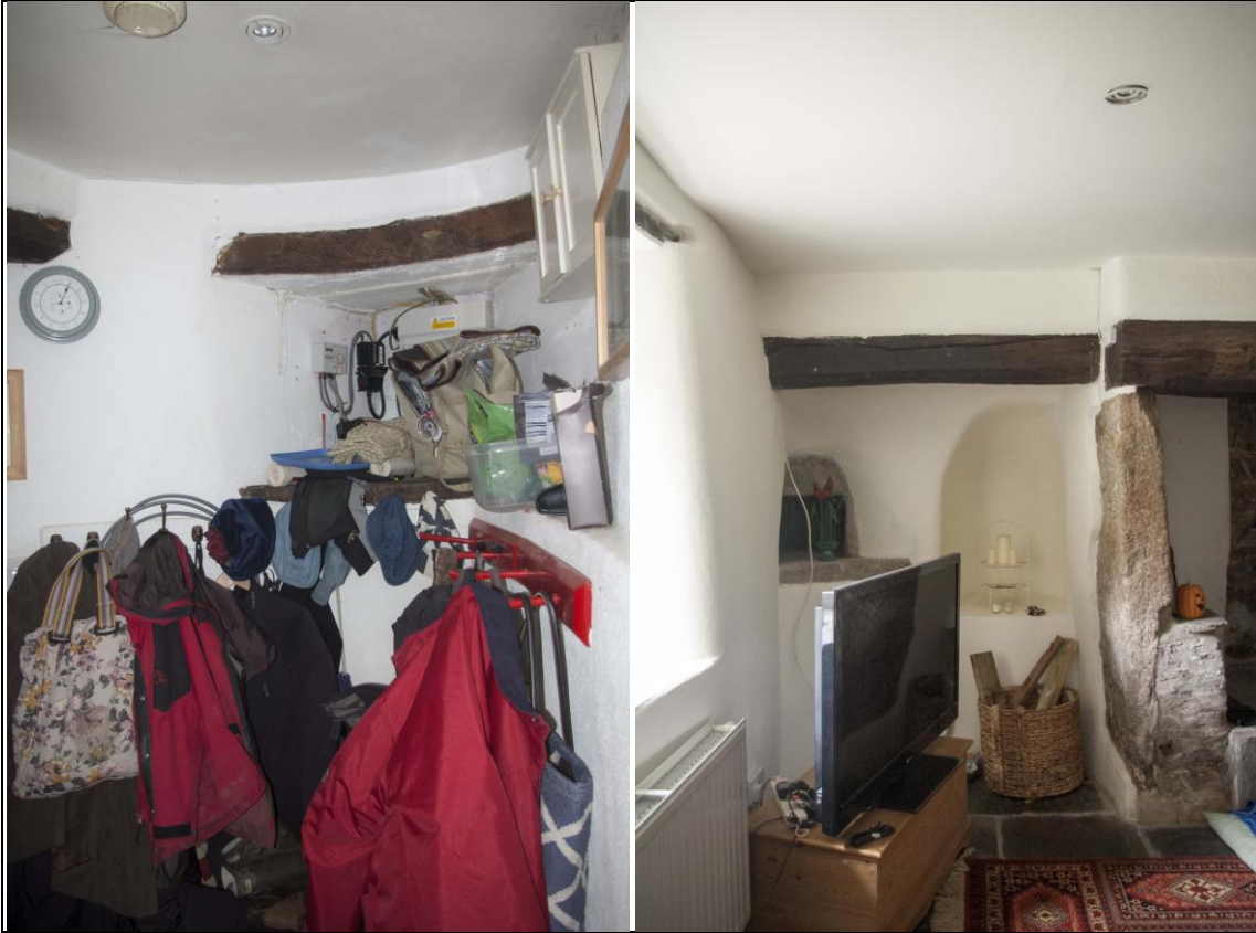
Left: View of the blocked window at ground floor level in the east stair turret; from the north-east. Right: Detailed view of oven and smoke chamber to the north wall of the east range; from the south.
