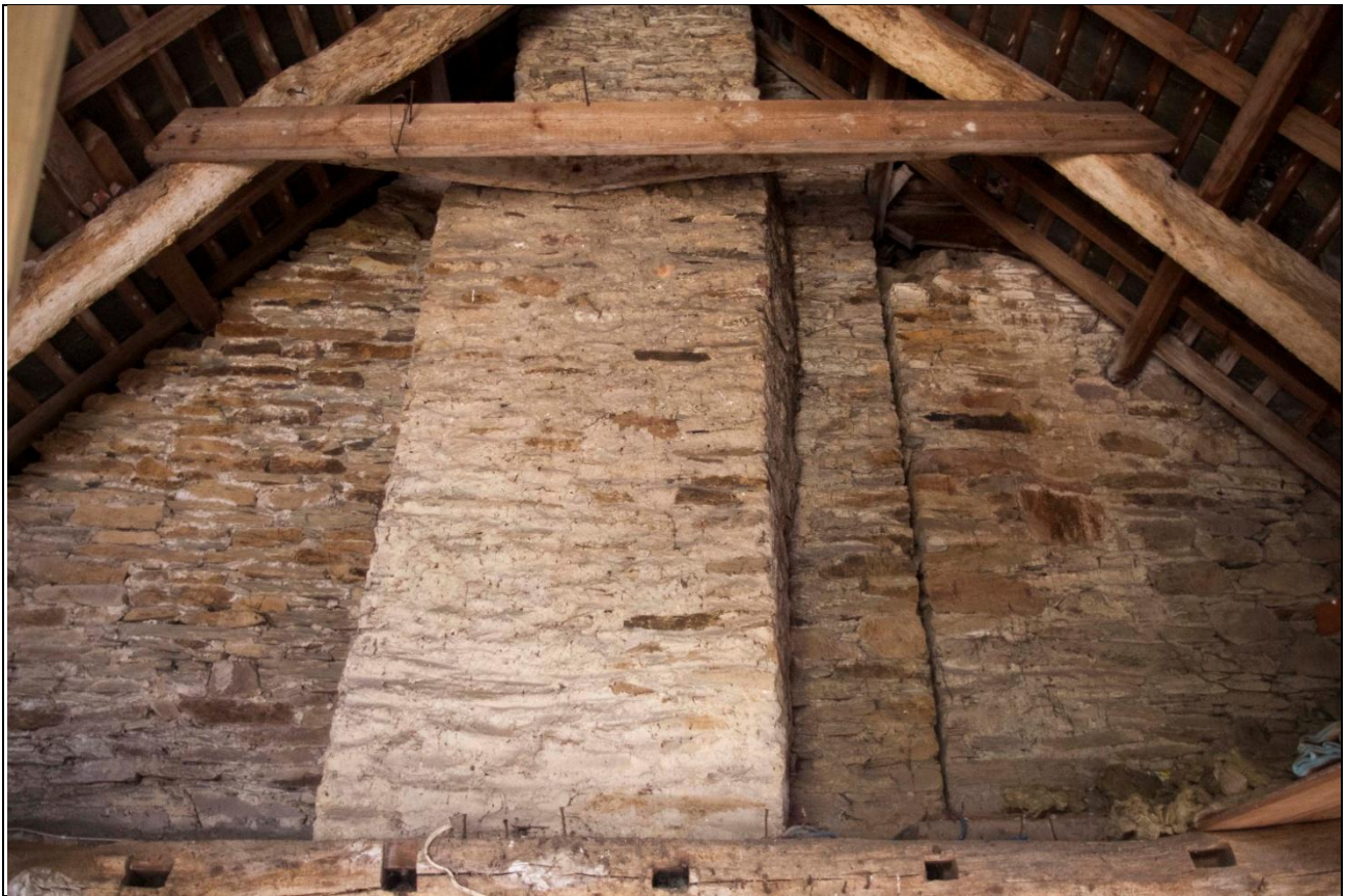
The two clear phases of chimney stack, within the roof of the north range, at the east end; from the west.
