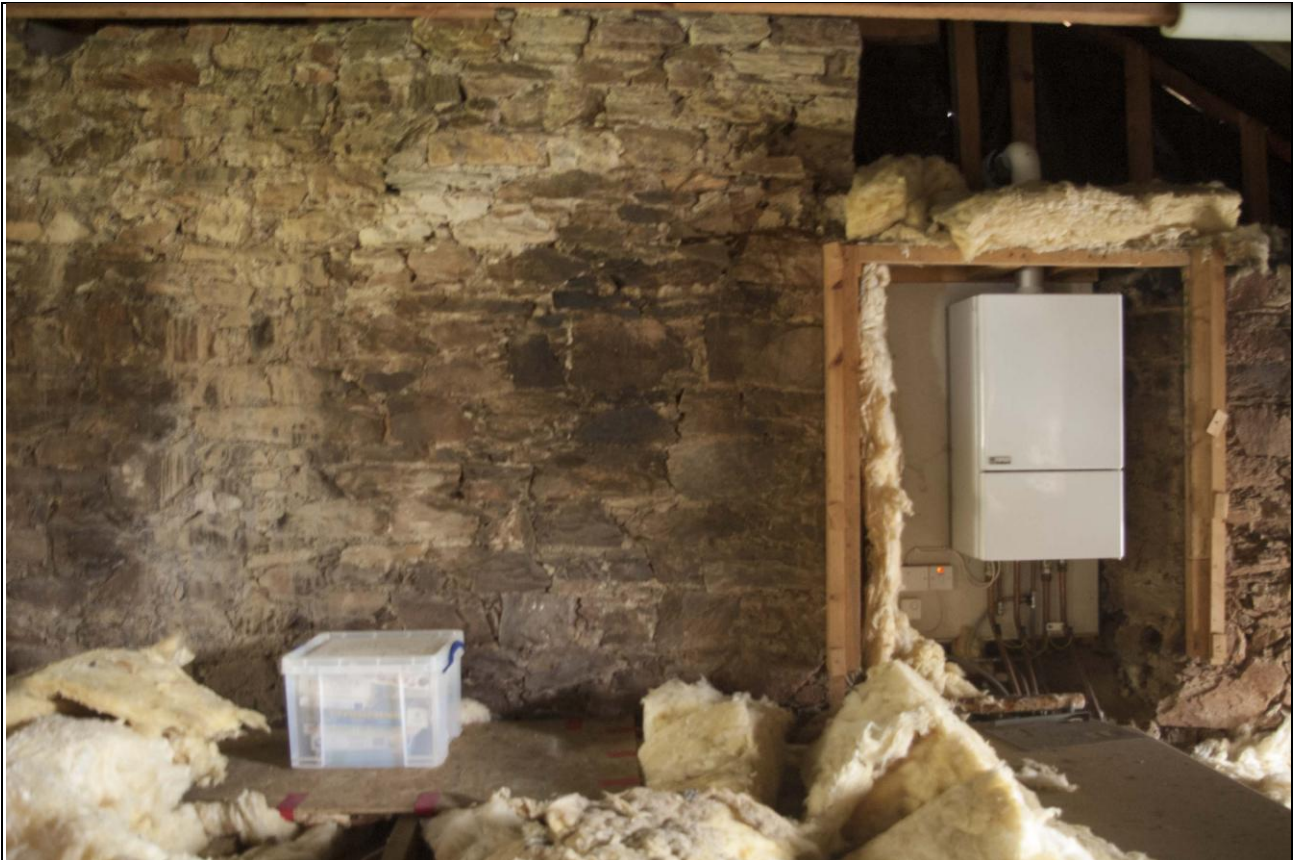
View of the section of medieval walling to the south end of the east range, showing large blocked window, with dressed quoins, now blocked by boiler; from the north.
