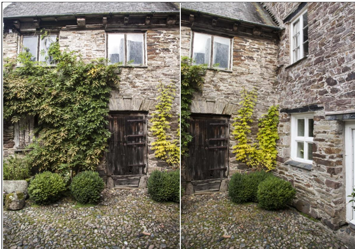
Left: Detail of front elevation of north range, showing dressed details and overhanging decorative eaves structure; from the south.
