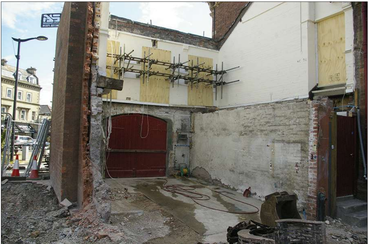
4. GENERAL SITE VIEW SHOWING DEMOLITION WORKS WITH EXISTING MUSEUM BUILDING WALL {522}; FROM THE SOUTH-WEST (NO SCALE).
