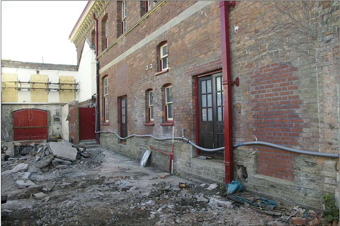
3. GENERAL SITE VIEW SHOWING DEMOLITION WORKS WITH EXISTING MUSEUM BUILDING {400}; FROM THE SOUTH-WEST (2M SCALE).
