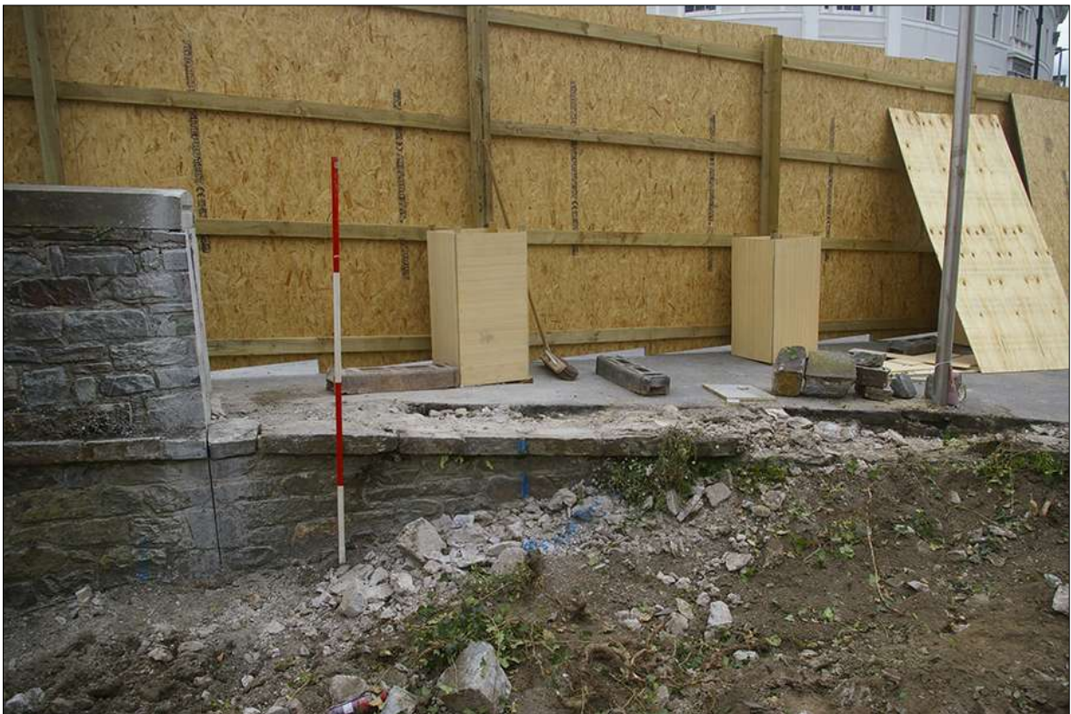
30. AREA 06, DETAIL OF MODERN ROAD BRIDGE WALL; FROM THE SOUTH (2M SCALE).
