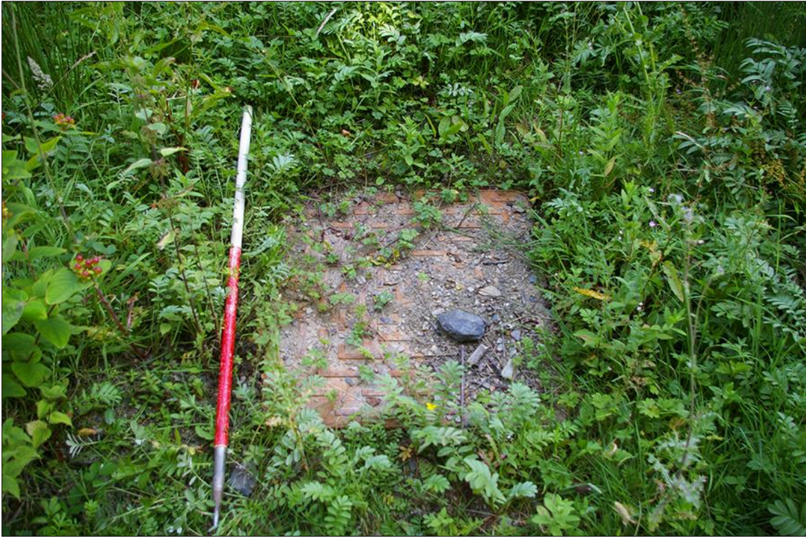
37. DETAIL OF THE MODERN MANHOLE COVER AT THE WESTERN EDGE OF F7, INDICATING DRAINAGE LINKED TO THAT IDENTIFIED WITHIN F6; VIEWED FROM THE WEST (1M SCALE).
