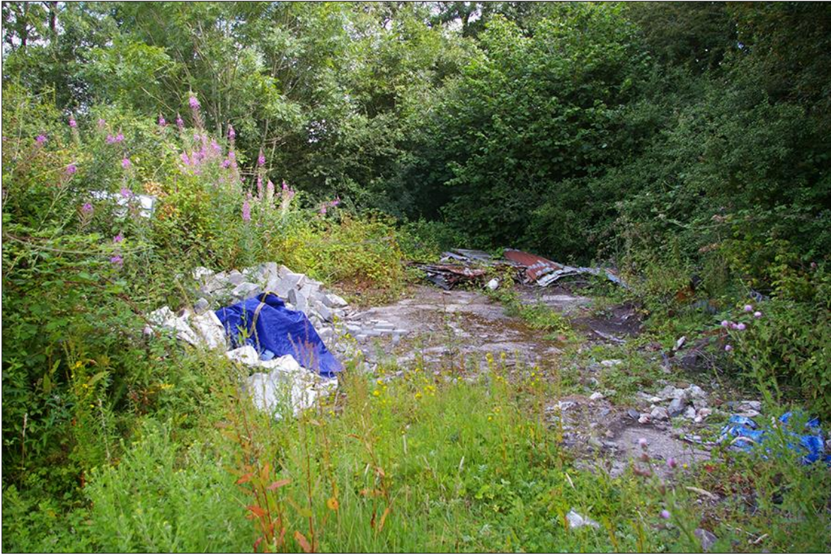
23. DETAIL OF THE CONCRETE SURFACE AND DEMOLISHED STRUCTURE AT THE EASTERN EDGE OF F5; VIEWED FROM THE SOUTH.
