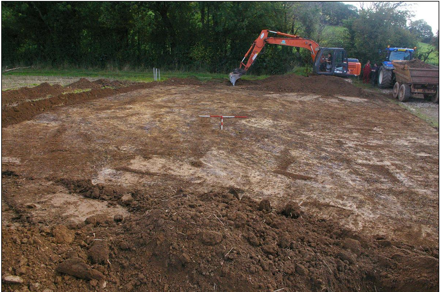
Figure 2: The footprint of the manure store, stripped to the natural (104); viewed from the west (scales 2m).
