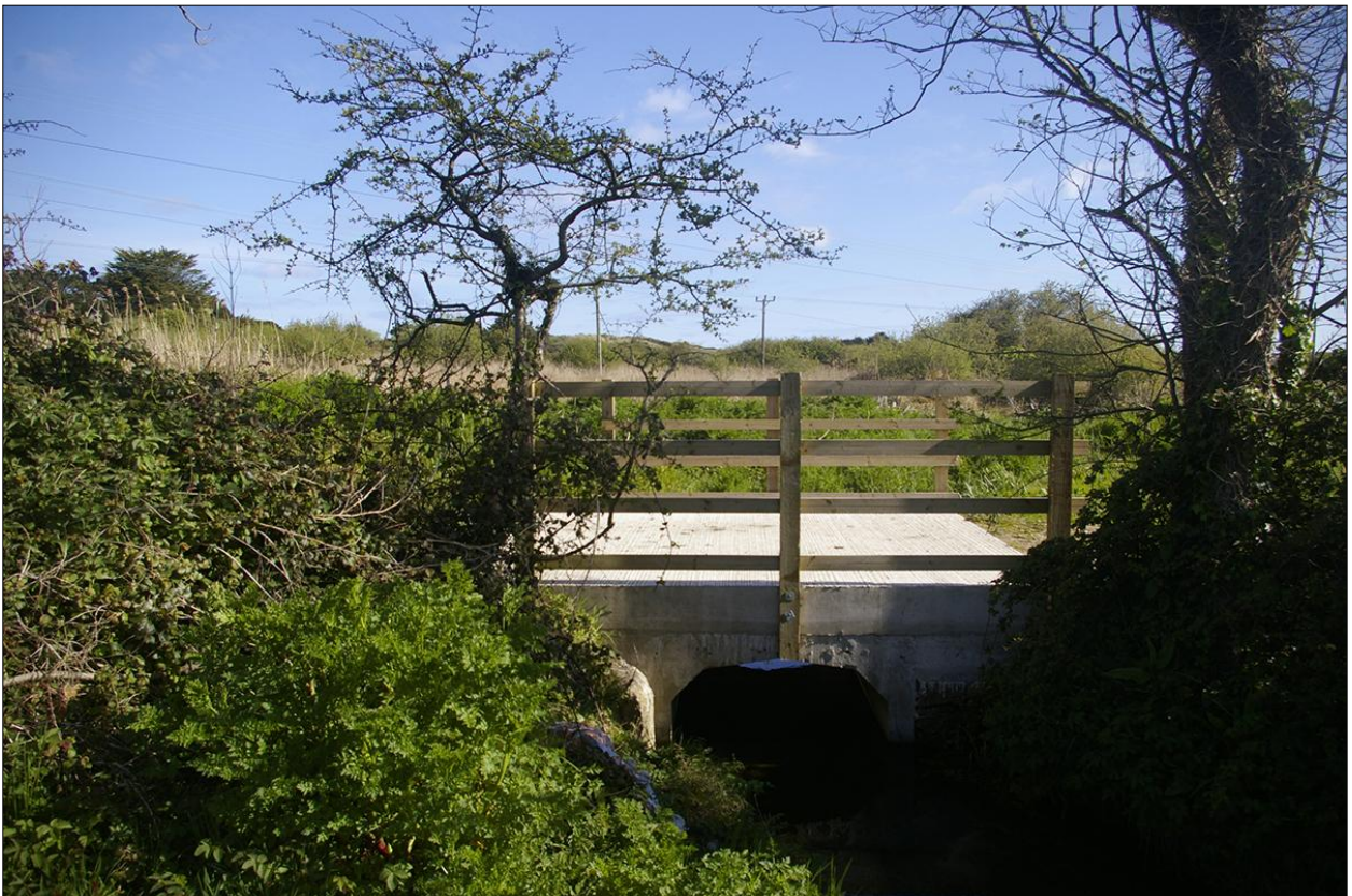
The new concrete bridge over the leat, just north of the site; viewed from the south, looking north.
