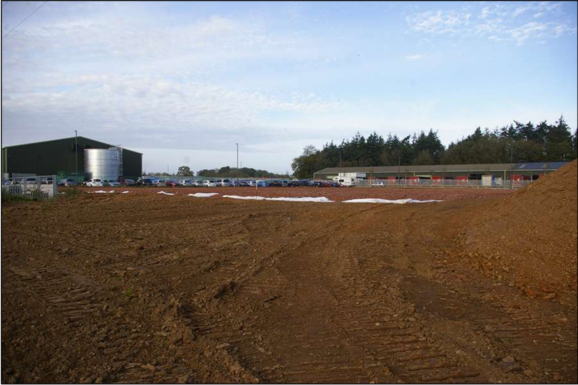
GENERAL SITE VIEW SHOWING STONED AREA FROM SOUTH-EAST CORNER; VIEWED FROM THE SOUTH-EAST (1M SCALE).
