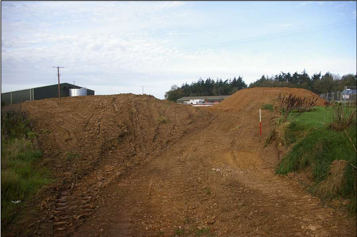
GENERAL SITE VIEW SHOWING BUNDS TO THE STONED AREA; VIEWED FROM THE SOUTH-EAST (1M SCALE).
