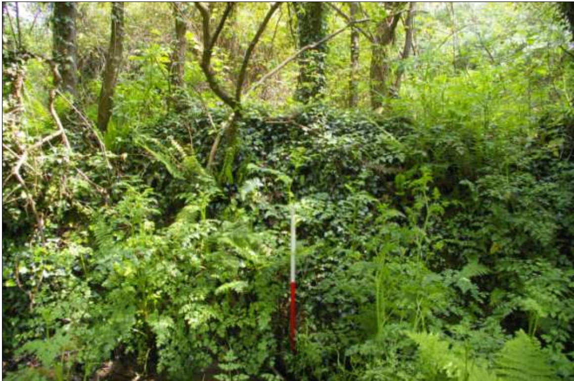
16. DETAIL OF THE EARTH BANK FORMING THE WEST BOUNDARY OF FIELD 3 (FROM FIELD 2) SHOWING HOW OVERGROWN IT HAS BECOME; VIEWED FROM THE NORTH-WEST, LOOKING SOUTH-EAST (1M SCALE).
