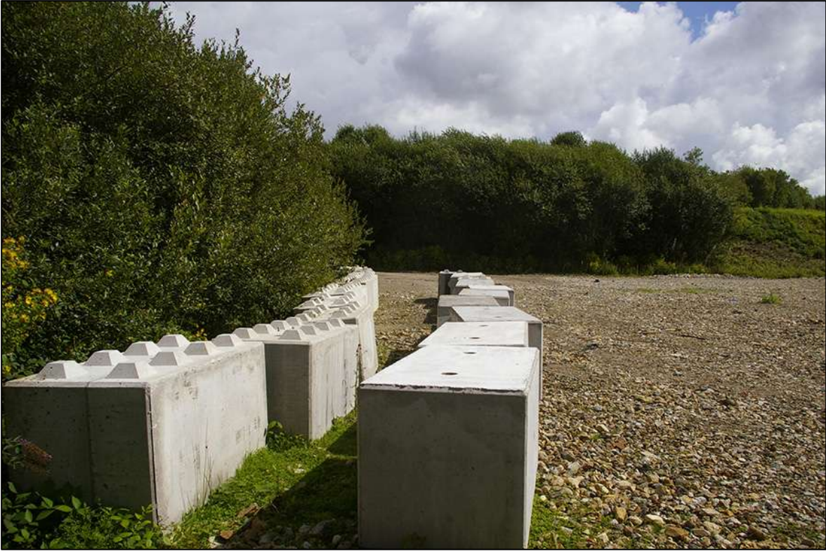
VIEW FROM THE WEST CORNER OF THE SITE; LOOKING NORTH-EAST (NO SCALE).
