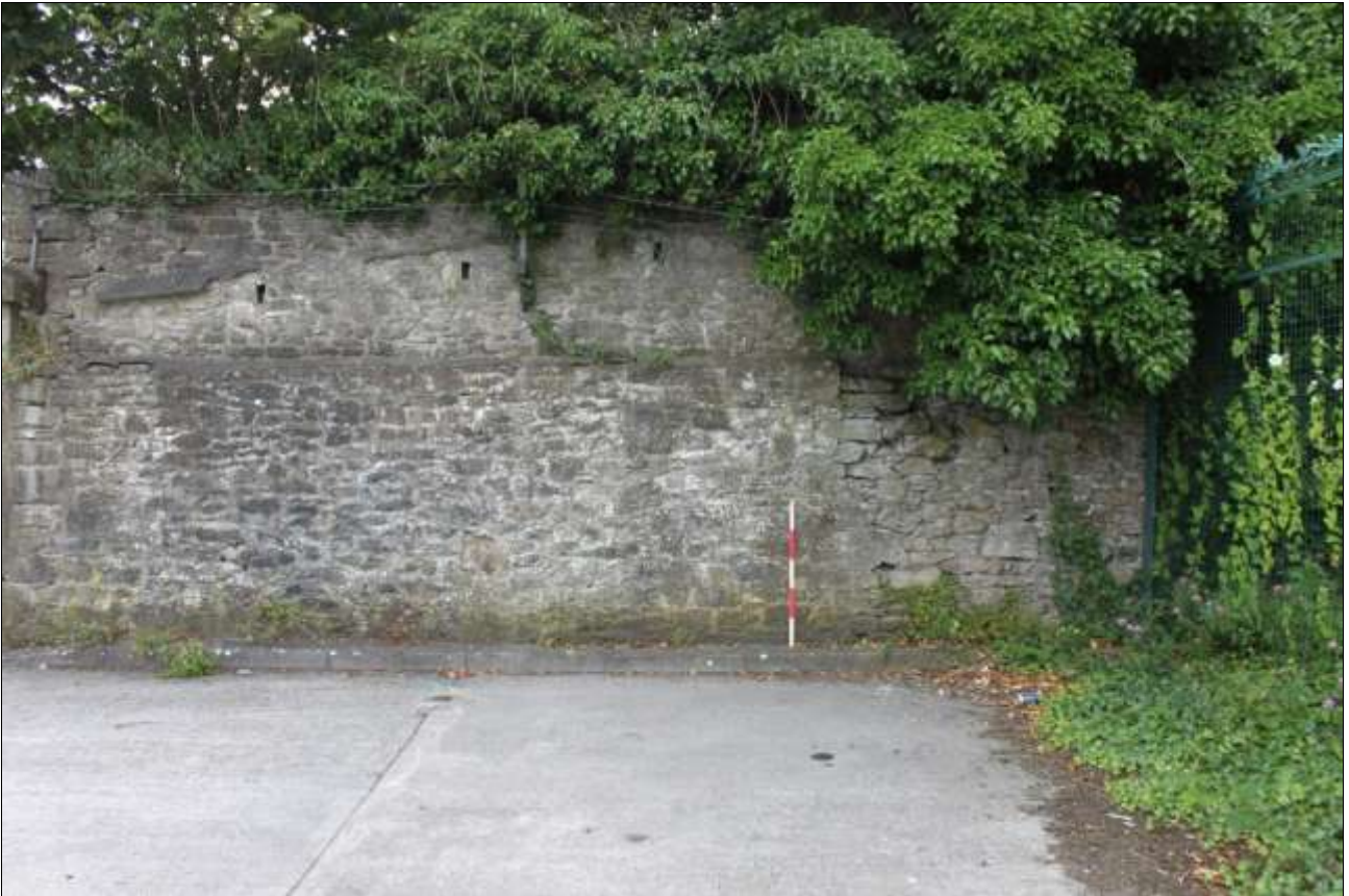
HISTORIC BOUNDARY WALL, WITH BUILDING SCAR, TO THE EAST OF THE WESTERN PARKING AREA, VIEWED FROM THE WEST (1M SCALE).
