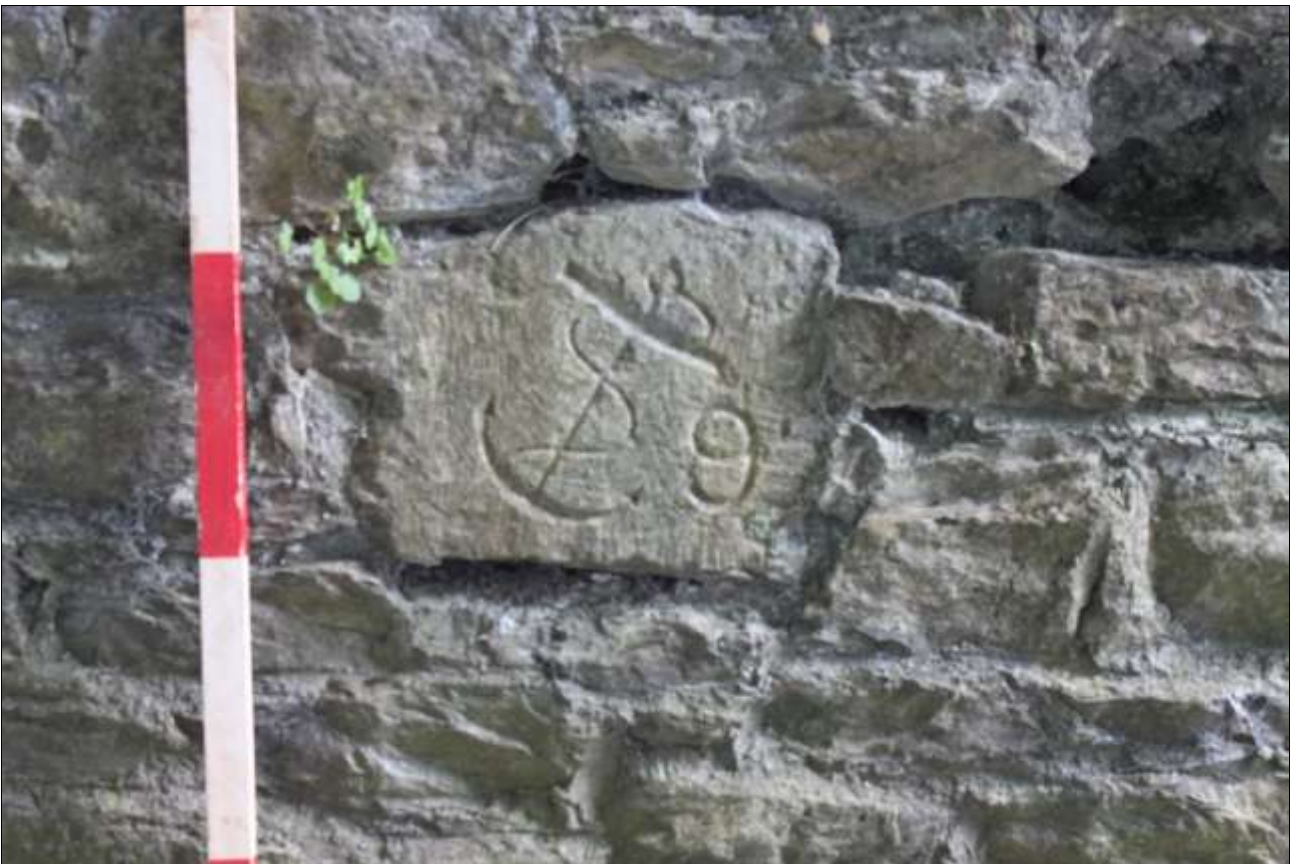
BOUNDARY STONE 9 IN SOUTHERN BOUNDARY WALL, VIEWED FROM THE SOUTH (1M SCALE).
