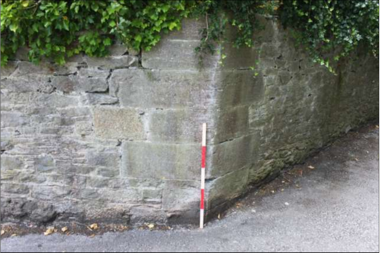
SHOT OF THE SOUTH-WEST CORNER OF THE BOUNDARY WALL, INCLUDING BOUNDARY STONE 8, VIEWED FROM THE SOUTH-WEST (1M SCALE).
