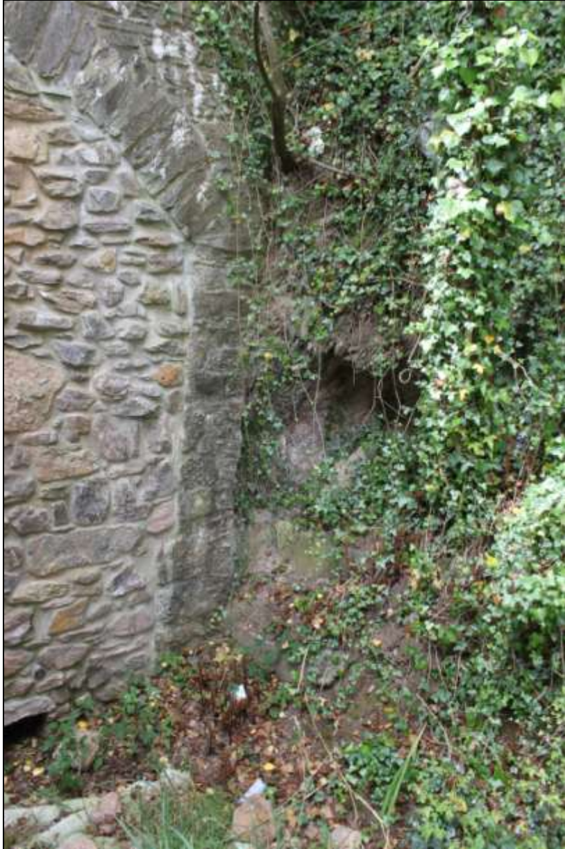
SHOT OF THE LIMESTONE BEDROCK SIDES EVIDENT IN THE TUNNEL CUTTING, VIEWED FROM THE NORTH-EAST.
