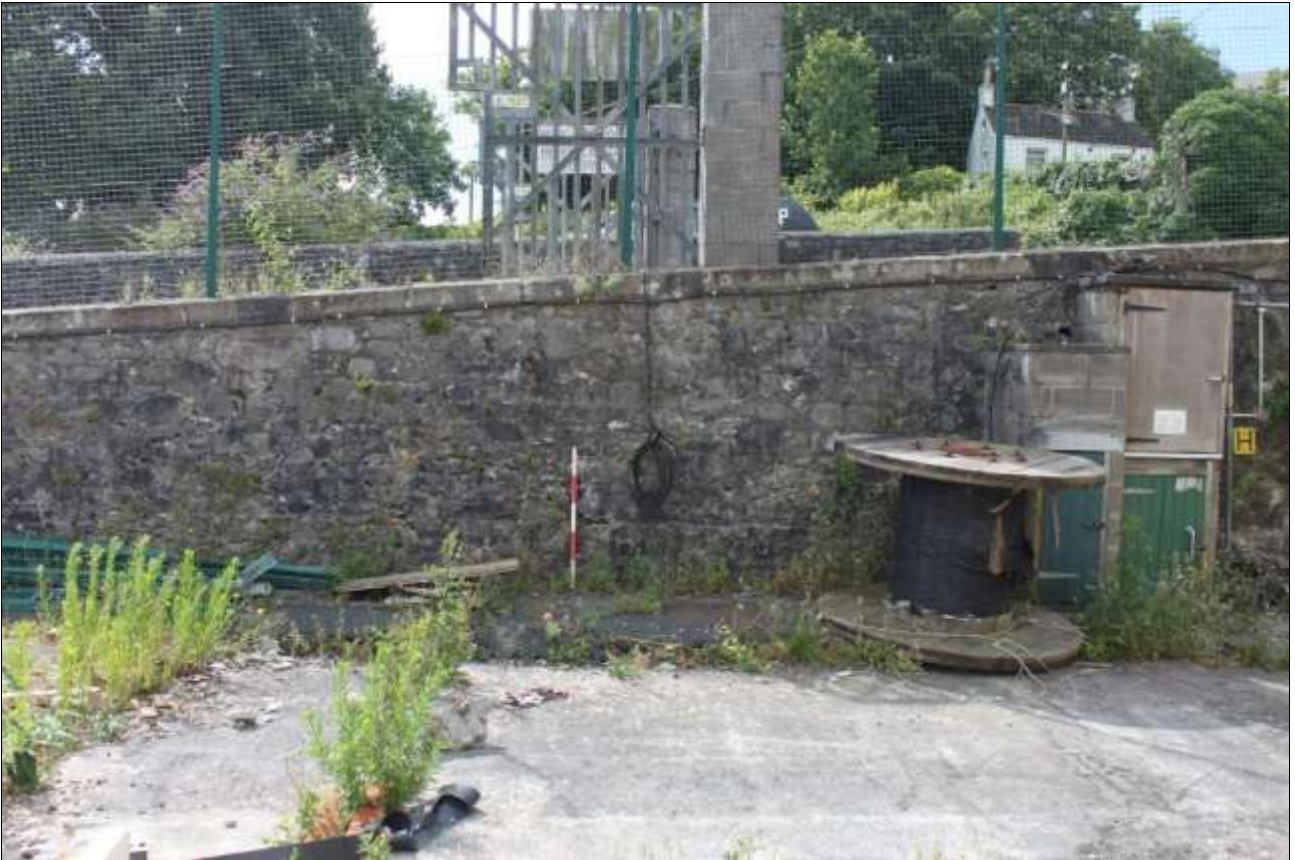
AS ABOVE, VIEWED FROM THE NORTH (1M SCALE). THE PUBLIC CAR PARK AND NO.4 KELLY COTTAGES CAN BE SEEN IN THE BACKGROUND.
