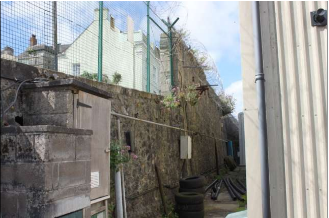
RETAINING WALL ALONG THE NORTHERN EDGE OF THE SITE, FLANKING BORINGDON ROAD, VIEWED FROM THE NORTH-EAST.
