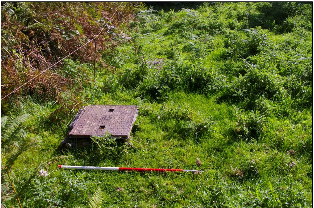
PHOTOGRAPH 16: VIEW OF MANHOLE COVERS ALONG EASTERN BOUNDARY OF FIELD 2; TAKEN FACING SOUTH (1M SCALE).
