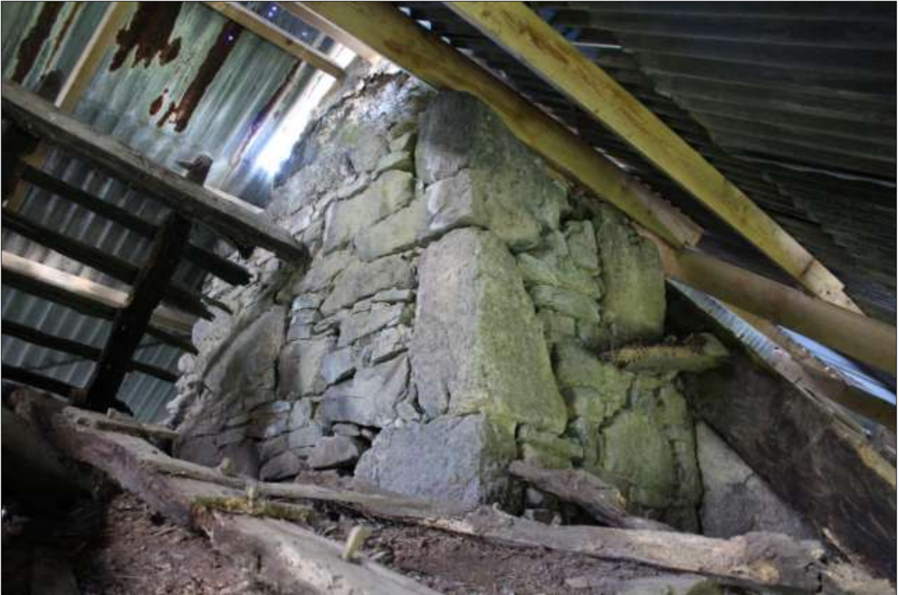
R5, THE BASE OF THE STACK WITHIN THE ROOF SPACE; VIEWED FROM THE SOUTH.
