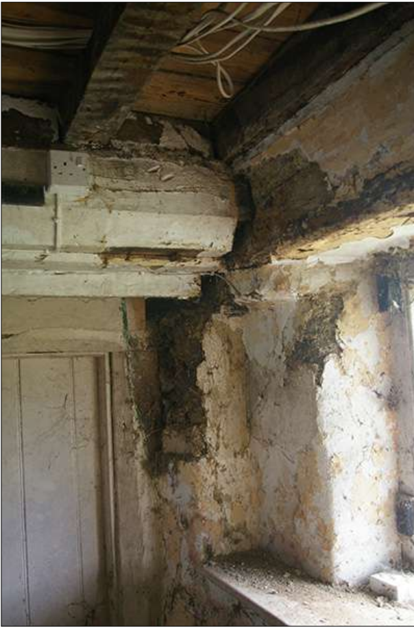
SOUTH ANGLE OF R1, SHOWING THE BEAM SOCKETED INTO THE WINDOW LINTEL; VIEWED FROM THE WEST.
