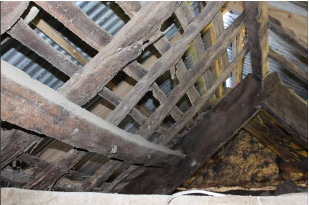
R4, DETAIL OF THE PEGGED PURLIN ON THE UPPER NORTH-EAST PITCH; VIEWED FROM THE NORTH-WEST.
