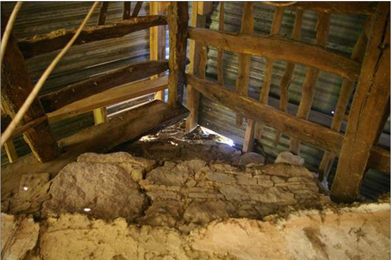
R4, THE APEX OF THE ROOF ABOVE THE STACK; VIEWED FROM THE SOUTH-EAST.
