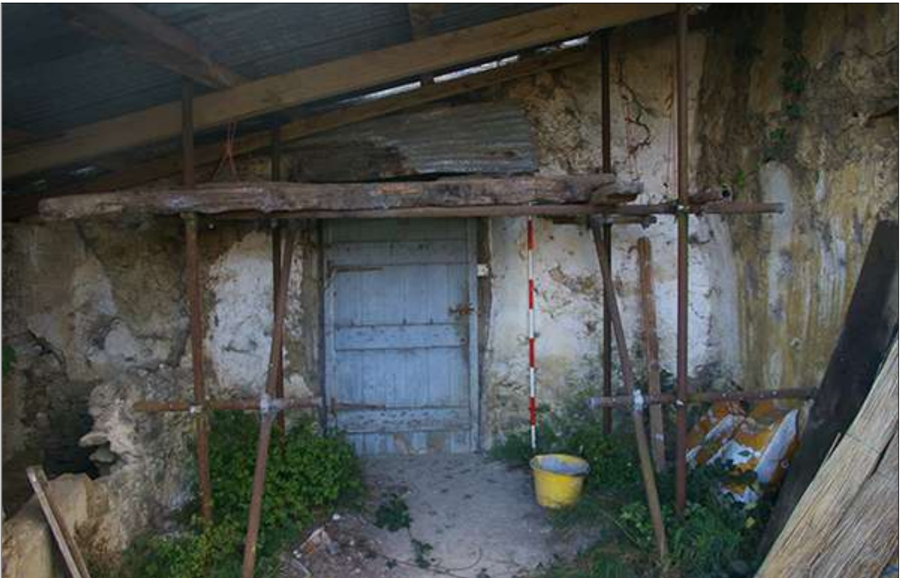
VIEW INTO THE SURVIVING SECTION OF HISTORIC LINHAY ABUTTING THE NORTH-EAST ELEVATION, WITH THE FORCED DOORWAY INTO R1; VIEWED FROM THE NORTH-EAST (SCALE 2M).
