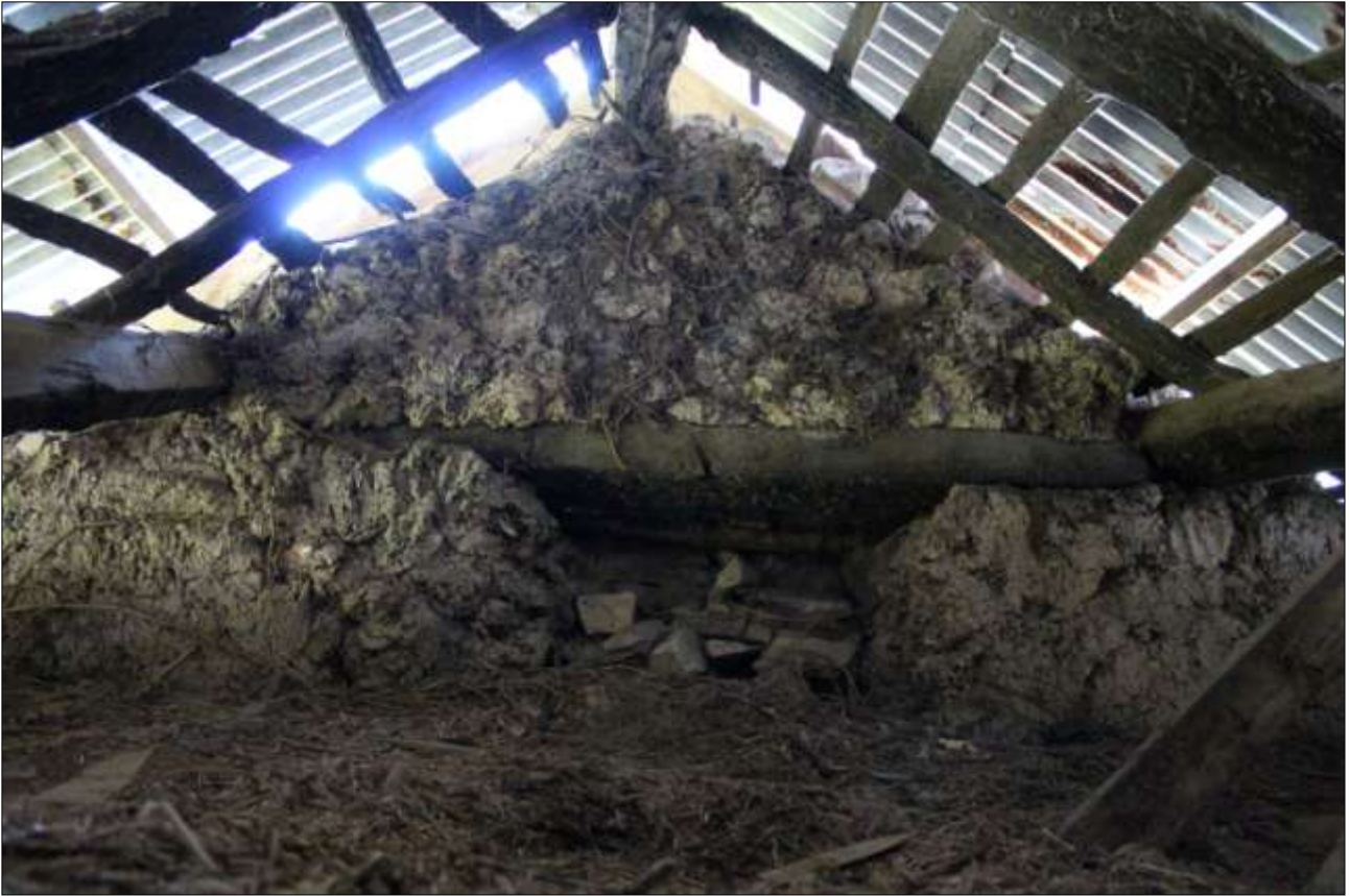
R5, THE BLOCKED SLIT VENT AT THE APEX OF THE NORTH-WEST GABLE; VIEWED FROM THE SOUTH-EAST.
