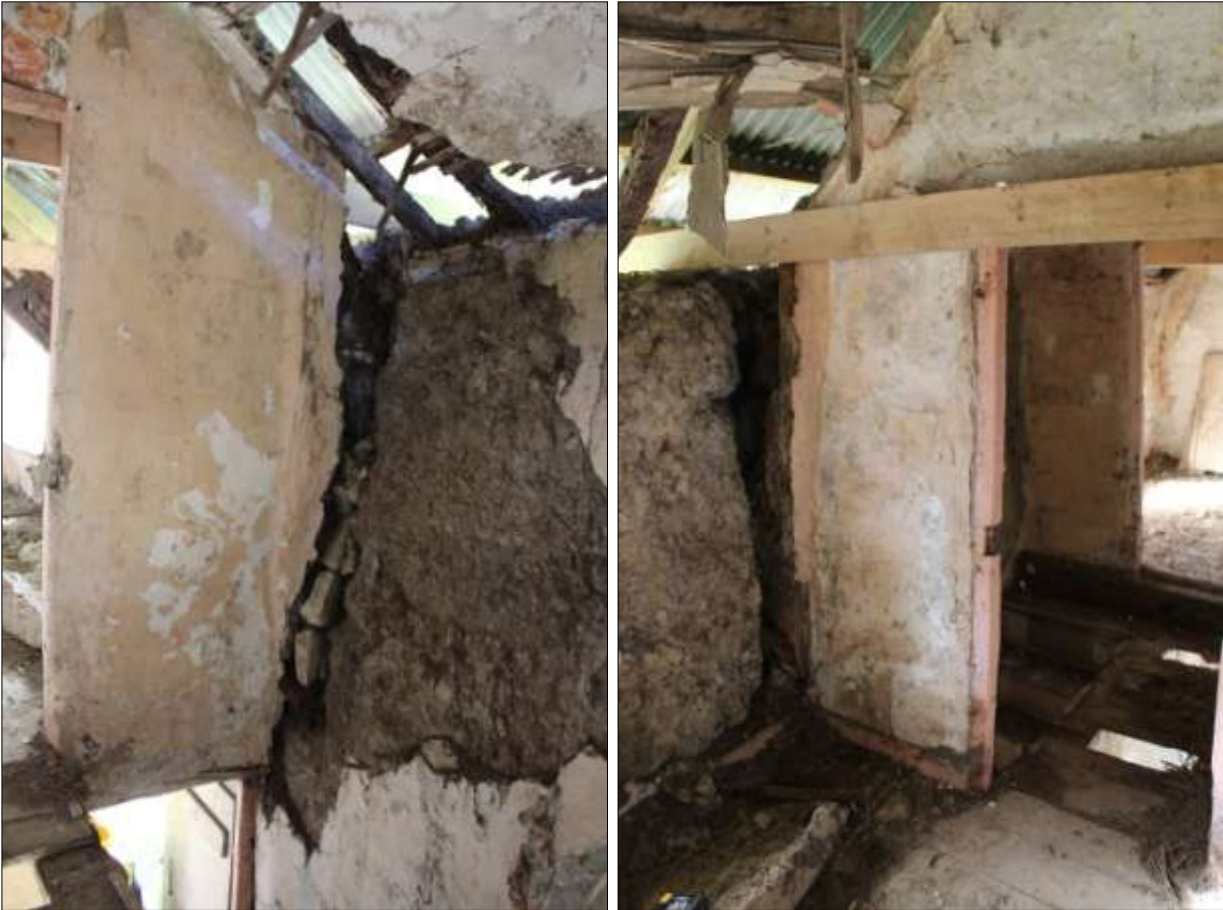
LEFT: THE SOUTH ANGLE OF R3, SHOWING THE EXTERNAL COB WALL FALLING AWAY FROM THE INTERNAL PARTITION; VIEWED FROM THE NORTH. RIGHT: THE WEST ANGLE OF R4, SHOWING THE SAME DETAIL; VIEWED FROM THE EAST.
