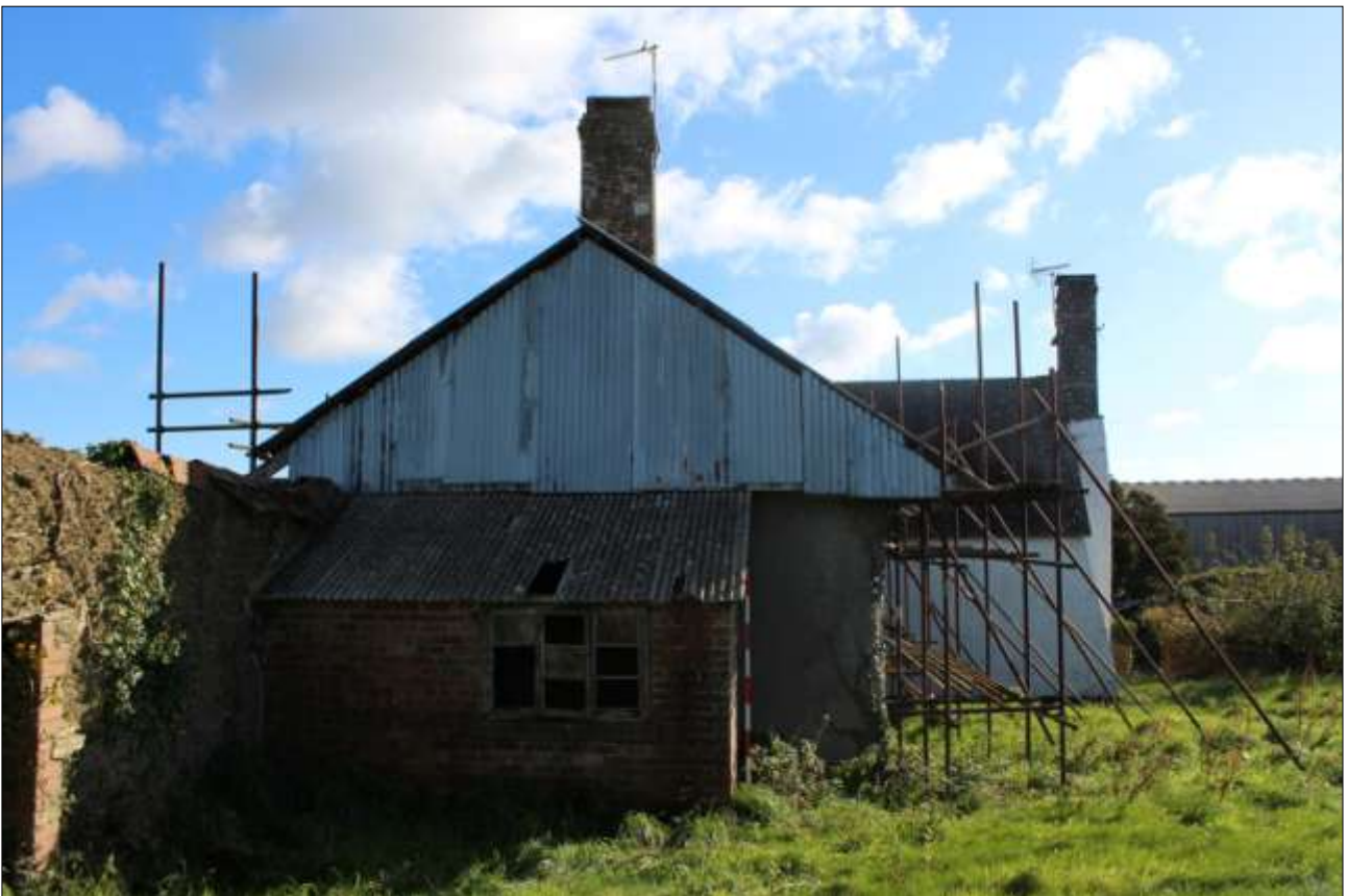
BRICK OUTHOUSE R6 BUILT ABUTTING THE NORTH-WEST GABLE; VIEWED FROM THE NORTH-WEST (SCALE 2M).
