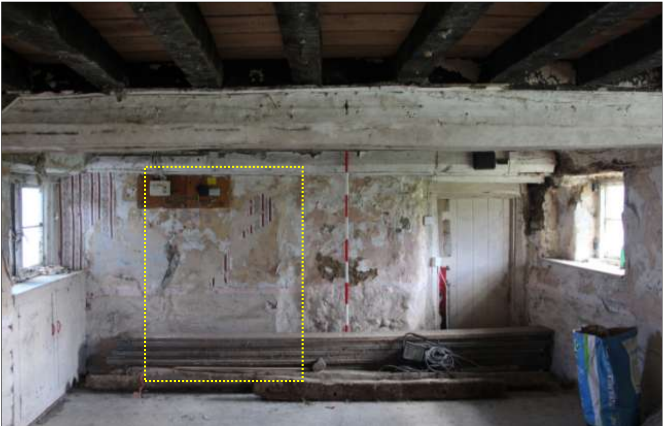
R1, SOUTH-EAST WALL FROM THE NORTH-WEST (SCALE 2M). THE BLOCKED OPENING IS INDICATED.
