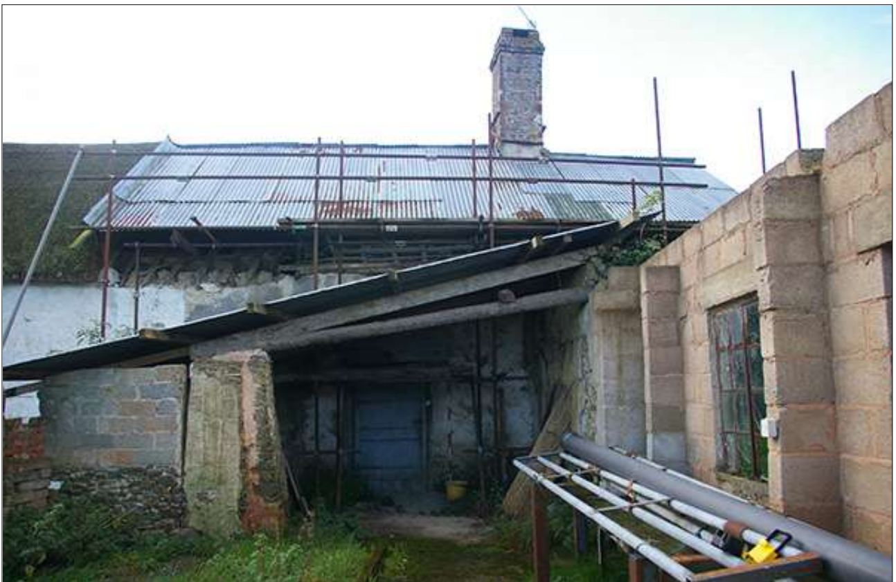
THE NORTH-EAST ELEVATION, EASTERN END, WHERE IT ABUTS THE LOST LINHAY. VIEWED FROM THE NORTH-EAST (SCALE 2M).
