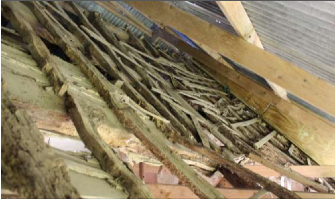
FIGURE 12: THE ROOF STRUCTURE ON THE SOUTH PITCH, VIEWED FROM THE WEST. NOTE THE PEGGED RAFTERS AND BATTENS.
