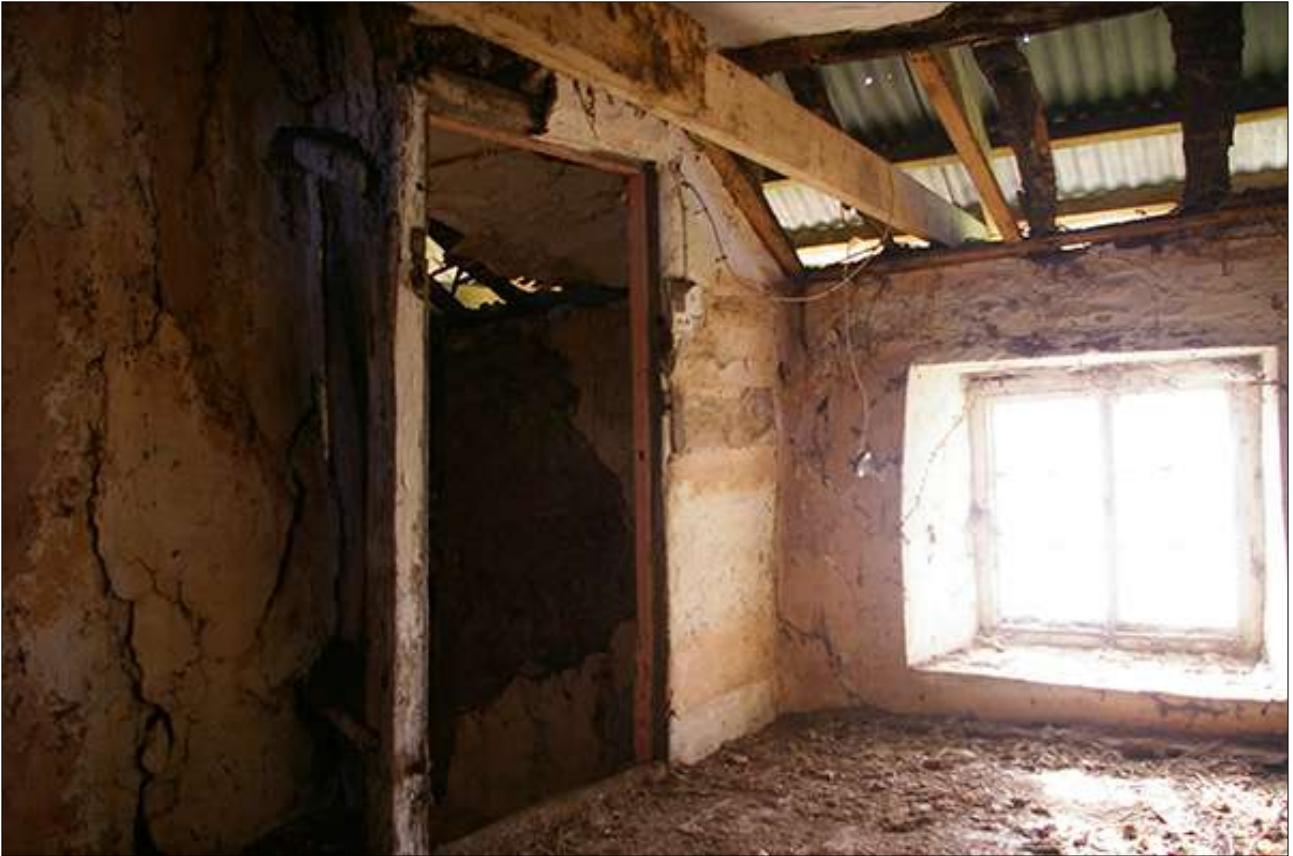
THE SOUTH ANGLE OF R5, SHOWING THE DOORWAY INTO R3; VIEWED FROM THE NORTH.
