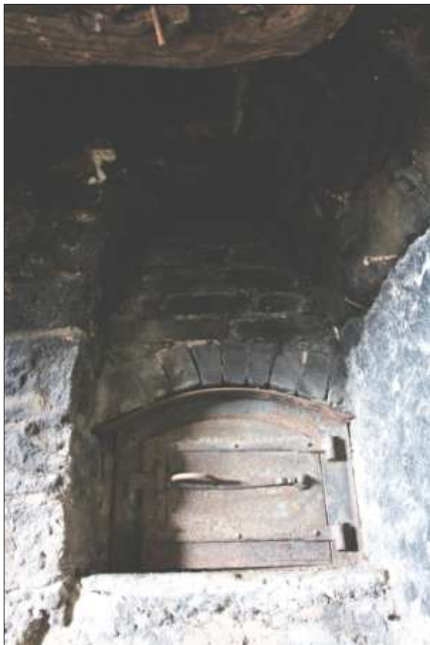
R1, THE C.1600 ARCHED OPENING TO THE FORMER BAKE OVEN; VIEWED FROM THE SOUTH-EAST.
