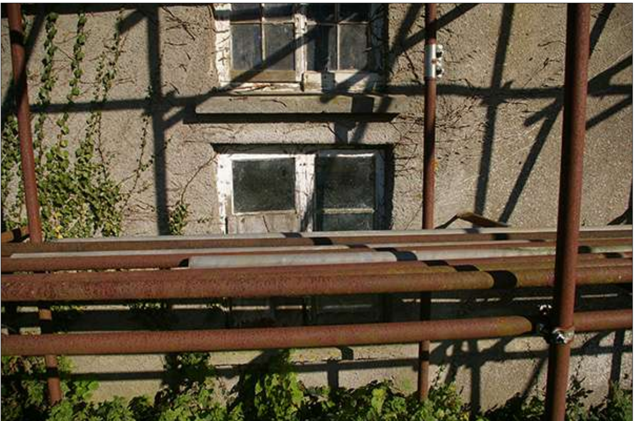
SOUTH-WEST ELEVATION, GF AND FF WINDOWS, R2 AND R5; VIEWED FROM THE SOUTH-WEST.
