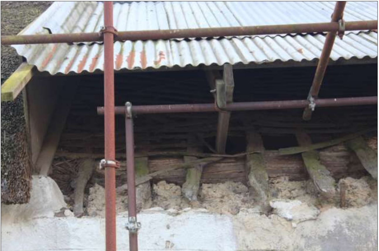
VIEW UNDER THE CORRUGATED SHEETING TO THE HISTORIC ROOF STRUCTURE; VIEWED FROM THE NORTH-EAST.
