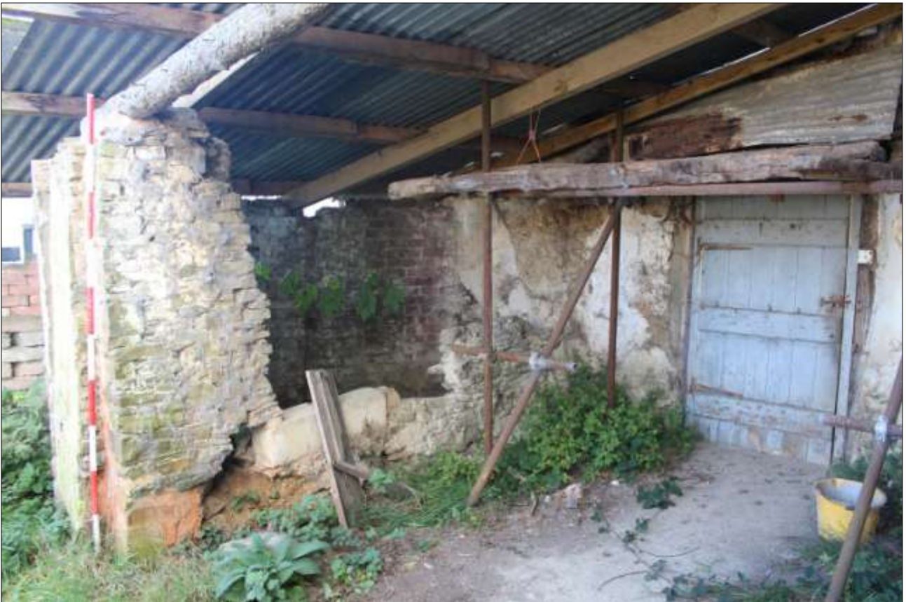
PART OF THE FORMER LINHAY ATTACHED TO THE COTTAGE; VIEWED FROM THE NORTH (SCALE 2M).
