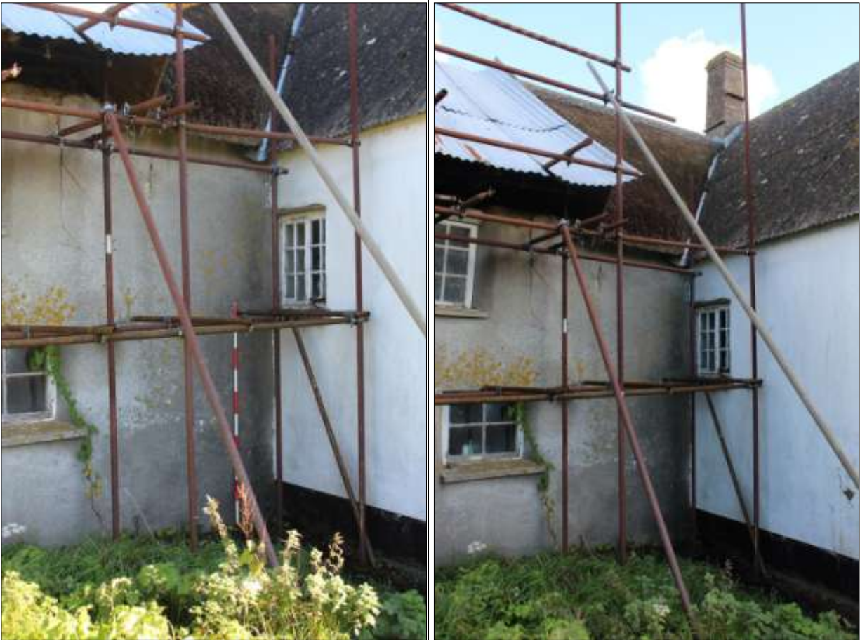
THE ANGLE BETWEEN THE COTTAGE AND THE REST OF THE FARMHOUSE; VIEWED FROM THE SOUTH-WEST (2M SCALE).
