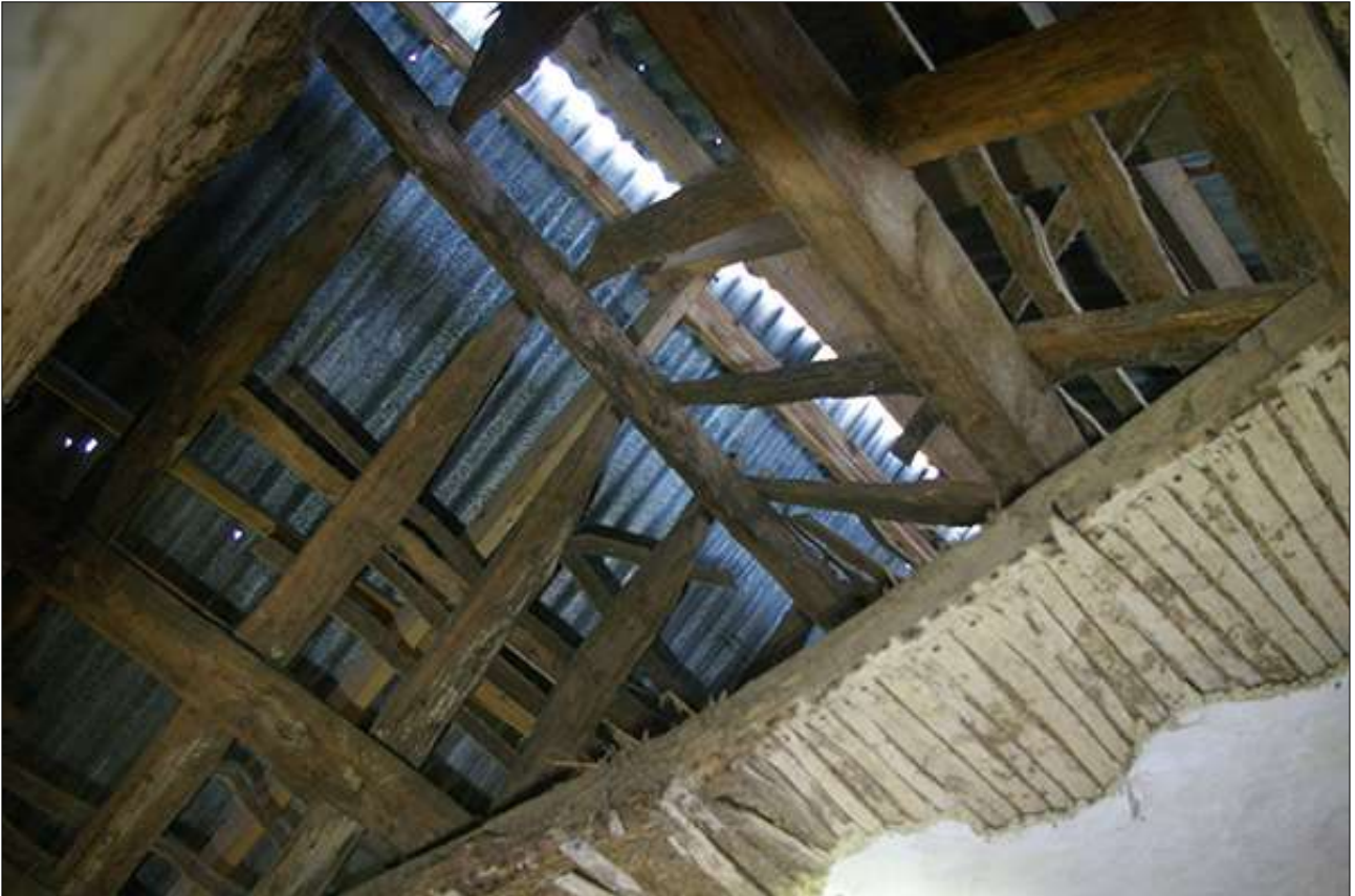
R4, THE RIDGEPOLE AND PEGGED RAFTERS; VIEWED FROM BELOW AND TO THE EAST.
