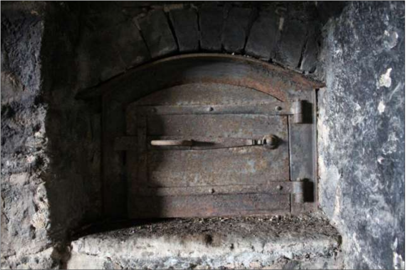
R1, THE 19 TH CENTURY CAST IRON DOOR TO THE FORMER BREAD OVEN; VIEWED FROM THE SOUTH-EAST.
