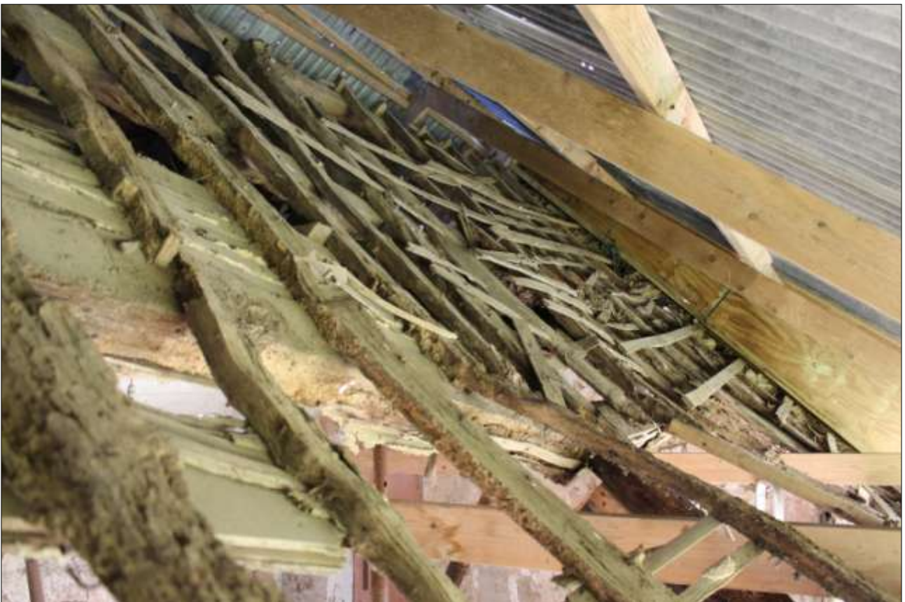
R4, THE SOUTH-WEST PITCH FROM ABOVE, SHOWING THE RAFTERS PEGGED TO THE TRUSS BLADE AND PURLINS, AND THE BATTENS PEGGED TO THE RAFTERS; VIEWED FROM THE SSW.
