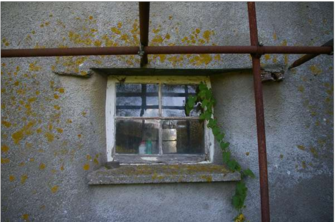
SOUTH-WEST ELEVATION, GF R1 EAST WINDOW, VIEWED FROM THE SOUTH-WEST. NOTE THE PROJECTING BEAM TOP RIGHT.
