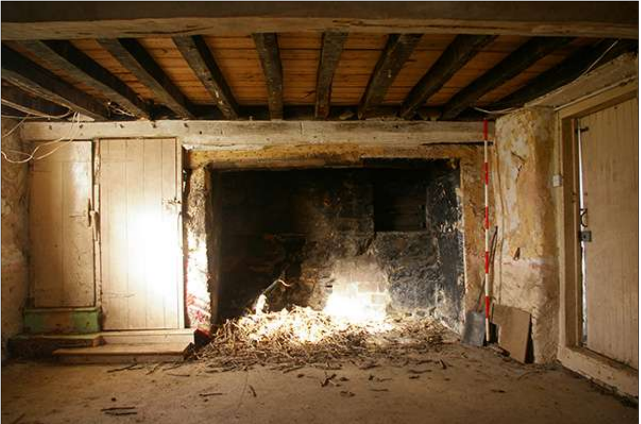
R1, NORTH-WEST WALL; VIEWED FROM THE SOUTH-EAST (SCALE 2M). THE WIDE HEARTH IS IMMEDIATELY APPARENT, WITH DOORS THROUGH TO R2 AND R3 TO THE LEFT.
