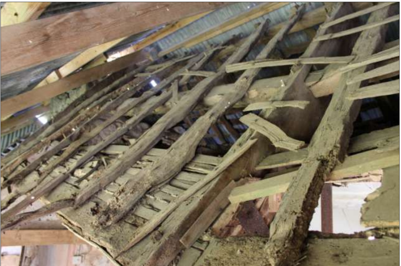
R4, THE SOUTH-WEST PITCH FROM ABOVE, SHOWING THE RAFTERS PEGGED TO THE TRUSS BLADE AND PURLINS, AND THE BATTENS PEGGED TO THE RAFTERS; VIEWED FROM THE SSE.
