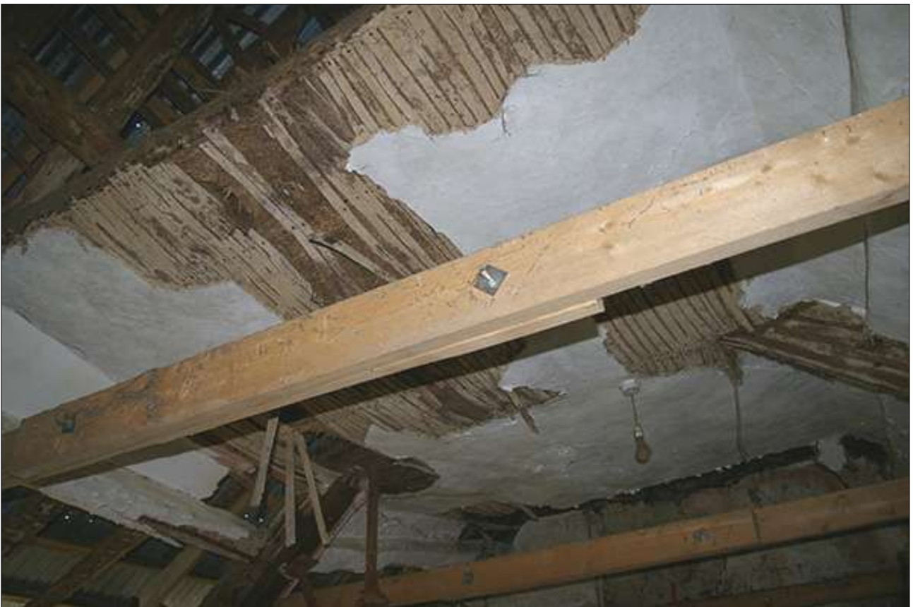
R4, VIEW OF THE INSERTED LATH-AND -PLASTER CEILING; VIEWED FROM THE EAST.
