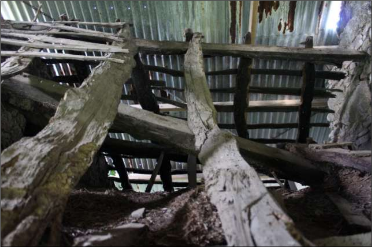
R5, DETAIL OF THE ROOF STRUCTURE (SOUTH-WEST PITCH); VIEWED FROM THE SOUTH-WEST.
