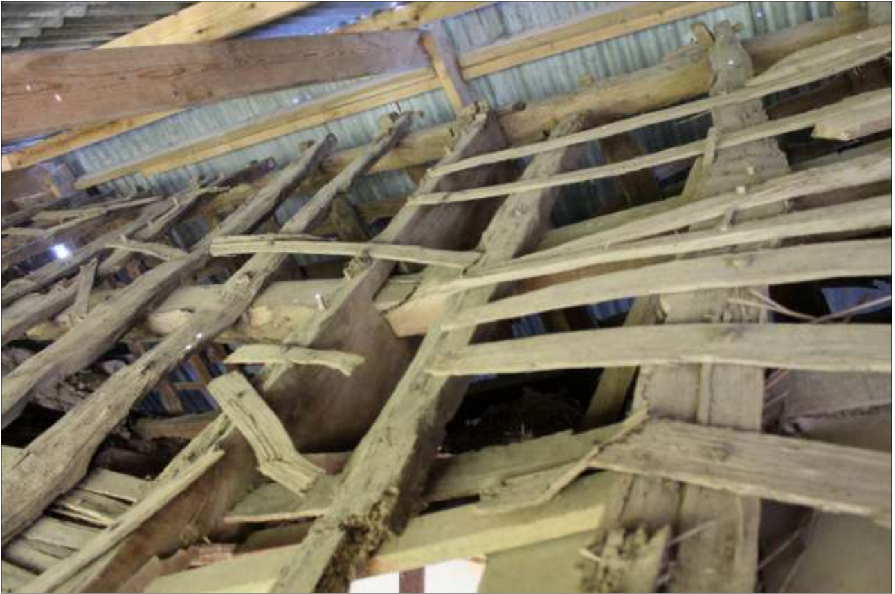
R4, AS ABOVE, SHOWING THE LAPPED PURLINS MEETING AT THE TRUSS BLADE; VIEWED FROM THE SOUTH.
