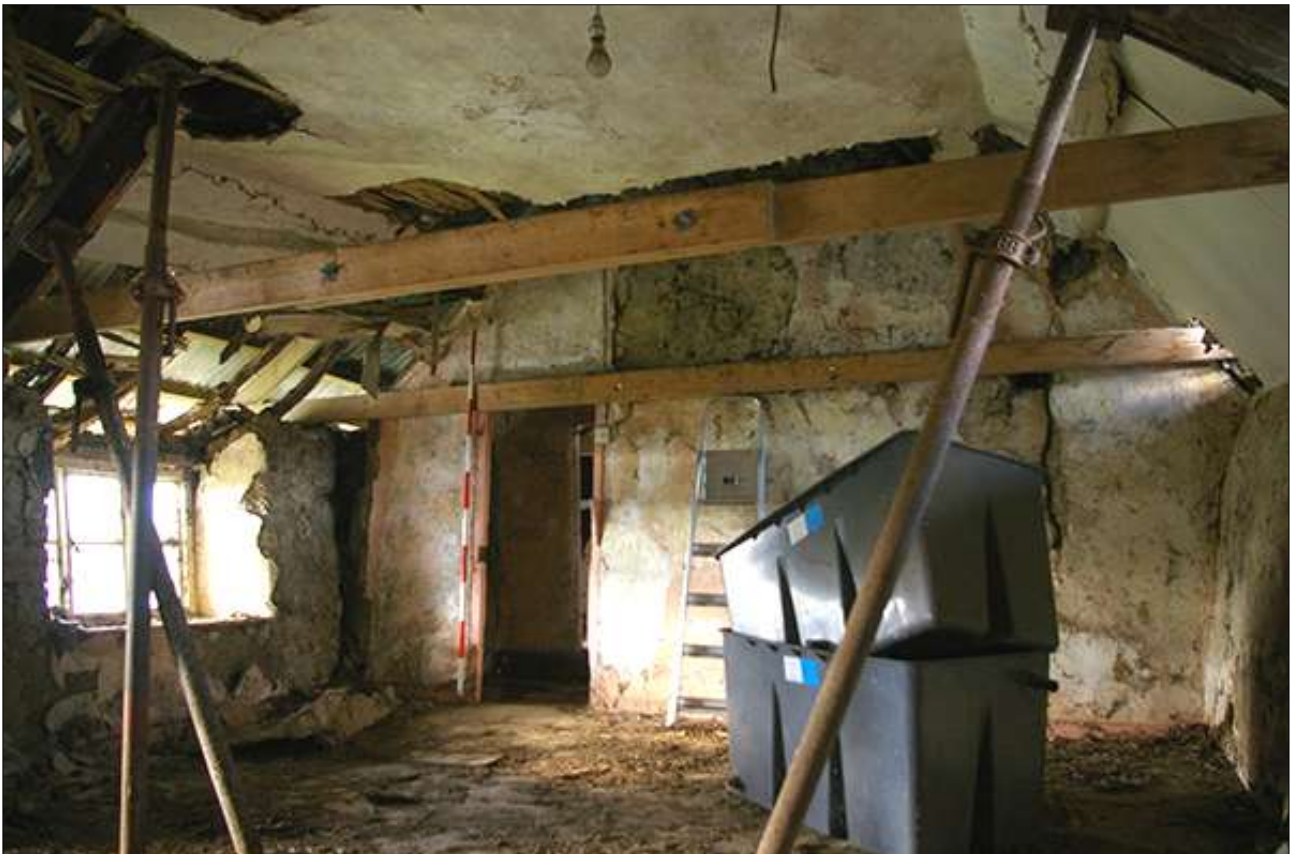
R4, NORTH-WEST WALL, WITH STACK AND DOORWAY TO R3; VIEWED FROM THE EAST.
