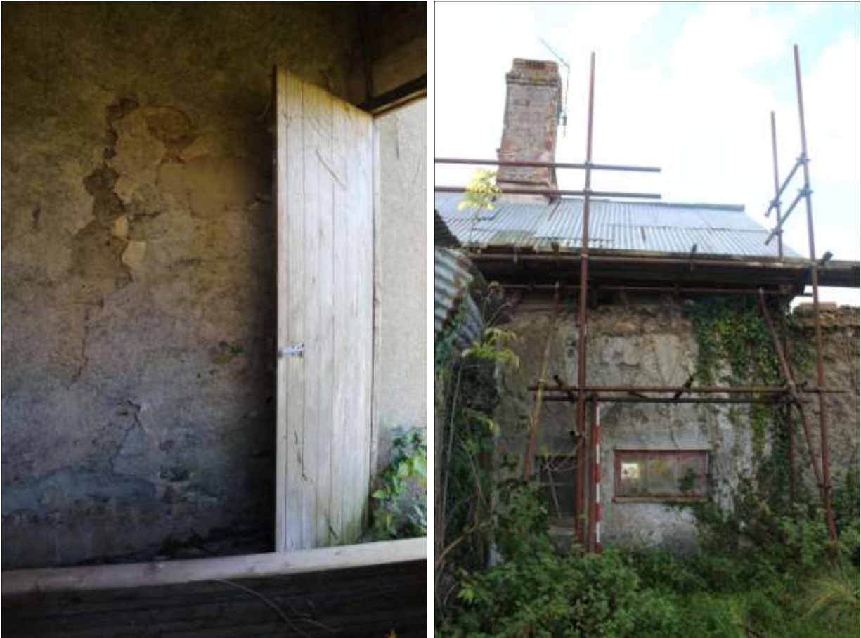
LEFT: INTERIOR OF B6, SHOWING THE BLOCKED OPENING; VIEWED FROM THE WEST.
