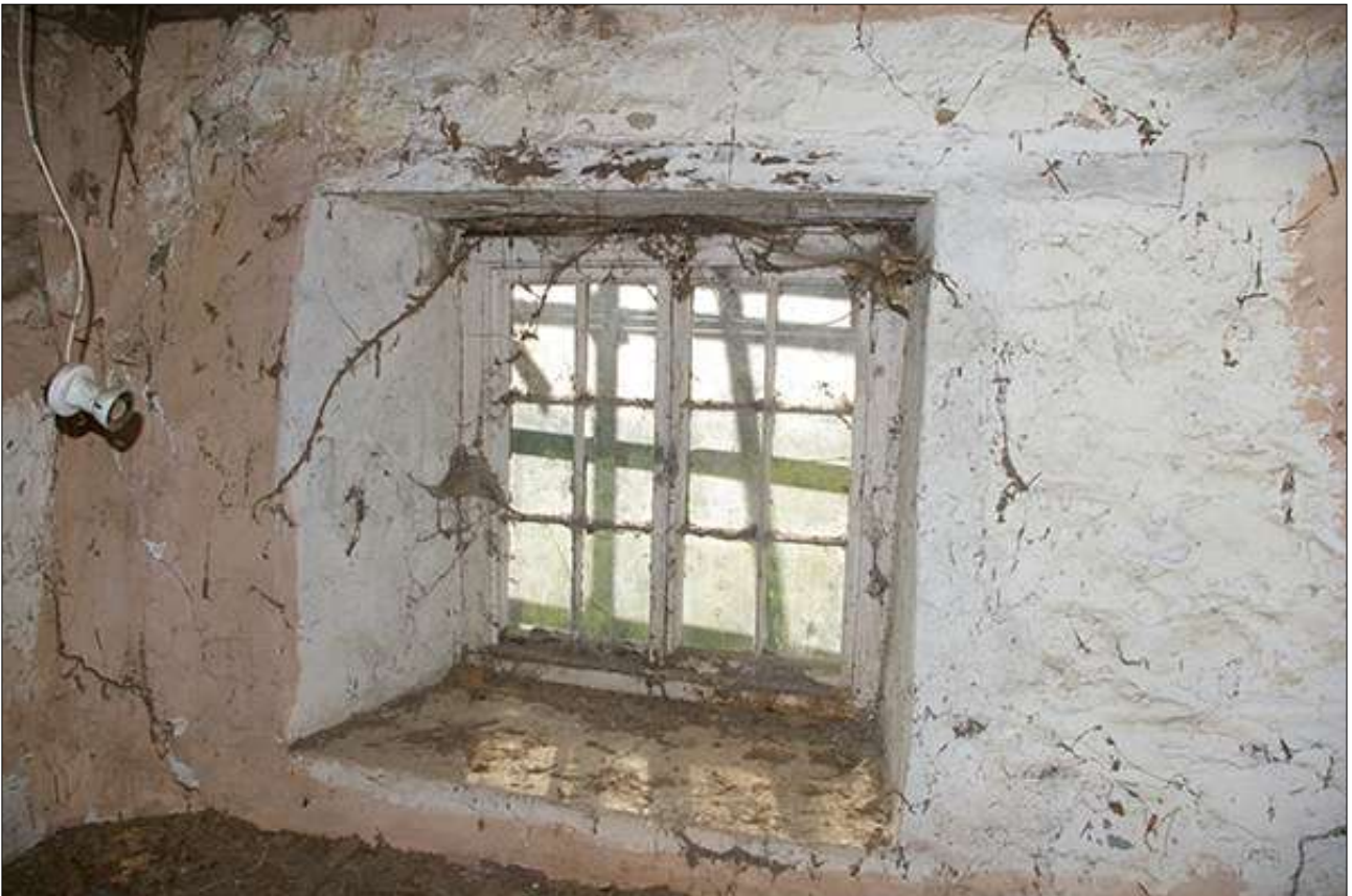
R5, DETAIL OF THE WINDOW IN THE SOUTH-WEST WALL; VIEWED FROM THE NORTH.
