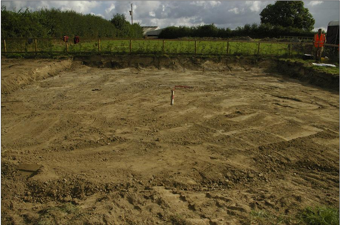
41. AREA 11, POST-EXCAVATION FOLLOWING MAIN SURFACE STRIP; VIEWED FROM THE SOUTH-WEST (1M & 2M SCALES).
