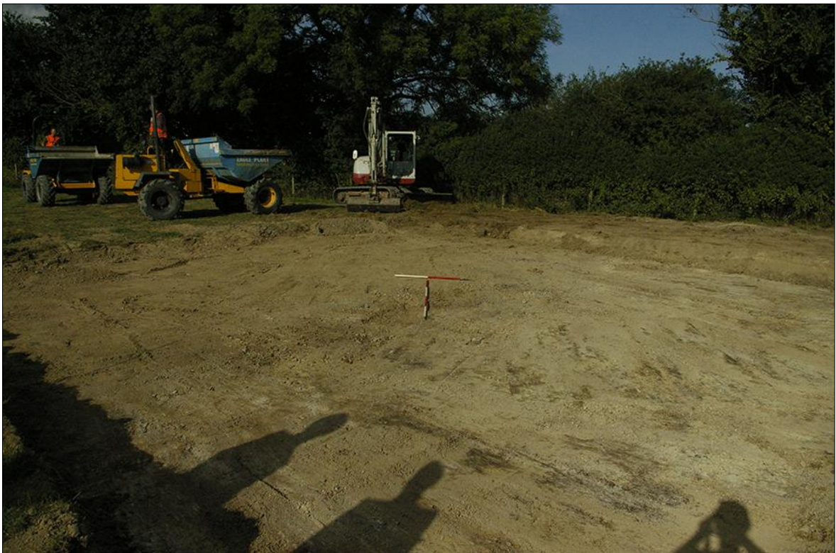
40. AREA 11, POST-EXCAVATION FOLLOWING MAIN SURFACE STRIP; VIEWED FROM THE NORTH-EAST (1M & 2M SCALES).
