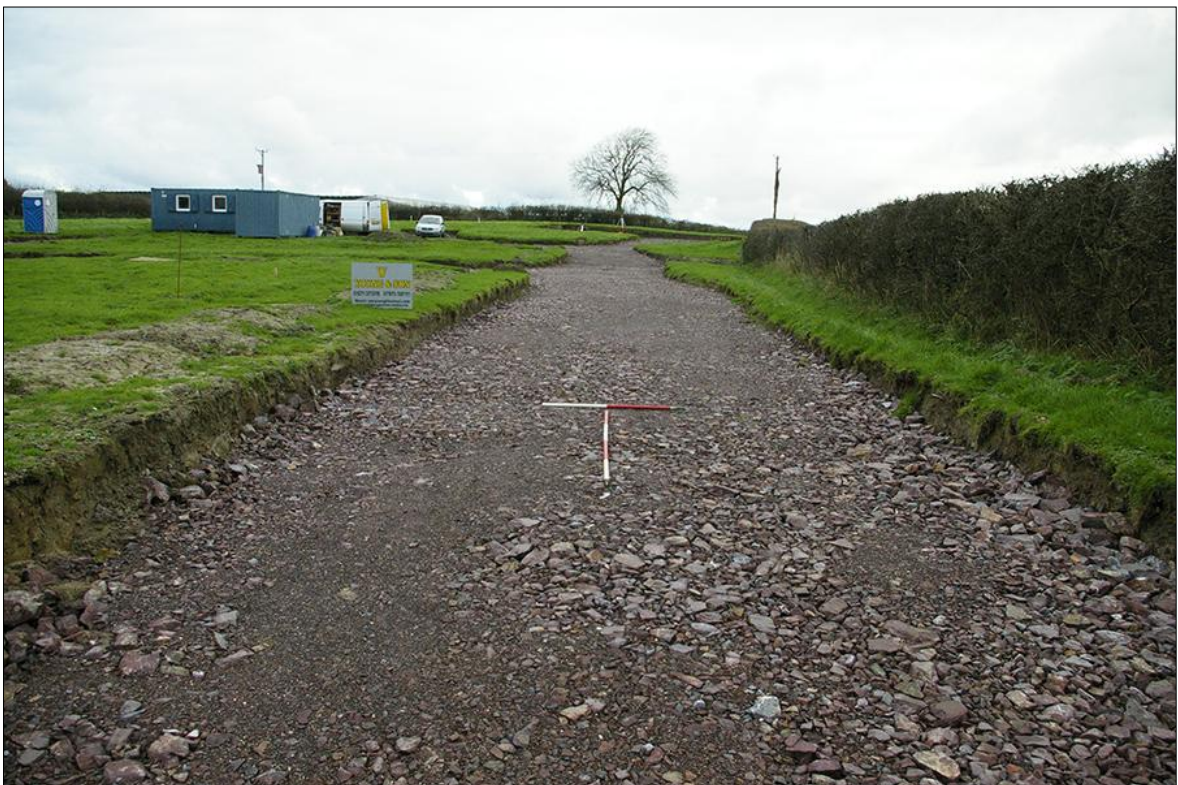
2. AREA 05 MAIN SECTION STRIPPED AND STONED; VIEWED FROM THE SOUTH-WEST (1M & 2M SCALES).
