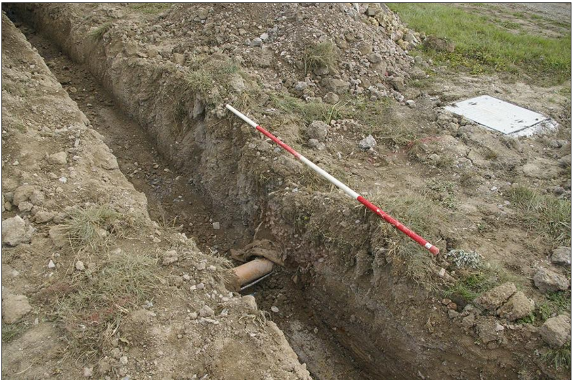
28. MODERN DRAIN WITHIN AREA 09, MAIN SECTION; VIEWED FROM THE SOUTH-WEST (2M SCALE).
