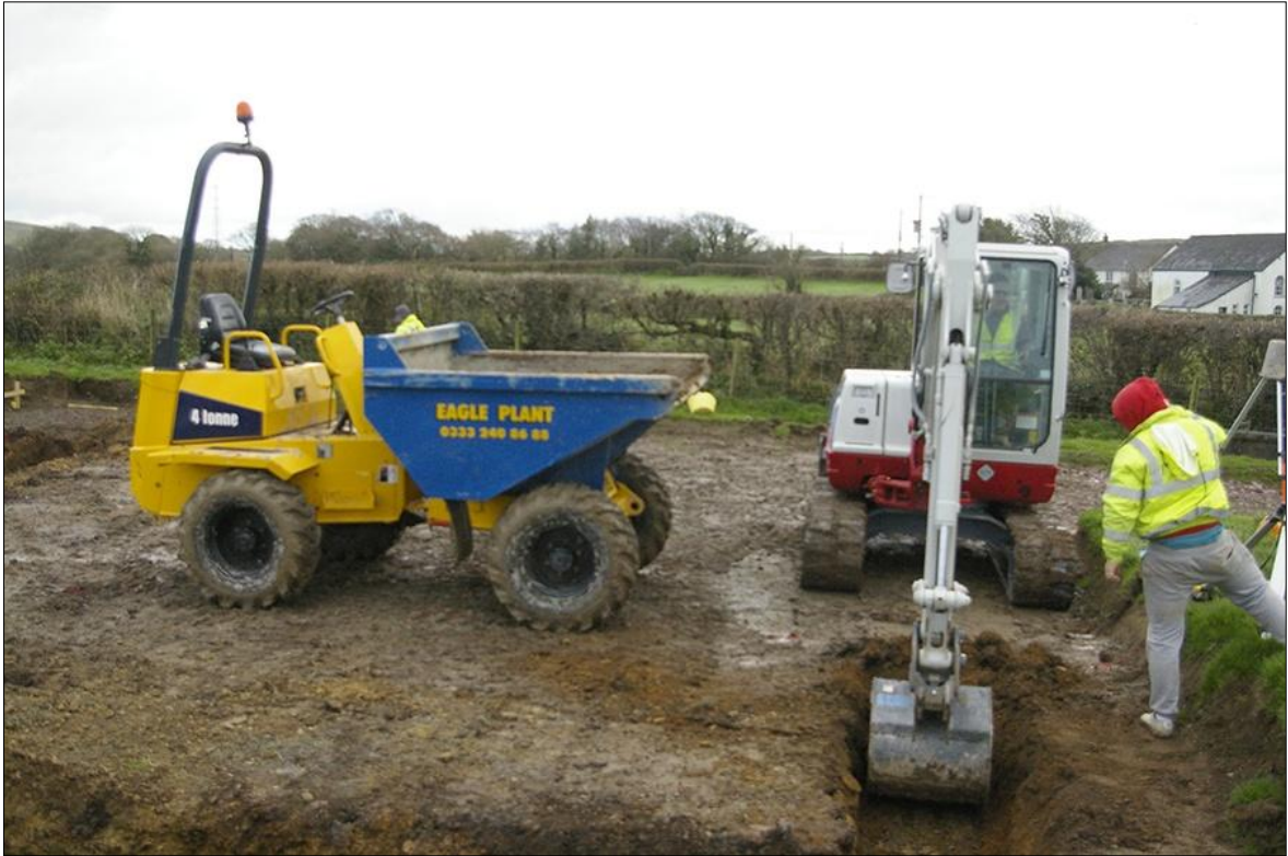
9. WORKING SHOT, EXCAVATION OF FOUNDATION TRENCHES WITHIN AREA 06; VIEWED FROM THE NORTH-WEST (NO SCALE).
