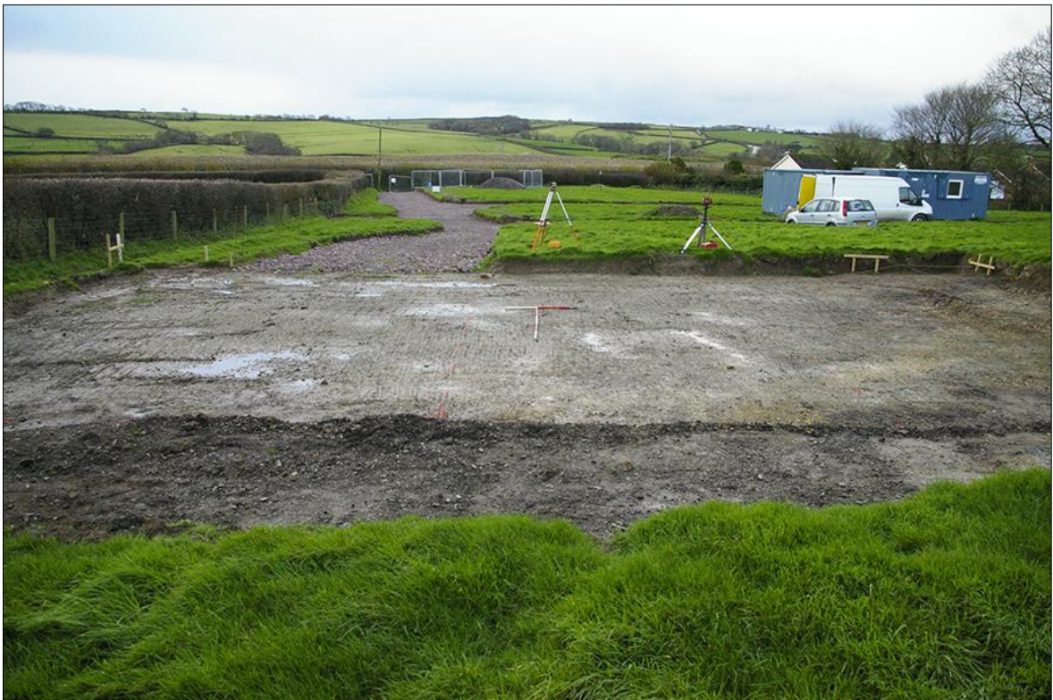
6. AREA 06 FOLLOWING MAIN SOIL STRIP; VIEWED FROM THE NORTH-EAST (1M & 2M SCALES).
