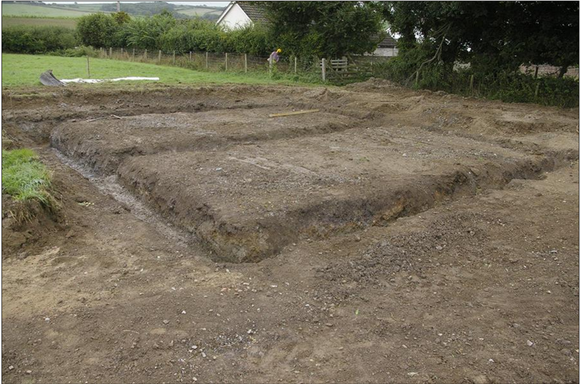
53. AREA 12, POST-EXCAVATION, FOLLOWING EXCAVATION OF FOUNDATION TRENCHES; VIEWED FROM THE NORTH-EAST (NO SCALE).
