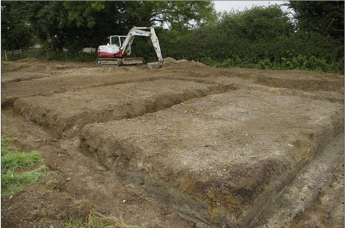
43. AREA 11, POST-EXCAVATION, FOLLOWING FOUNDATION TRENCH EXCAVATION; VIEWED FROM THE NORTH-EAST (NO SCALE).
