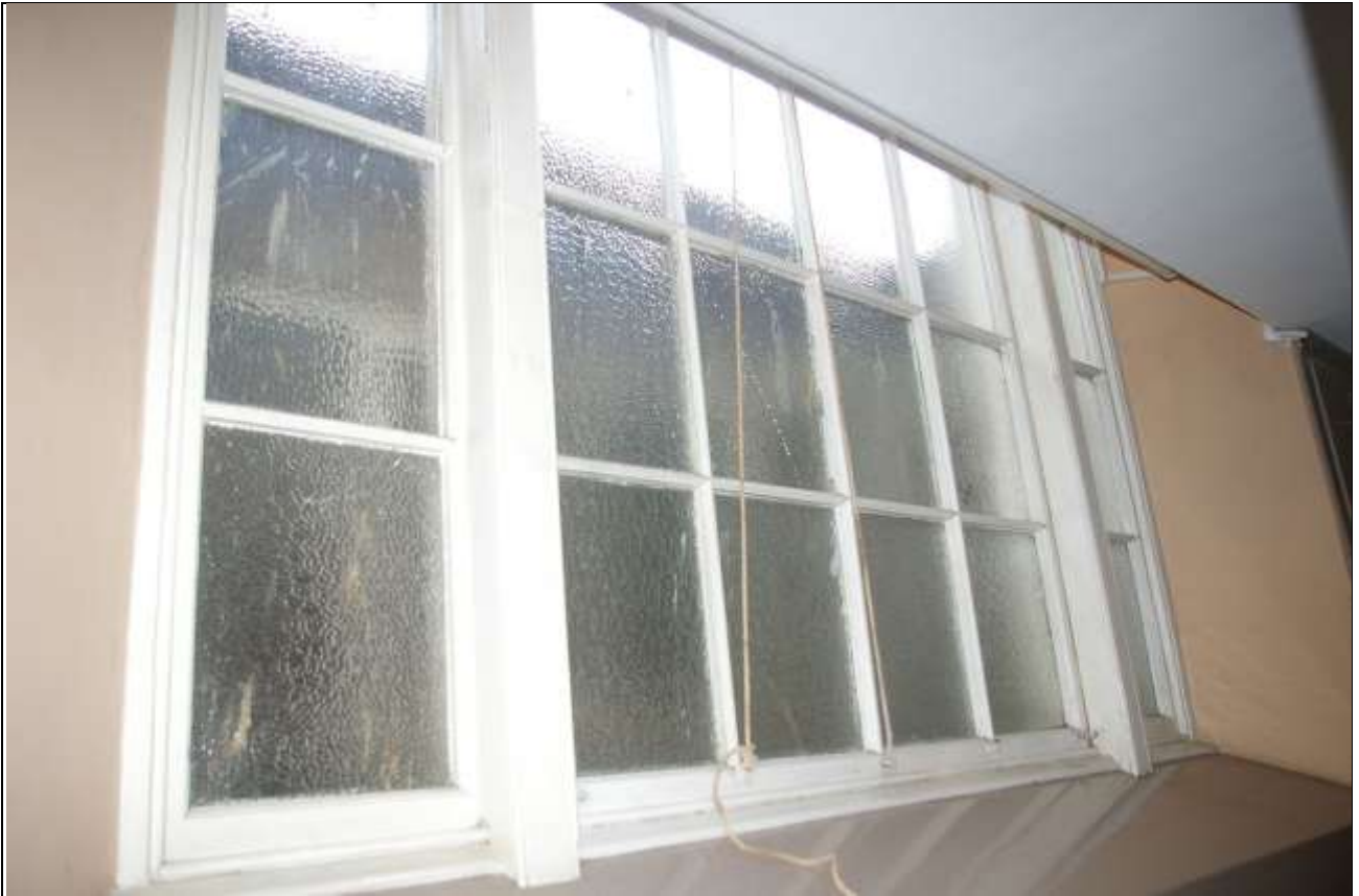
ROOM 6; THE POST-1855 THREE-LIGHT HORNED SASH WINDOW IN THE EAST WALL OF THE MAIN CHAMBER; FROM THE NORTH-WEST.
