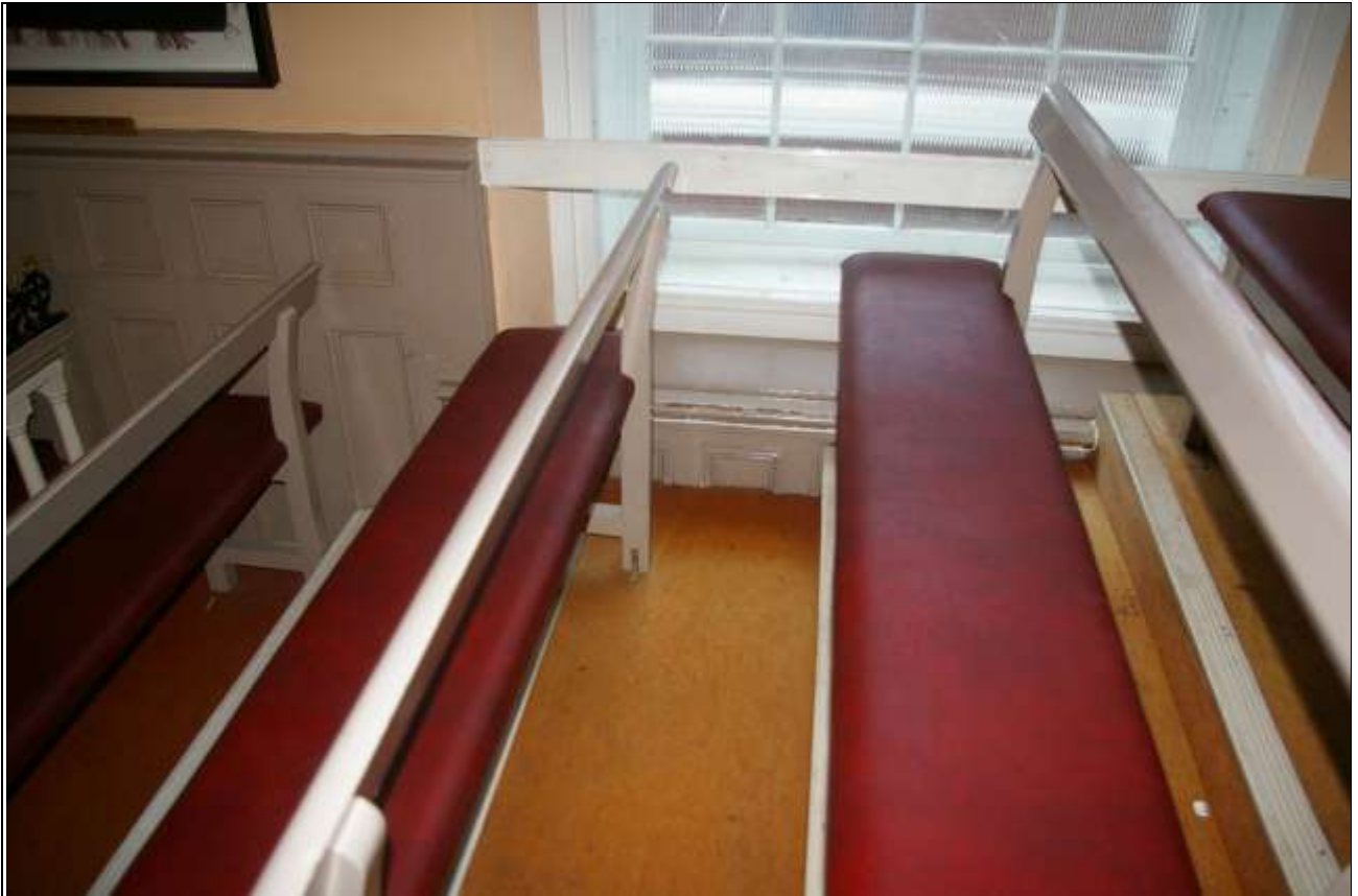
ROOM 6; THE PANELLING TO THE SIDES OF THE TIERED PUBLIC GALLERY SEATING, SHOWING PANELS CUT IN HALF, SUGGESTING THE TIERS OF SEATING HAVE BEEN RESET OR RECONFIGURED; FROM THE EAST-NORTH-EAST.
