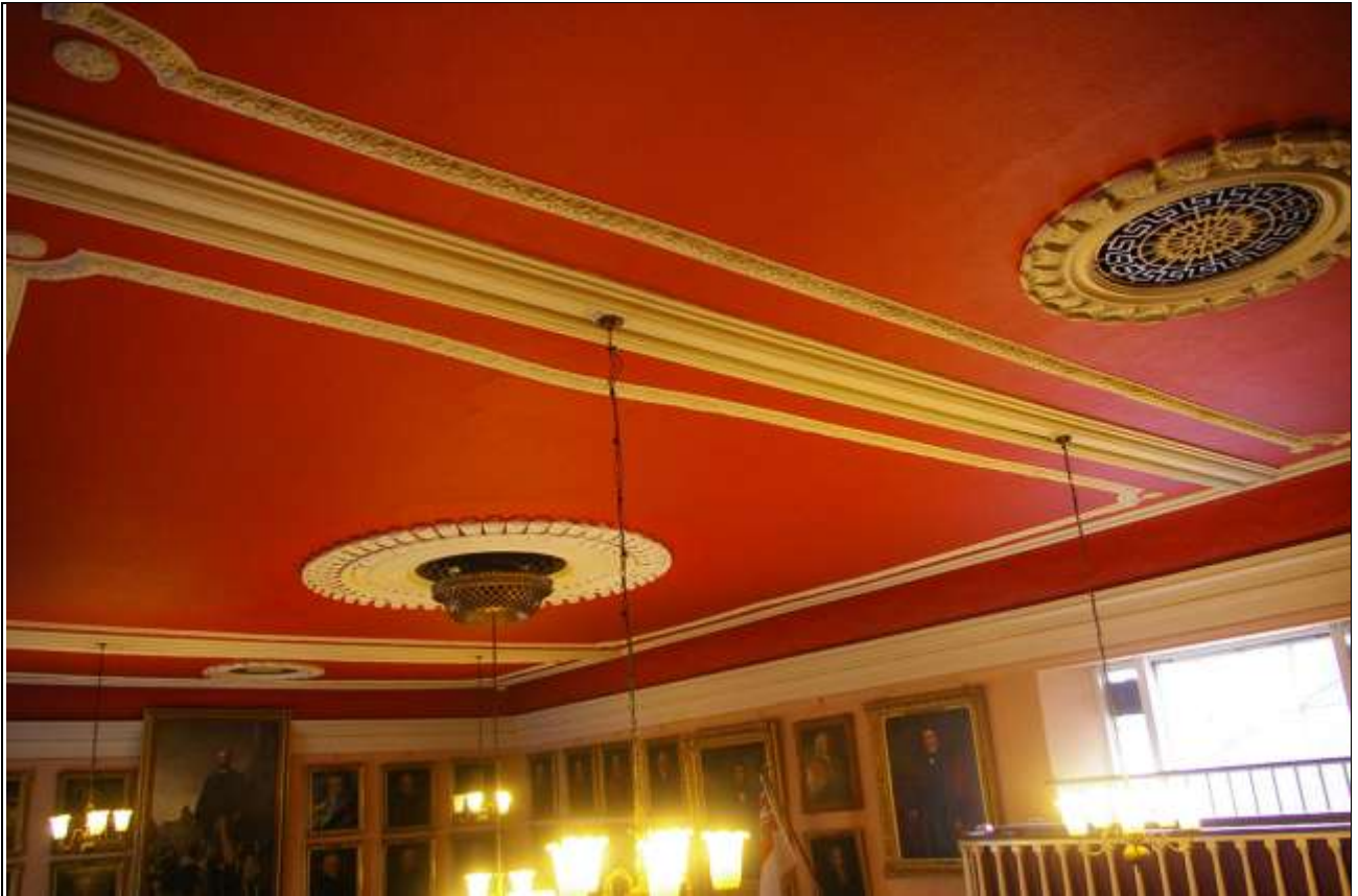
THE BEAUTIFUL PLASTER ROOF OF THE MAIN CHAMBER (ROOM 6); FROM THE SOUTH-WEST
