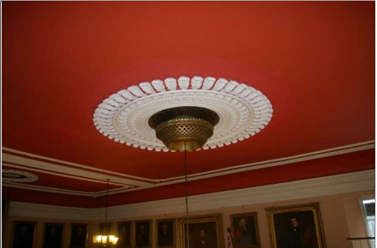
THE LARGEST OF THE TWO CEILING ROSES ON THE MAIN CHAMBER CEILING (ROOM 6), WHICH HAS BEEN RESTORED AFTER A COLLAPSE.
