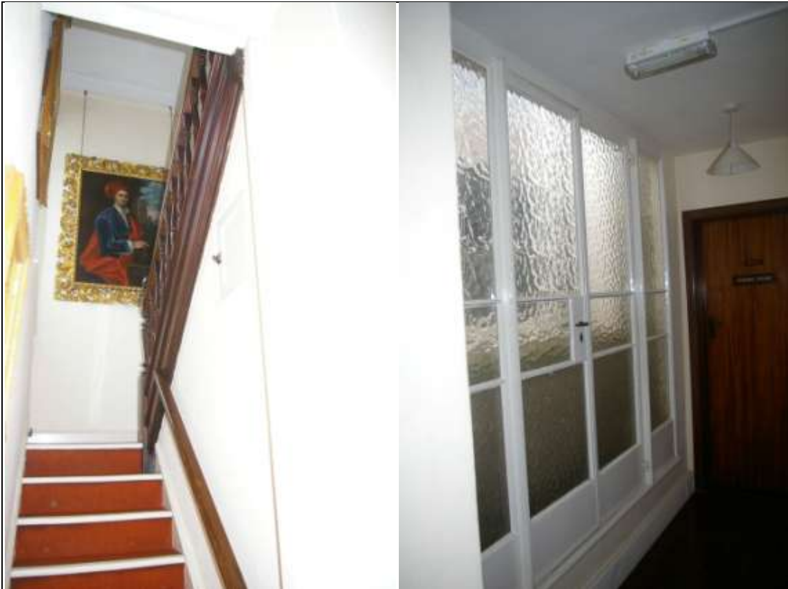
LEFT: ROOM 4/ROOM 2; THE STAIRS TO THE SECOND FLOOR, A 20 TH CENTURY STAIR, A HISTORIC COPY; FROM THE NORTH. RIGHT: THE GLAZED WALL WITHIN ROOM 8, OF METAL FRAMED CRITTAL STYLE; FROM THE SOUTH-EAST.
