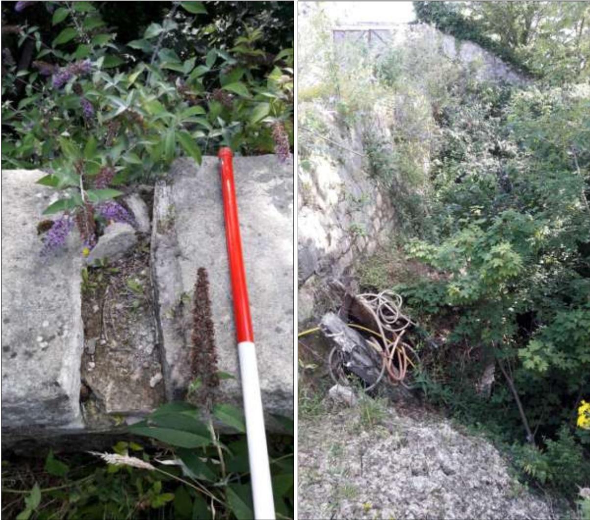
LEFT: A groove cut in the wall separating the drying floor and the linhay, corresponding to the concrete gully below B2 (above).
