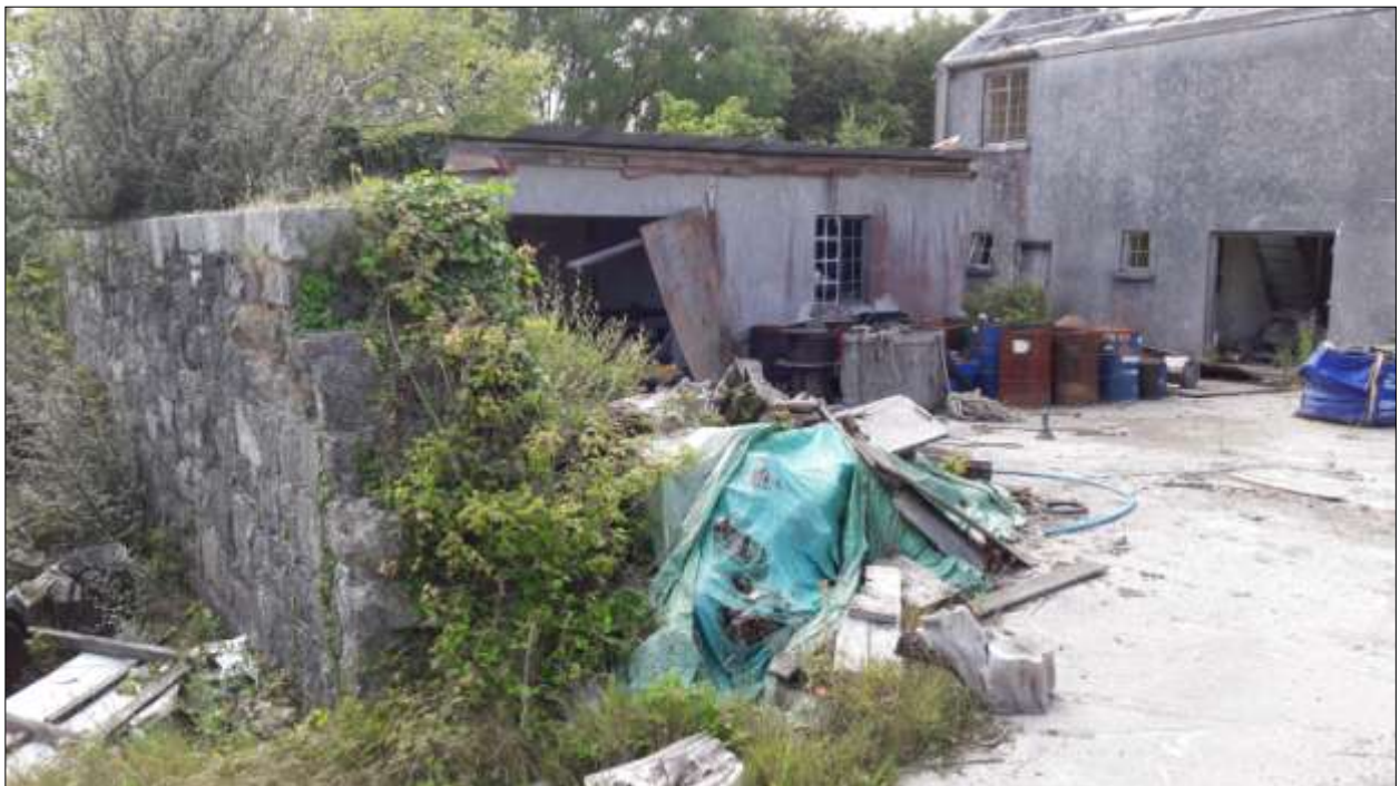
The breach in the south wall of T8, showing the yard with B3 and B2; viewed from the east.
