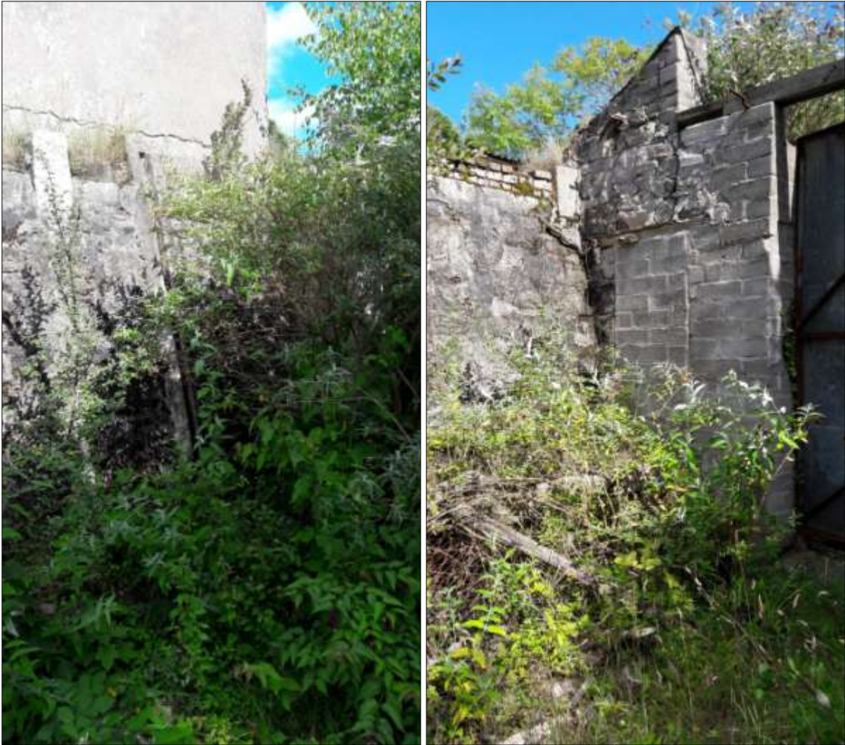
LEFT: The west wall of T7 below B2, showing a concrete gully running down the battered surface of the wall; viewed from the north-west.
