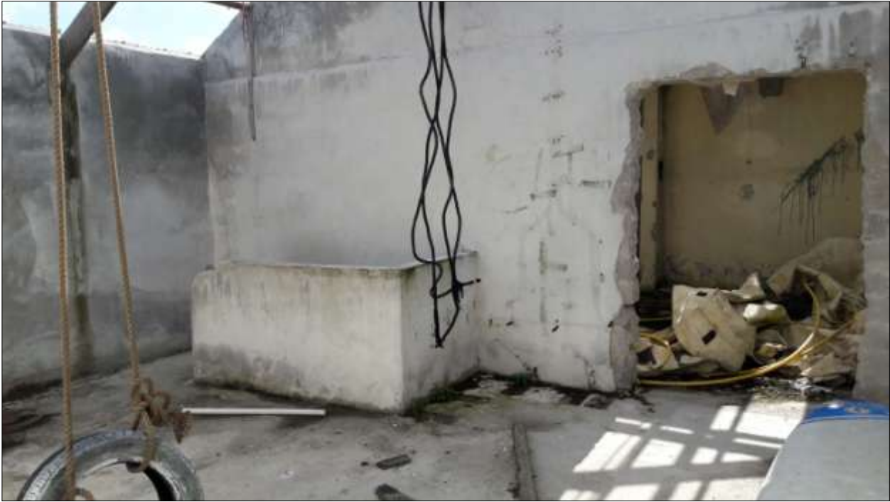
B2, the first floor interior of the pump house showing the breach to the staff welfare; viewed from the north-east.
