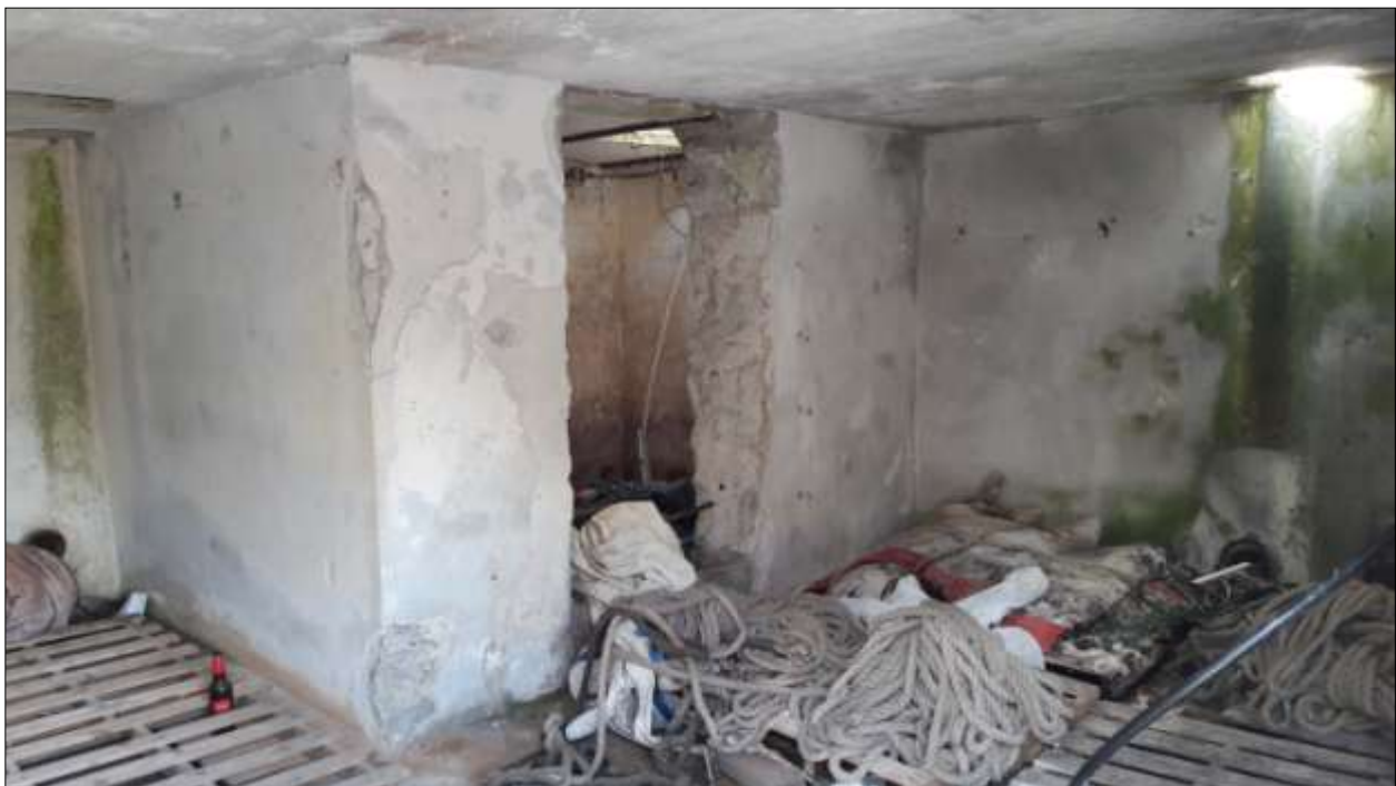
B2, the ground floor interior of the pump house; viewed from the south-west.
