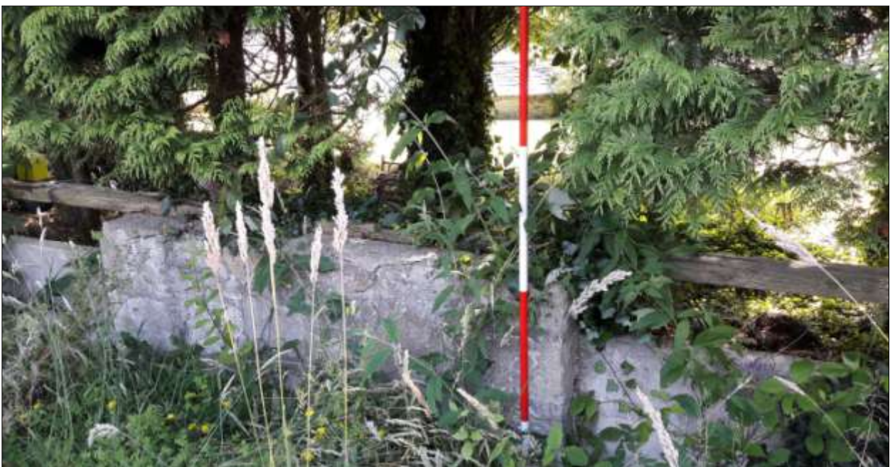
The west wall of the linhay, showing one of the stone sections; viewed from the east (scale 2m).
