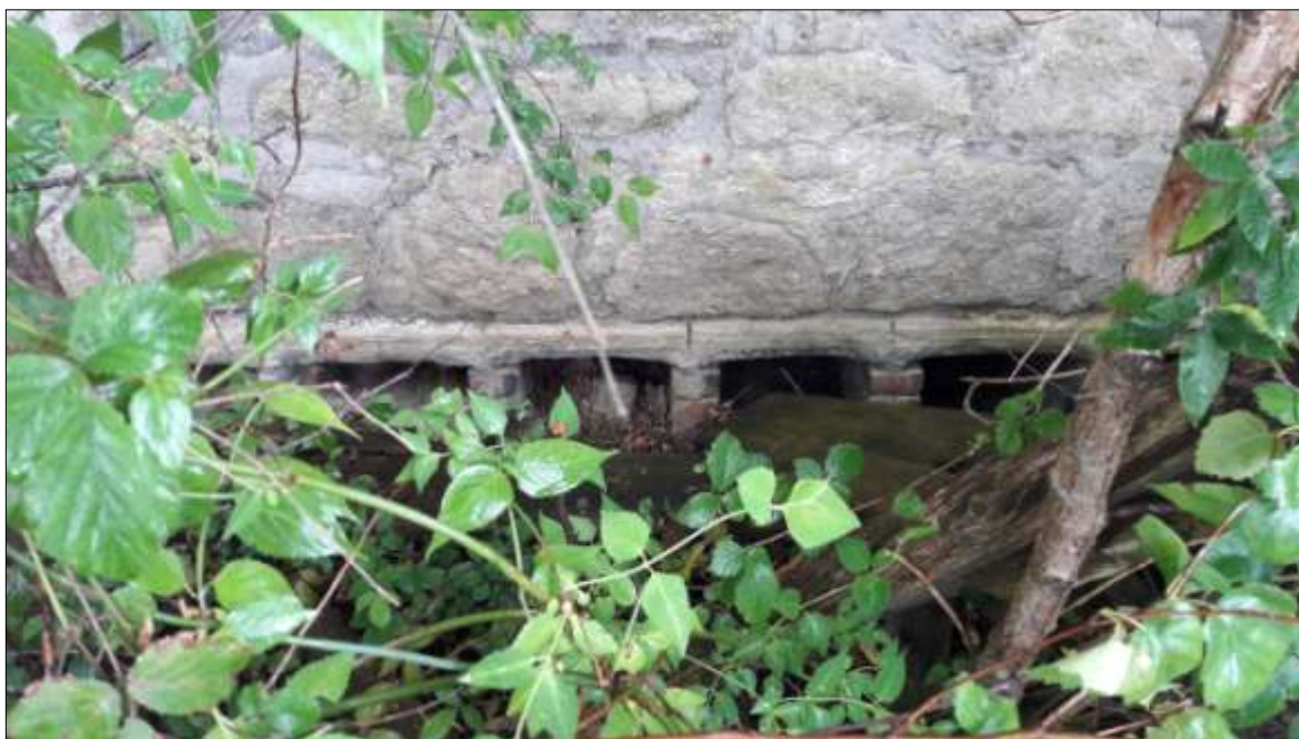
FIGURE 18: THE FLUES ENTERING THE BASE OF THE CHIMNEY, VIEWED FROM THE SSE.
