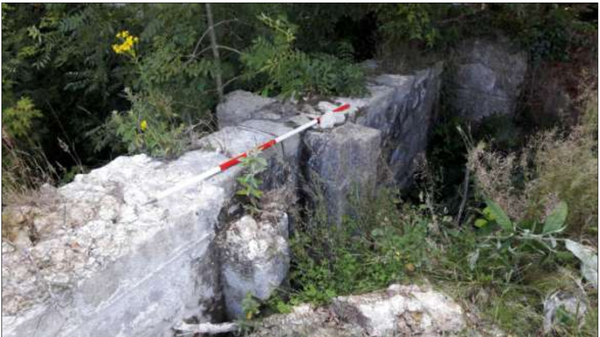
FIGURE 21: THE WALL SEPARATING C4 AND C5, SHOWING THE POSSIBLE OPENING WITH REINFORCED PROJECTING REVEALS; VIEWED FROM THE NORTH-EAST (SCALE 2M).
