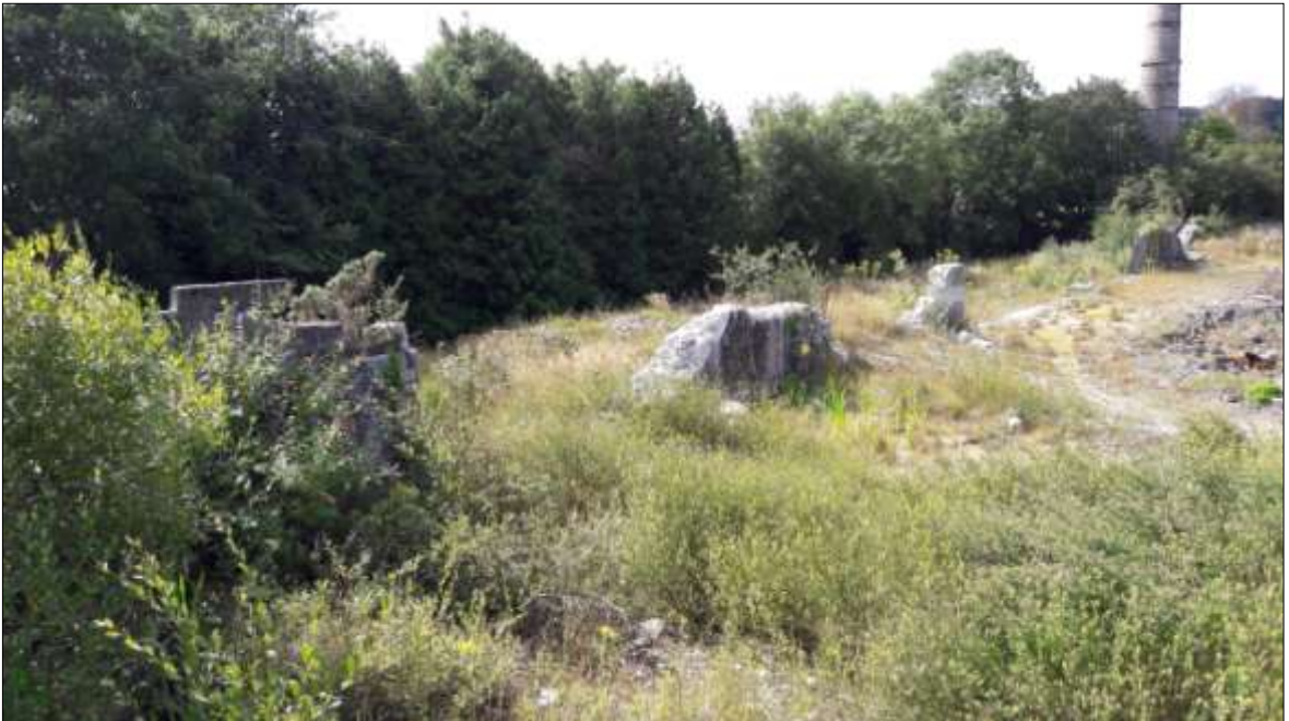
FIGURE 12: THE REMAINS OF THE WEST WALL OF THE SETTLING TANKS, VIEWED FROM THE SOUTH-EAST.
