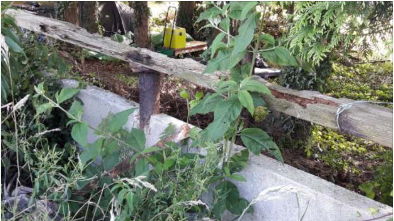
The west wall of the linhay, showing the iron pillars, wooden wallplate, and concrete blocking; viewed from the north-east.
