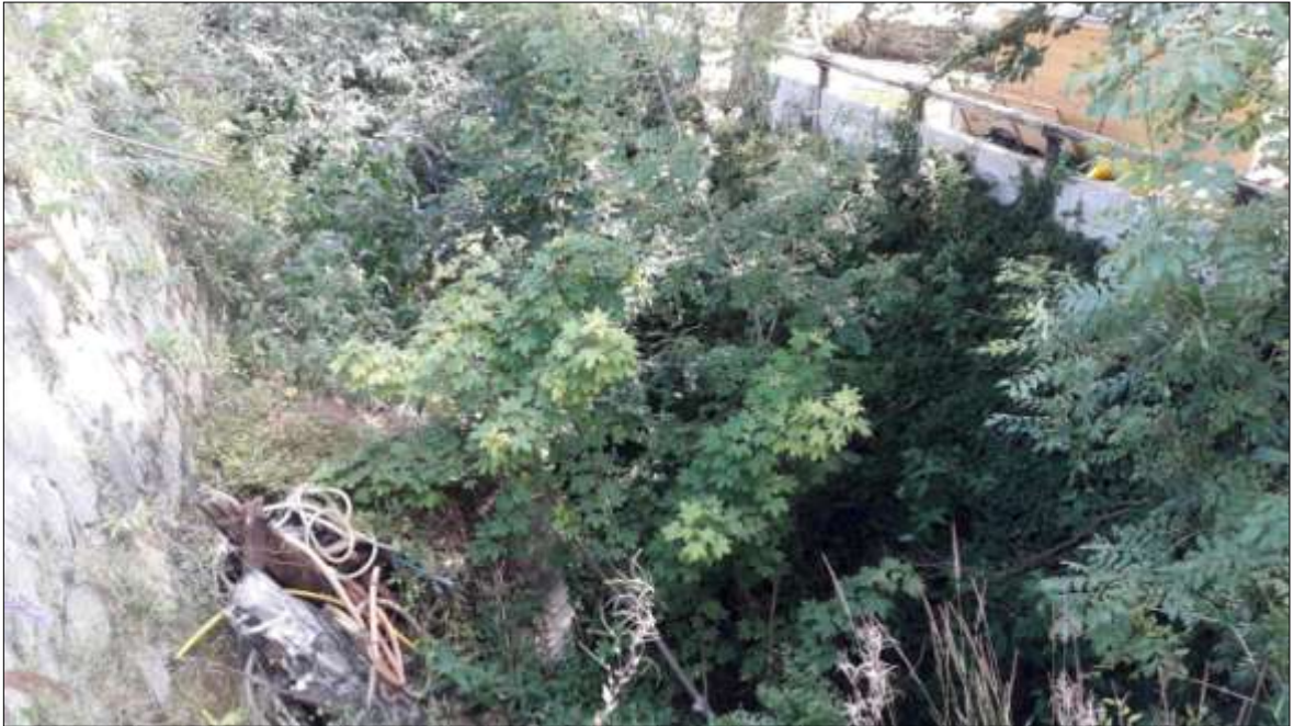
FIGURE 20: C5, SHOWING THE DEPTH OF THE FEATURE, AND THE RUBBISH/UNDERGROWTH; VIEWED FROM THE NORTH.
