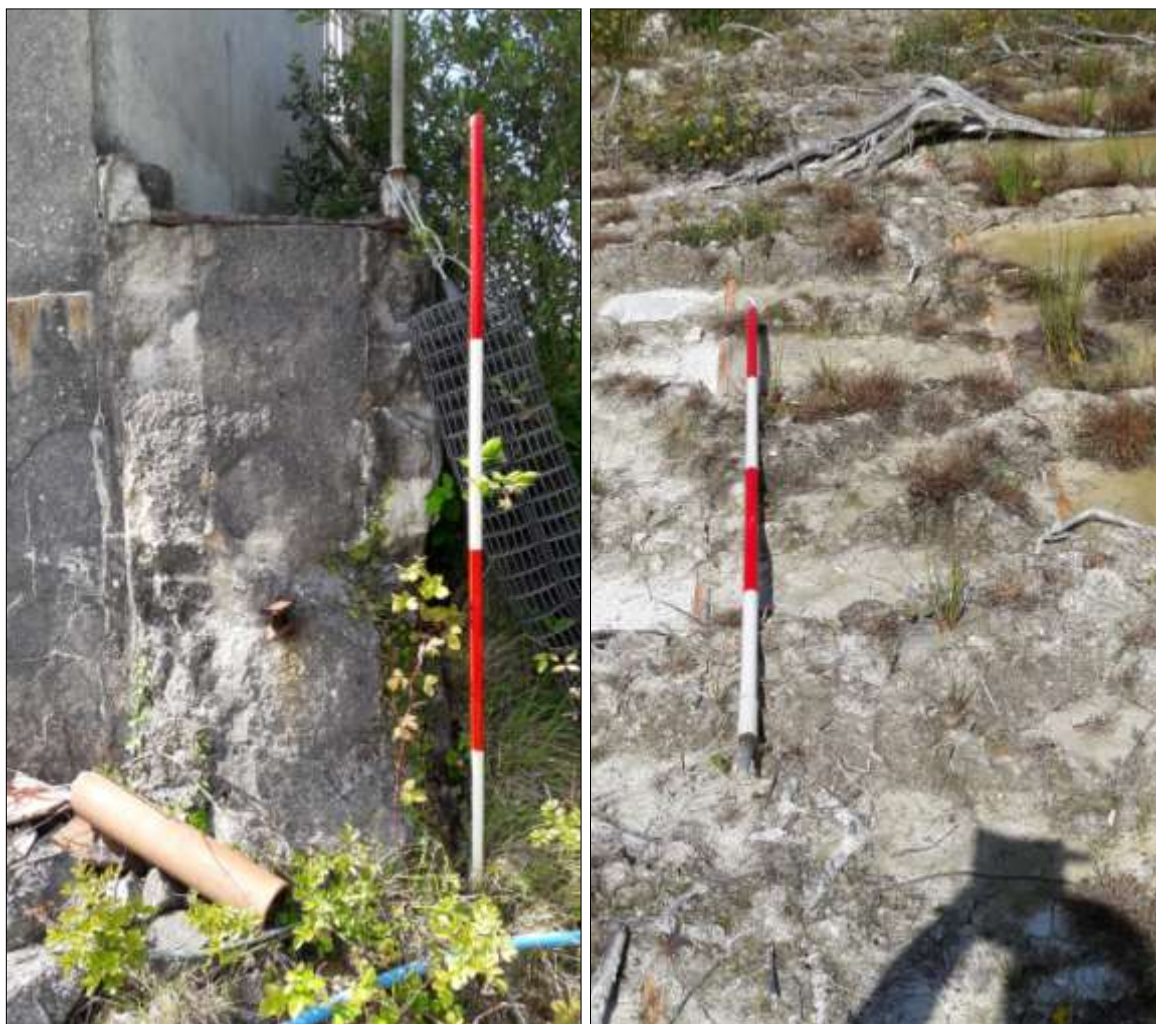
LEFT FIGURE 13: SECTION THROUGH THE 1945×55 TANK WALL ADJACENT TO B2; VIEWED FROM THE SOUTH (SCALE 2M). RIGHT FIGURE 14: THE TRAM RAILS IN THE BASE OF T3, VIEWED FROM THE WEST (SCALE 2M).
