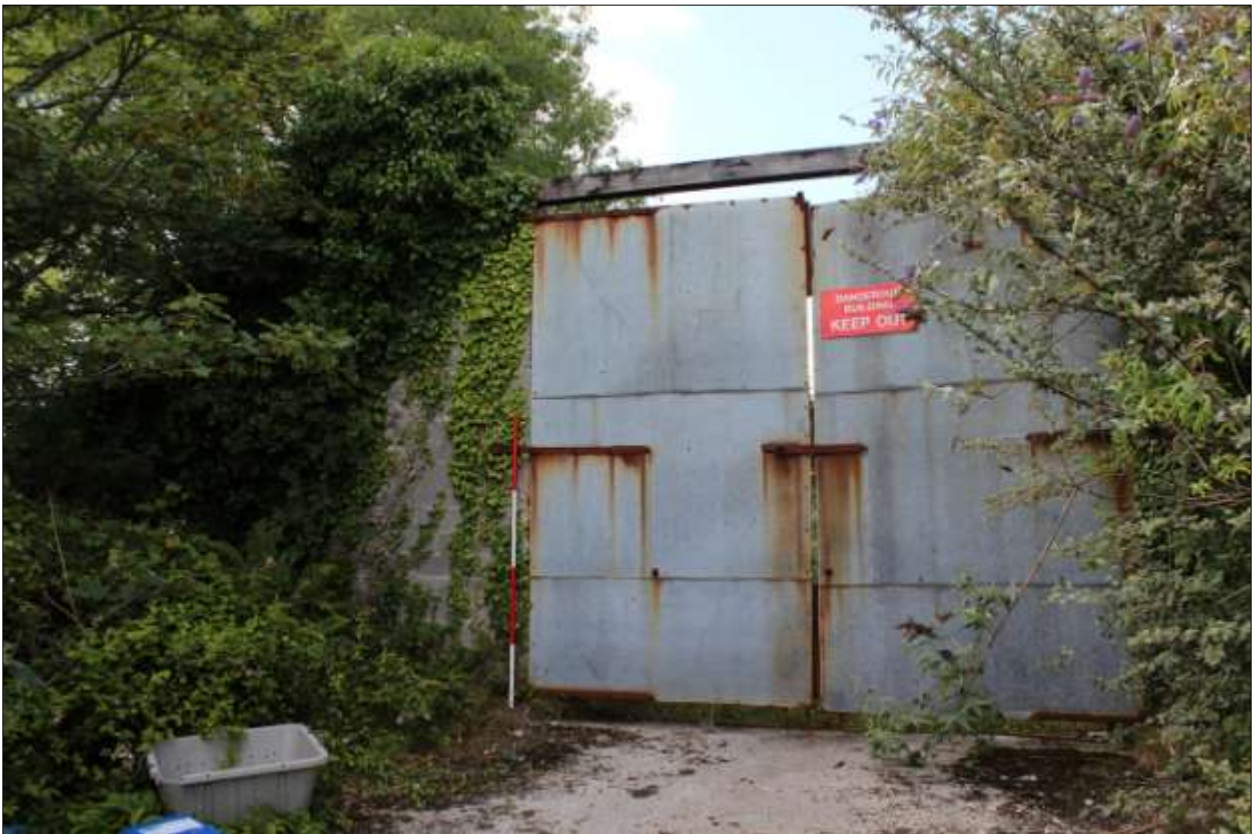
The south doors of the drying floor; viewed from the south (scale 2m).
