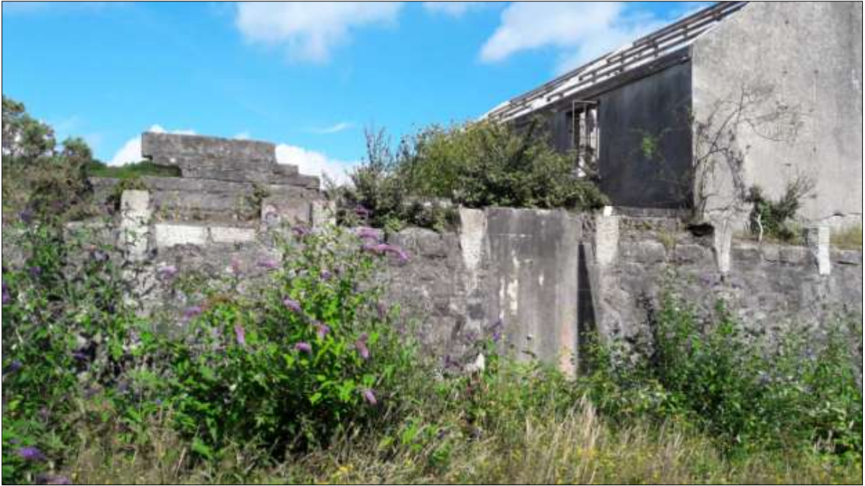
The west wall of T7, with B2 and the blocked sluice gate; viewed from the west. Note the projecting granite blocks along the wall top to carry the timber wallplate, and the extra blockwork to the left; the latter is presumably part of the building shown here on the 1969 OS map.
