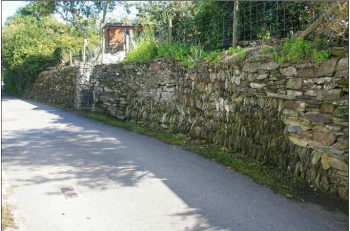
FIGURE 5: VIEW ALONG HOCKENS LANE FROM THE WEST, SHOWING THE WALL IN QUESTION.
