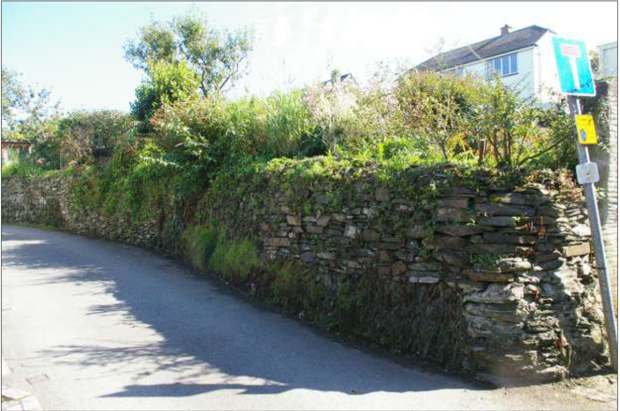
THE RETAINING WALL ON HOCKENS LANE; VIEWED FROM THE WEST. NOTE THE EXTENSIVE REBUILDING.
