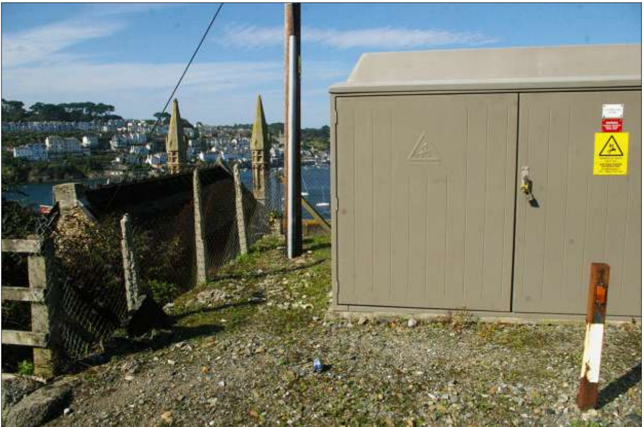
THE ELECTRICAL SUBSTATION OVERLOOKING THE LISTED CHAPEL; VIEWED FROM THE SOUTH.
