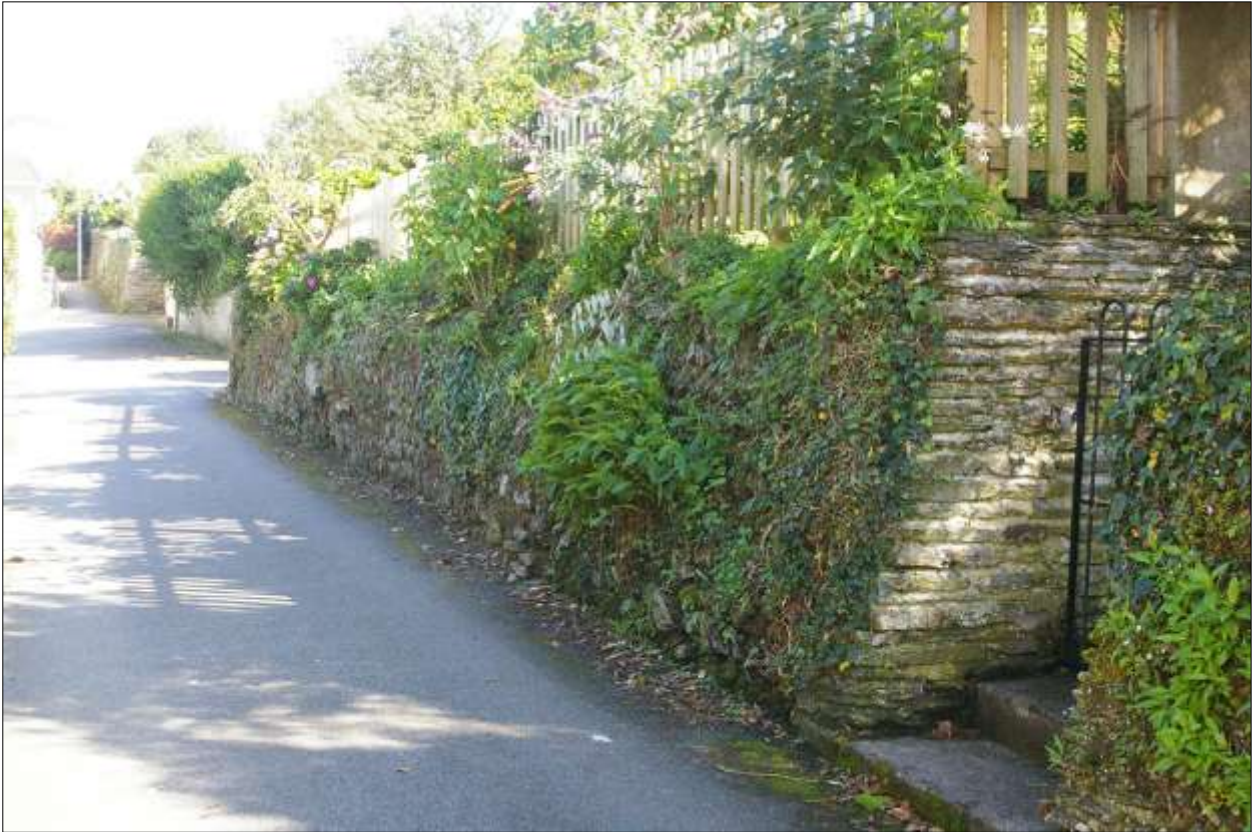
THE RETAINING WALL ON HOCKENS LANE, TOWARDS THE EASTERN END; VIEWED FROM THE WEST.
