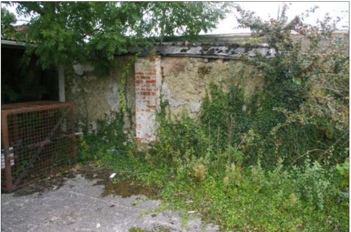
FIGURE 23: THE REMNANT STONE AND COB WALL ALONG THE NORTH-EASTERN EDGE OF THE SITE; VIEWED FROM THE WEST.
