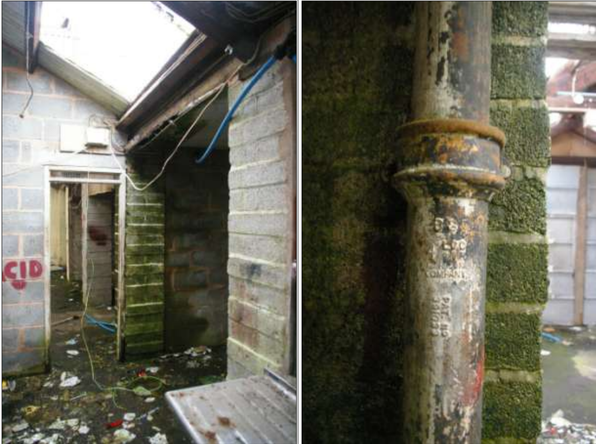
LEFT: Building 4, showing the line of concrete block pillars; viewed from the east. RIGHT: Building 4, detail of a cast iron downspout; viewed from the west.
