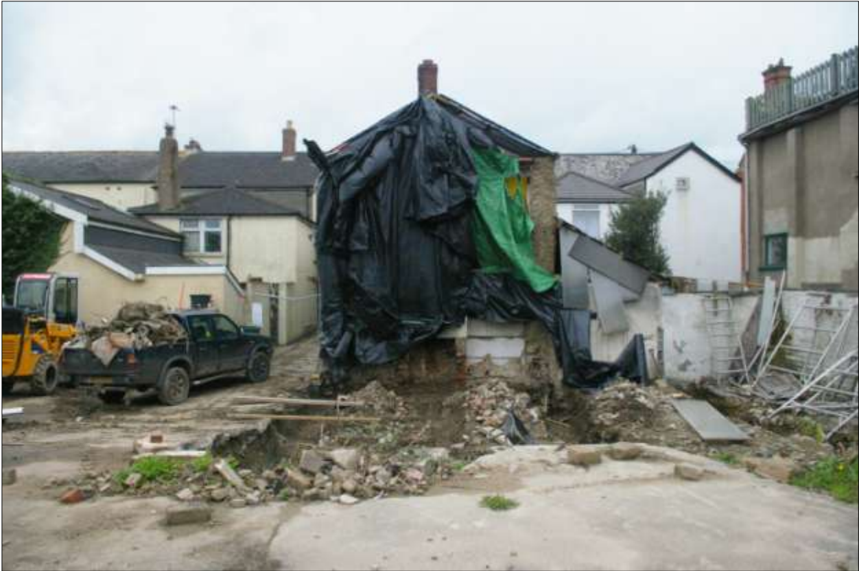
The building on Albion Place in the process of reconstruction; viewed from the east.
