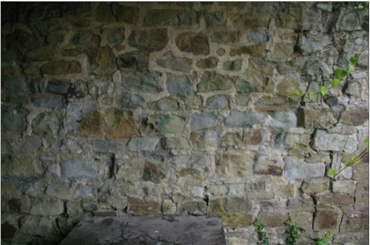
Detail of the west wall of the garages/rear wall of the burgage plots; viewed from the east.
