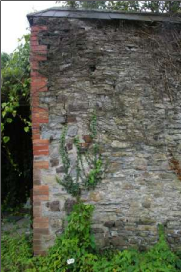
The rebuilt corner of the historic wall to the west of the central yard; viewed from the north.
