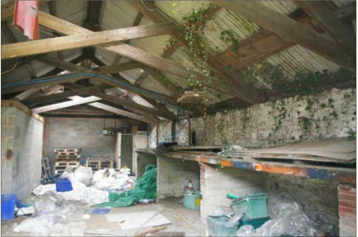
FIGURE 22: THE INTERIOR OF B3, SHOWING THE SCISSOR-TRUSSES RESTING ON A HISTORIC STONE WALL; VIEWED FROM THE EAST.
