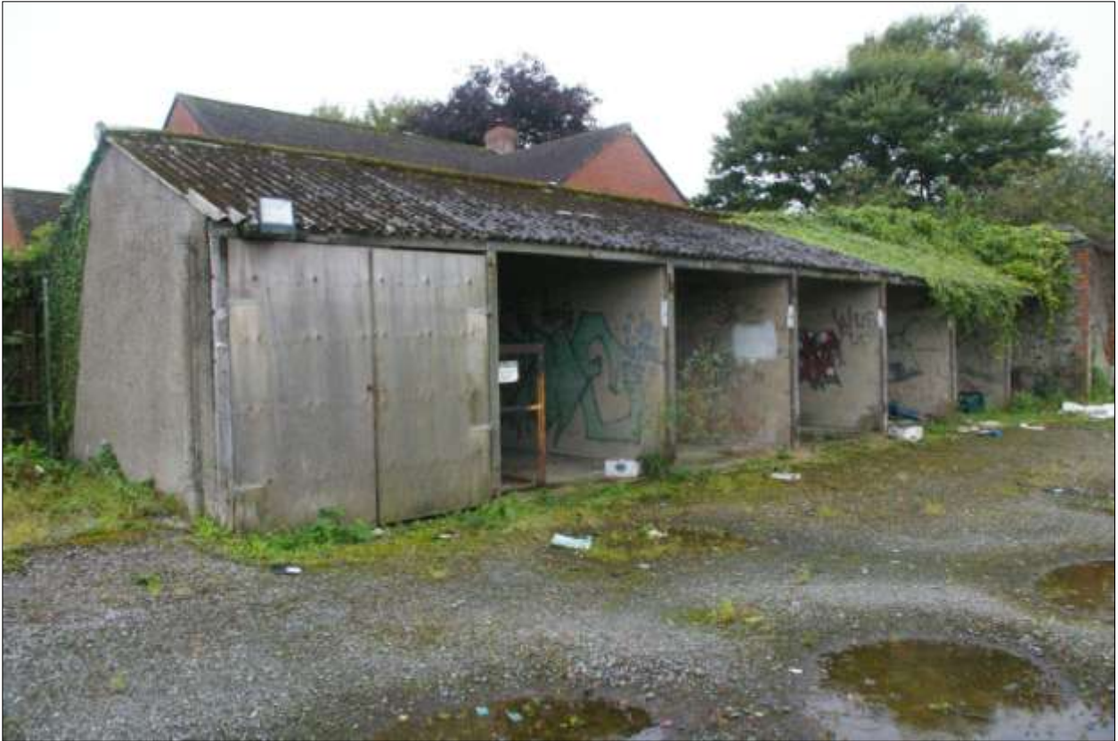
The disused garages on the southern edge of the central yard; viewed from the north-east.
