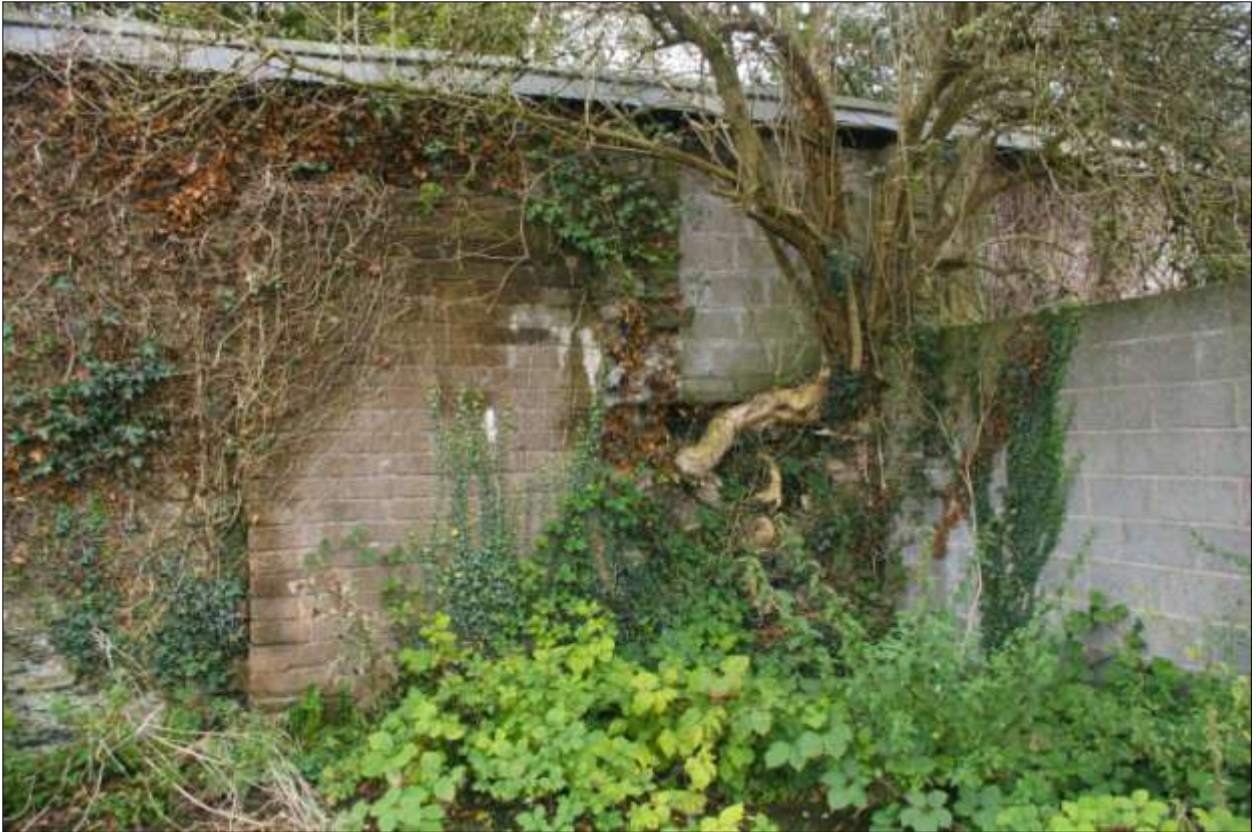
As above, showing a buttress in concrete block, and a return on the stone wall; viewed from the NNE.
