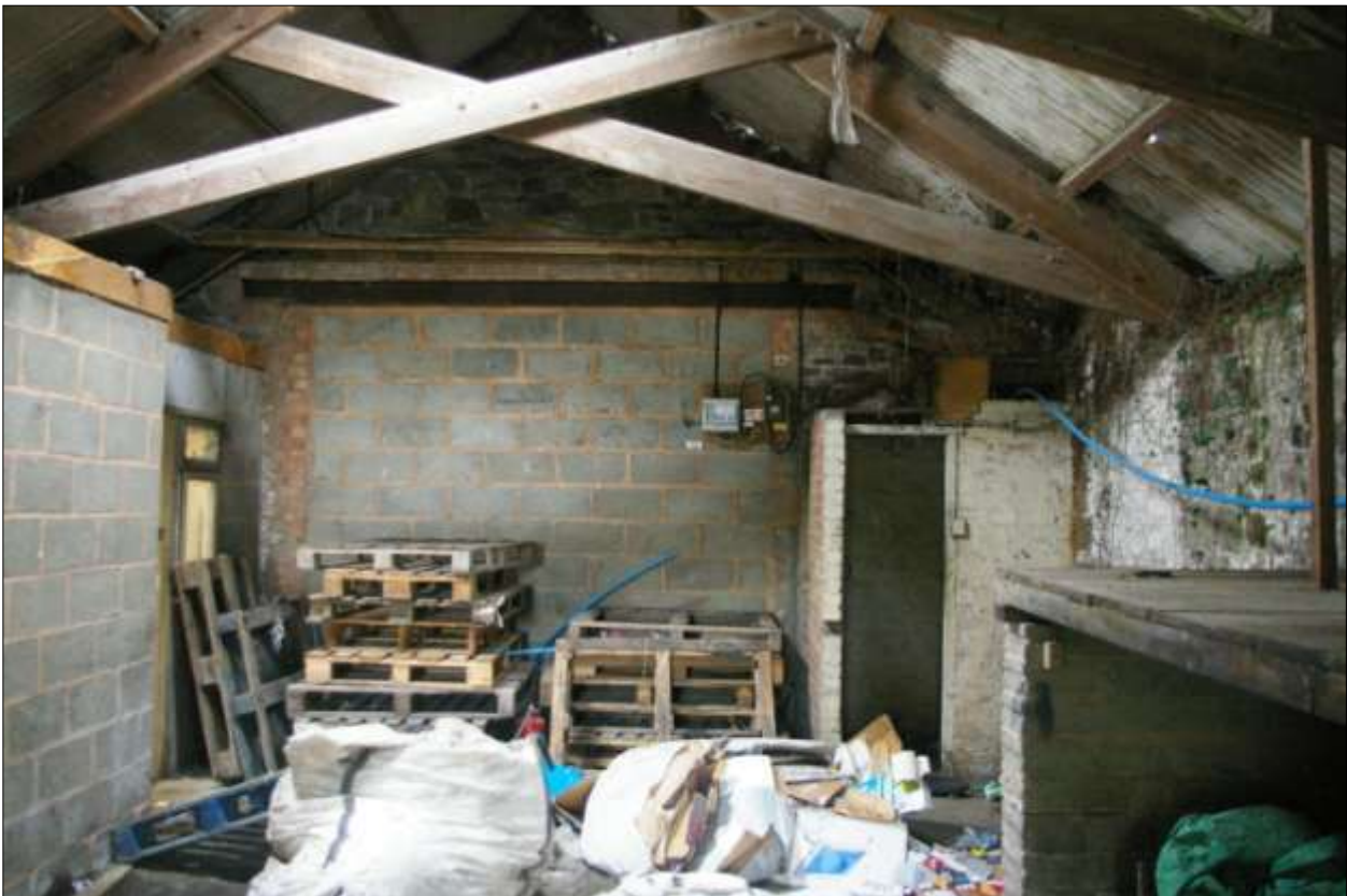
The western end of the interior of Building 3, showing the blocked forced opening in the wall of the adjacent building; viewed from the east.
