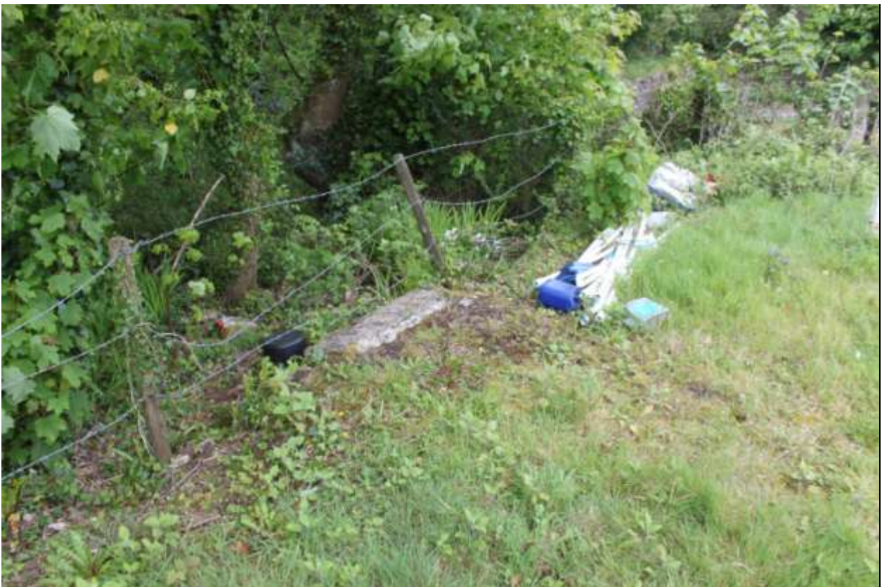
General shot of the western boundary of the southern ore yard, in poor condition, viewed from the south.
