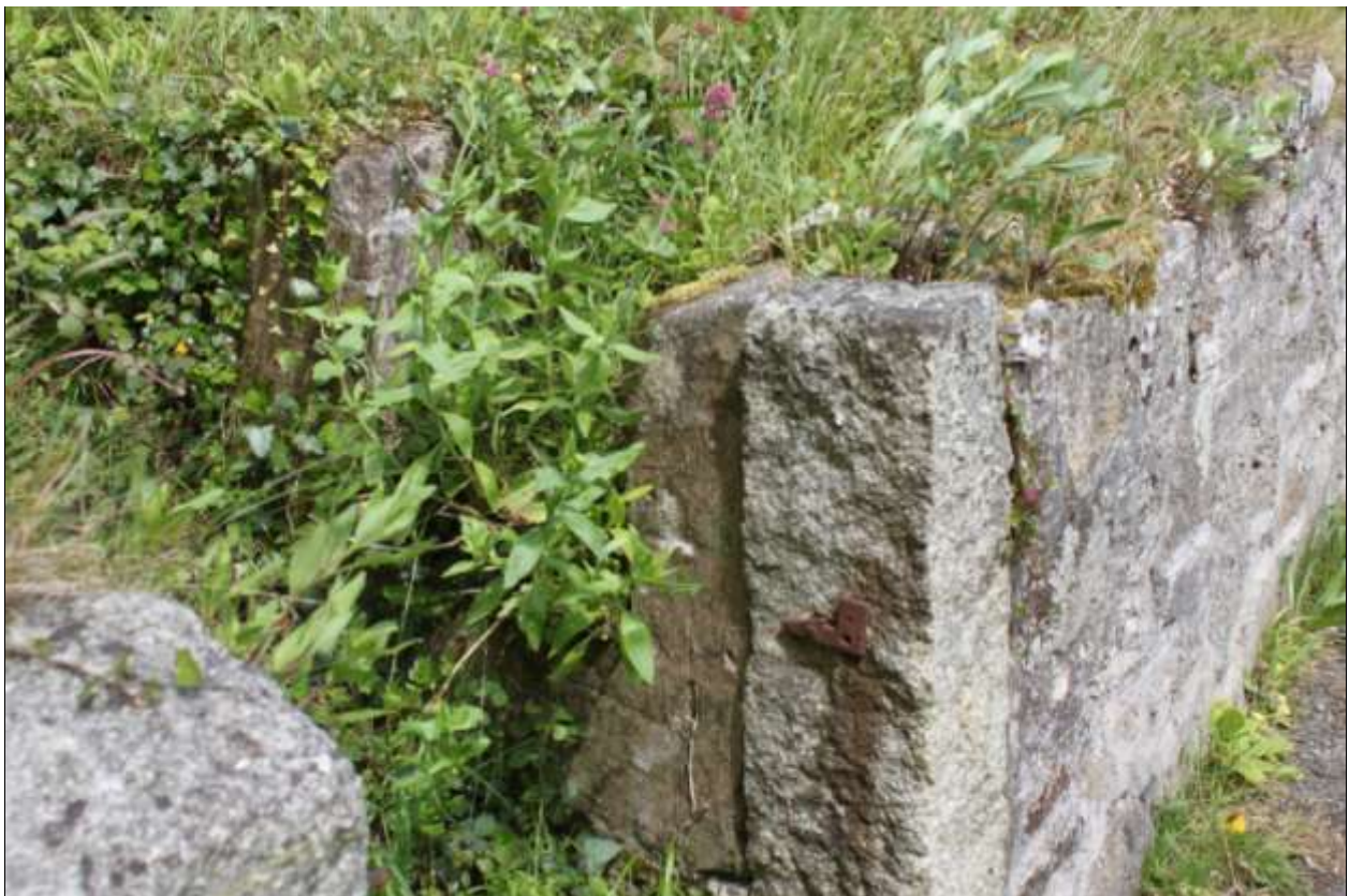
Shot showing the remains of cast iron gate fittings noted on each set of granite gate posts, and the step which led up to the eastern garden from each access point, viewed from the west-south-west.
