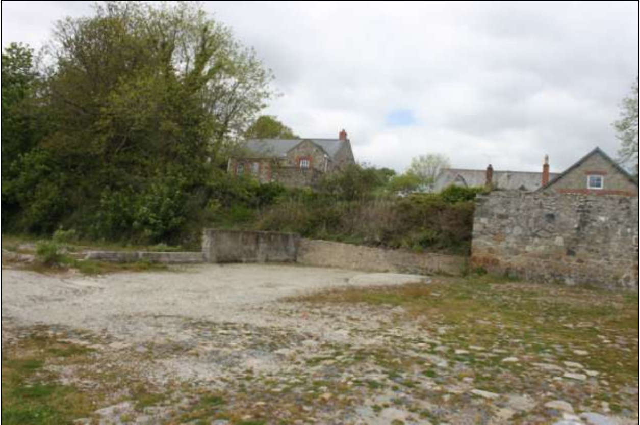
Shot of the generally better condition, though worn nature of the northern ore floor, viewed from the south.
