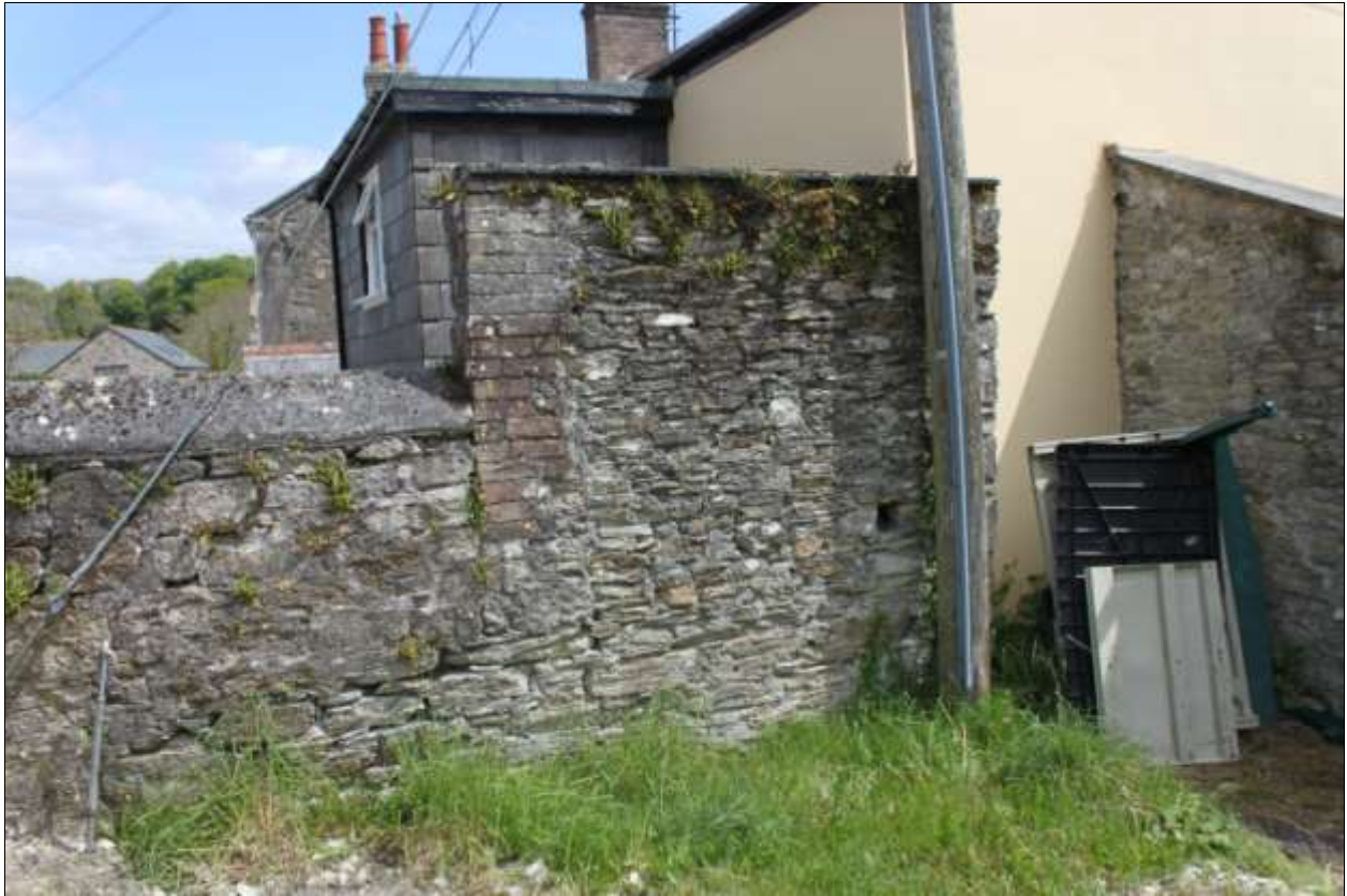
Phasing evident in the eastern boundary of the former yard, viewed from the west.
