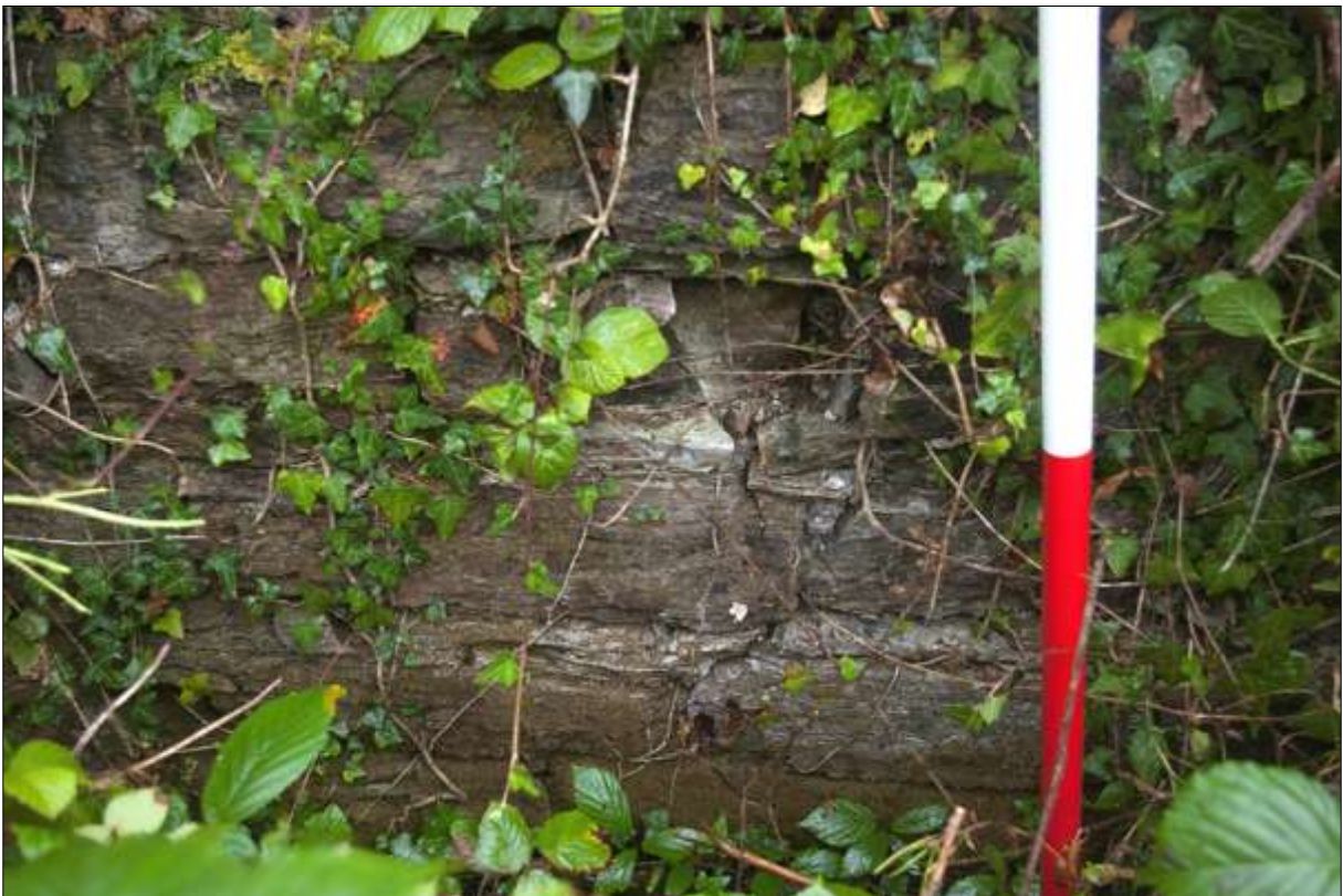
Detail of the build of the south wall of B4 (scale 2m).
