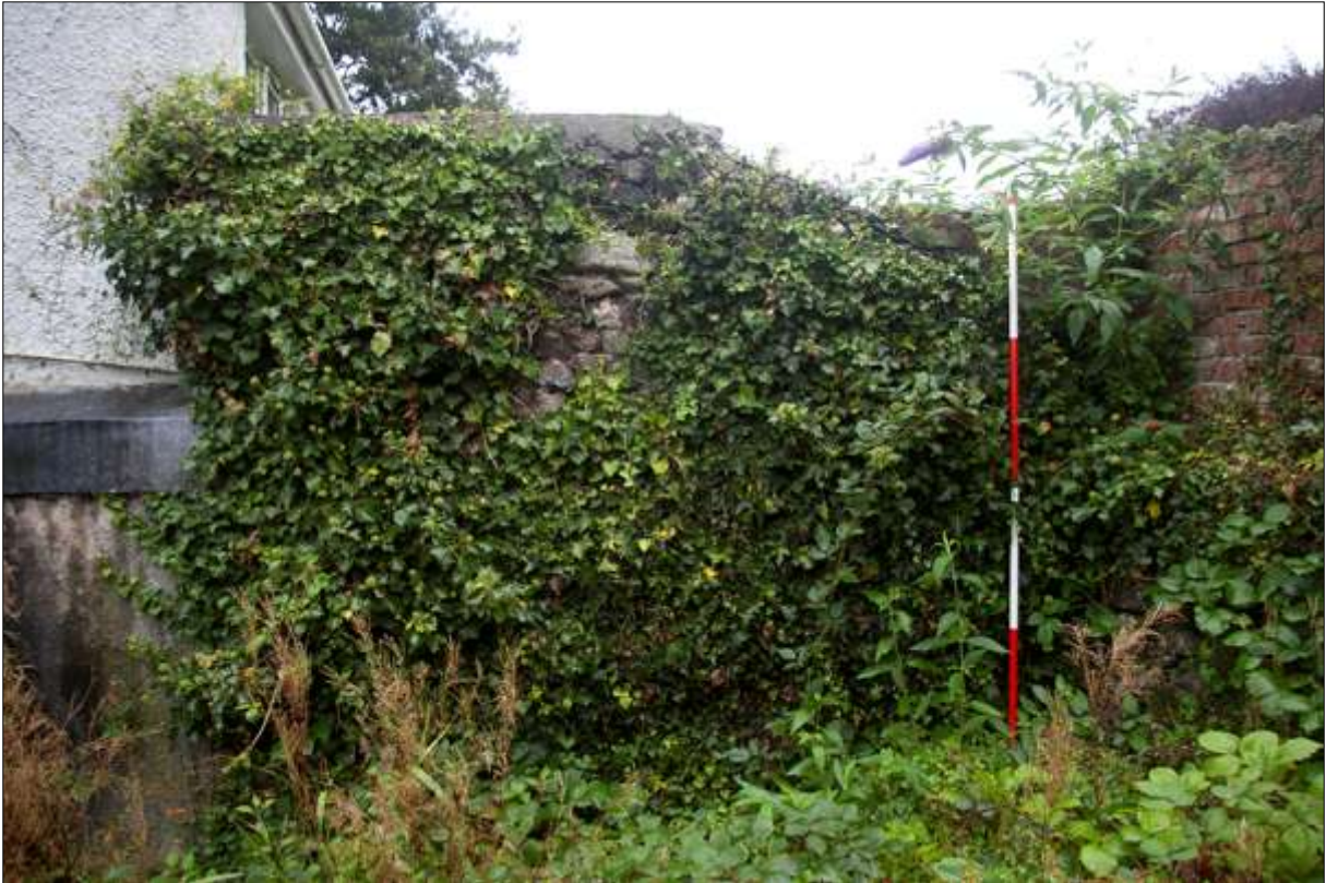
The south-east corner of B6, showing the partial survival of the gable; viewed from the north-west, looking south-east (scale 2m).
