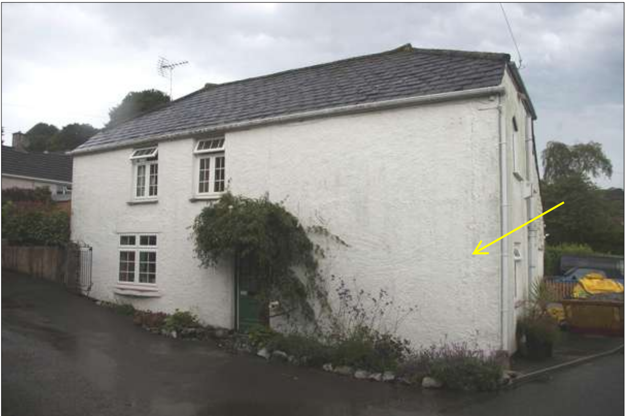
The south elevation of the house adjacent to the north; viewed from the south, looking north. Note the vertical scar in the render (indicated) which may indicate the south wall was partly open.
