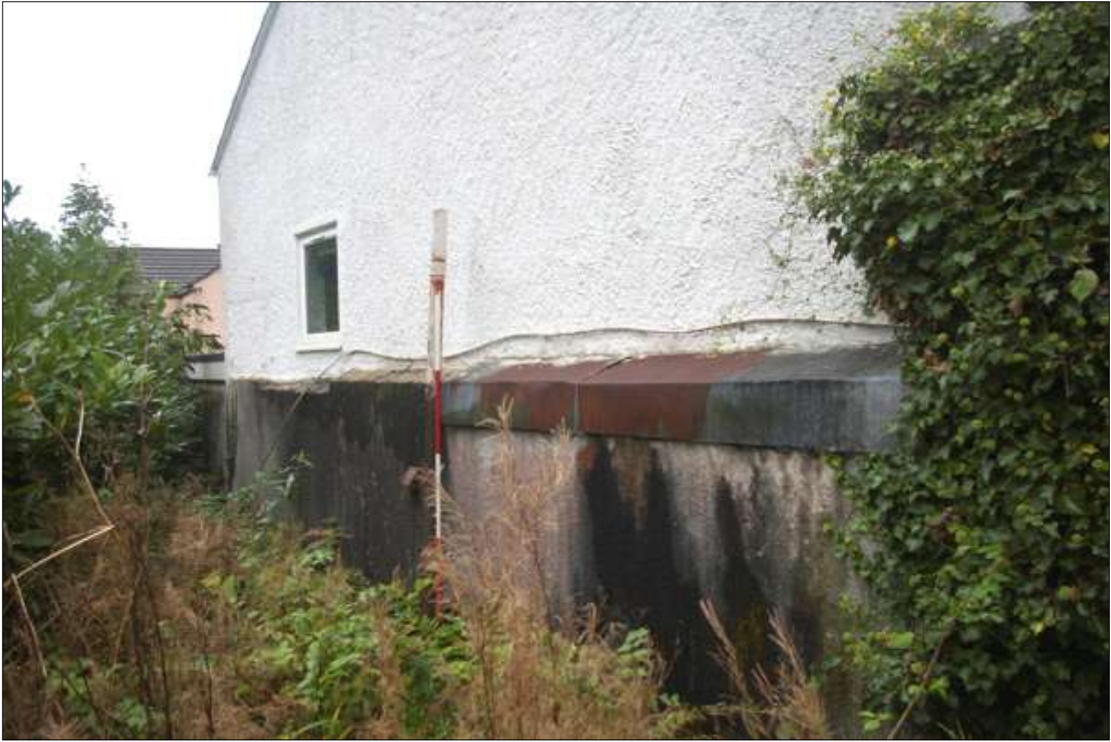
The west gable wall of the adjoining house, showing how it is built out and across the boundary wall of the property; viewed from the south, looking north (scale 2m).
