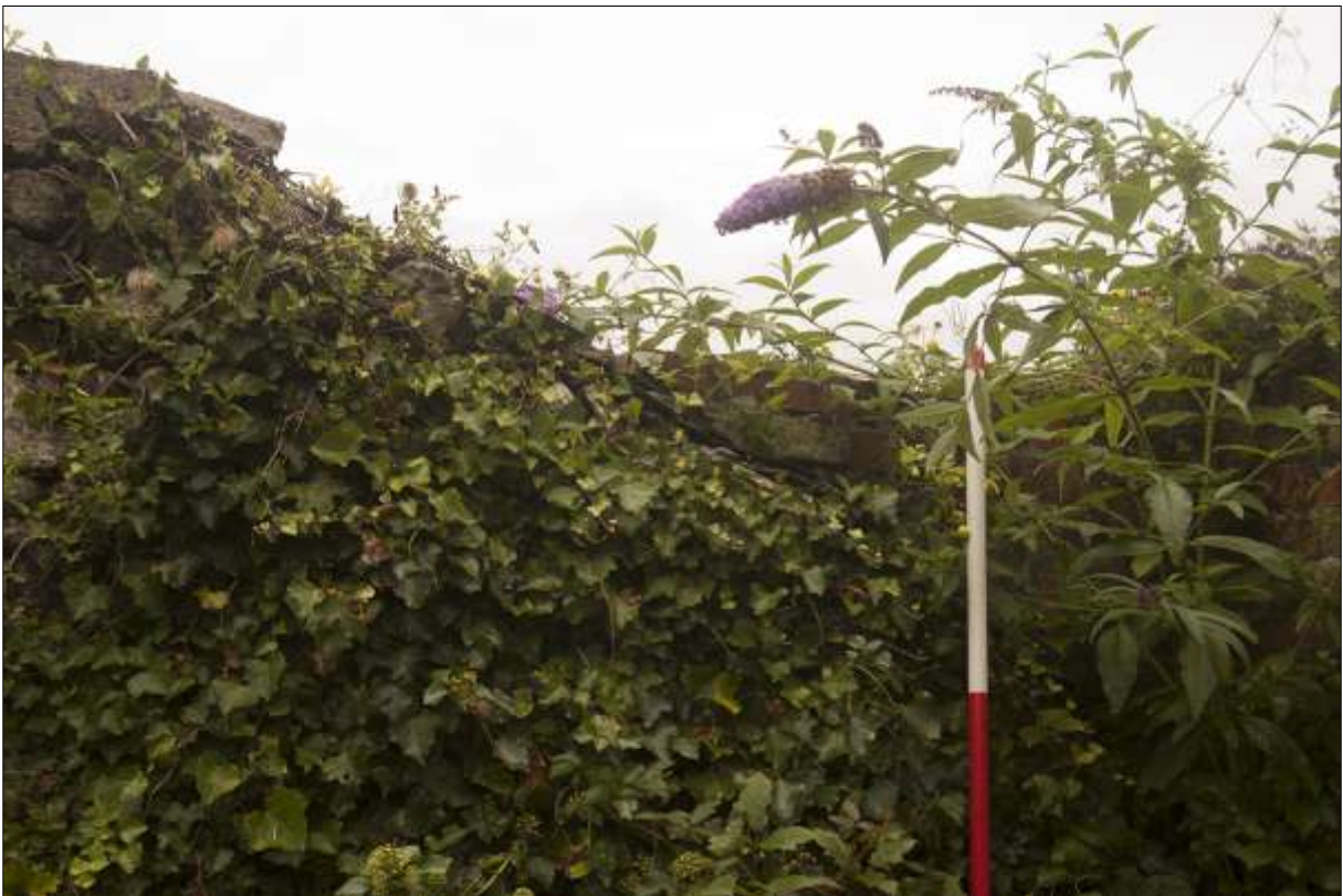
As above, detail of the slates still in situ ; viewed from the north-west, looking south-east (scale 2m).
