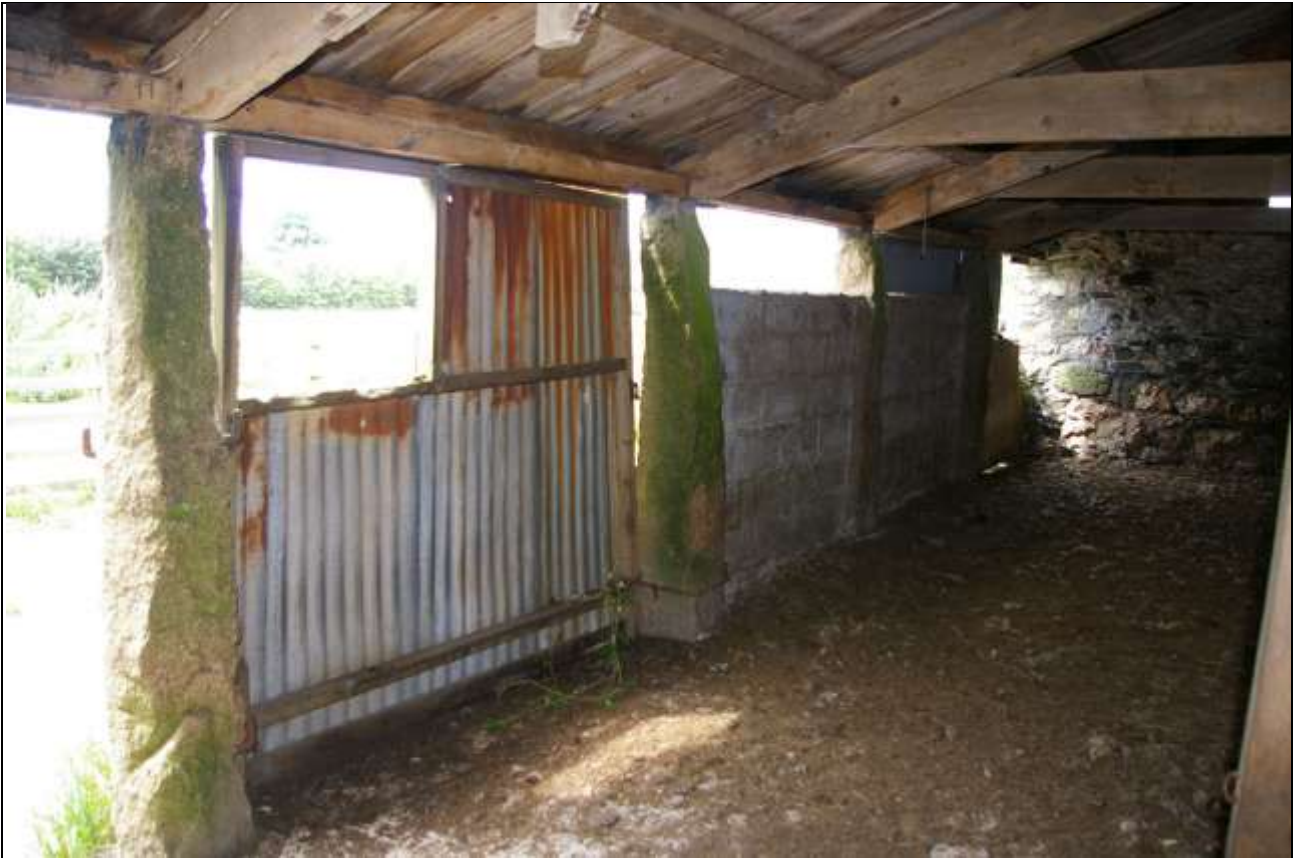
The south front of Barn 3, interior face, more clearly showing the granite piers; from the north-east corner.
