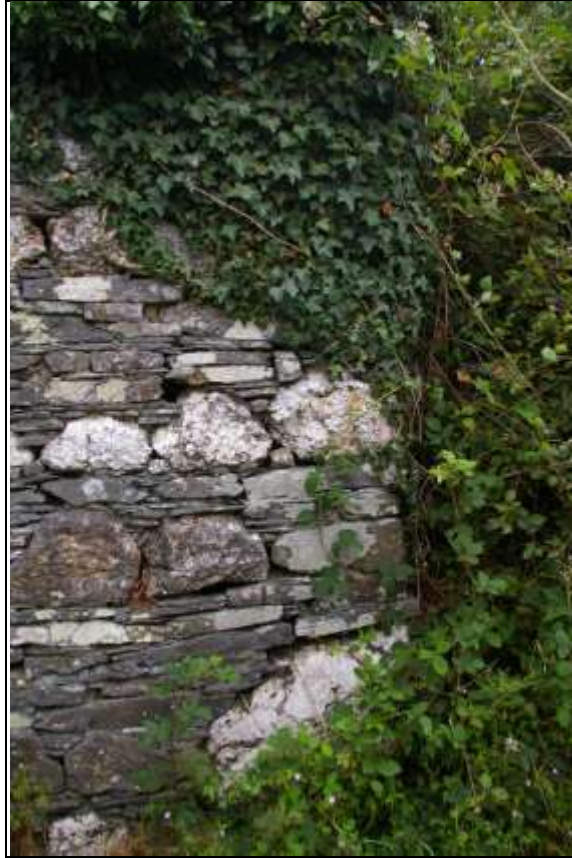
The heavy quoins to the north-east corner of Barn 1; from the east-south-east.
