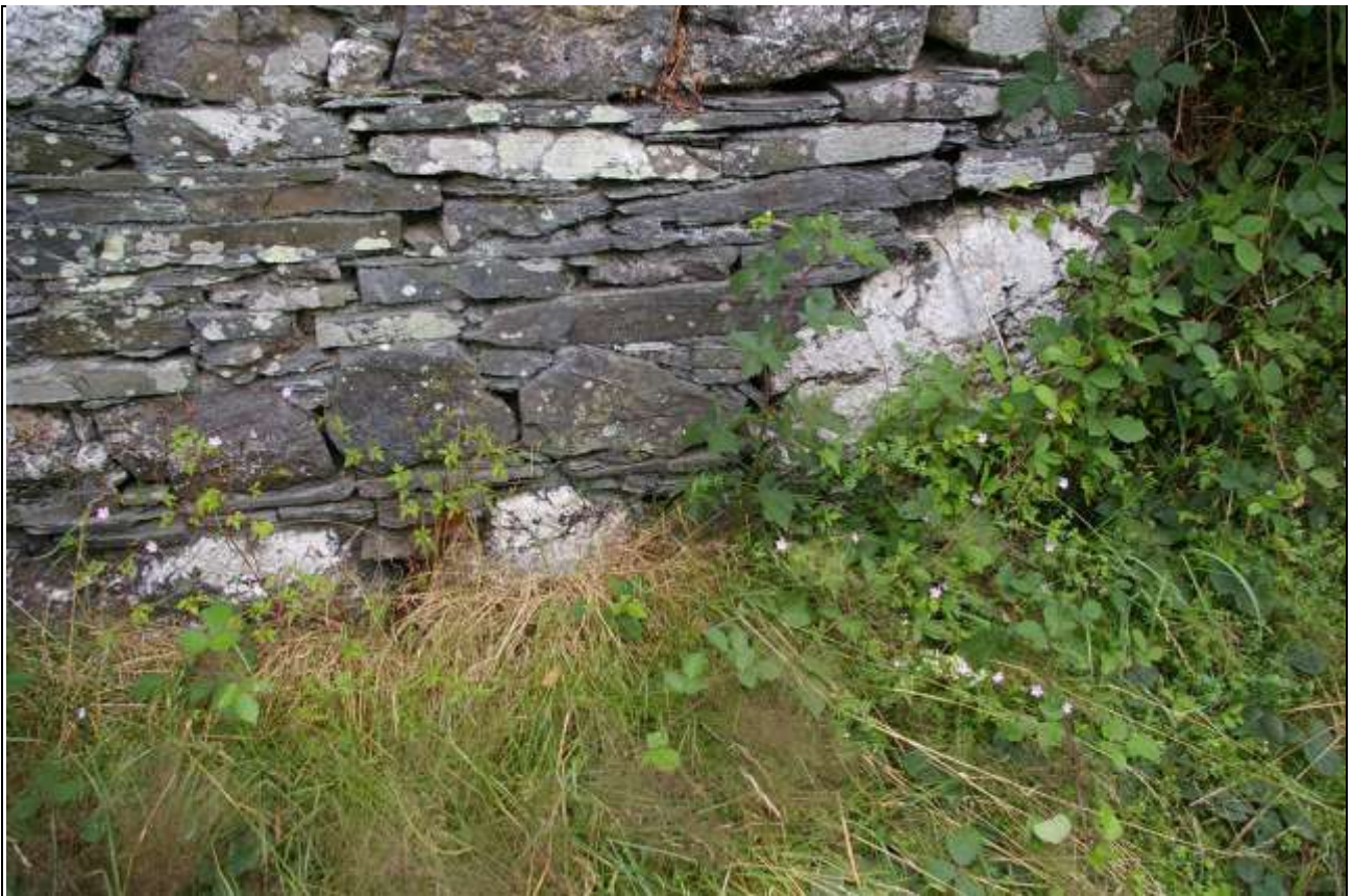
The massive quartz boulders upon which Barn 1 is built, seen in the east elevation; from the south-east.
