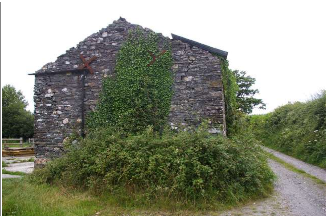
The south elevation of Barn 2, with x-ties and large structural cracks. The change in roofline is very clear; from the south-east.
