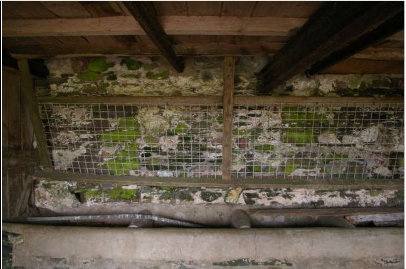
The interior face of the east elevation of Barn 2, with blocked doorway defined by former quoins; from the west.
