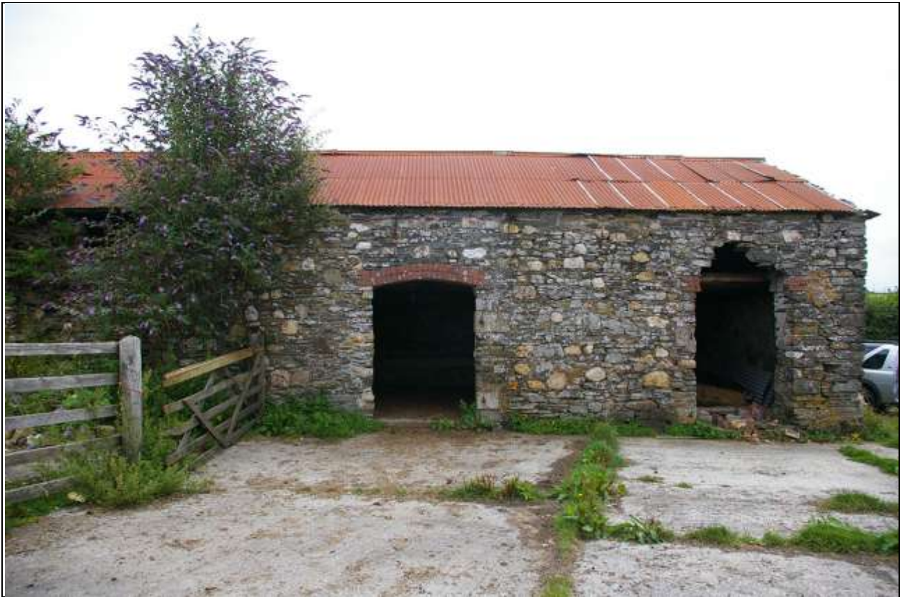
The west elevation of Barn 2, with pair of stables doors facing the yard; from the west.
