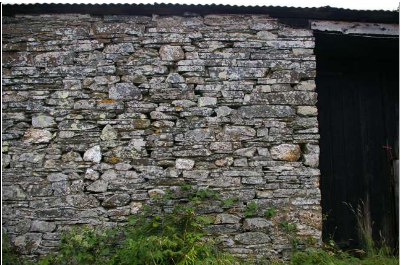
The stonework just south of the threshing door in the east elevation of Barn 1, with less quartz and a lack of formal courses; from the east.
