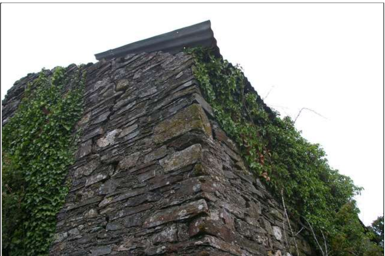
The slatestone quoins in the south-east corner of Barn 2, with two small dressed and faced formal grey limestone type blocks used in the quoins from elsewhere, one which may have been carved; from the south-east.
