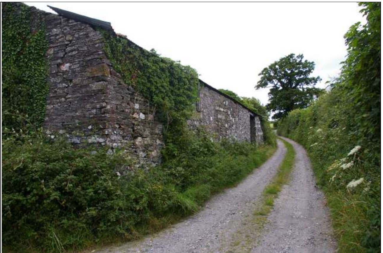
The east elevation of the barn range and farm lane; from the south-south-east.
