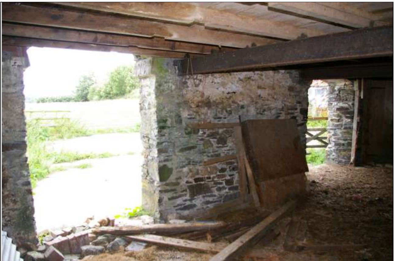
Interior face of the west wall of Barn 2, with two heightened doors; from the south-east corner.
