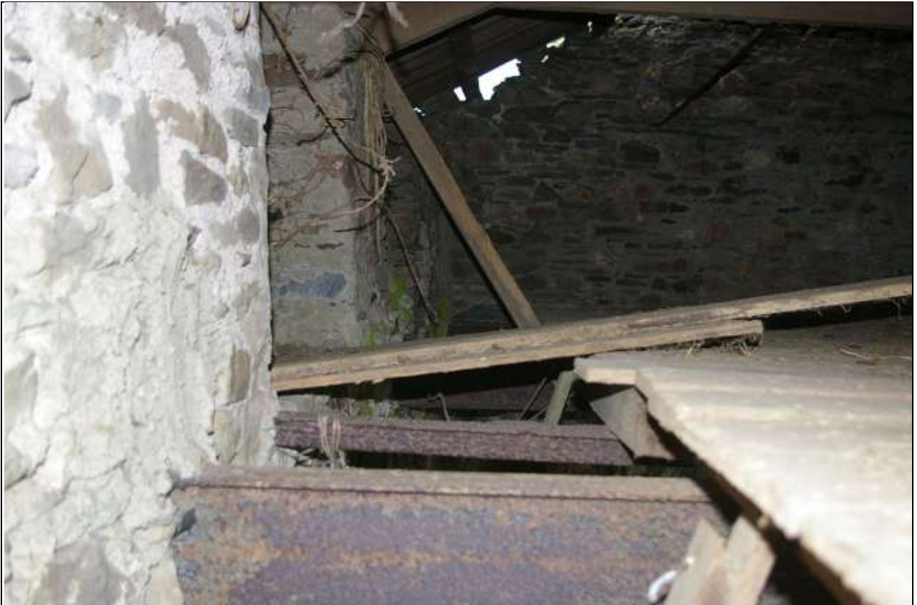
View along the east elevation of Barn 2, showing that it has been reduced in height and the ragged top of the south elevation; from the north.
