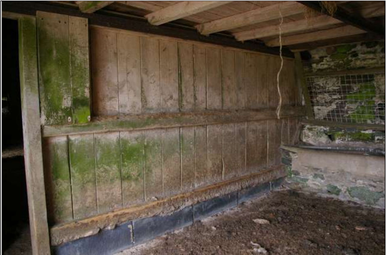
The timber partition between Barn 1 and Barn 2, viewed from within Barn 2; from the west-south-west.
