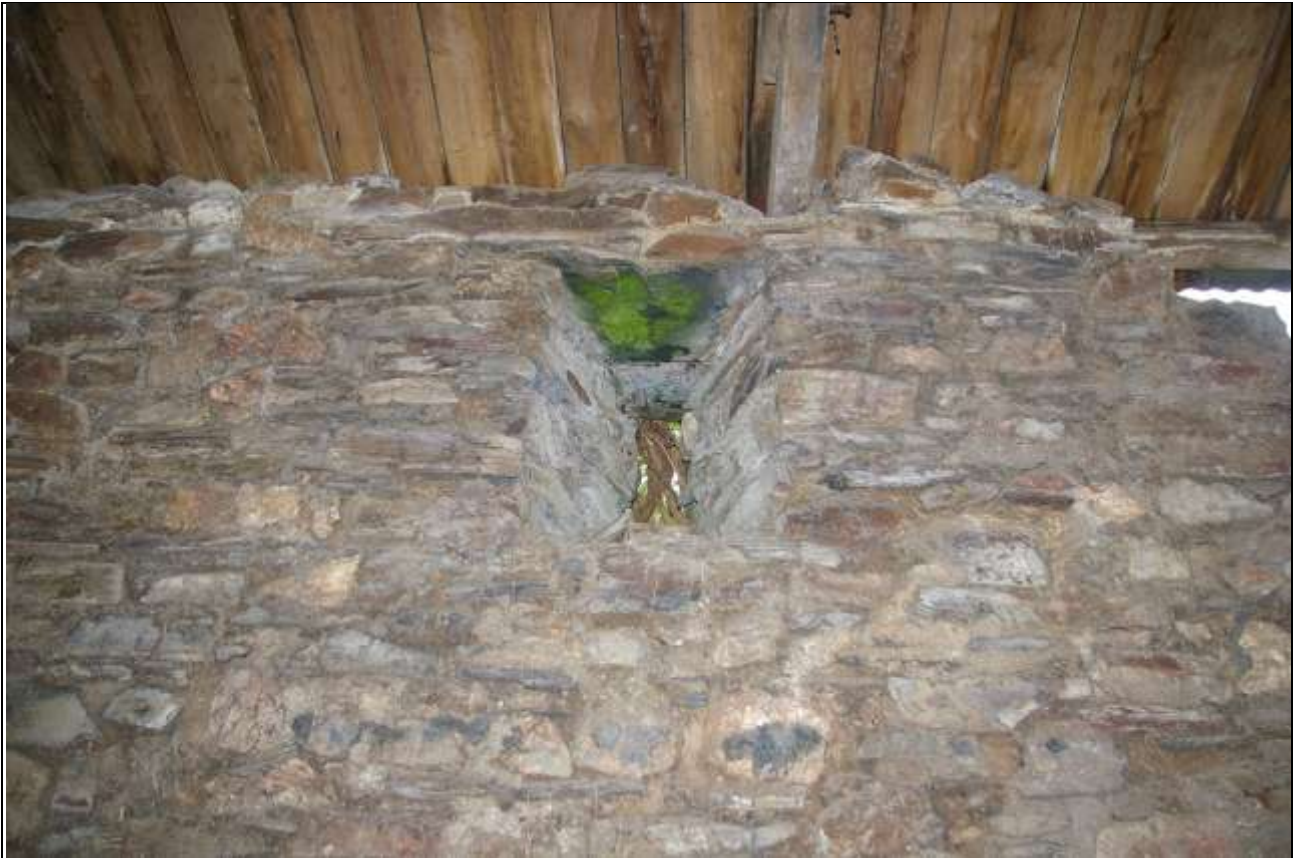
The interior face of the slit air vent in the west wall of Barn 1; from the east.
