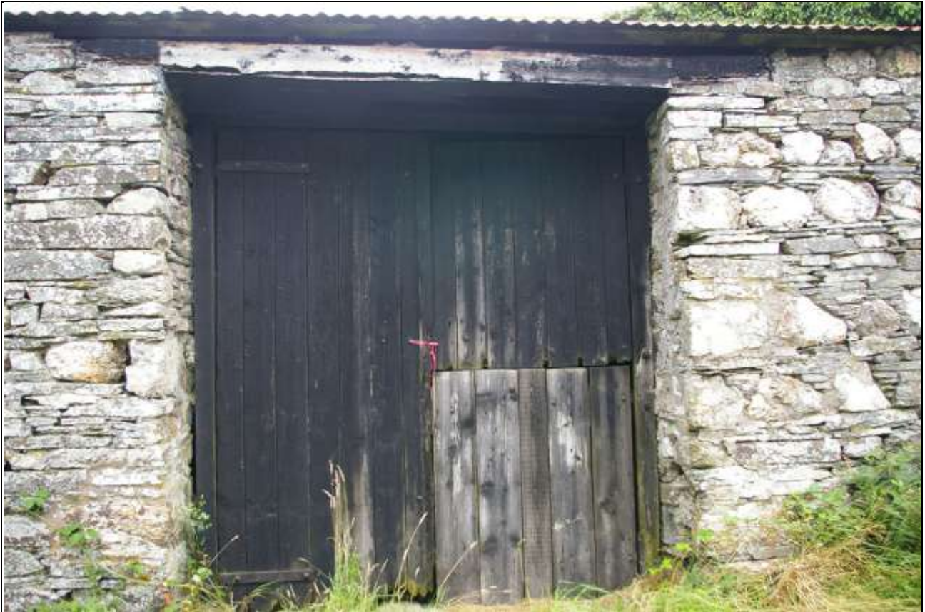
The threshing doors in the east elevation of Barn 1; from the east.
