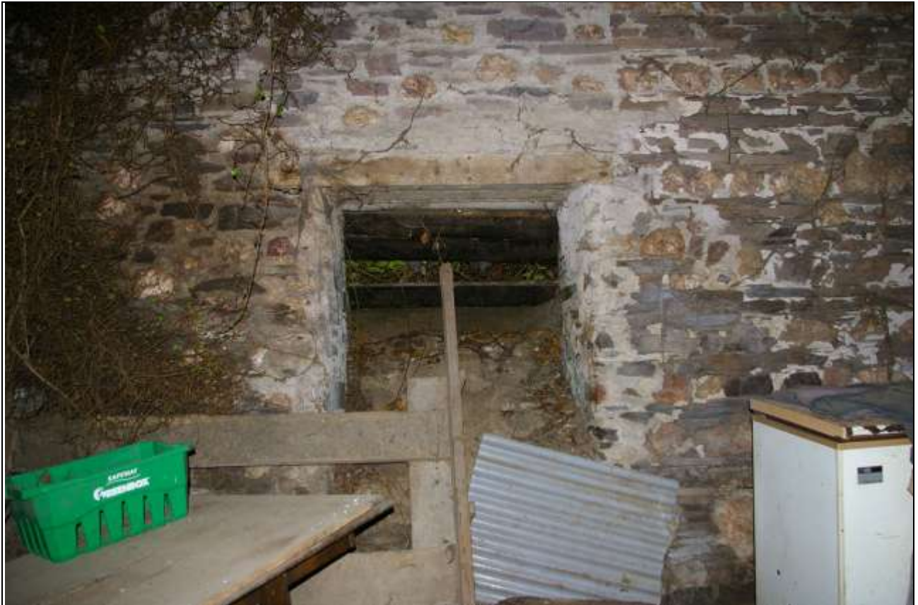
The opening in the north elevation, possibly forced as sides rebuilt and patched with cement; from the south.
