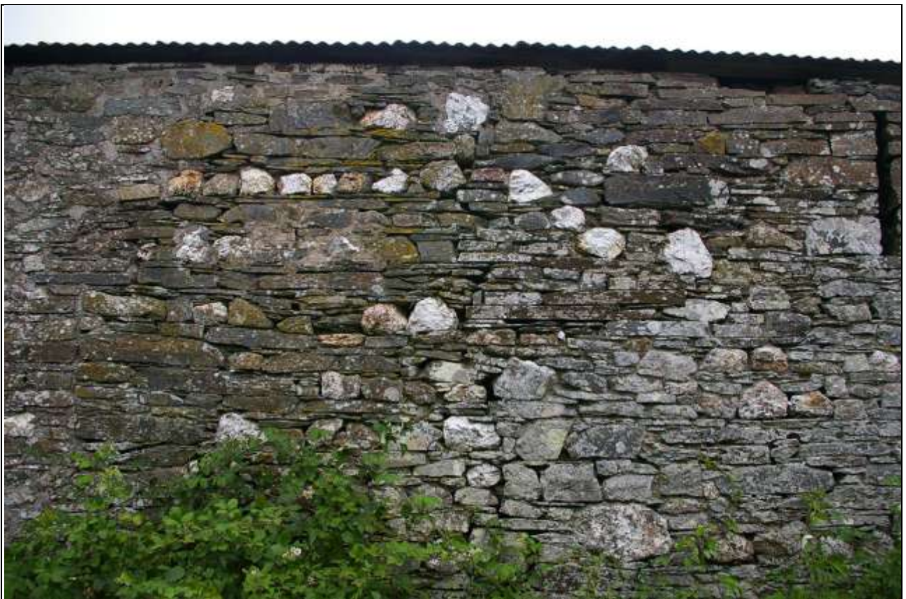
The better section of stonework in the east elevation of Barn 2; from the east
