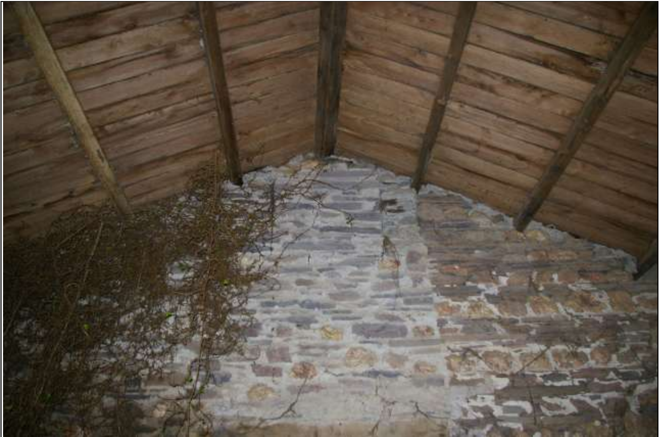
The slit air vent blocked in the north gable end of Barn 1, showing the roofline has been altered and the elevation reduced; from the south.
