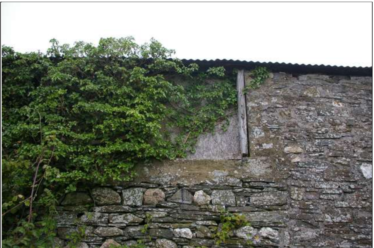
The forced loading door opening in the east elevation of Barn 2; from the east.
