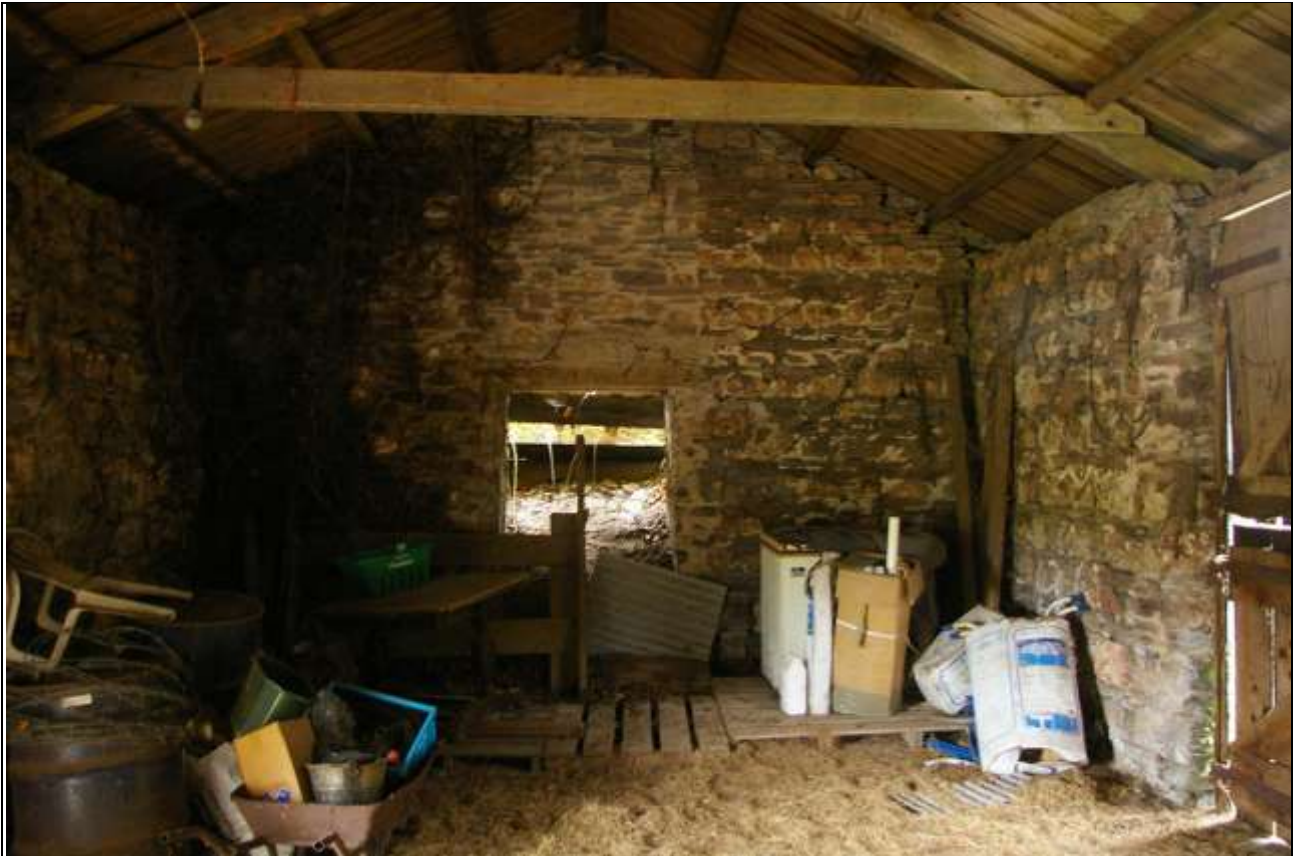
The better quality formally coursed slate slab and quartz stonework to the north end of Barn 1; from the south.
