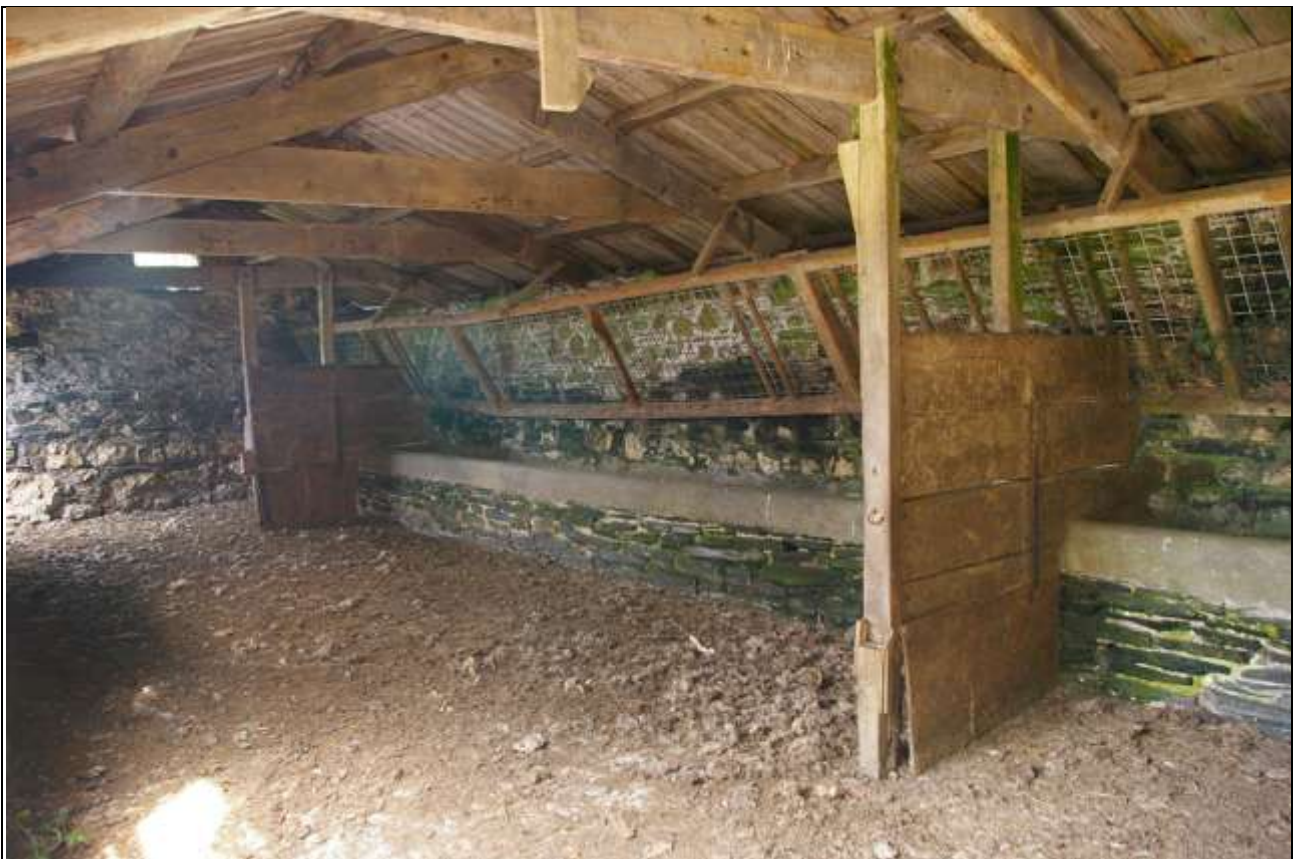
The north wall of Barn 3 and later troughs, hay ricks and partitions; from the south-east.
