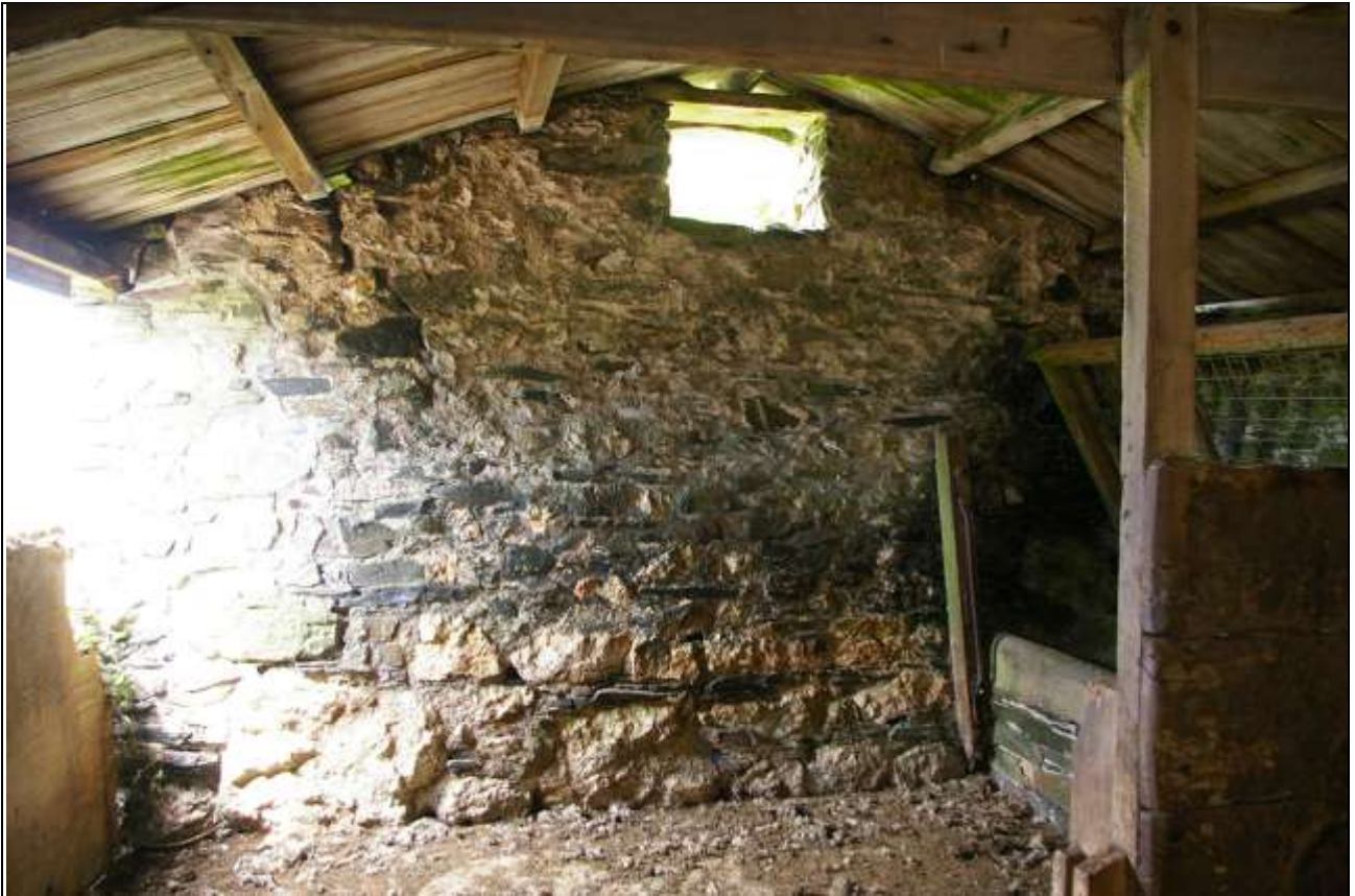
The interior face of the west gable end wall of Barn 3; from the east-south-east.
