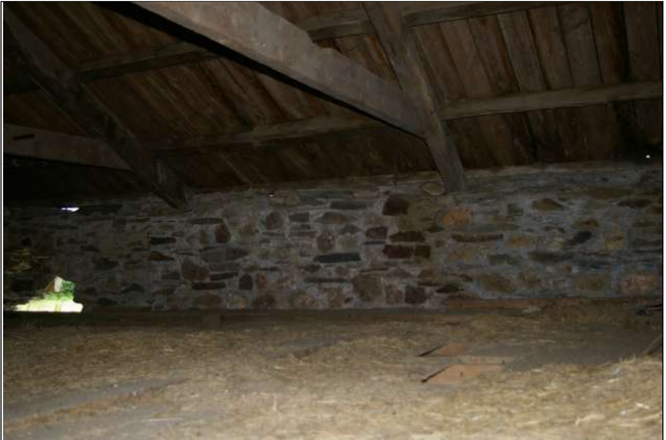
The upper west elevation of Barn 2, showing the blocked air vent, the repairs and that the elevation has been lowered; from the north-east.
