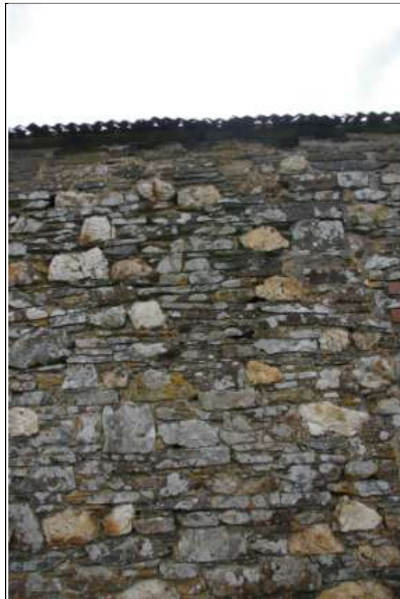
Area of disturbed slatestone which may indicate a blocked air vent in the west elevation of Barn 2; from the west.
