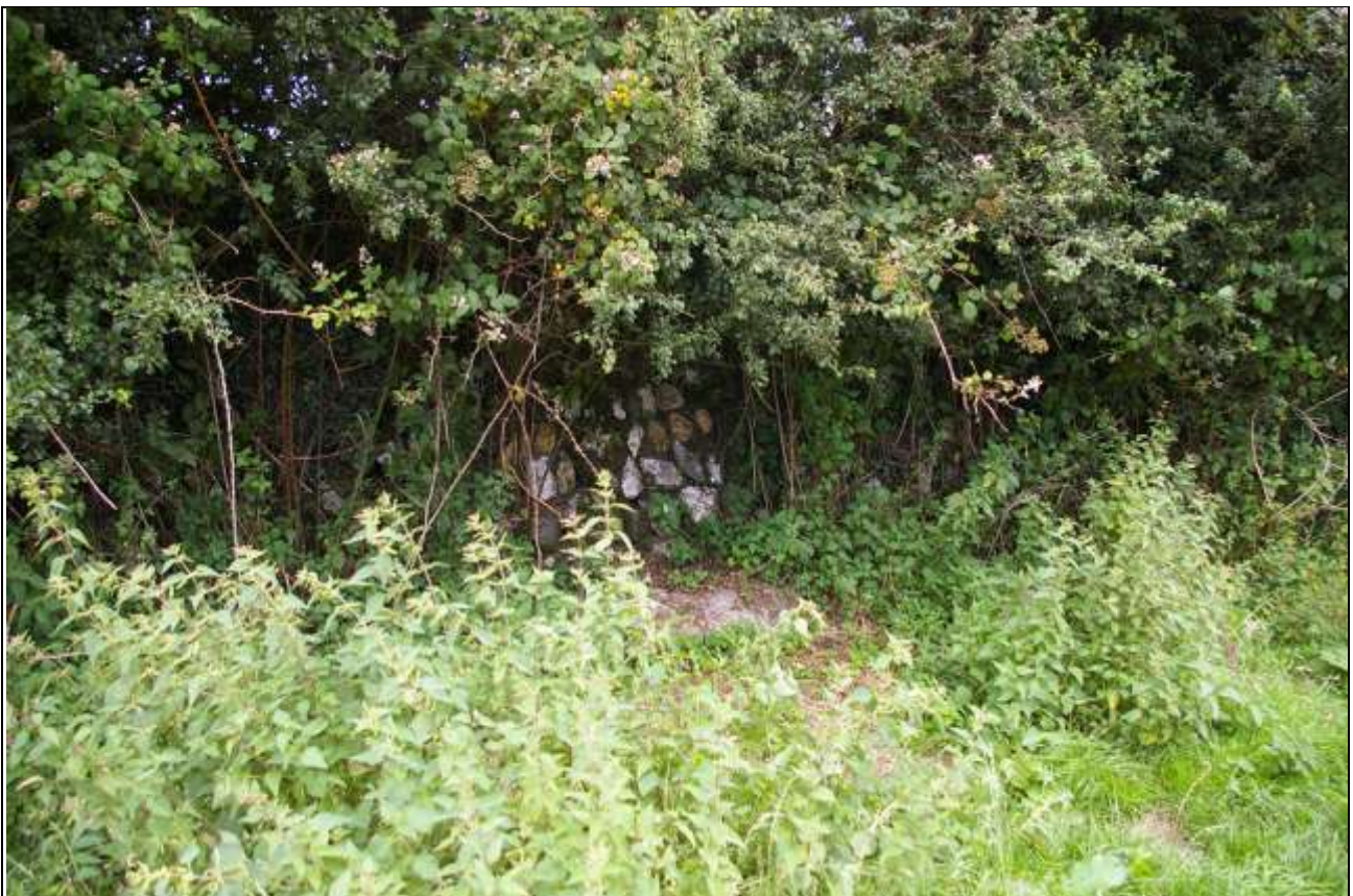
The quartz and stone build of the adjacent hedgebank, similar in style to the barns; from the south.
