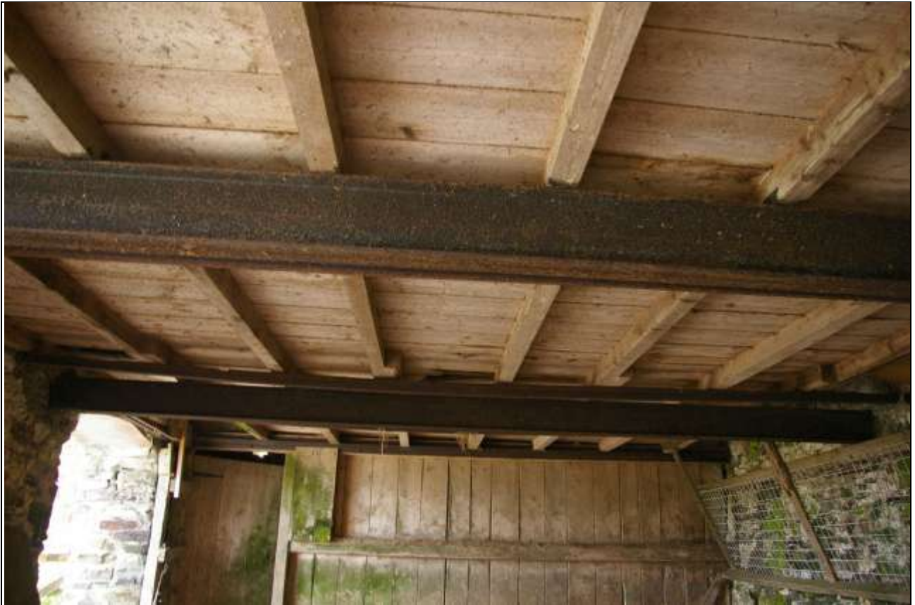
View of the iron girders and loft floor in Barn 2; from the south.
