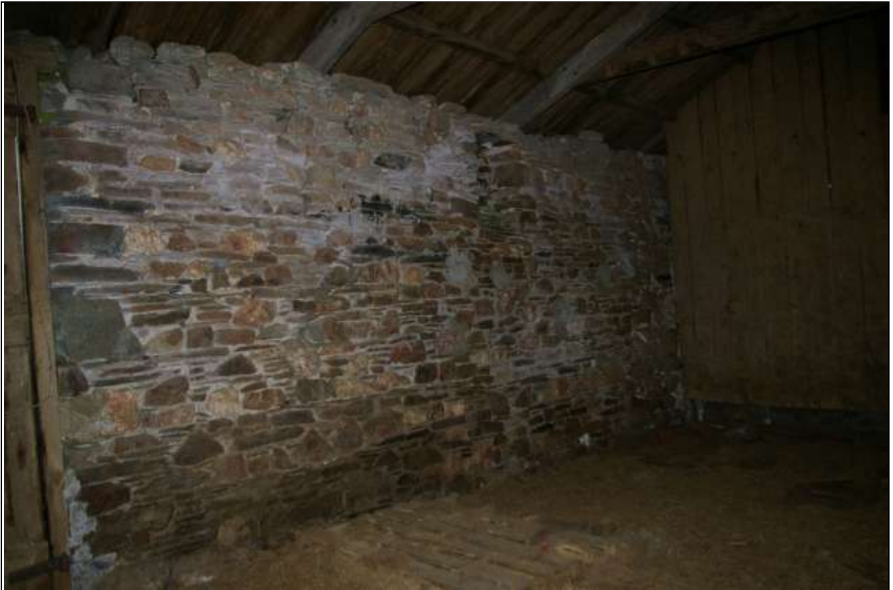
The inner face of the east wall of Barn 1, of similar quality to that to the north end; from the north-west corner.
