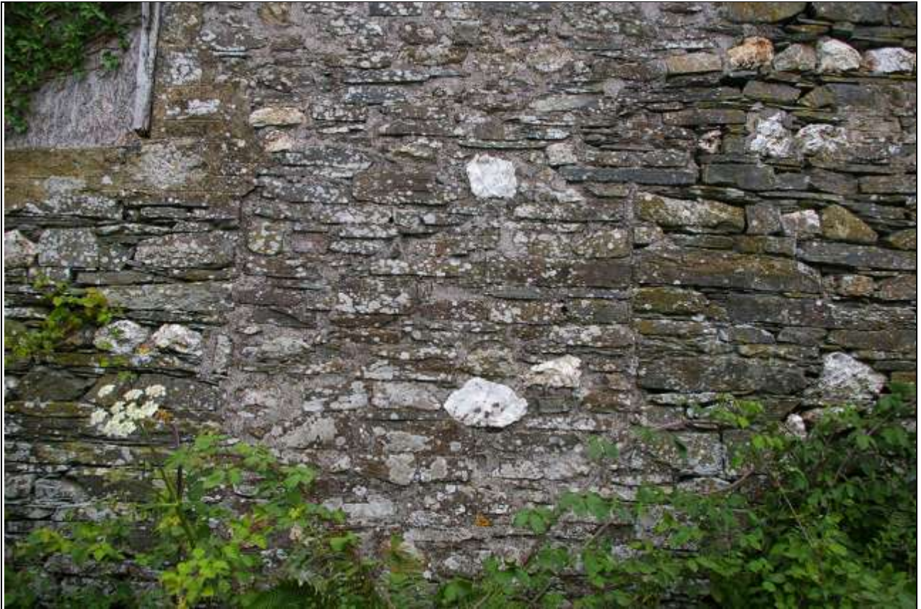
The blocked doorway in the east elevation of Barn 2; from the east.
