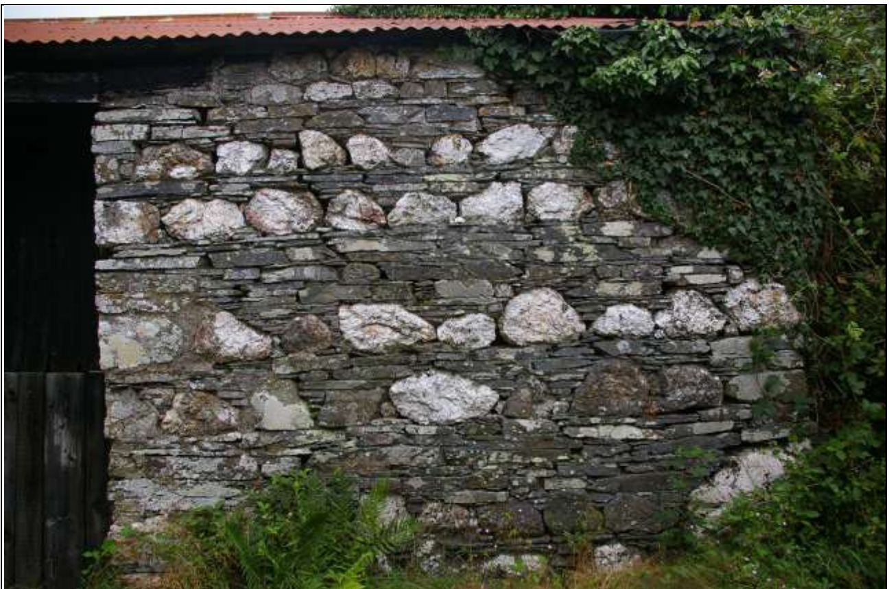
The east elevation of Barn 1, north end with coursed stonework; from the east.
