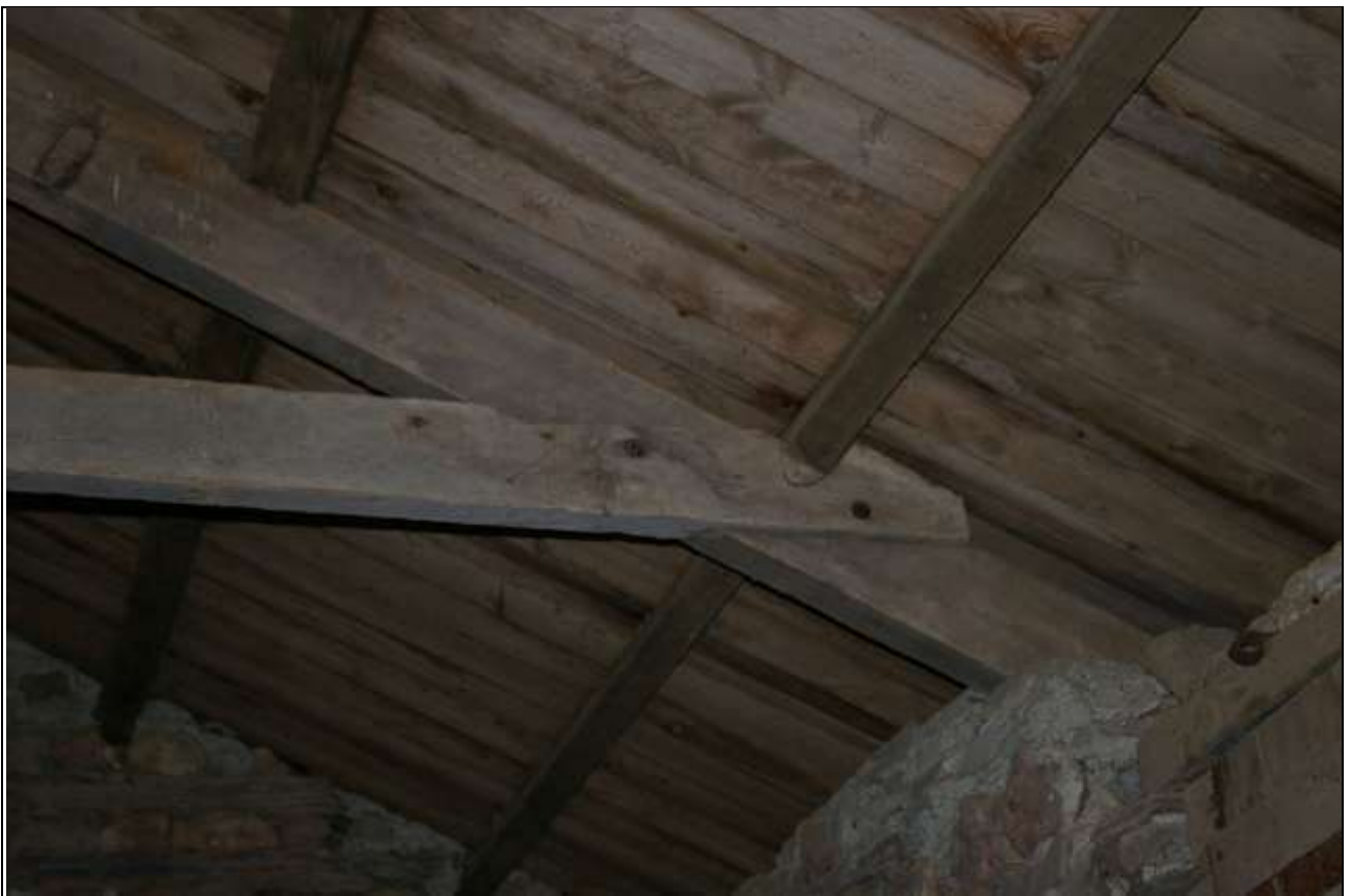
The notched lap joint to the collars, in Barn 1; from the south-west.
