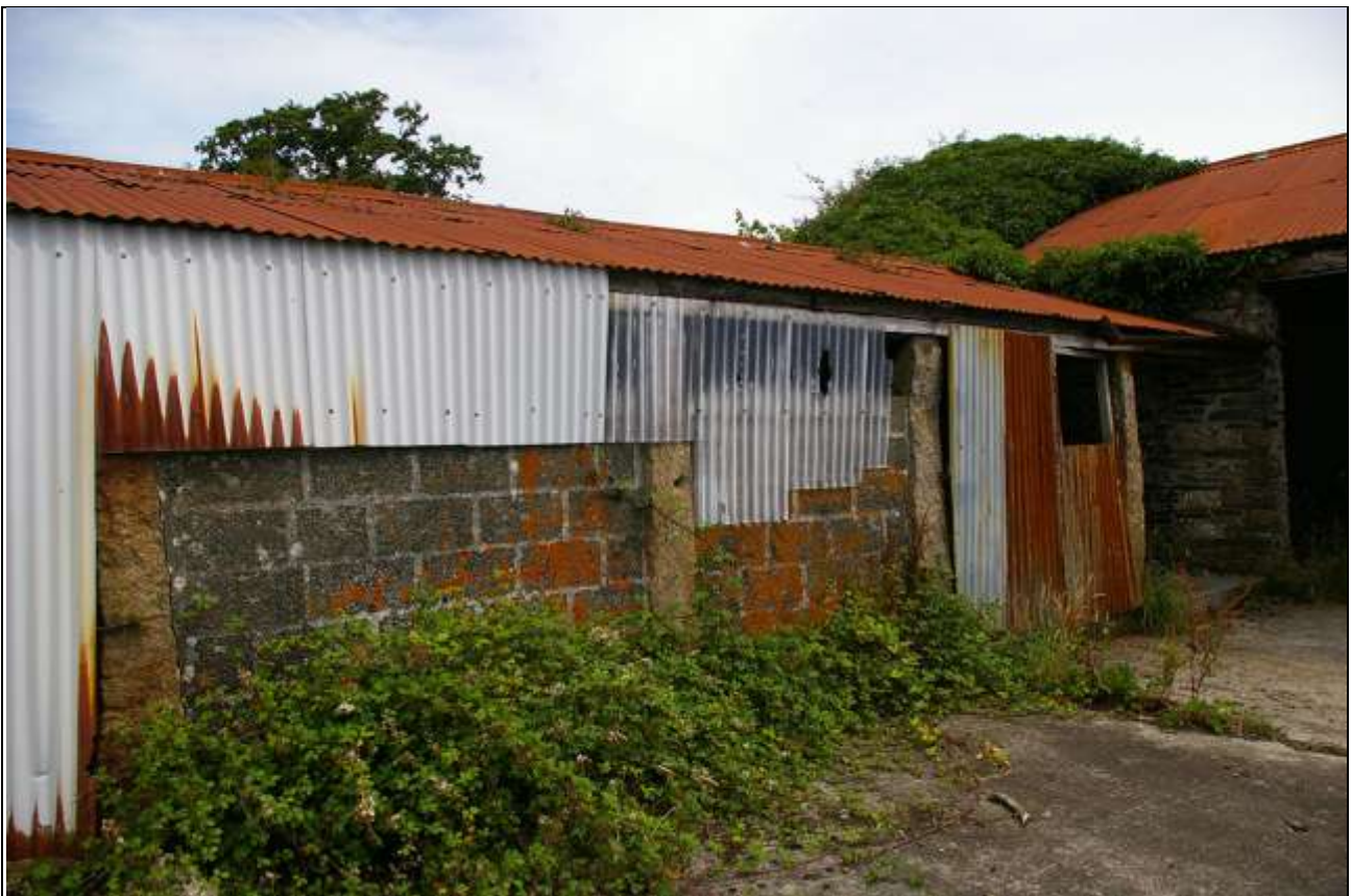
The south open-front of Barn 3, infilled with corrugated sheeting and concrete blocks; from the west-south-west.
