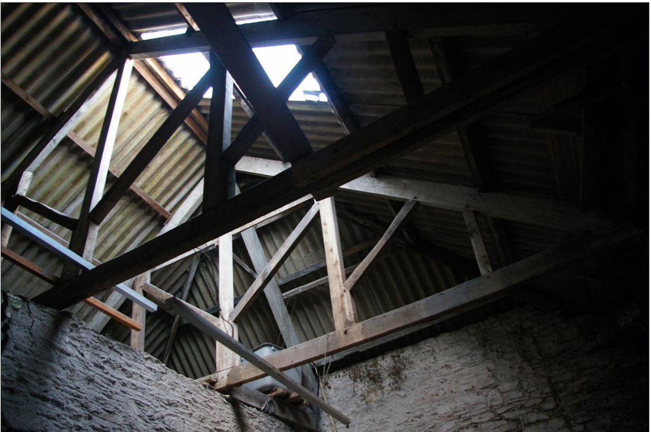
89. B1 FF R3, DETAIL OF THE ROOF STRUCTURE OVER R2 AND R3; VIEWED FROM THE NORTH-WEST.
