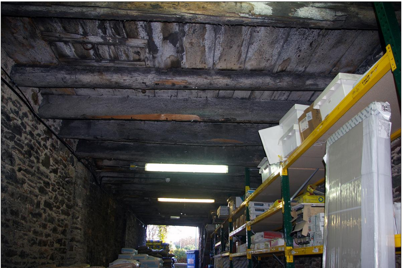
150. B3 GF INTERIOR, DETAIL OF THE MANY RE-USED BEAMS, INCLUDING SHIPS TIMBERS; VIEWED FROM THE NORTH.
