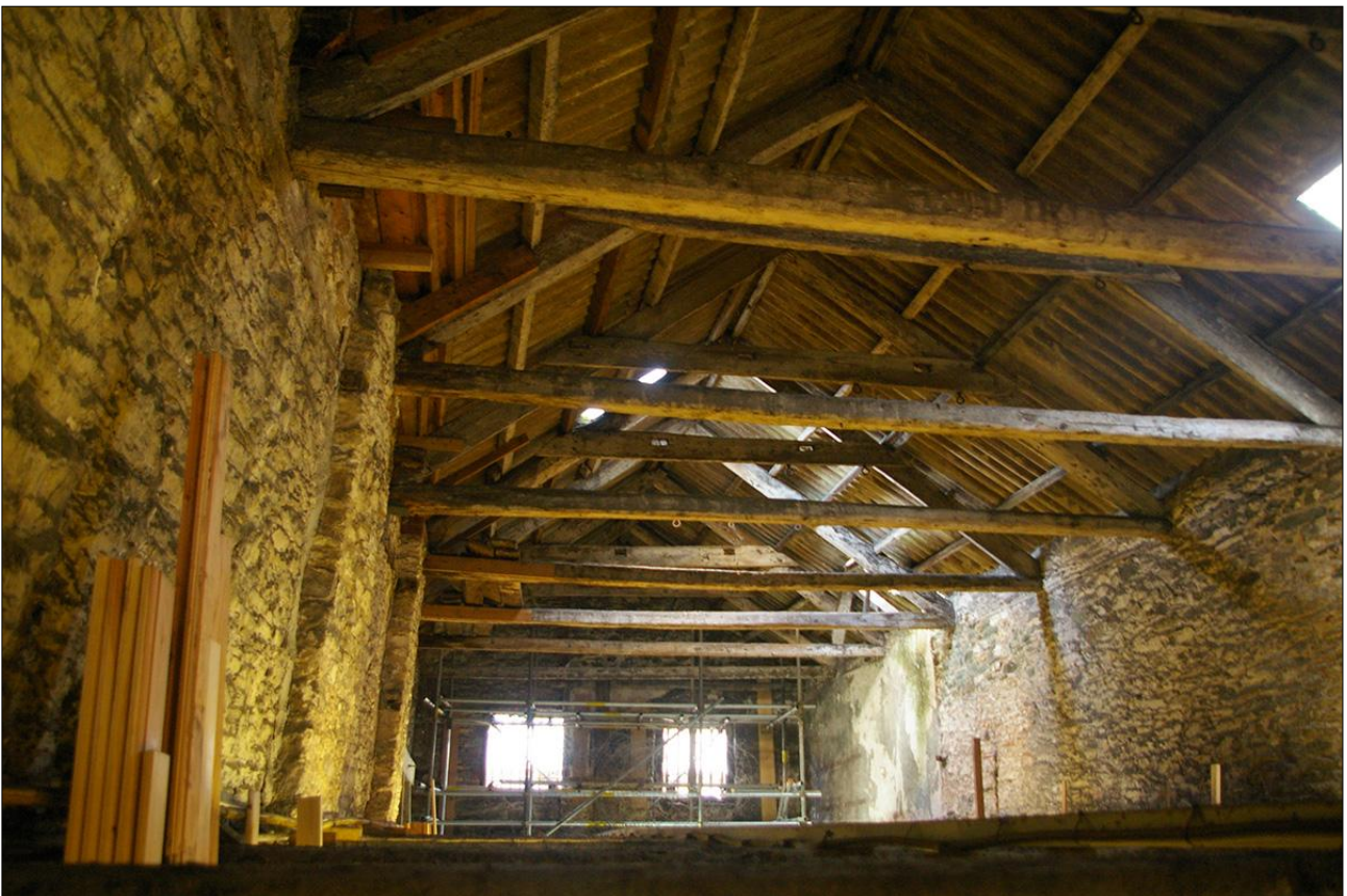
122. B2 SF INTERIOR; THE ROOF STRUCTURE OVER THE NORTHERN END OF B2, W20 AND W21; VIEWED FROM THE SSW.
