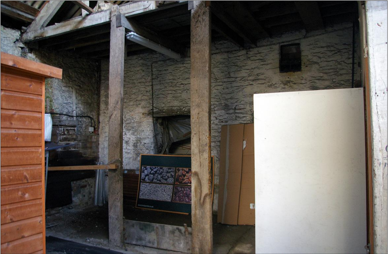
55. B1 FF R1, THE SOUTHERN END OF THE ROOM; VIEWED FROM THE WNW.
