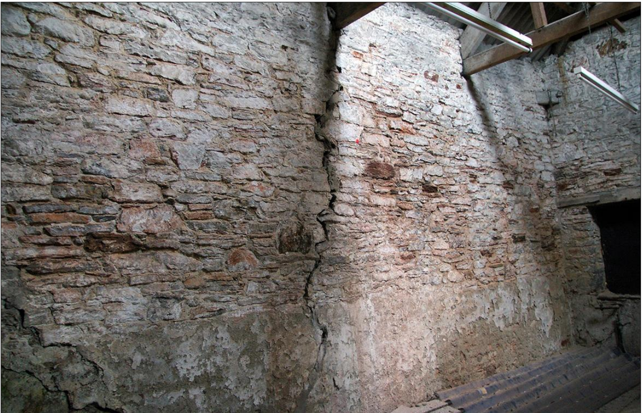
83. B1 FF R3, THE WEST WALL OF R3 SHOWING ITS STRUCTURAL CRACKS; VIEWED FROM THE SOUTH-EAST.
