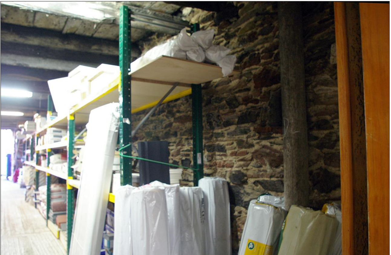
148. B3 GF INTERIOR, THE WEST WALL OF B3 (EAST WALL OF B2); VIEWED FROM THE NNE.
