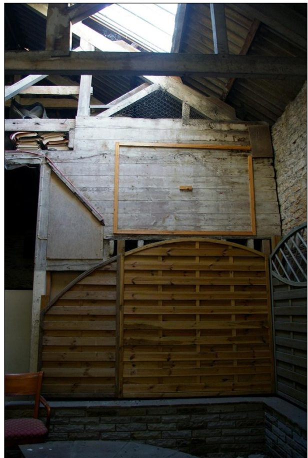
51. RIGHT: B1 FF R1, DETAIL OF THE NORTH SIDE OF THE LARGE TIMBER HOPPER S18; VIEWED FROM THE NORTH.
