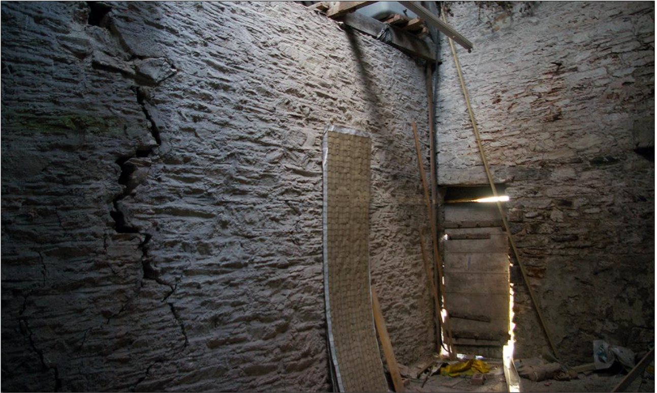
74. B1 FF R2, VIEW OF THE STRUCTURAL CRACK IN THE WEST WALL, AND D22 IN THE NORTH WALL; VIEWED FROM THE SSE.
