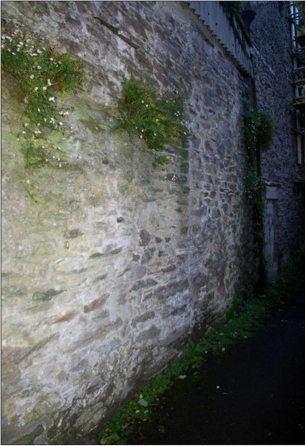
188. THE NORTH WALL OF B4, SHOWING A BLOCKED OPENING; VIEWED FROM THE ENE.
