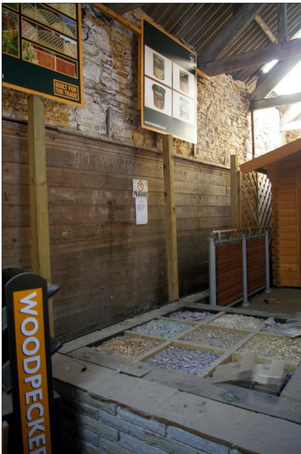
50. LEFT: AS ABOVE, DETAIL OF THE PANELLING (S8); VIEWED FROM THE SOUTH-EAST.
