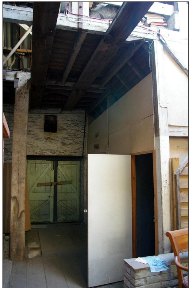
54. RIGHT: B1 FF R1, VIEW TO FF LOADING DOORS D16, WITH FORCED OPENING S15 AND BAG HOIST S16 ABOVE; VIEWED FROM THE NORTH.
