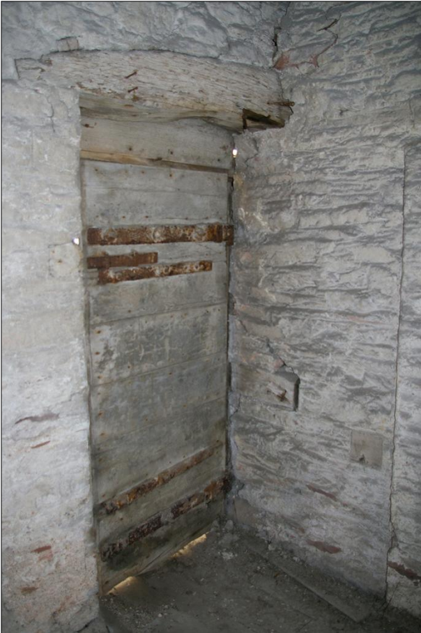
86. B1 FF R3, DETAIL OF D21 SHOWING ITS YOKED LINTEL AND THE RECESS BUILT INTO THE EAST WALL TO TAKE THE DOOR; VIEWED FROM THE SOUTH-WEST.
