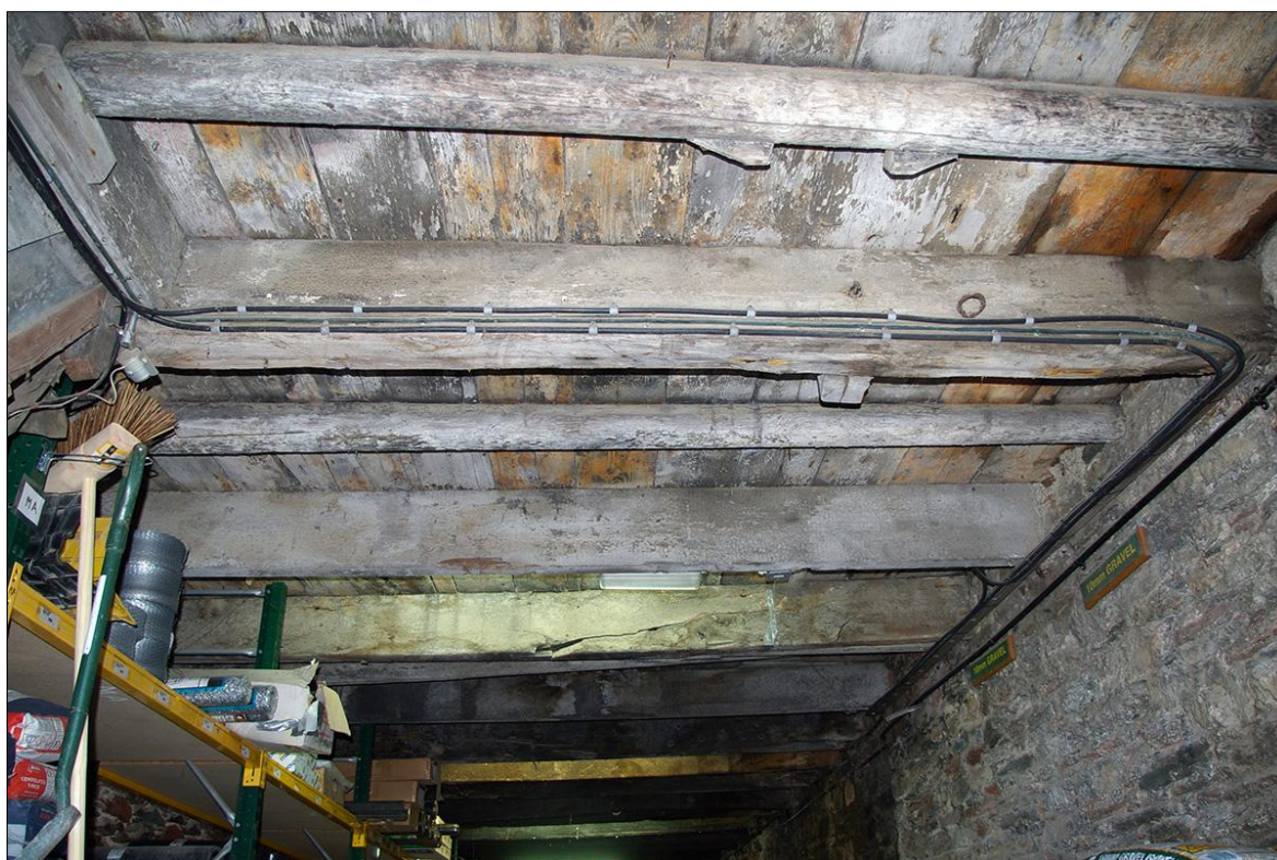
FIGURE 30: SOME OF THE JOISTS IN B3, SHOWING THE REUSE OF SHIPS TIMBERS; VIEWED FROM THE SOUTH.
