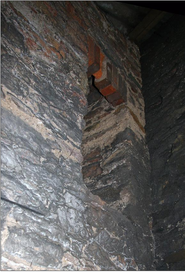
170. B3 SF INTERIOR, DETAIL OF FP4 ABOVE THE STAIRS; VIEWED FROM THE NORTH-EAST.
