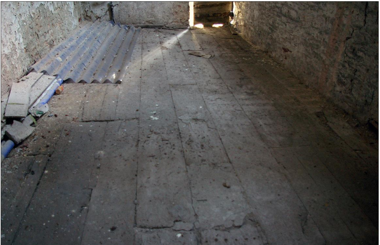
87. B1 FF R3, DETAIL OF THE HISTORIC FLOORBOARDS (S9); VIEWED FROM THE SOUTH.
