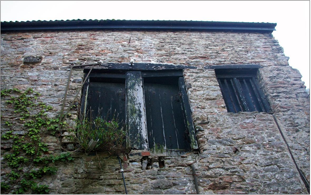
4. THE NORTH ELEVATION OF B1, SHOWING W11 AND FF DOOR 21 (D21) AND DOOR 22 (D22); VIEWED FROM THE NORTH.
