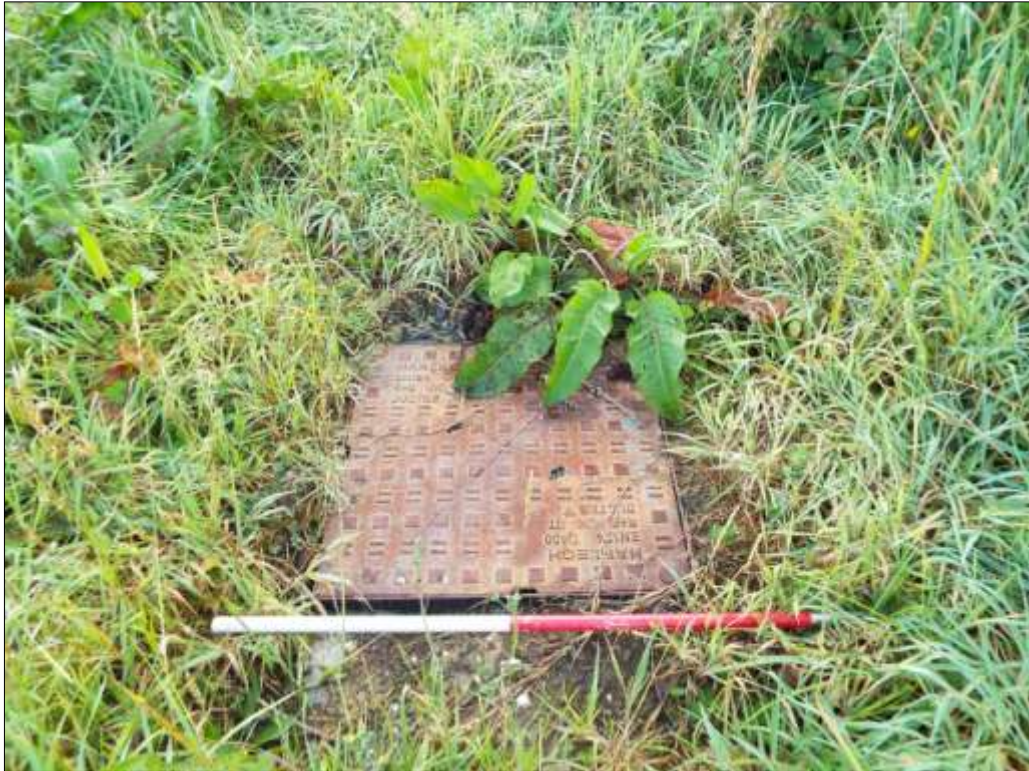
13. Detail of a modern man-hole cover for the drainage system installed across the site; viewed from the south-west (1m scale).
