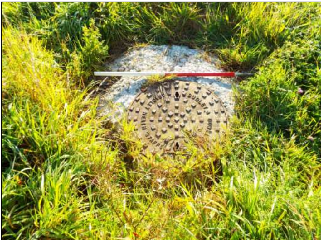
14. Detail of a modern man-hole cover for the drainage system installed across the site; viewed from the south-west (1m scale).
