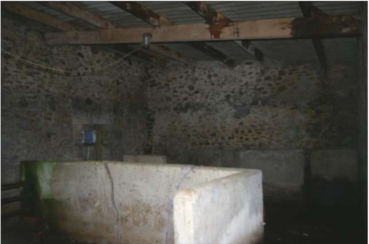
THE INTERIOR OF BARN 1: THE CONCRETE PENS IN THE BARN; VIEWED FROM THE SOUTH-EAST.
