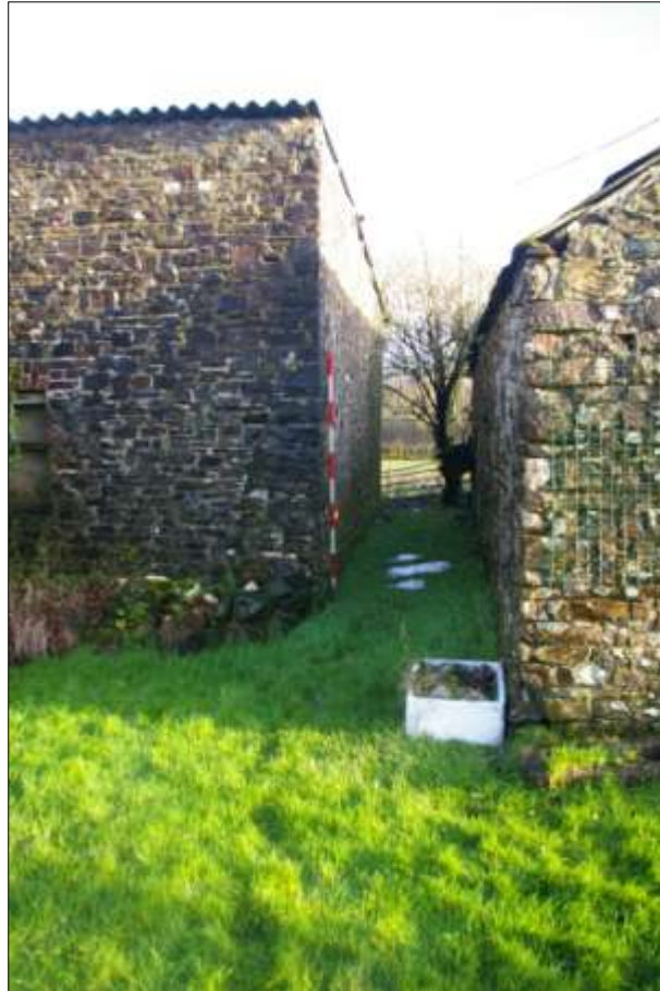
THE SOUTH AND SOUTH-WEST CORNER OF BARN 1, WITH 2M SCALE; FROM THE WEST, SOUTH-WEST.
