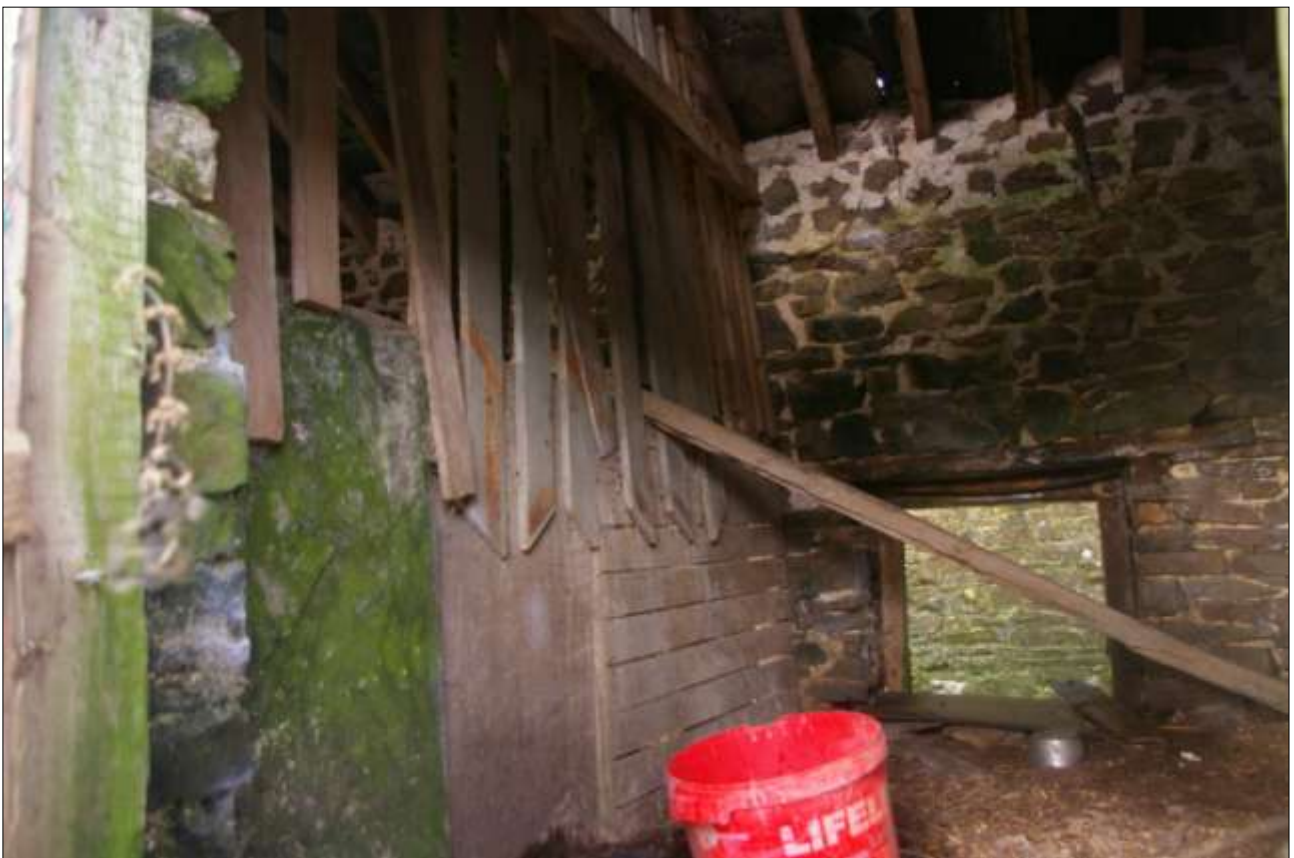
ONE OF THE PENS FORM THE LOW DOORWAY OF THE EAST PEN (BARN 2), SHOWING THE MORE MODERN TIMBER SCREEN ERECTED BETWEEN IT AND THE CENTRAL AND WEST PEN, FORMING A MORE MODERN POULTRY SHED TO THE WEST END OF THE FORMER PIGSTY; FROM THE SOUTH, SOUTH-EAST.
