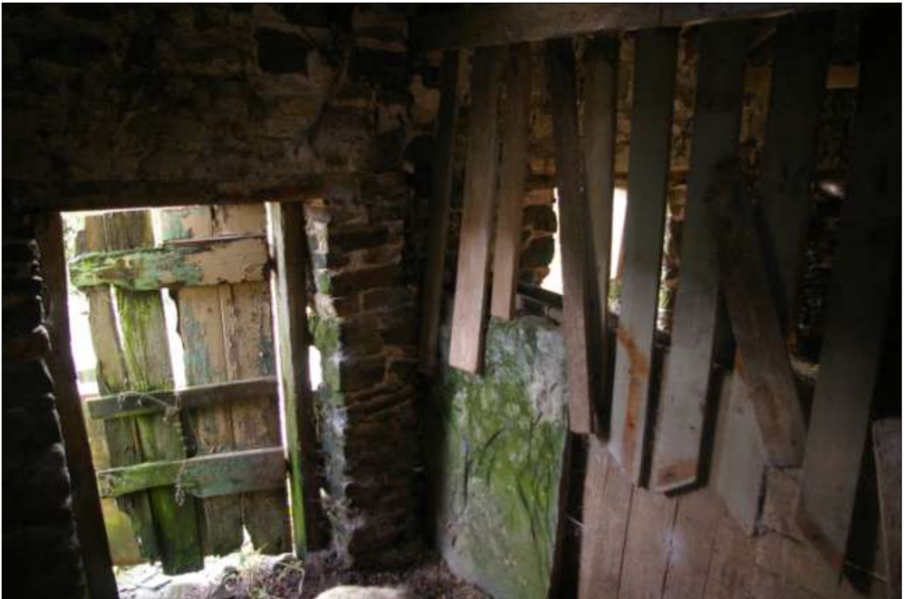
VIEW OF THE UPRIGHT SLATE SLAB SET IN DETAIL AND IN ITS CONTEXT, ATTACHED TO THE SOUTH WALL, BETWEEN THE EAST AND MIDDLE PEN IN THE PIGSTY (BARN 2); FROM THE NORTH-EAST.
