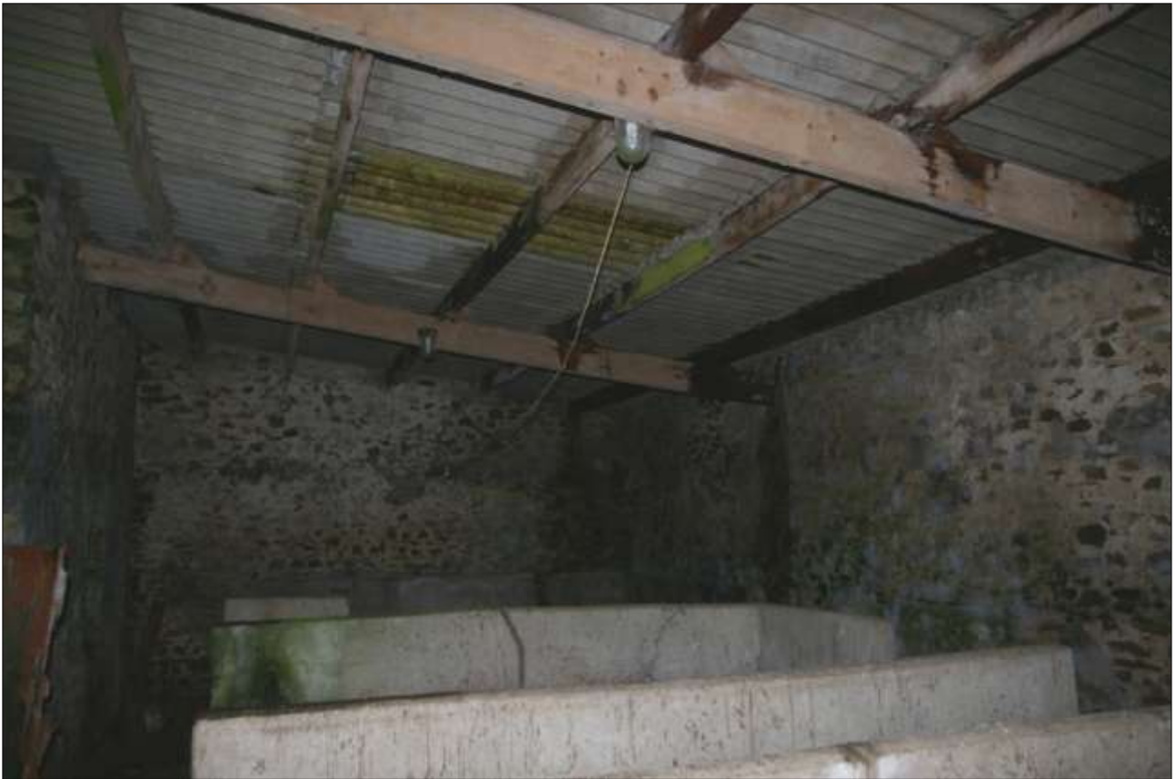
THE INTERIOR OF BARN 1: SHOWING THE MONO-PITCH REPLACEMENT ROOF OF CORRUGATED ASBESTOS; VIEWED FROM THE SOUTH-WEST.
