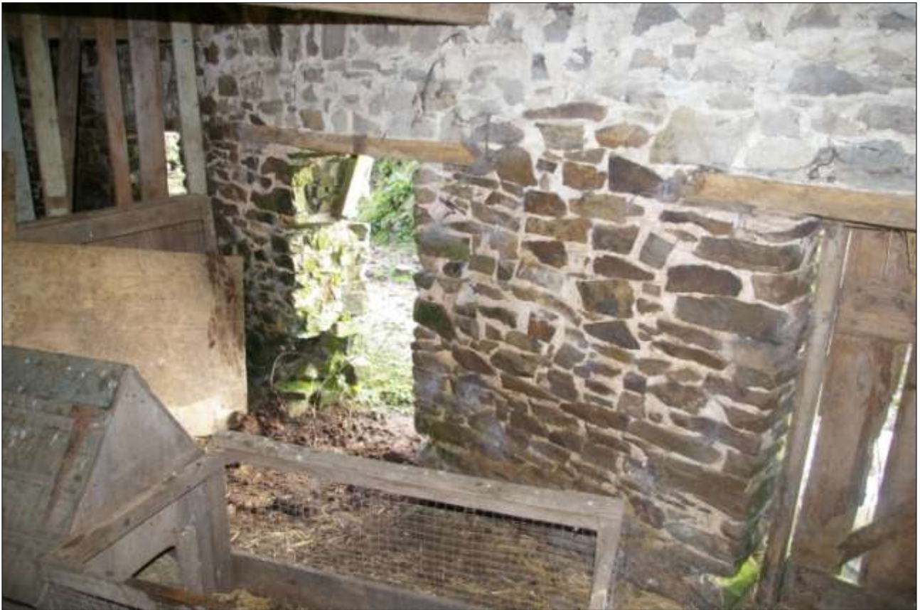
VIEW OF THE LOW DOORWAY IN THE SOUTH WALL, FROM WITHIN THE PIGSTY (BARN 2); FROM THE NORTH-WEST.
