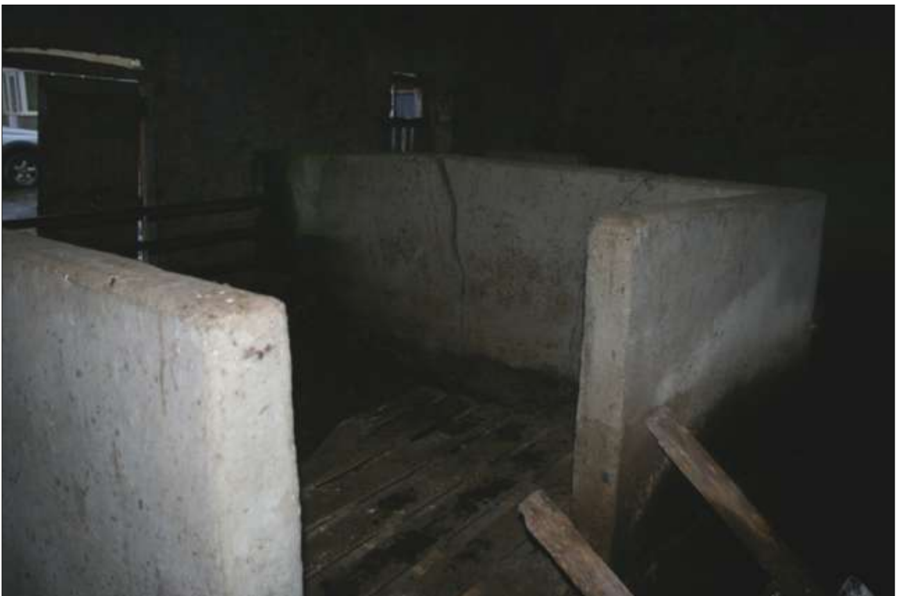
THE INTERIOR OF BARN 1: DETAIL OF THE PRE-FABRICATED CONCRETE PENS; VIEWED FROM THE SOUTH-EAST.
