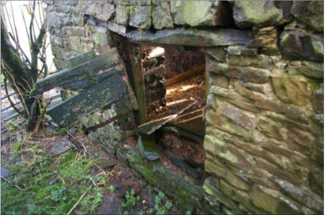
THE PARTLY SURVIVING PLANK SHUTTER TO THE EAST ON THE NORTH ELEVATION OF THE PIGSTY (BARN 2), SERVING THE FORMER FEED HATCH TO THE PEN; FROM THE WEST, NORTH-WEST.
