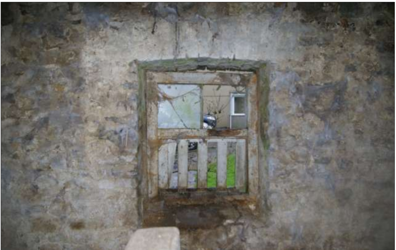
THE INTERIOR OF BARN 1: THE NORTH WINDOW IN THE WEST WALL; VIEWED FROM THE EAST.
