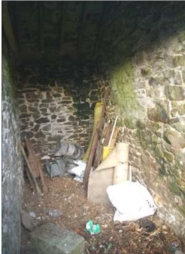
THE OPEN WESTERN COMPARTMENT OF THE PIGSTY (BARN 2); FROM THE SOUTH, SOUTH-WEST.
