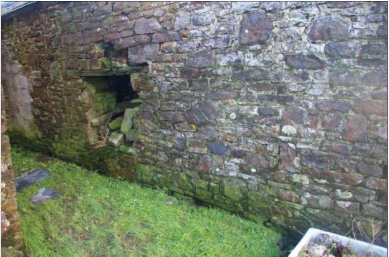
POSSIBLE BLOCKED OPENING IN THE WESTERN END OF THE NORTH WALL OF THE PIGSTY (BARN 2); FROM THE NORTH-WEST
