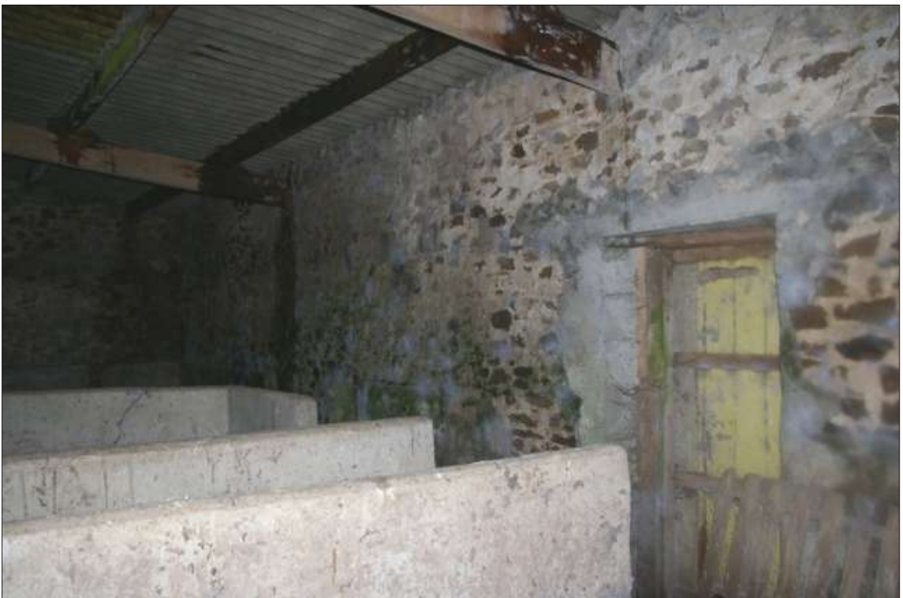
THE INTERIOR OF BARN 1: THE EAST WALL WITH FORCED DOORWAY; VIEWED FROM THE SOUTH-SOUTH-WEST.
