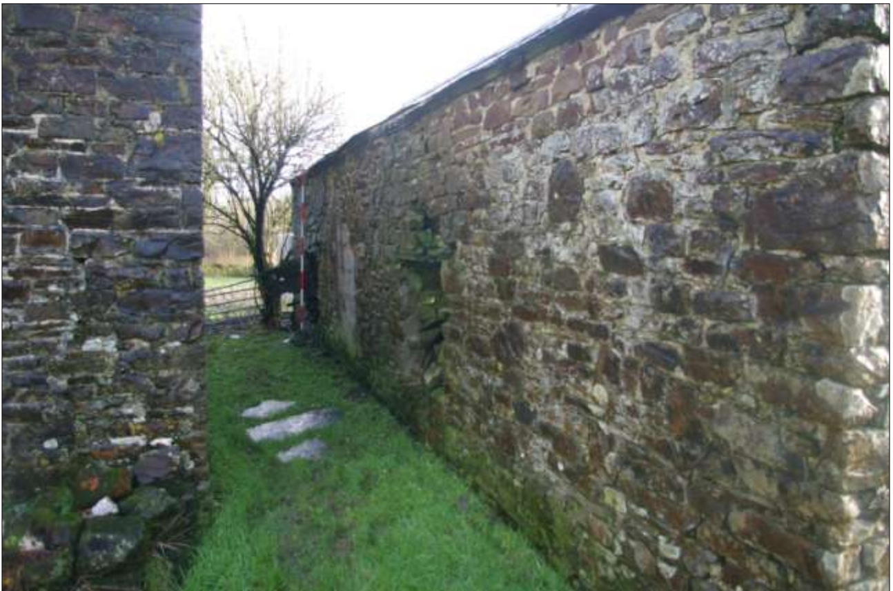
THE NORTH ELEVATION OF THE PIGSTY (BARN 2), WITH 2M SCALE; FROM THE NORTH-WEST.
