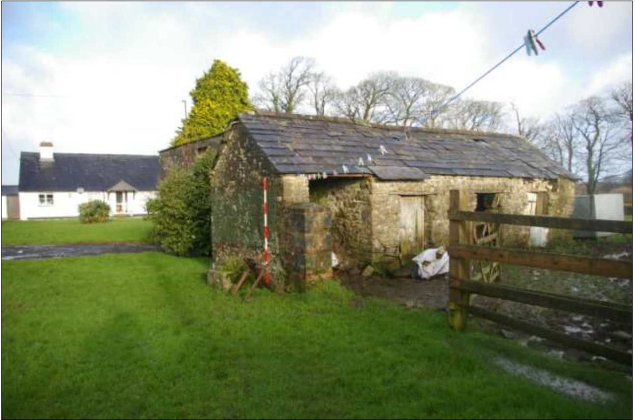
THE WEST AND SOUTH WALL OF THE PIGSTY (BARN 2), WITH 2M SCALE; FROM THE SOUTH-WEST.
