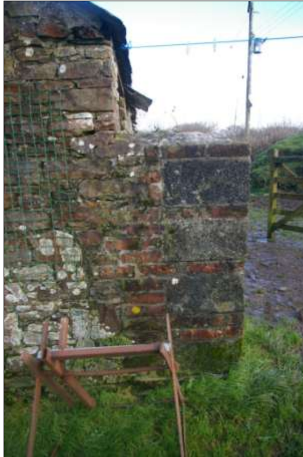
CONCRETE AND BRICK EXTENSION TO THE WEST WALL OF BARN 2, ENCLOSING THE YARD; FROM THE WEST.
