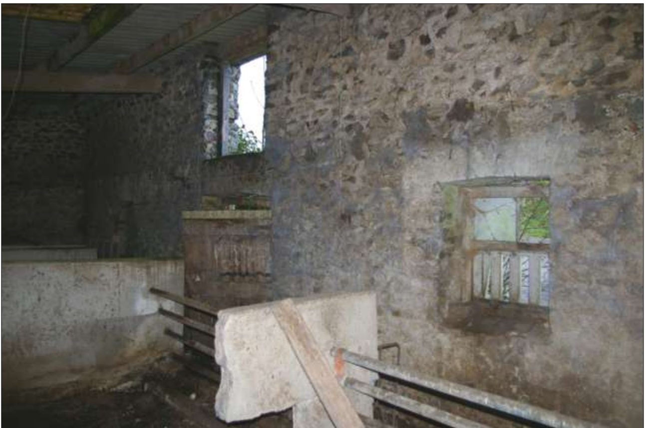
THE INTERIOR OF BARN 1: THE WEST WALL OF THE BARN WITH DOOR, LOADING DOOR AND WINDOW; VIEWED FROM THE NORTH-EAST.
