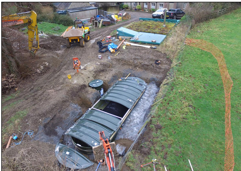
FIGURE 5: SITE SHOT, POST INSERTION OF NEW SEPTIC TANK VIEWED FROM ABOVE AND THE NORTH-WEST (NO SCALE).
