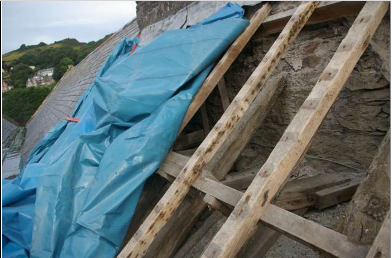
HISTORIC ROOFLINE, SHOWING COMPLETELY DIFFERENT PITCH WITHIN ROOF SPACE AGAINST SOUTH SIDE OF TOWER; FROM THE SOUTH-EAST.
