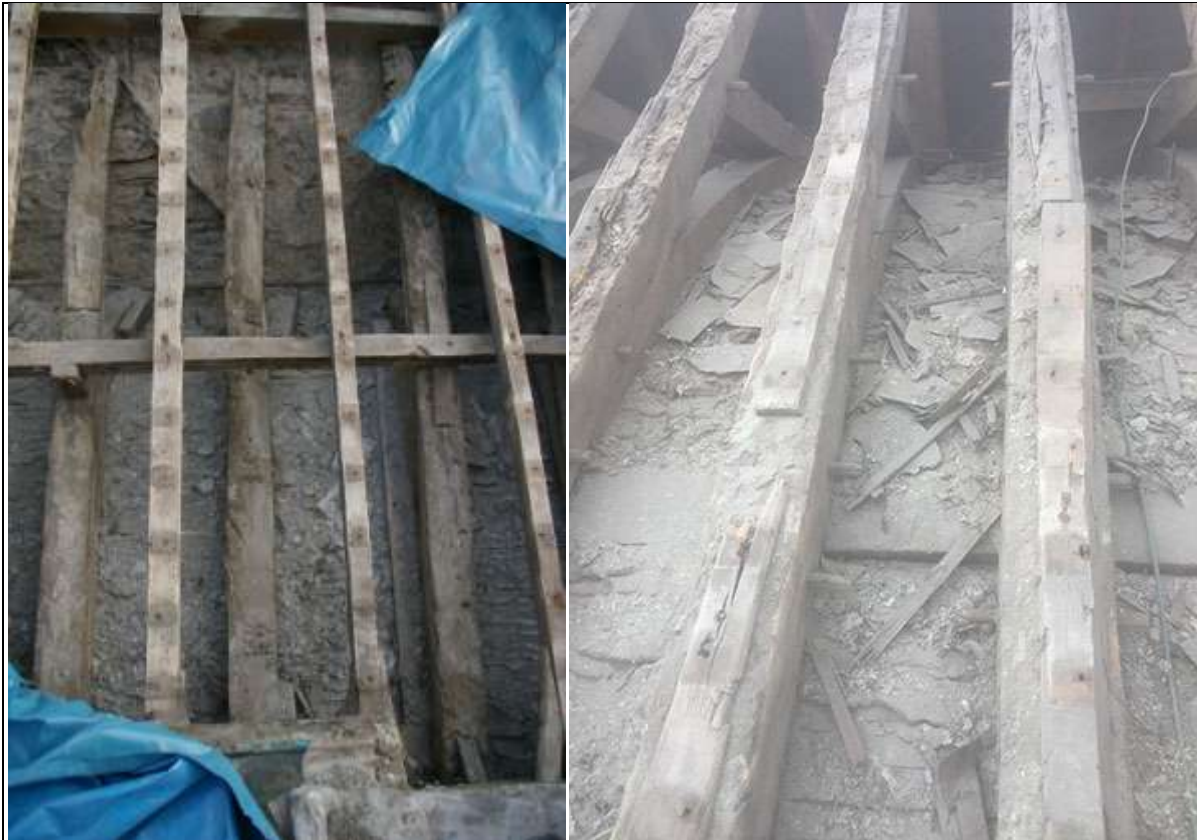
LEFT: THREE REUSED TIMBERS WITHIN ROOF OF NORTH AISLE, BUILT AROUND NORTH TRANSEPT TOWER, PART OF A FORMER PARTITION; ALSO SHOWING FORMER ROOFLINE ON TOWER WALL, FROM THE SOUTH-SOUTH-EAST. RIGHT: HEAVIER TRUSSES OVER THE SOUTH AISLE ROOF.
