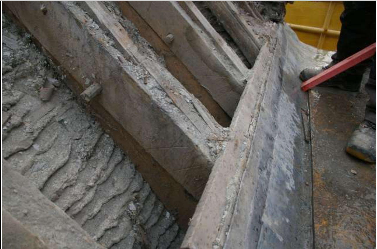
THE CARPENTERS MARKS ON THE NORTH AISLE ROOF TIMBERS; FROM THE WEST-SOUTH-WEST.
