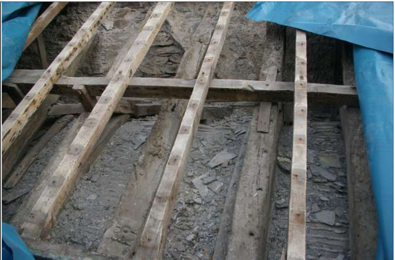
DETAIL OF REUSED TIMBERS IN NORTH AISLE ROOF, SOUTH FACE, AGAINST TOWER; FROM THE SOUTH, SOUTH-EAST
