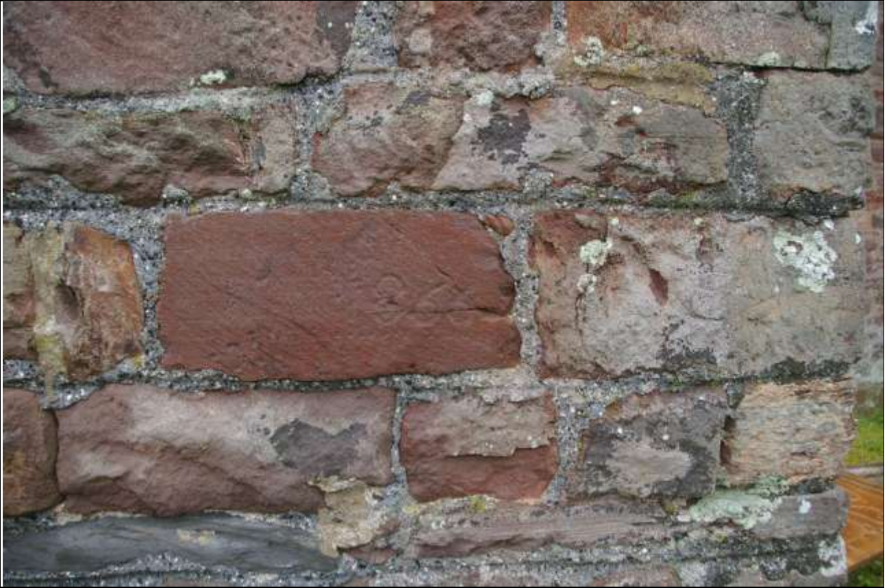
INSCRIBED STONE TO RIGHT OF ARCHED OPENING TO NORTH PORCH, WITH DATE OF 1866; FROM THE NORTH.
