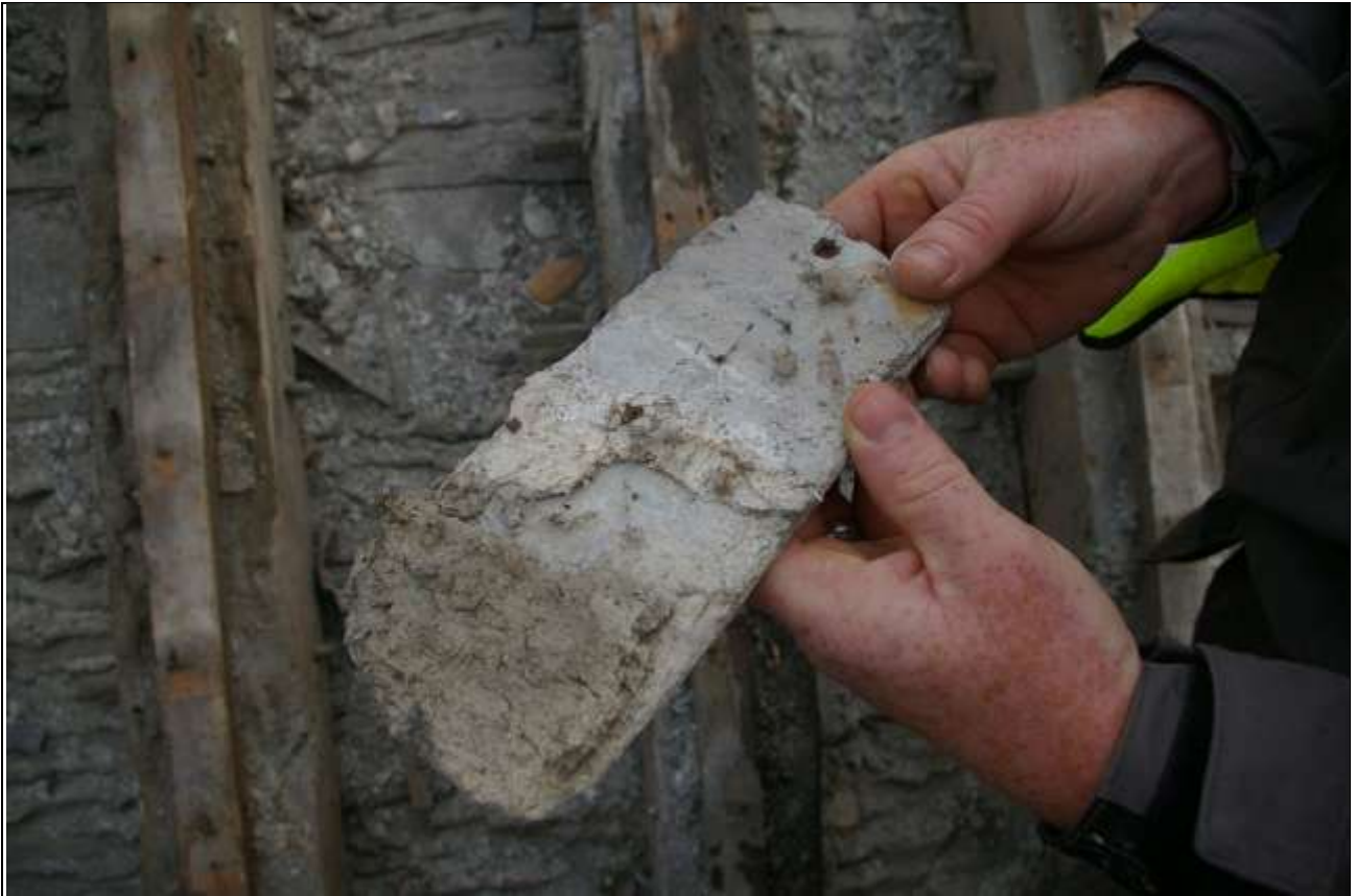
PEG SLATE, INDICATING SCANTLE SLATE ROOF WITH OAK PEGS, RECOVERED FROM SOUTH FACE OF NORTH AISLE ROOF.
