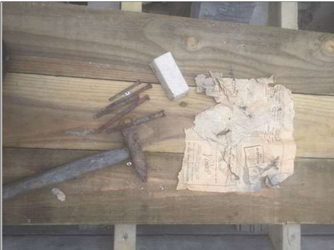
HAMMER AND HANDMADE IRON TACKS/NAILS FOR ROOFING, FOUND IN SOUTH AISLE ROOF, INDICATING AN EARLY 20 TH CENTURY PHASE OF RESLATING/REPAIRS.
