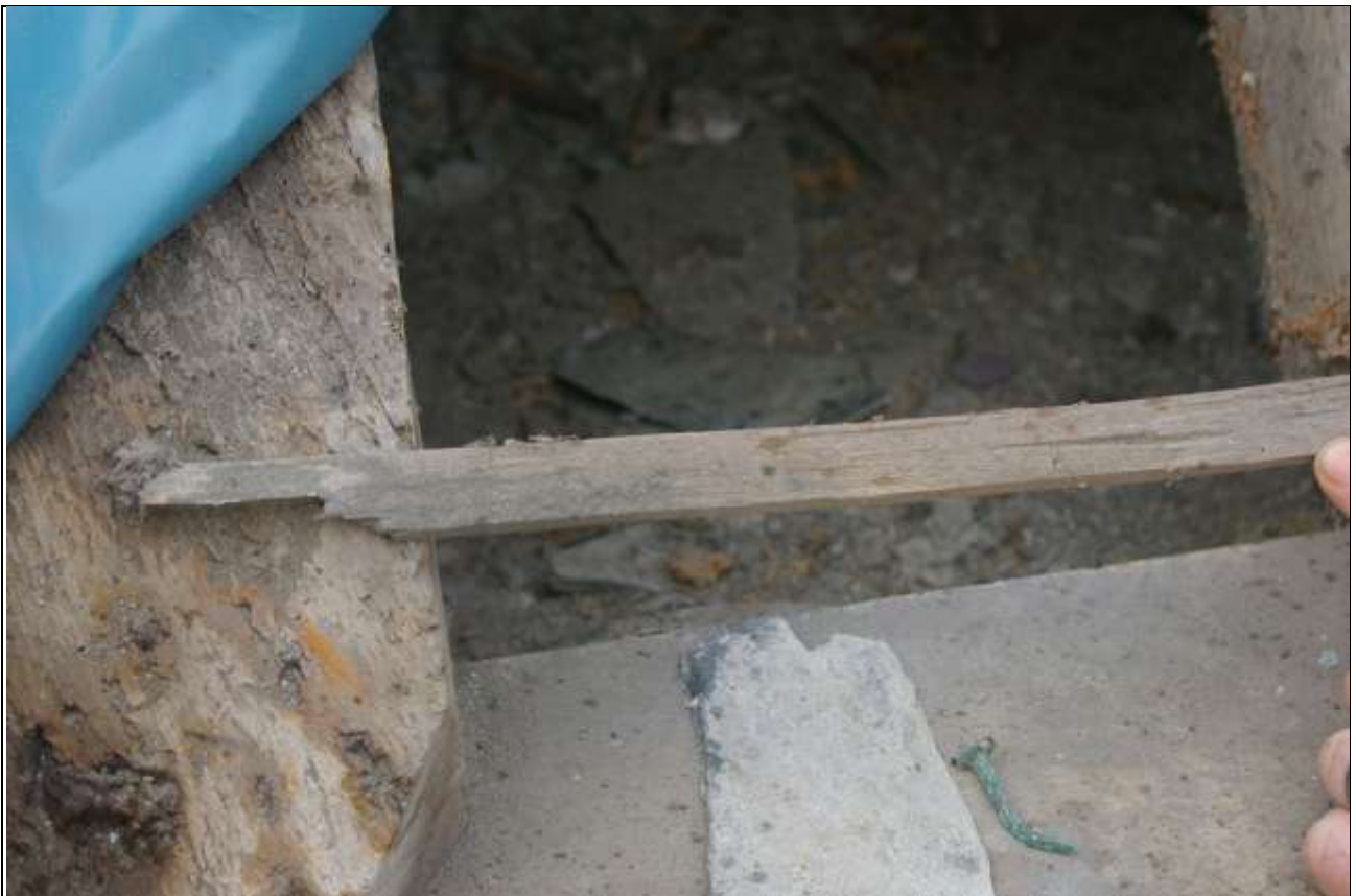
SPLIT OAK LATHE USED IN SCANTLE SLATE ROOF, RECOVERED FROM THE SOUTH FACE OF THE NORTH AISLE ROOF.
