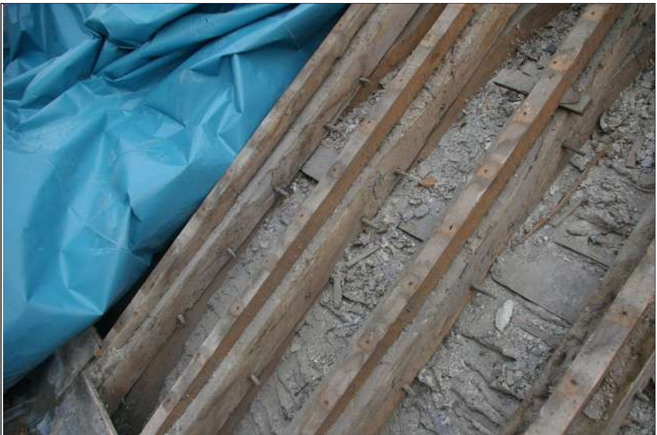
LIGHTWEIGHT JOINTED TRUSSES WHICH CARRY THE BARREL VAULTED CEILINGS OVER THE NORTH AISLE, SHOWING PEGGED JOINTS AND MODERN TIMBERS ATTACHED TO BACK OF BLADES TO CARRY THE SLATED ROOF; FROM THE EAST, SOUTH-EAST.
