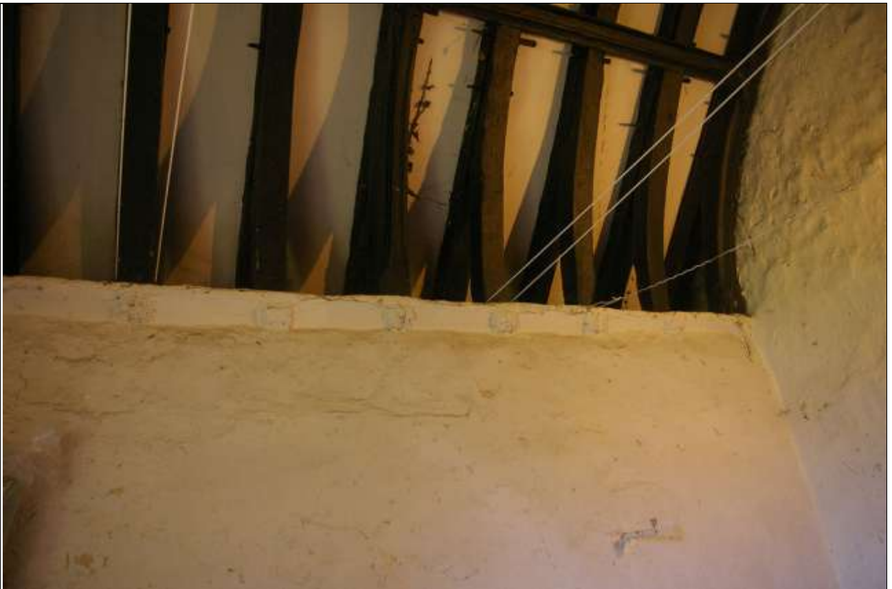
THE OPEN WAGON ROOF IN THE NORTH PORCH, SHOWING THE SECTIONS OF WALLPLATE WITH SQUARE LEAF AND FOLIATE GEOMETRIC DESIGNS, THE SAME AS THAT ON THE REUSED TIMBERS IN THE NORTH AISLE ROOF; FROM THE NORTH-WEST.
