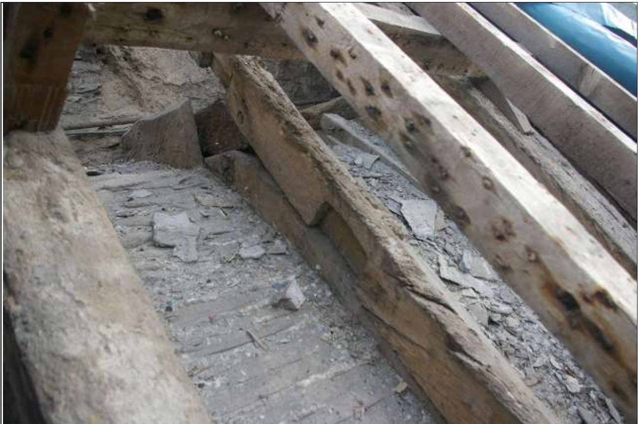
SOCKETS IN ONE OF THE REUSED BEAMS, SOUTH SIDE OF THE TOWER, SHOWING OTHER REUSED BEAMS USED TO FORM THE BARREL CEILING; FROM THE SOUTH-WEST.
