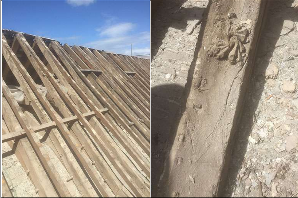
LEFT: 20 TH CENTURY TIMBERS NAILED TO TRUSSES ON SOUTH AISLE TO CORRECT SAGGING AND BRACE AND REPLACE ROTTEN SECTIONS, SHOW A PHASE OF EARLY 20 TH CENTURY REPAIR AND RESLATING.
