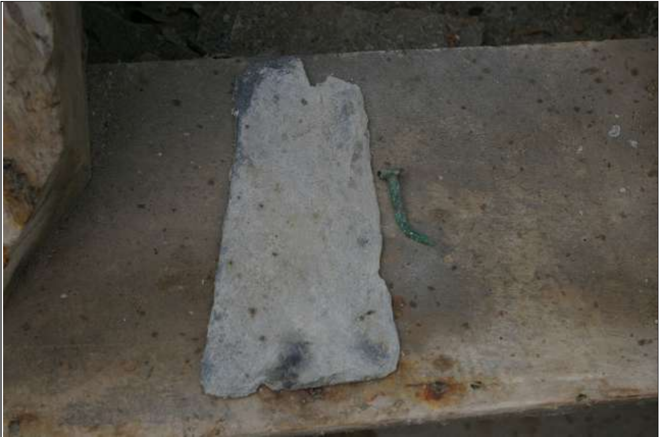
PEG SLATE, FROM SCANTLE ROOF COVERING OVER NAVE AND NORTH AISLE, WITH ORIGINAL COPPER PIN/PEG.
