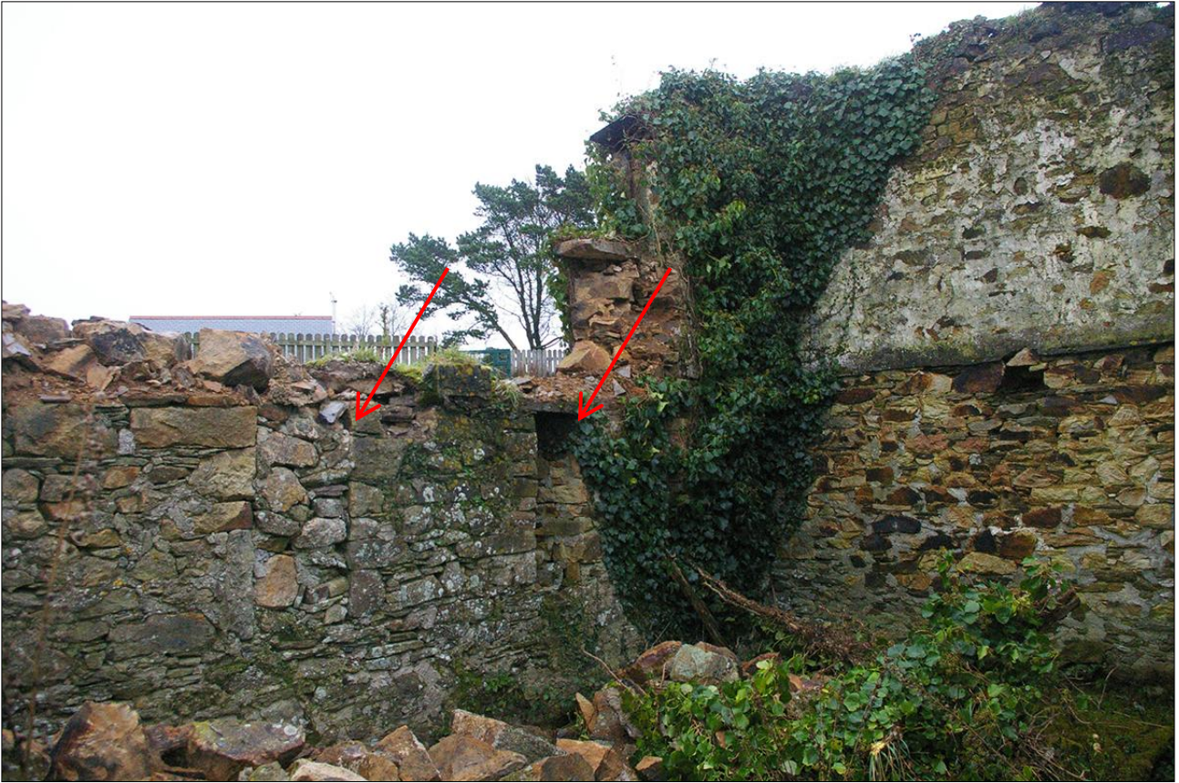
THE INTERIOR OF B4B (SOUTH-EAST CORNER) SHOWING THE SLIT VENTS (INDICATED); VIEWED FROM THE NORTH-WEST.
