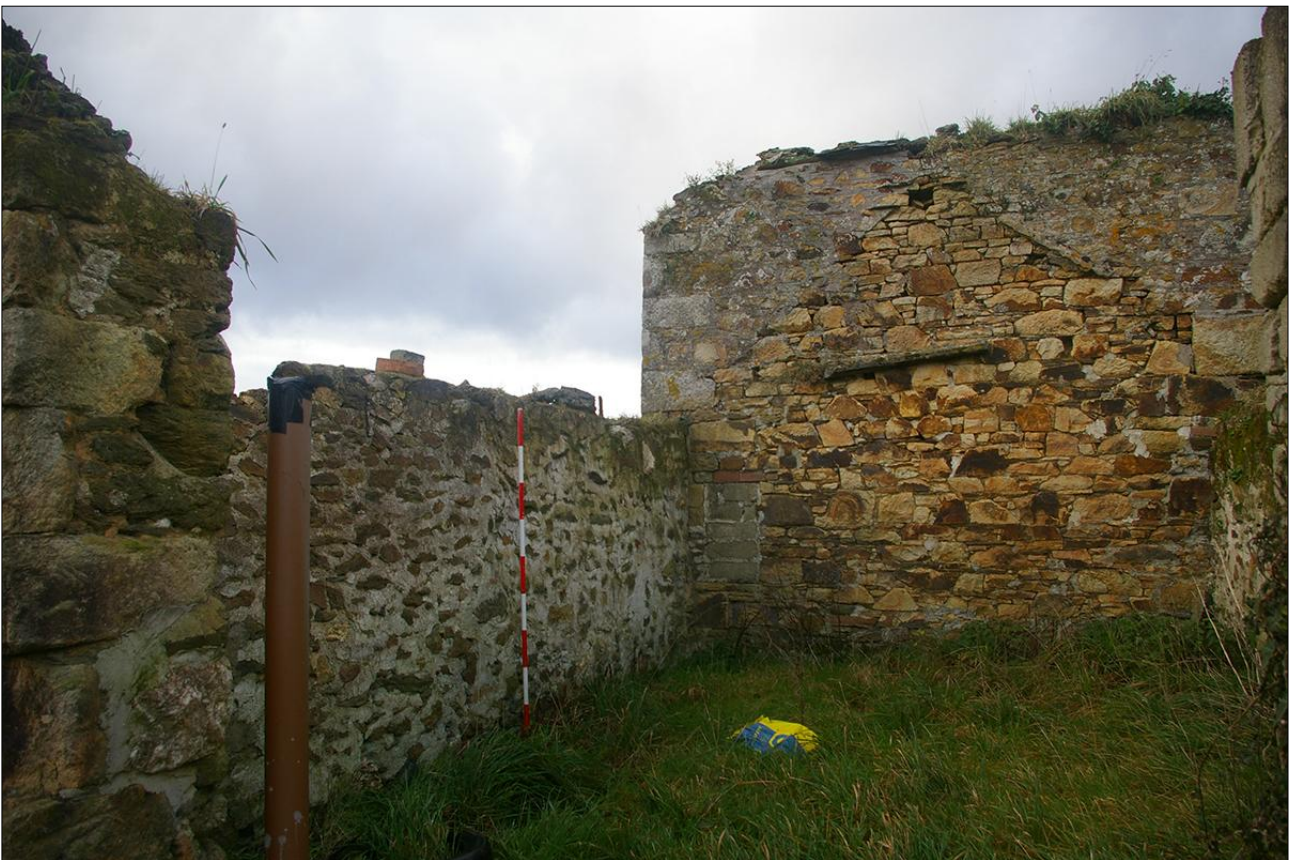
THE INTERIOR OF B4C, SOUTH-WEST WALL AND FORMER GABLE OF B4B; VIEWED FROM THE SOUTH (SCALE 2M)
