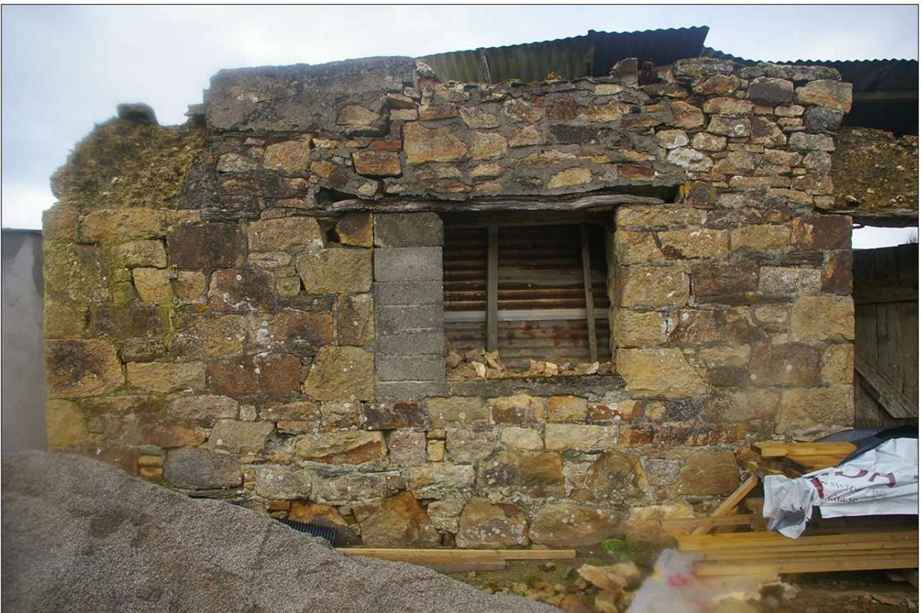
THE WEST WINDOW IN THE SOUTH ELEVATION OF B1; VIEWED FROM THE SOUTH.
