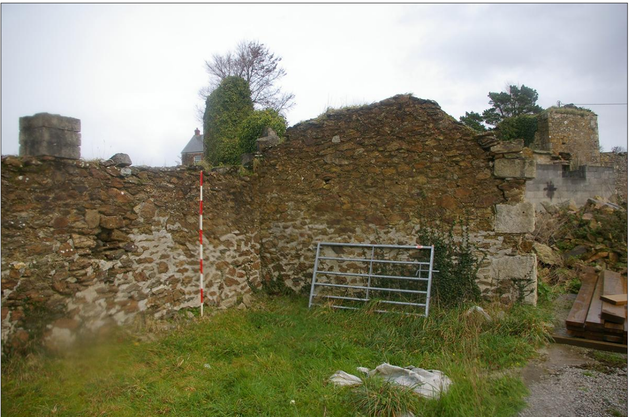
B2, THE INTERNAL EAST GABLE WALL; VIEWED FROM THE SOUTH-WEST (SCALE 2M).
