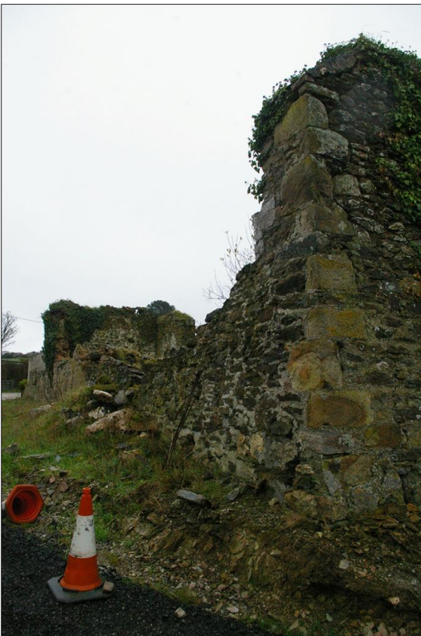
THE NORTH-WEST CORNER OF B4A AND COLLAPSED REAR WALL; VIEWED FROM THE NORTH-WEST.
