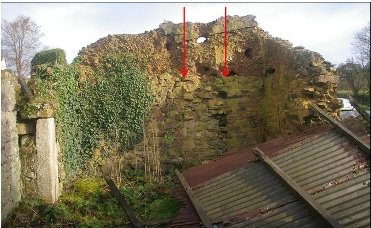
FIGURE 12: INTERNAL EAST GABLE OF B1, SHOWING THE FIREPLACE (LEFT) AND WALL SCAR (INDICATED); VIEWED FROM THE WSW.
