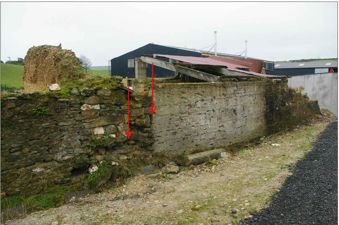
AS ABOVE; THE RAGGED MASONRY (INDICATED) IS WHERE THE NORTH SIDE OF THE FIREPLACE HAS BEEN REDUCED IN WIDTH. VIEWED FROM THE NORTH-EAST.
