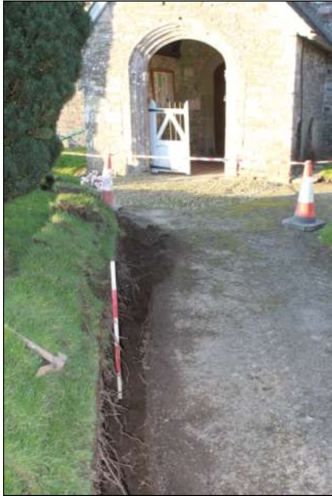
FIGURE 2: SHOT OF TRENCH RUNNING ALONG CHURCH PATH, VIEWED FROM THE SOUTH (1M SCALE).
