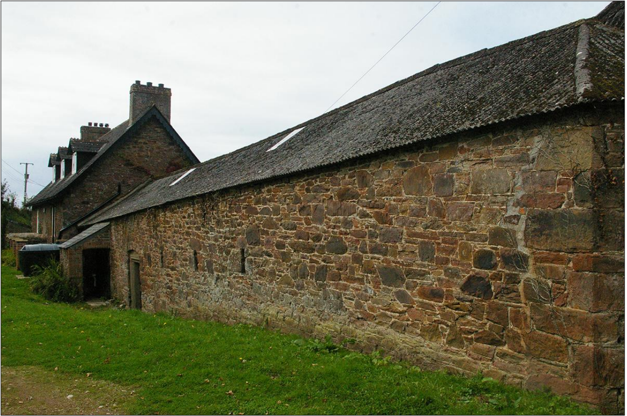
THE REAR (SOUTH) WALL OF B1.1, SHOWING THE CONTINUOUS BUILD; VIEWED FROM THE SOUTH-EAST.
