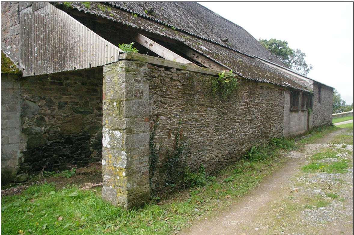
FIGURE 24: THE EAST ELEVATION OF B1.5 (B1.5B IN THE FOREGROUND); VIEWED FROM THE SOUTH-EAST.
