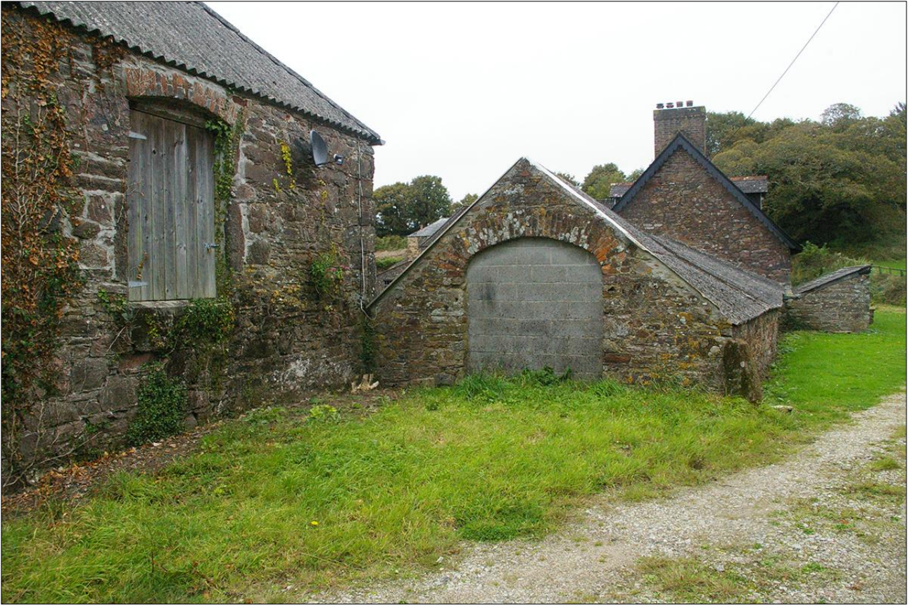
THE WEST GABLE OF B4 SHOWING THE DEPRESSED ARCH, WITH THE SOUTH WALL OF B5 TO THE LEFT; VIEWED FROM THE WEST.
