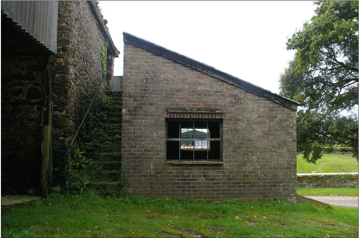
FIGURE 23: THE EAST ELEVATION OF B1.4 AND STAIRS TO THE FIRST FLOOR OF B1.3; VIEWED FROM THE EAST.
