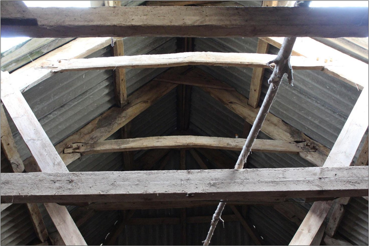
DETAIL OF THE ROOF STRUCTURE IN B5, SHOWING THE UPSIDE DOWN NOTCHED LAPPED COLLAR; VIEWED FROM THE SOUTH.
