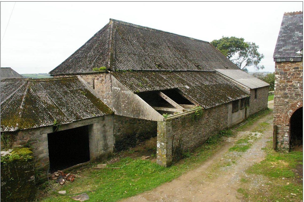
THE EAST ELEVATIONS OF B1.2, B1.3 AND B1.5; VIEWED FROM THE SOUTH-EAST.
