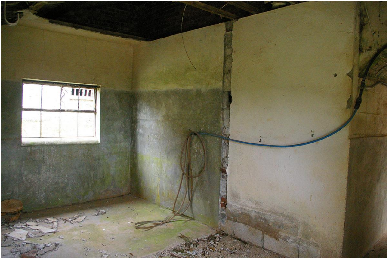
THE INTERIOR OF B1.4; VIEWED FROM THE NORTH-WEST. THE PASSAGEWAY TO B1.3 IS ON THE RIGHT.
