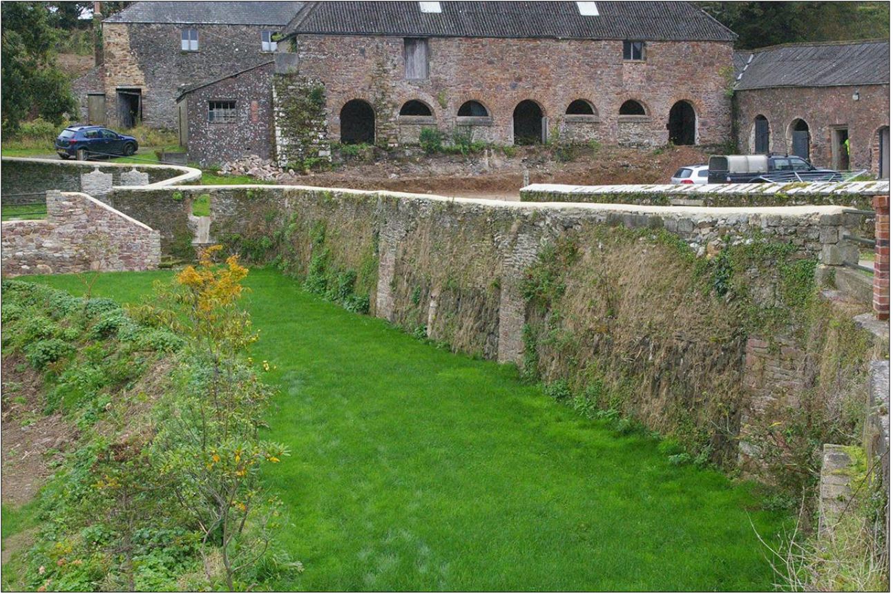
AS ABOVE, DETAIL OF THE RETAINING WALL SHOWING THE PILLARS OF DRESSED MASONRY SEPARATED BY PITCHED DRY STONE WALLS; VIEWED FROM THE NORTH-WEST.
