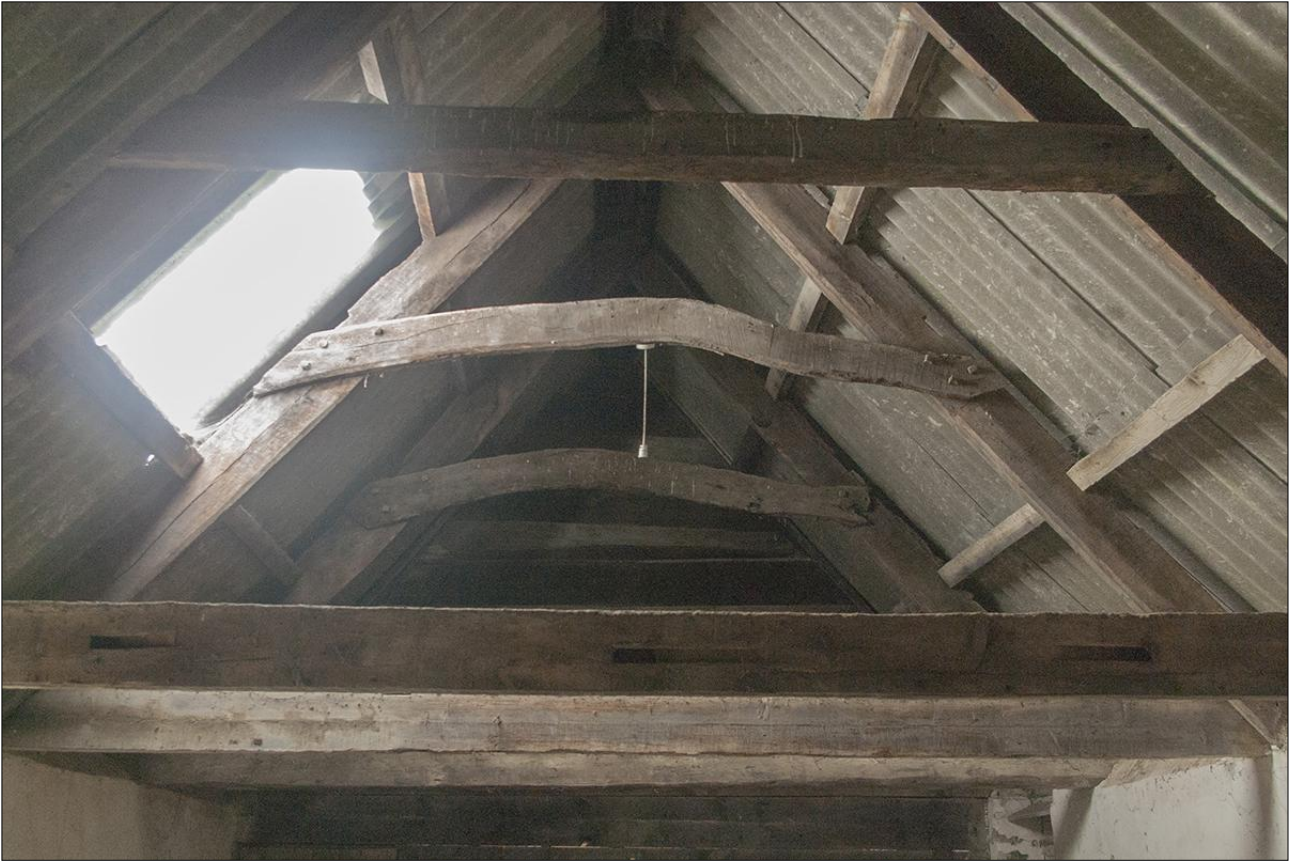
THE FIRST-FLOOR ROOF STRUCTURE IN B1.3 (SOUTH ROOM); VIEWED FROM THE SOUTH.
