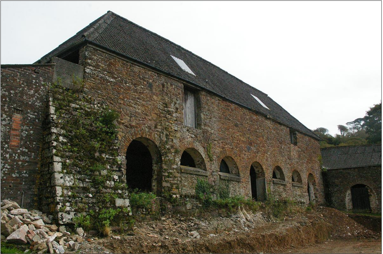
THE FRONT (WEST) ELEVATION OF B1.3, WITH HEAVY BUTTRESS IN THE FOREGROUND; VIEWED FROM THE NORTH-WEST.
