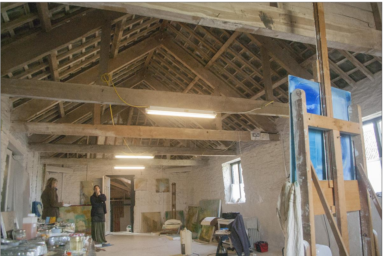
THE INTERIOR OF B2.1 AT FIRST-FLOOR LEVEL, SHOWING THE ROOF STRUCTURE; VIEWED FROM THE NORTH.
