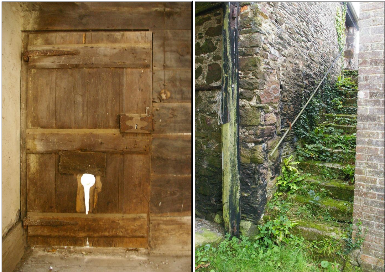
LEFT: THE DOOR AT FIRST-FLOOR LEVEL IN B1.3; VIEWED FROM THE SOUTH.
