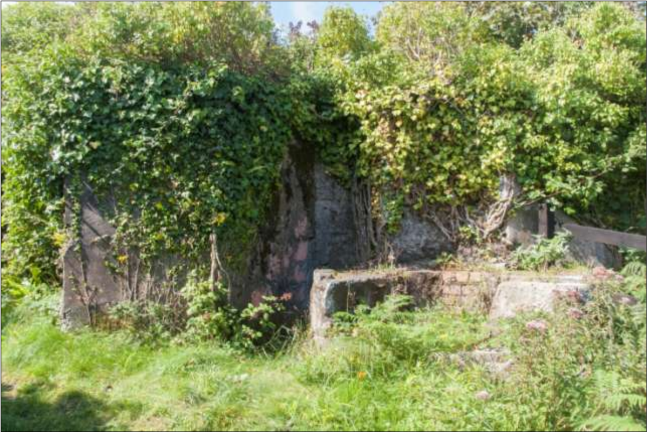
THE SOUTH-EAST CORNER OF THE PHASE 3 CONCRETE RESERVOIR, WITH PROBABLE CHIMNEY BASE; VIEWED FROM THE NORTH-EAST.
