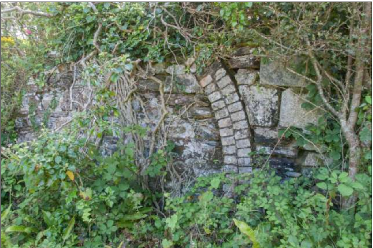
THE NORTH-WEST CORNER OF THE PHASE 2 COMPRESSOR HOUSE/WHIM OPENING WITH BRICK ARCH, BLOCKED IN PHASE 3; VIEWED FROM THE NORTH-WEST.
