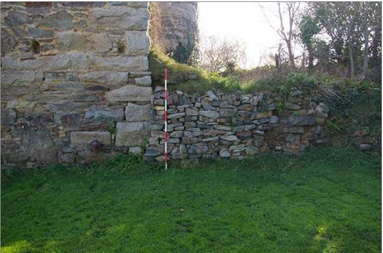
THE ENGINE HOUSE AND THE REBUILT WALL OF THE BOILERHOUSE; FROM THE NORTH-WEST (SCALE 2M).
