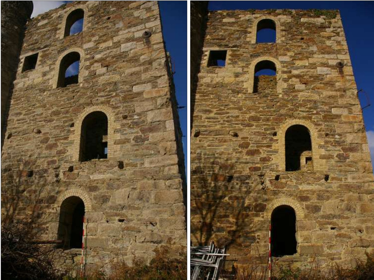
THE SOUTH-EAST ELEVATION OF THE ENGINE HOUSE; VIEWED FROM THE EAST-SOUTH-EAST (SCALE 2M).
