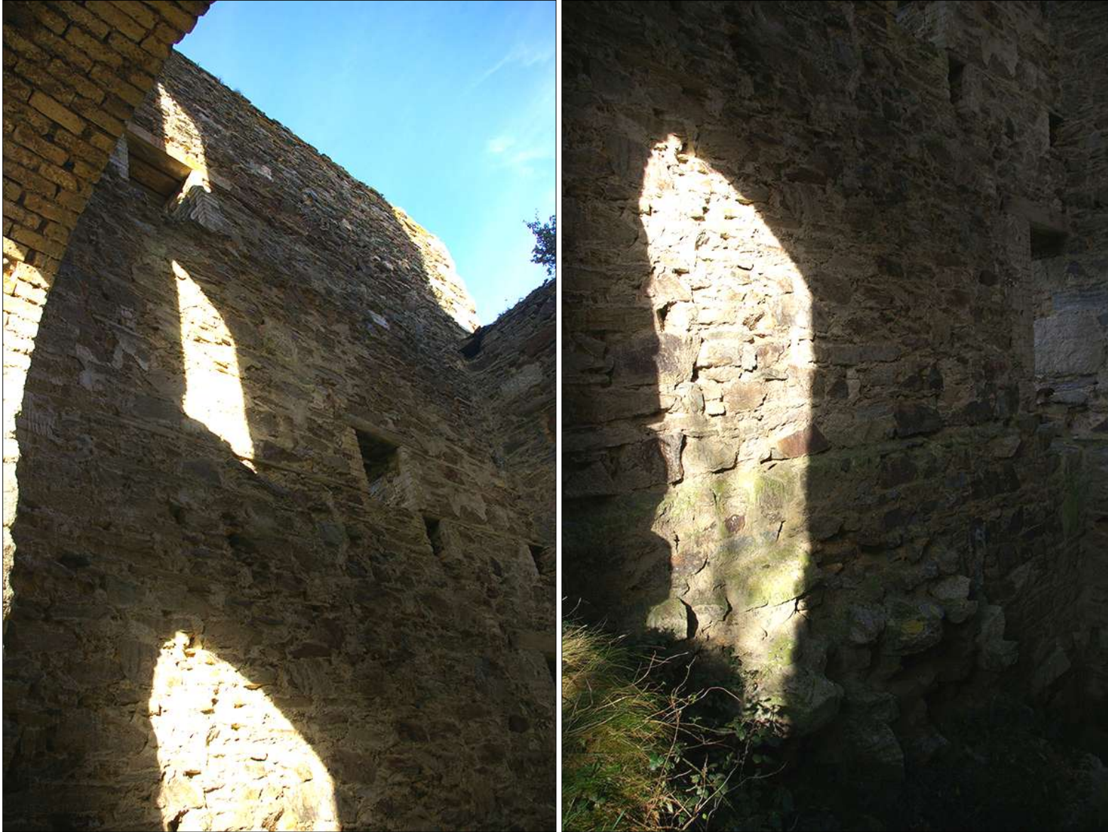
THE INNER FACE OF THE NORTH-WEST OF THE ENGINE HOUSE; FROM THE SOUTH.
