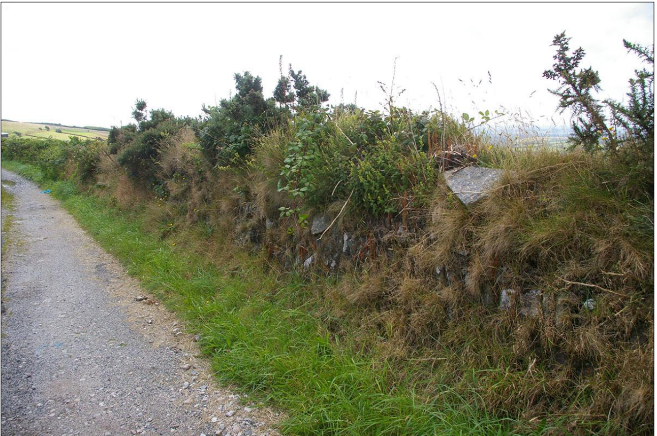
THE STONE-FACED HEDGEBANK ENCLOSING THE NORTH-EASTERN SIDE OF THE SITE; VIEWED FROM THE NNE, LOOKING SSW.
