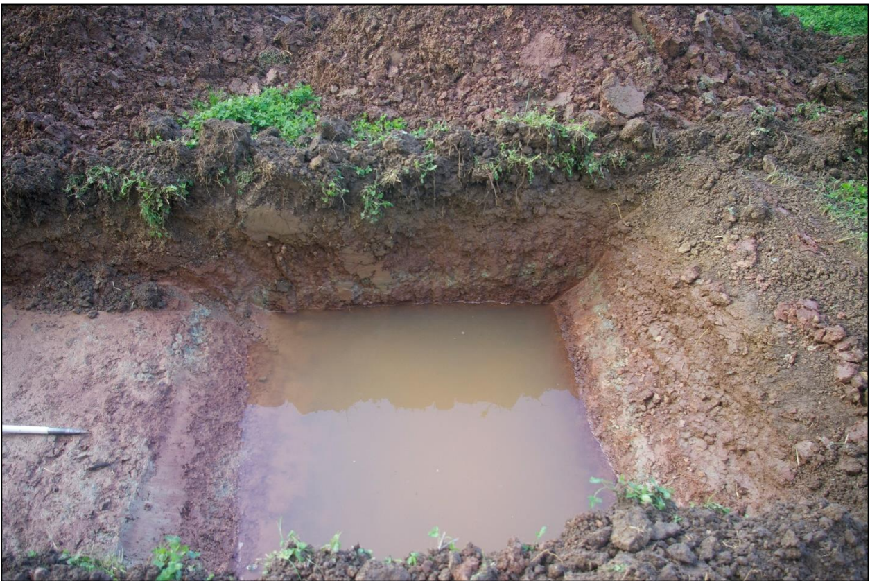
Drainage sump at northern end of trench 03; viewed from the east (no scale).
