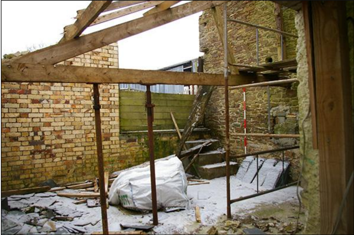
THE ROOM TO THE NORTH OF THE LEAN-TO, WITH LARGE OPENING TO THE NORTH PART OF THE YARD AND FEED ROOM/ROOT HOUSE; FROM THE WEST-SOUTH-WEST (2M SCALE).
