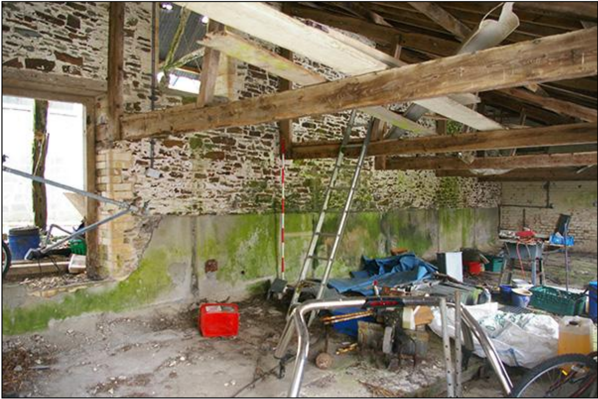
THE WEST WALL OF THE LINHAY BARN, AS SEEN WITHIN THE LEAN-TO, WITH FORCED DOORWAYS GIVING ACCESS TO THE EXTENSION, FROM THE WEST-NORTH-WEST (2M SCALE).
