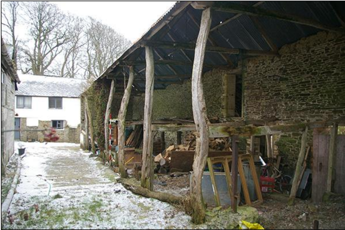
THE OPEN EAST ELEVATION, WITH STRONG TIMBER POSTS, FROM THE NORTH-EAST (2M SCALE).
