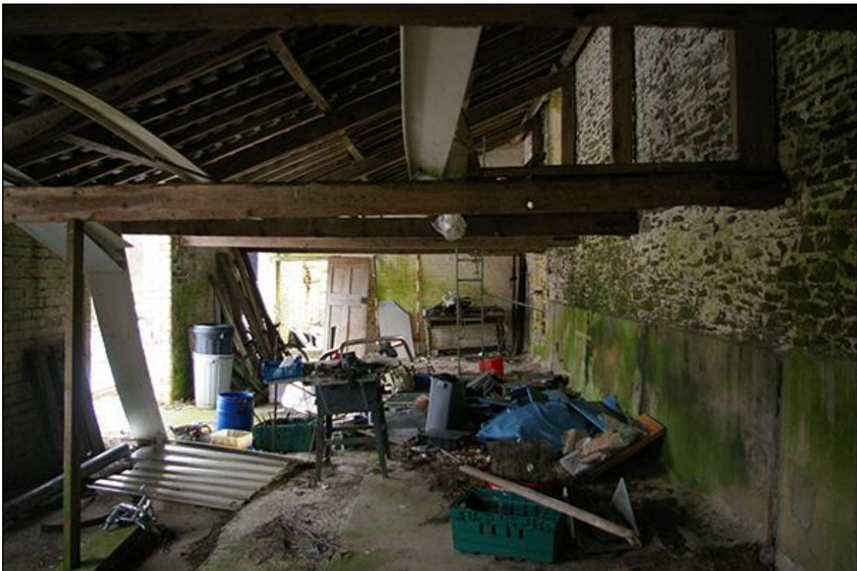
THE INTERIOR OF THE COW BYRE LEAN-TO, FROM THE SOUTH (2M SCALE).
