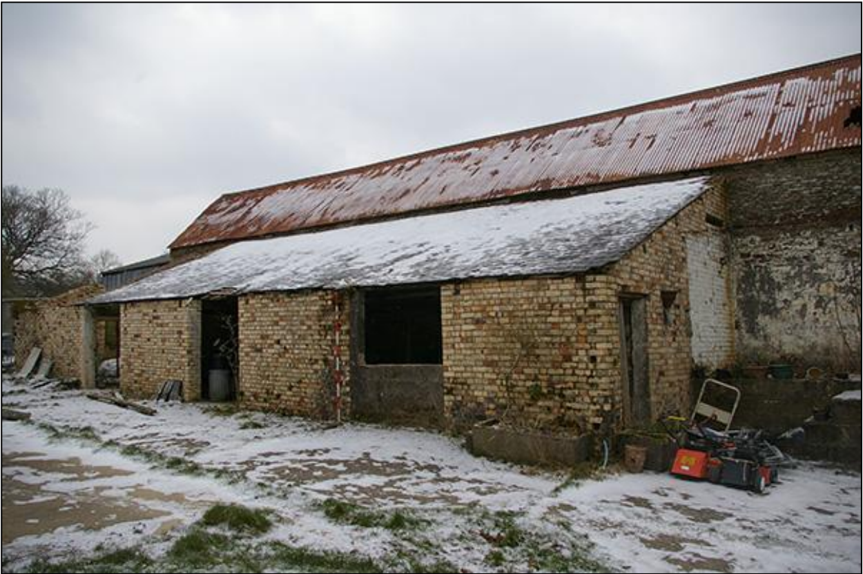
THE BRICK LEAN-TO AND WEST ELEVATION OF THE BARN, FROM THE SOUTH-WEST (2M SCALE).
