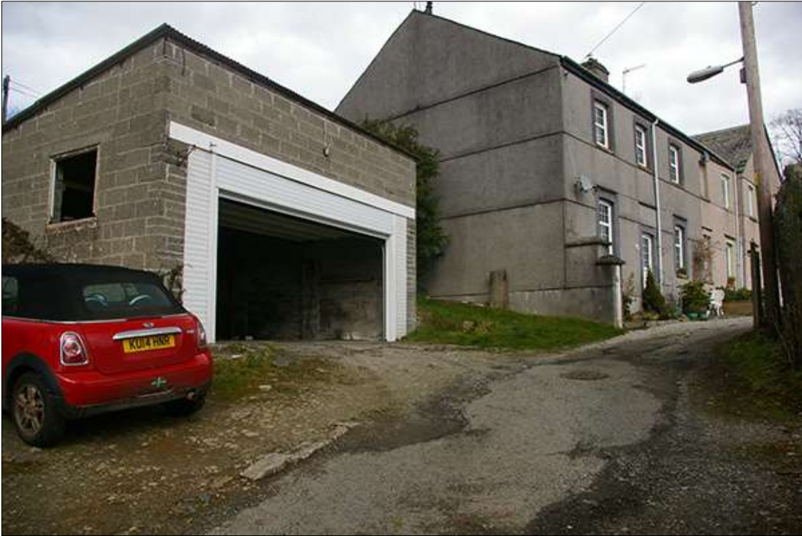
28. THE CONCRETE GARAGE BUILDING DUE TO BE DEMOLISHED ON THE SECOND PLOT; FROM SOUTH, SOUTH-WEST.
