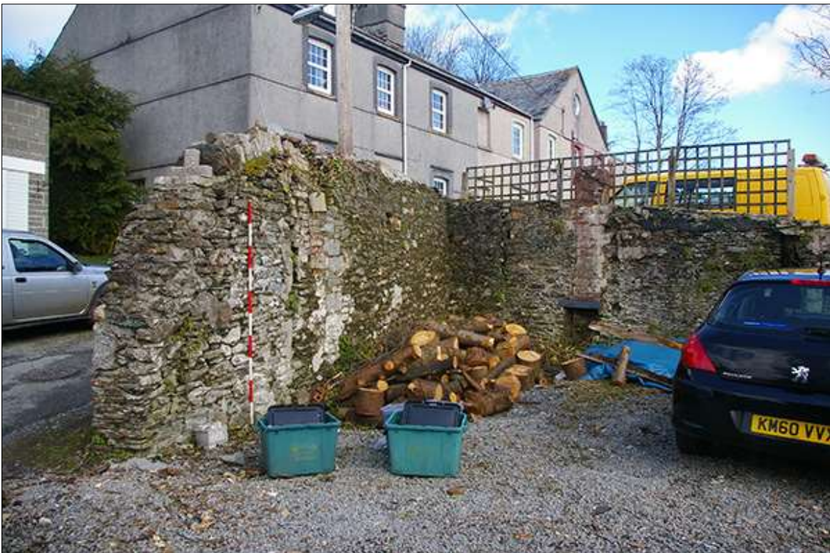
12. THE LOWER SITE; THE NORTH-WEST AND NORTH-EAST WALLS OF THE 'OLD RUINS', SHOWING A BLOCKED FLUE, WALL SCARS FROM DEMOLISHED STRUCTURES, AS WELL AS AN IN SITU FLUE AND FIREPLACE; VIEWED FROM THE SOUTH (SCALE 2M).
