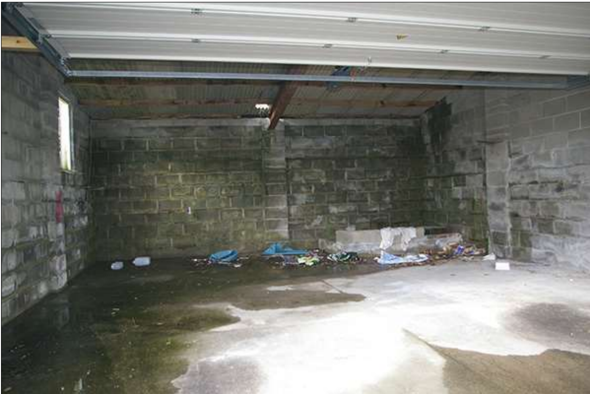
27. THE CONCRETE GARAGE BUILDING DUE TO BE DEMOLISHED ON THE SECOND PLOT; FROM THE EAST.
