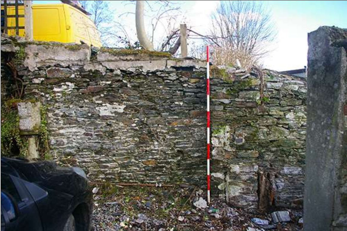
16. THE LOWER SITE; SHALLOW BUTTRESS TO THE EAST OF THE NORTH-EAST WALL, WITH 2M SCALE; FROM THE SOUTH-WEST.
